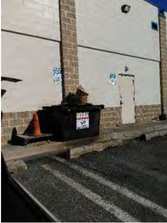
Figure 3: Grease trap with oil/grease leaks present and visible on sidewalk.
