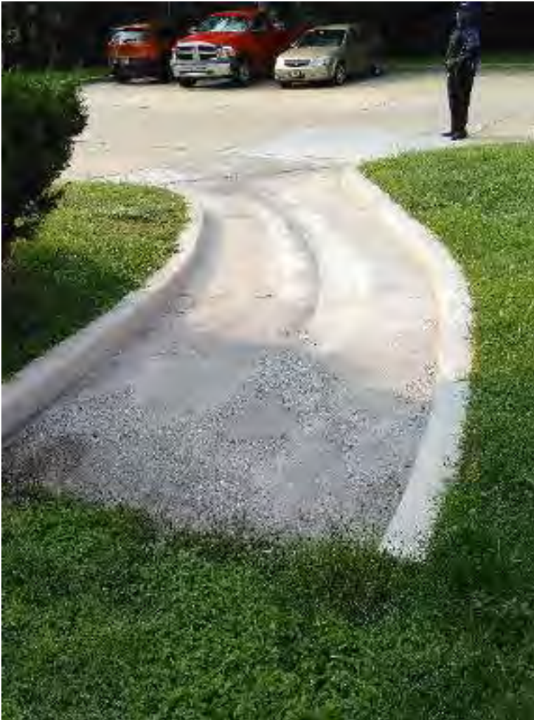
Figure 2: Washwater residue on parking lot outlet to pervious lawn.
