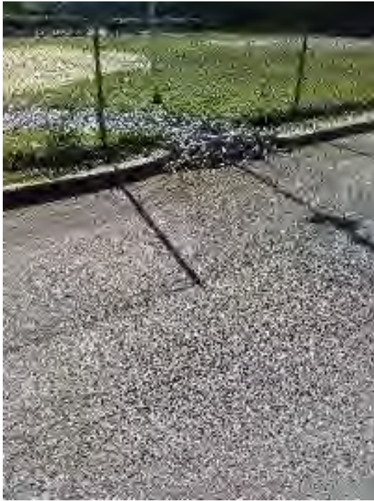
Figure 2: Curb cut to BMP1 with evidence of ponding.
