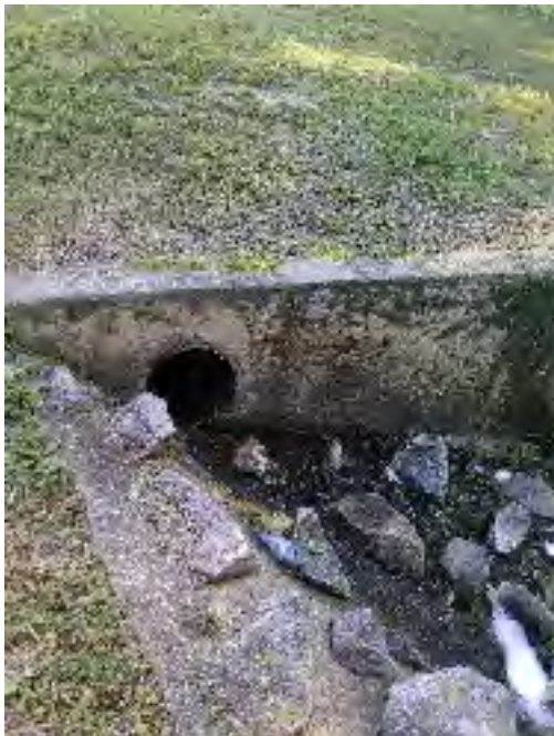
Figure 5: Outfall during first test and washing activity.
