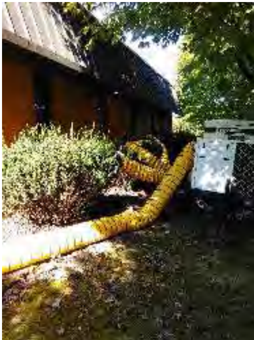
Figure 3: Potential air conditioning generator.
