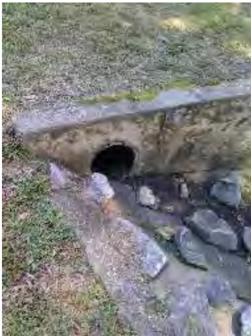
Figure 7: Outfall during second test, after washing activity and not actively flowing.
