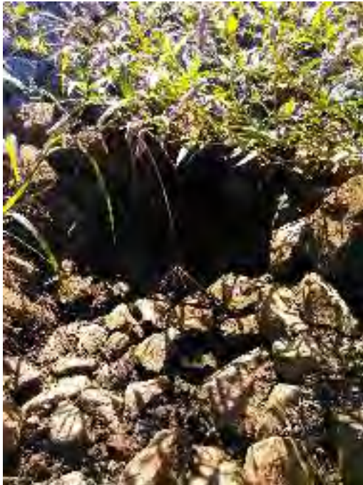
Figure 8: Outfall just upstream of clogging BMP.
