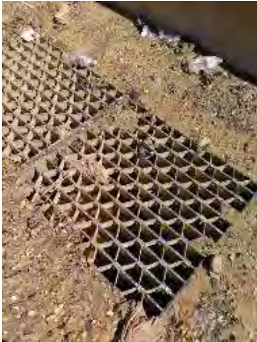
Figure 8: clogged outlet near bulk solid storage.
