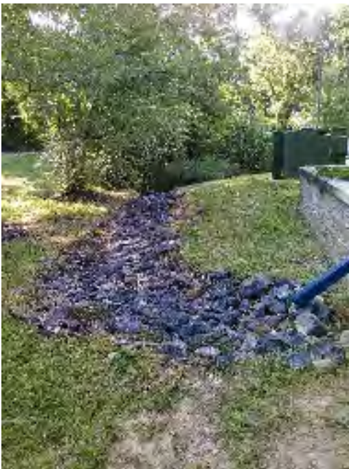
Figure 5: Downspout into stone lined conveyance channel leading to rain garden
