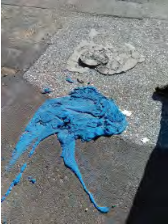
Figure 4: Notable patches of hardened Dryvit product on pavement in rear of vacant retail space. Blue and gray patches of spilled product are approximately 2 ft in diameter.
