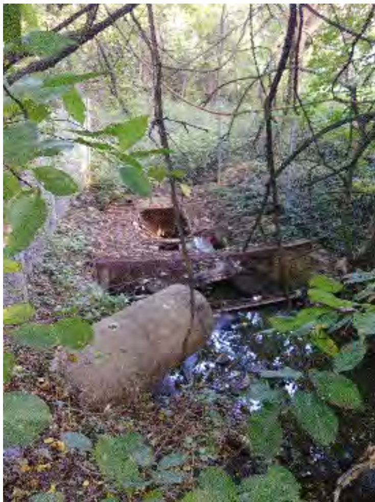
Figure 2: Outfall L10O007 pictured in poor condition behind damaged stabilizing structure/trash trap. Outfall L10O010 pictured in foreground.
