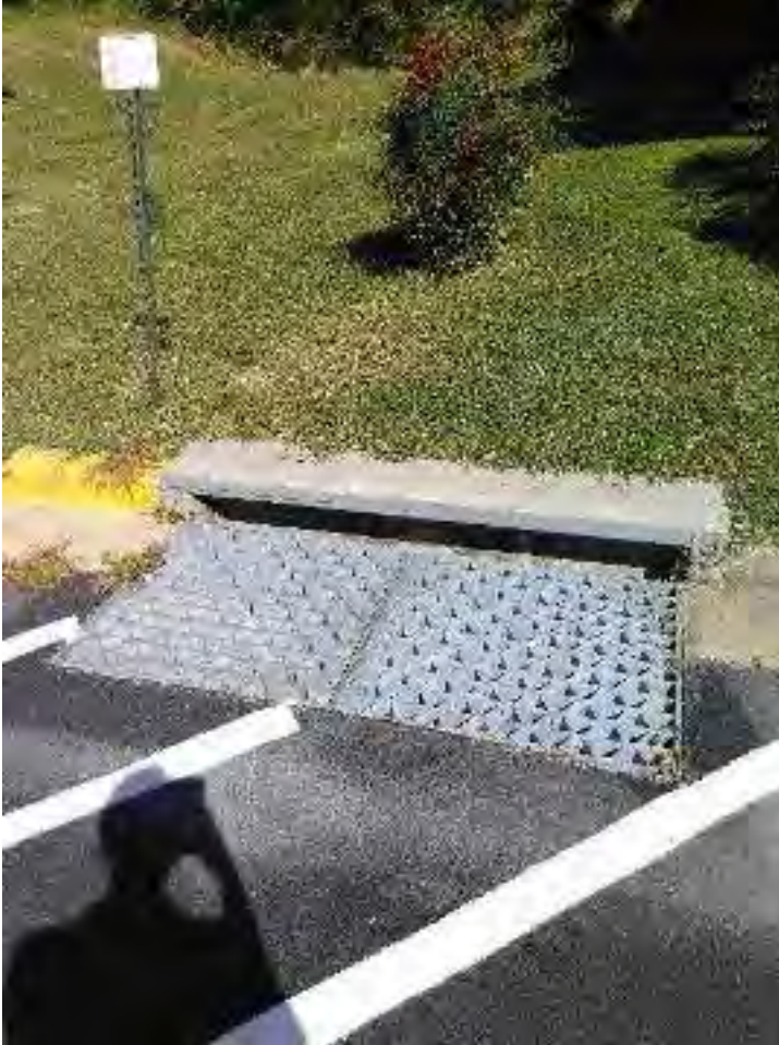
Figure 3: Typical Police Headquarters inlet.
