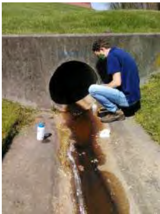
Figure 1: Outfall Ko2O016 flowing on 4/20/21
