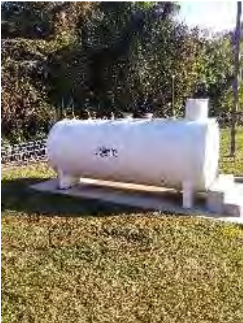
Figure 3: large liquid storage tank assumed to be filled with fuel.
