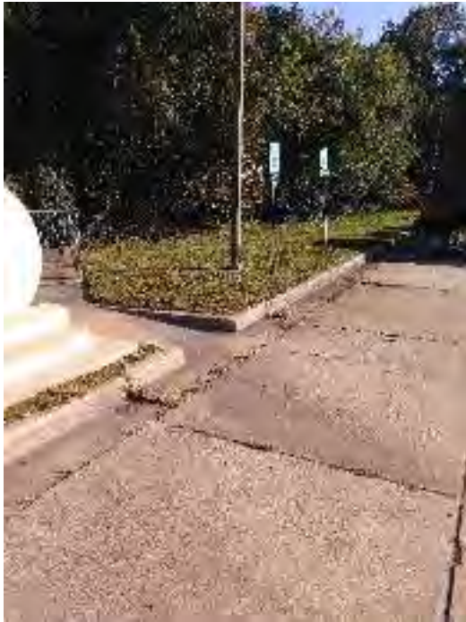
Figure 6: pavement staining of potential washing activity.
