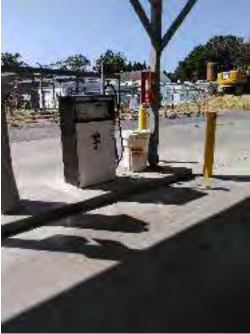
Figure 2: Fueling station with emergency spill kit
