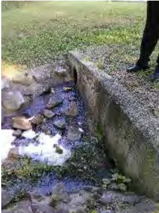
Figure 4: Outfall during first test and washing activity.
