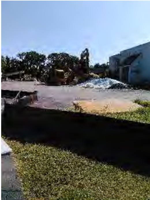
Figure 4: Uncovered soil behind silt fence.
