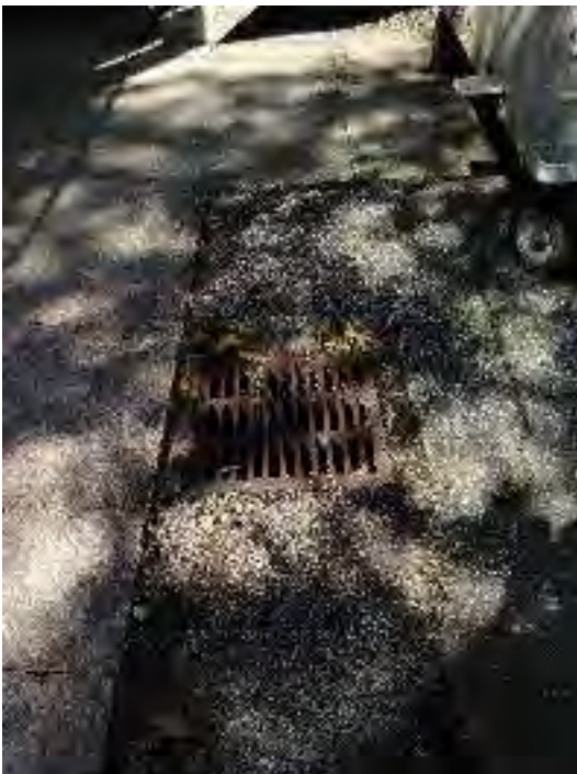
Figure 5: High water elevation in catch basin at east end of property
