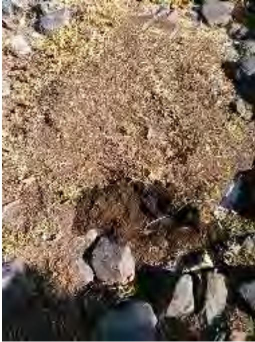
Figure 2: Blocked inlet which is mulched over.
