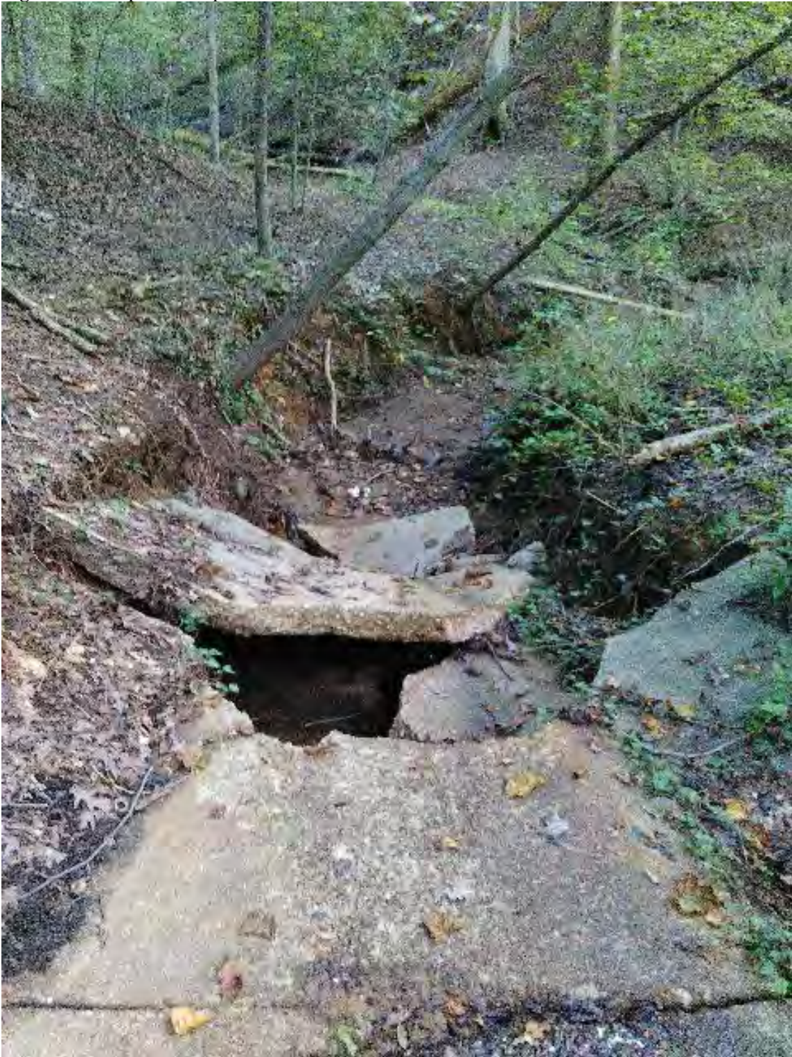
Figure 4: Collapsed flow path from Outfall T150059 and downstream erosion
