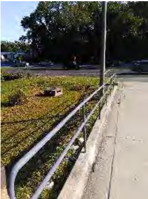
Figure 4: Dry pond riser structure and curb flow path to dry pond
