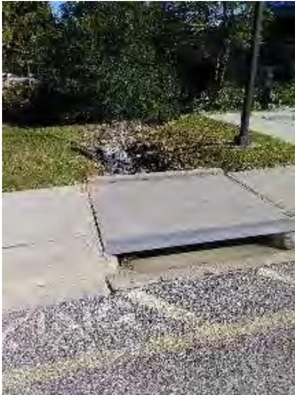
Figure 6: Parking lot inlet routing flow to micro bioretention.
