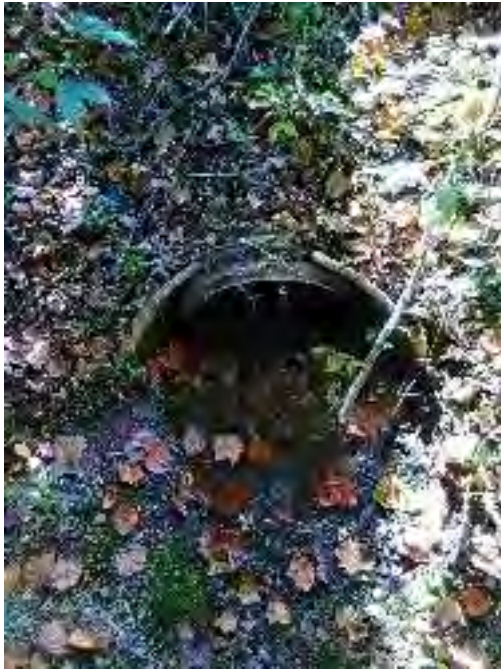
Figure 2: Large outfall directing flow offsite.
