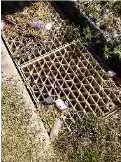
Figure 10: Trash present in outfall on west edge of detention facility.
