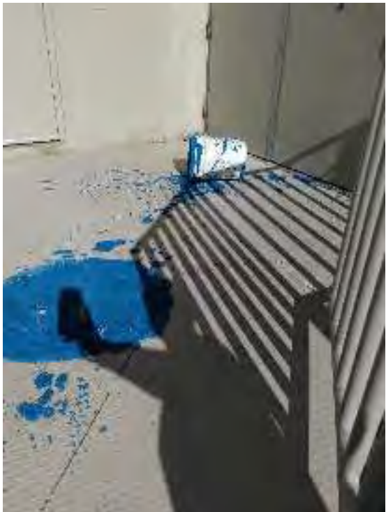
Figure 3: Bucket of unknown Dryvit product spilled and hardened on the back stoop of vacant retail space.
