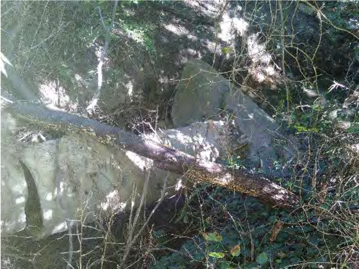
Figure 3: Broken and collapsed end section of Outfall L090021.
