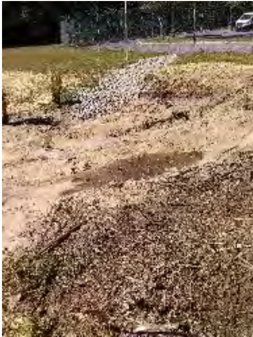
Figure 4: erosion and lack of vegetation in BMP1.
