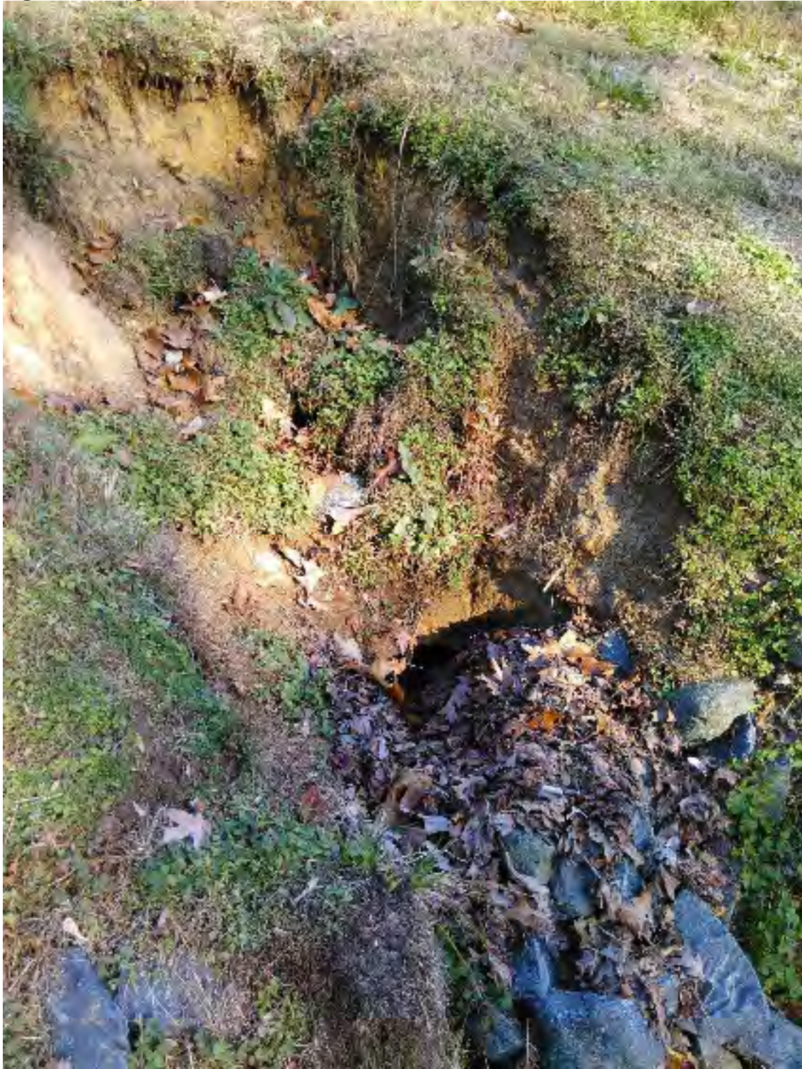
Figure 2: Collapsed Outfall (T150001)
