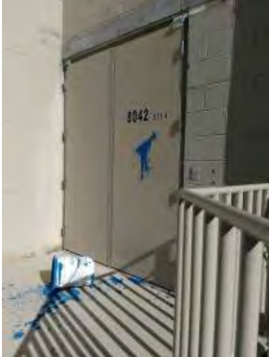
Figure 2: Bucket of unknown Dryvit product spilled on the back stoop of vacant retail space.
