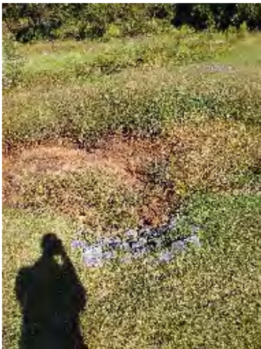
Figure 7: BMP clogging just downstream of outlet.
