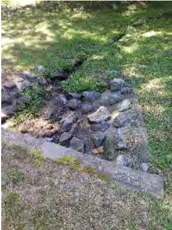
Figure 8: Outfall discharge area during second test, after washing activity and not actively flowing.
