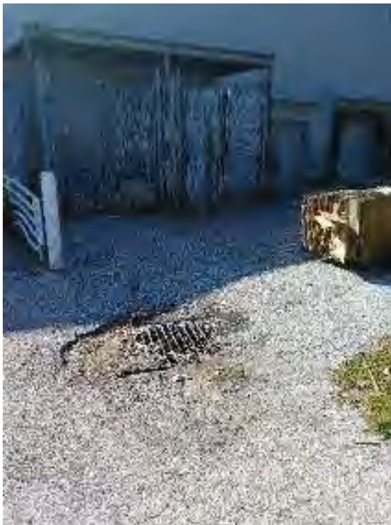
Figure 4: Bulk cardboard storage, scattered trash originating from enclosed dumpster, and potential receiving catch basin.
