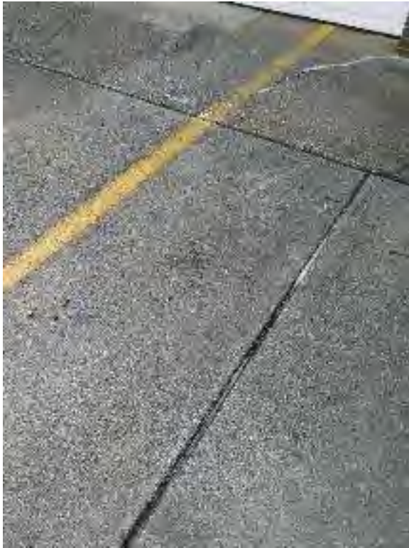
Figure 4: Residual suds in front of the site, likely washing location.
