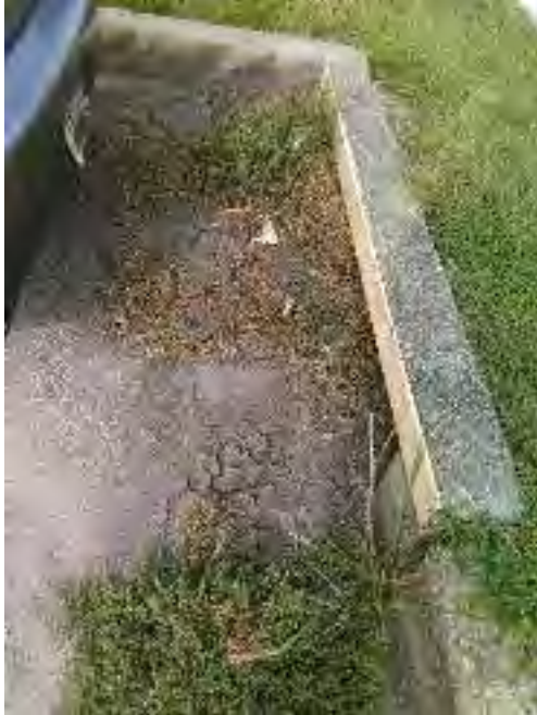
Figure 2: Partially blocked inlet at the Northern District Police Station
