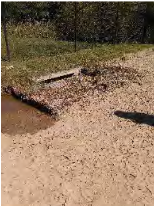
Figure 9: clogged outlet near bulk solid storage.
