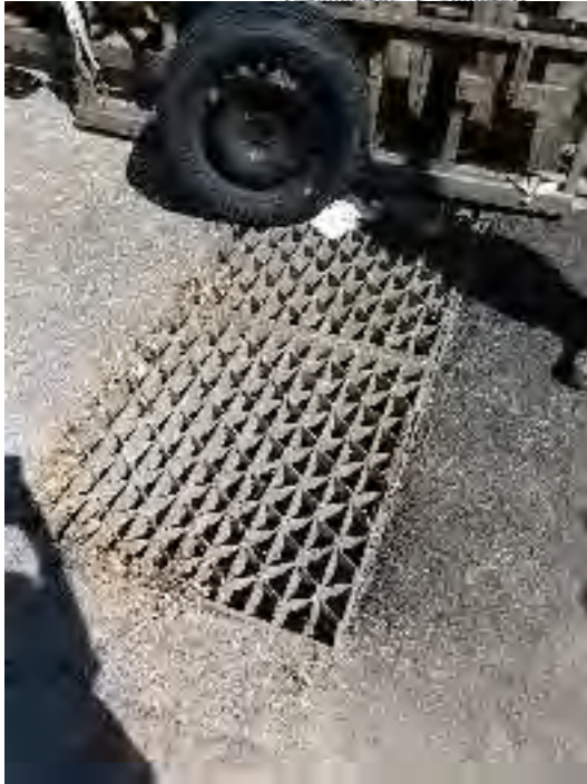
Figure 4: High water elevation in catch basin at SW end of property
