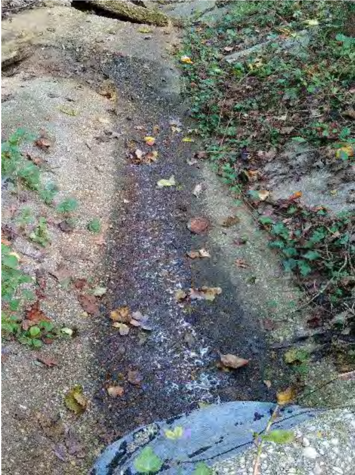
Figure 3: Collapsed flow path from Outfall T150059
