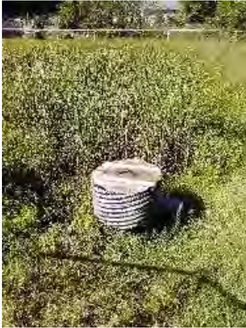
Figure 4: Wet pond riser structure.
