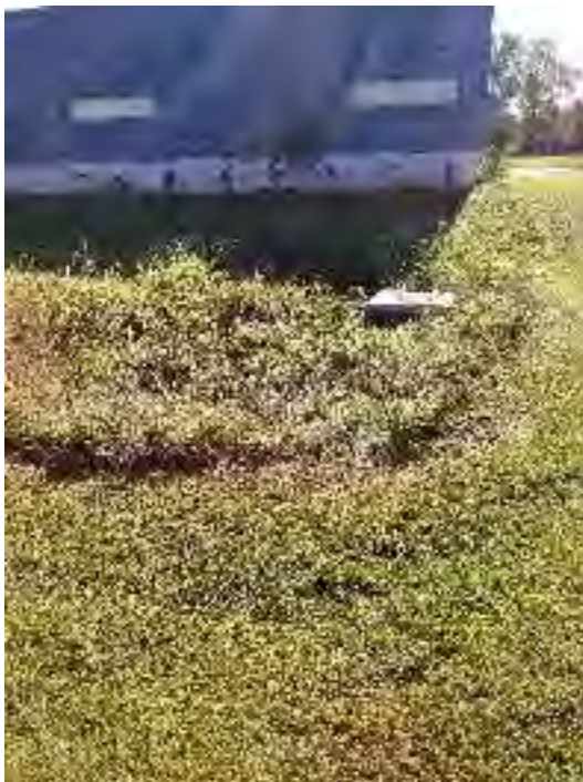
Figure 13: Newly installed BMP near administrative building.
