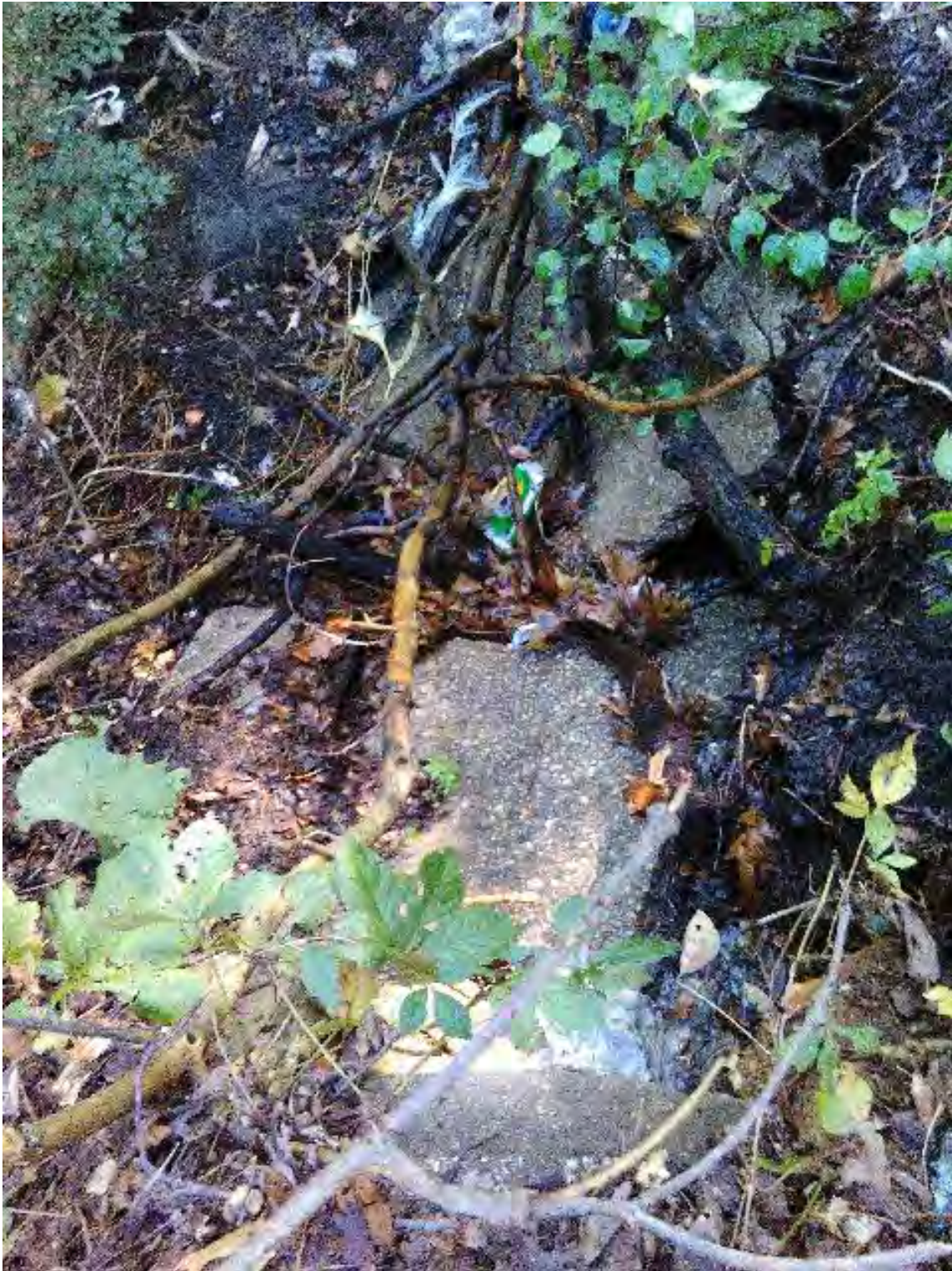
Figure 3: Debris downstream of Outfall M09O060
