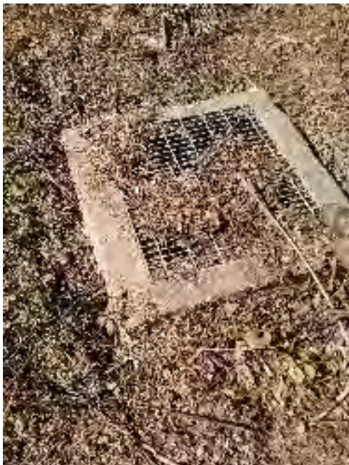
Figure 5: overflow structure for BMP1 is somewhat clogged and should be cleaned.
