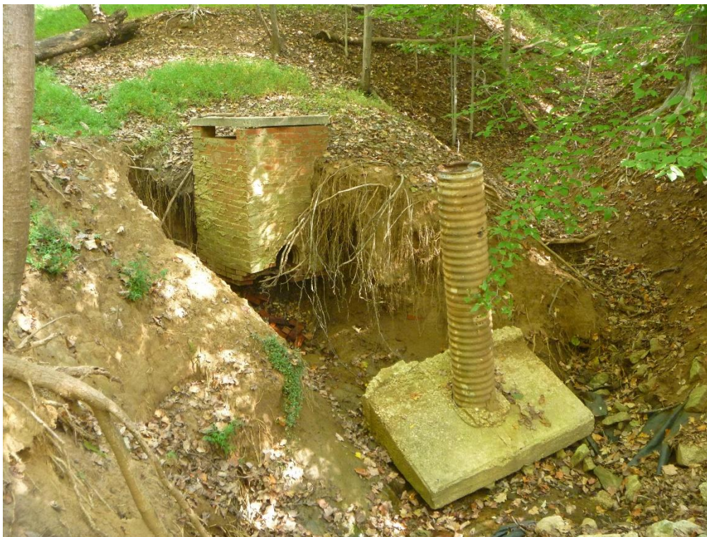
Figure 1. A view of a completely detached pipe and headwall at outfall N20O020; the adjacent inlet (left) is N20O004
