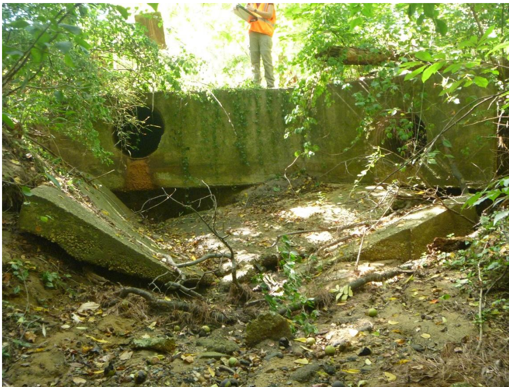
Figure 1. A view of collapsed decking below outfalls Q21O003 (right) and Q21O003a (left)
