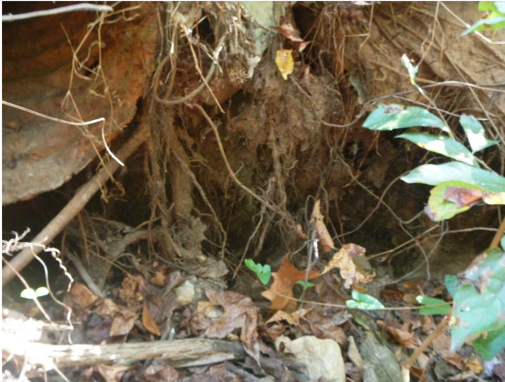
Figure 2. A view of one end of the driveway culvert showing exposed roots and undermined pipe
