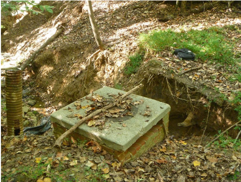
Figure 2. A view from the side of inlet N20I004, adjacent to displaced outfall N20O020, showing extensive undercutting of the sediment
