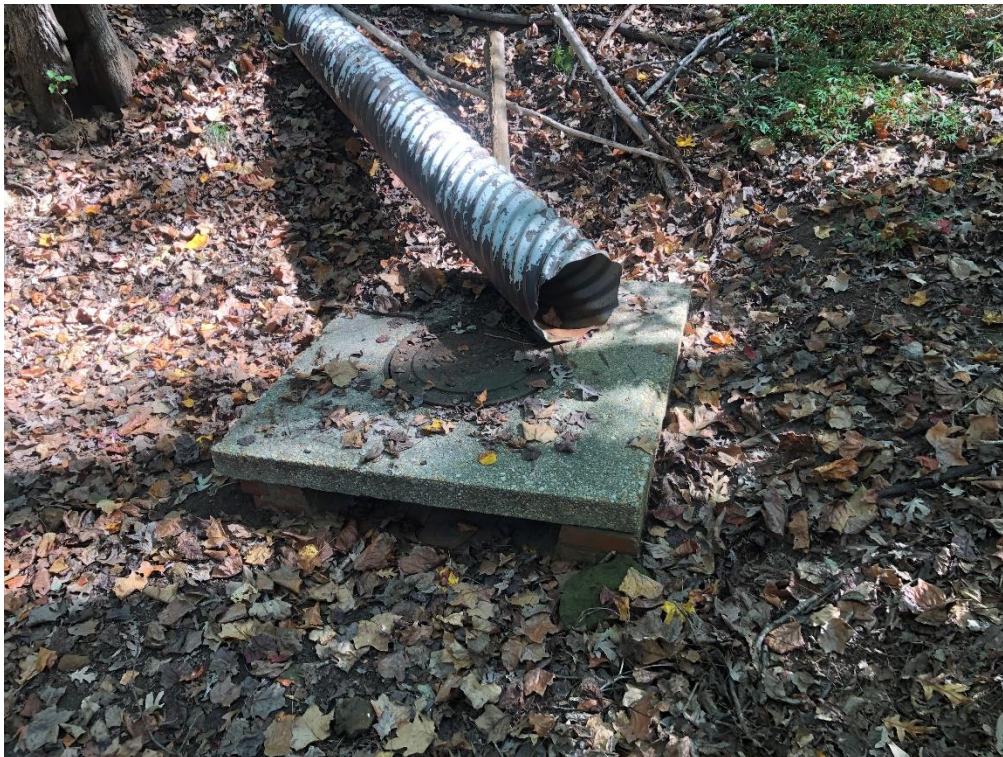
Figure 3. A view of the outfall N20O009, up-network of outfall N20O020, which discharges directly onto a concrete cap for an inlet
