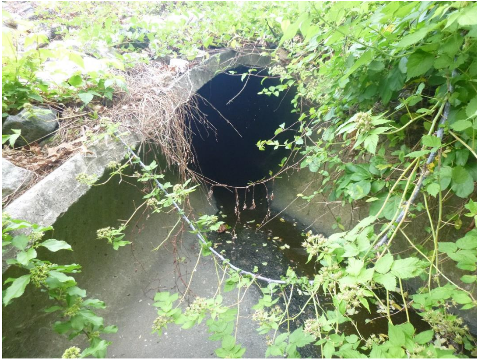
Figure 1. Flowing effluent from outfall F09FO005, as observed on May 27, 2020
