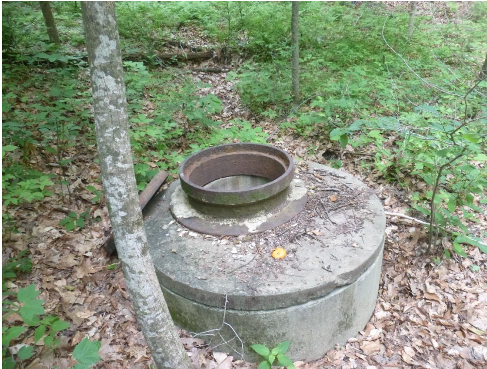
Figure 2. A view of a manhole with a dislodged cover along the pipe network for outfall M23O004
