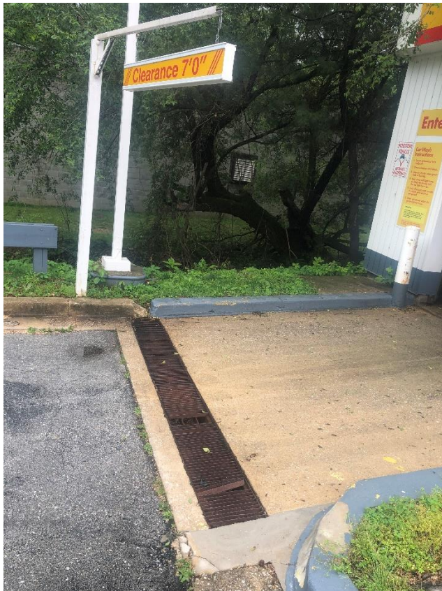
Figure 2. A trench drain at the entrance to the car wash associated with the Shell gas station
