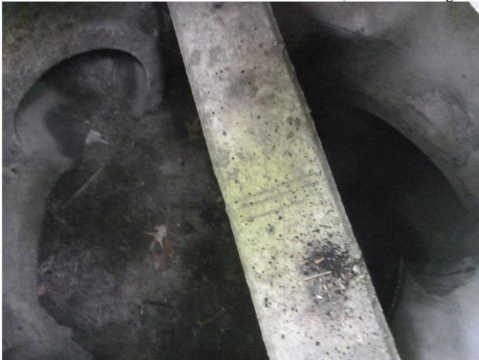
Figure 3. A view of stagnant water in manhole O22M102 on June 2, 2020
