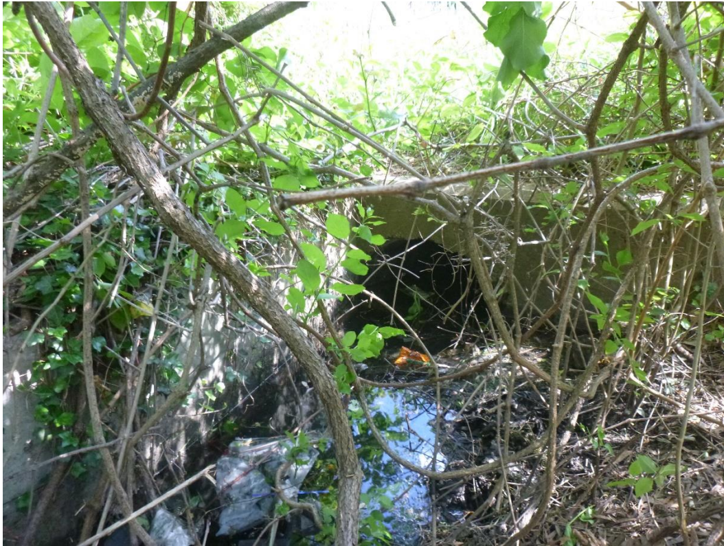
Figure 1. Conditions at outfall T16O006 on May 12
