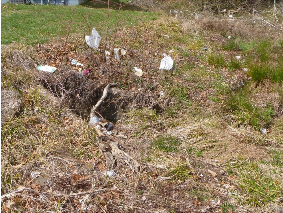
Figure 3. A view of the entrance to the culvert partially blocked by excessive vegetation; note the accumulated debris near the entrance
