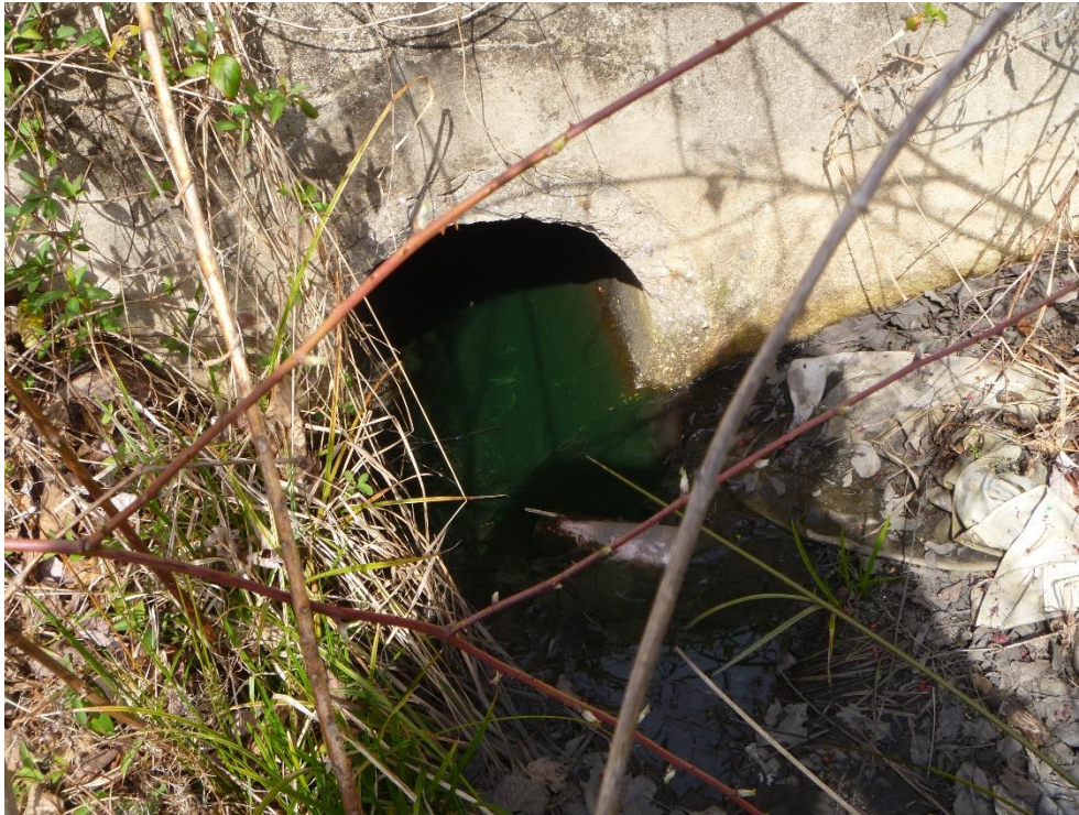
Figure 1. Green stagnant water evident in the outfall F09O003, which is immediately adjacent to the car wash of the Shell gas station
