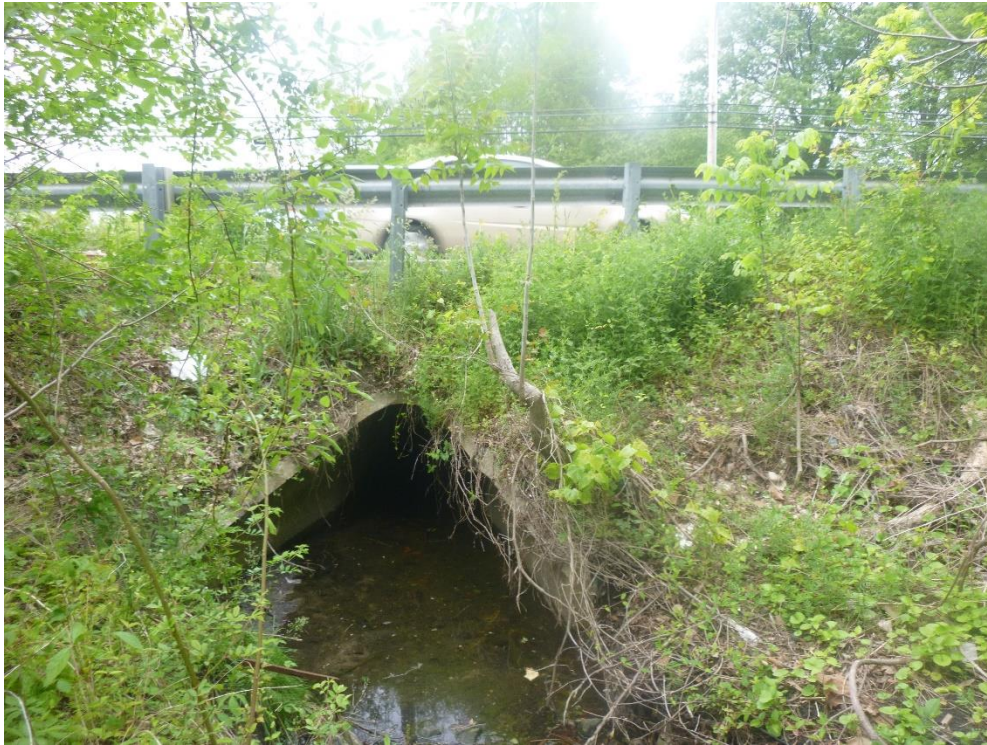
Figure 1. Conditions at outfall P200003 on May 14
