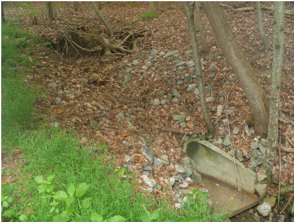
Figure 1. A view of ground subsidence (upper left) approximately 12 feet up-network of outfall O200010 (lower right)
