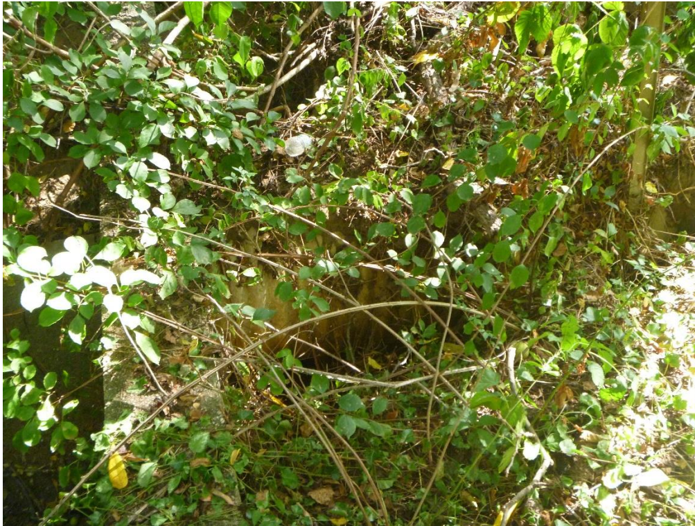
Figure 2. Evidence of erosion undermining the pipe leading to outfall Q21O003 behind the headwall
