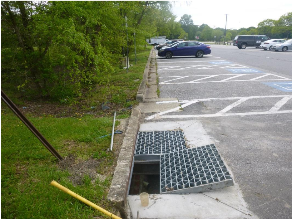
Figure 3. Inlet at edge of parking lot in front of Annapolis High School
