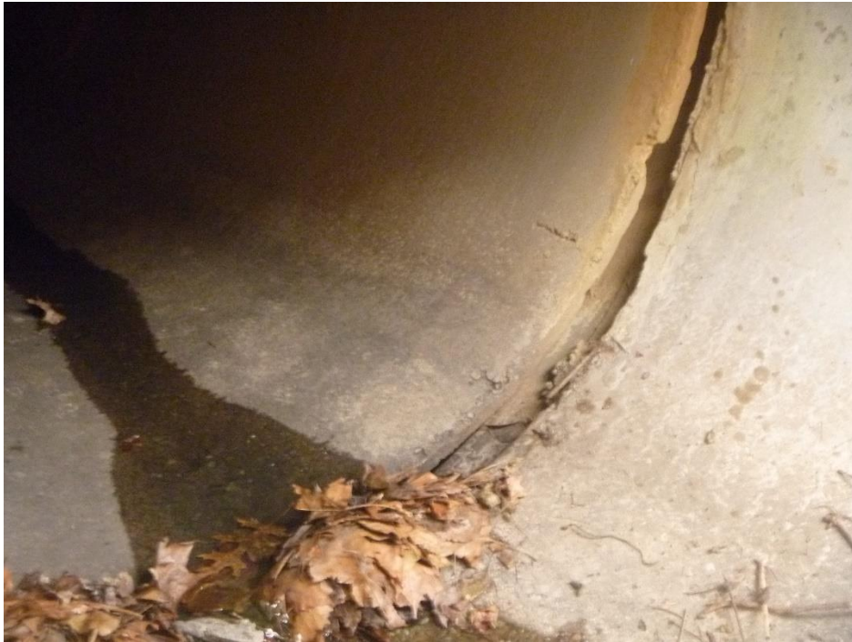
Figure 1. Conditions at outfall J04O004 on January 23
