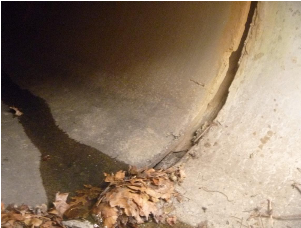
Figure 1. A view of the partially detached end pipe (lower right) at outfall J04O004, which allows water to flow under the structure and further erode the supporting soil
