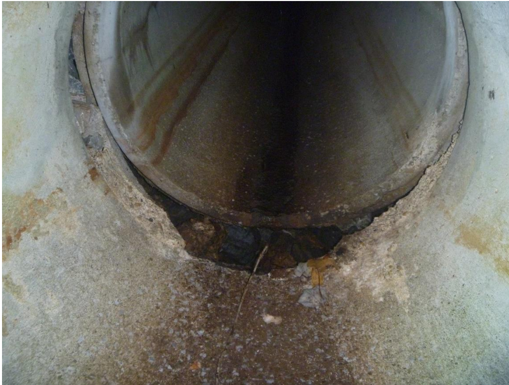
Figure 2. A view of the disconnected flared end section of outfall O200010
