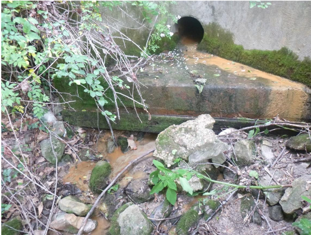
Figure 2. A view of the water flowing under the apron of the endwall of outfall L23O001 (left foreground)
