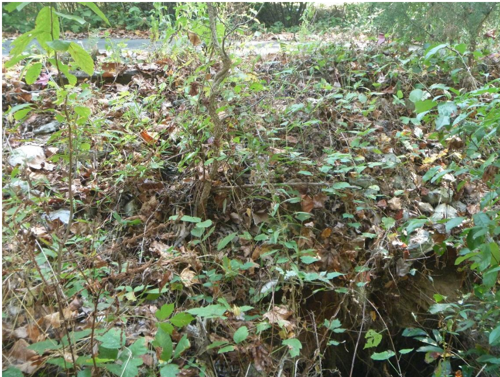
Figure 1. A view of the pipe (center-right foreground) forming a culvert under the driveway (background) at 6664 Old Solomons Island Road; note the eroded bank (lower right)
