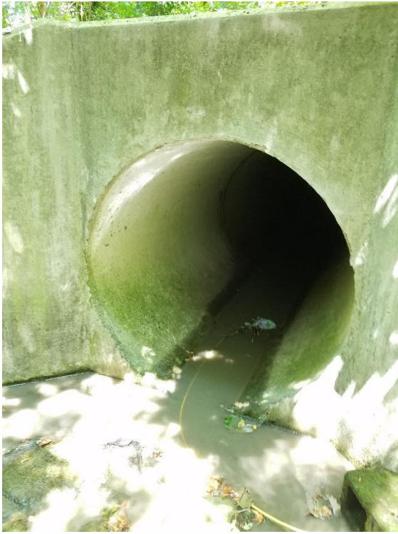
Figure 1. A view of grey, cloudy discharge in the outfall R200017 on June 26
