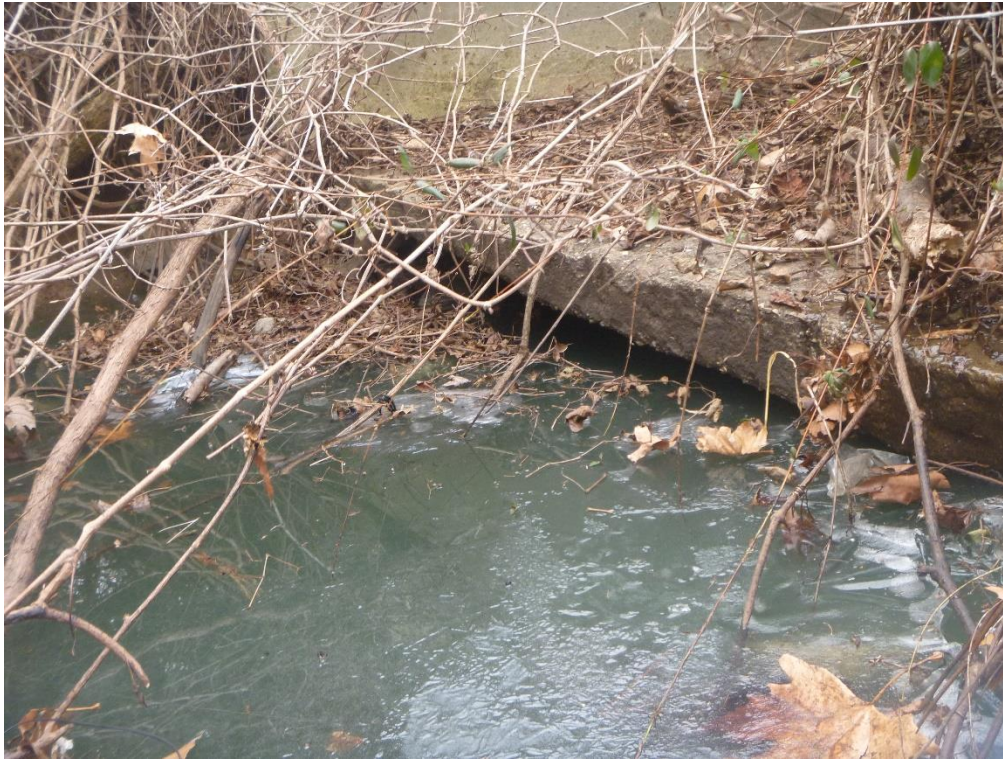
Figure 2. A view of the base of the flared end of the outfall J04O004, showing evidence of the tilted end section which facilitates erosion under the structure
