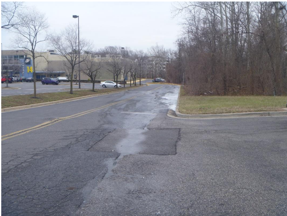
Figure 3. View of the path (foreground to background) of the discharge from the car wash toward the inlet near Hoyt's West Nursery Cinema 14; the photograph was taken on January 23
