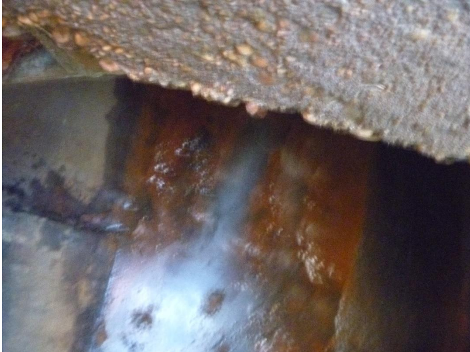
Figure 2. A view inside the inlet immediately up-network from the outfall; note evidence of bacterial colonies similar to those seen at the outfall, as shown in Figure 1
