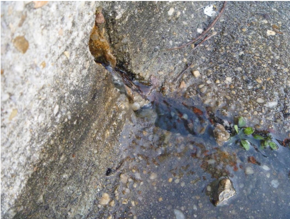
Figure 5. A view of discharge leaking through a seam in the curb along the north side of the car wash; the photograph was taken on January 24
