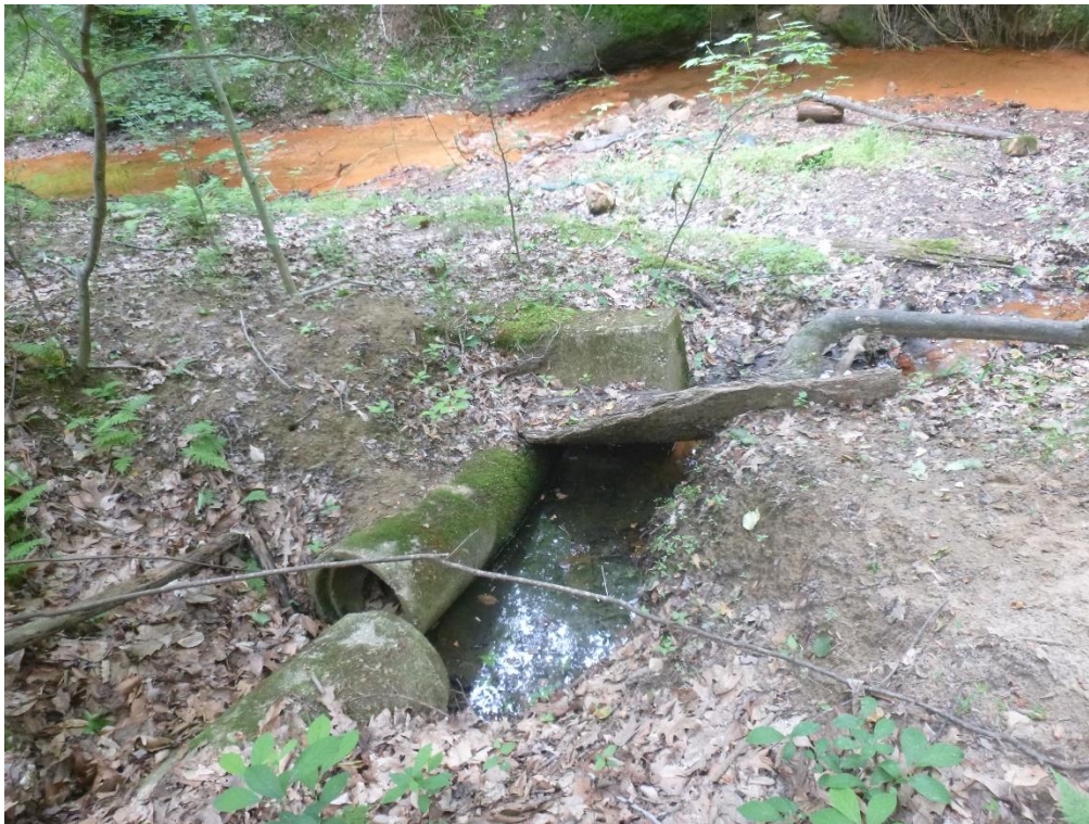
Figure 1. A view of the disconnected pipe system at outfall M23O004; note the severed pipe and endwall (left center) partially covered in sediment and the impromptu channel from the acting receiving pool to the stream (center right)
