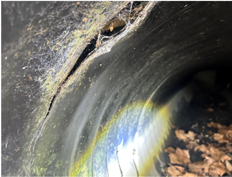
3/15/2023 Inspection – Outfall R200005 damage.
