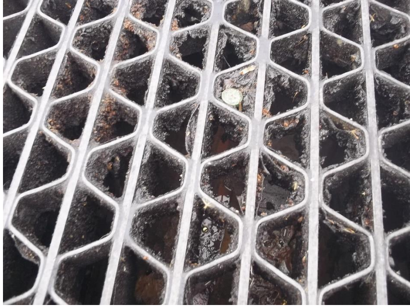
2/22/2023 Inspection – Kitchen grease on catch basin grate
