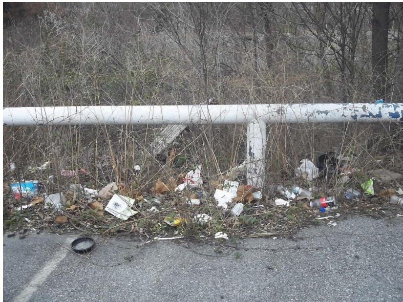
2/22/2023 Inspection – Trash in brush along parking lot
