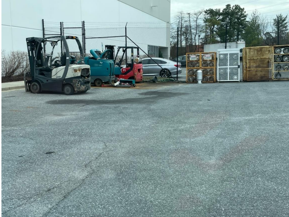
2/24/2023 Inspection – Dark stain on pavement in storage area. Slight red stains indicate a potential transmission leak.
