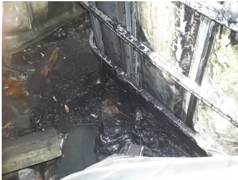
3/9/2023 Inspection – Leaking tote when it rains.
