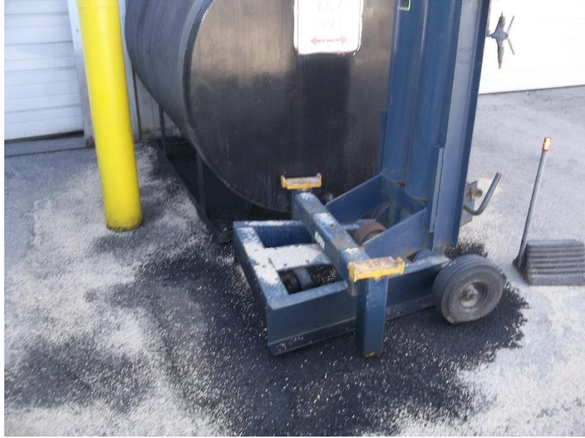
3/7/2023 Inspection – Oil on pavement around 500-gallon used oil tank
