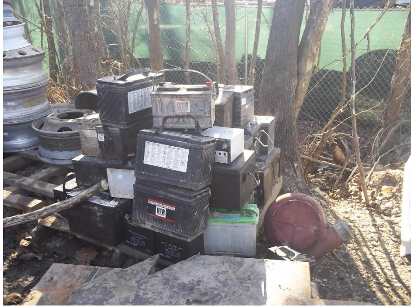
2/23/2023 Inspection – Batteries not under cover
