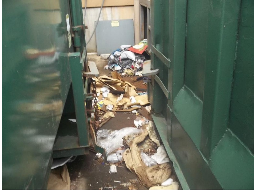
2/22/2023 Inspection – Trash around dumpsters
