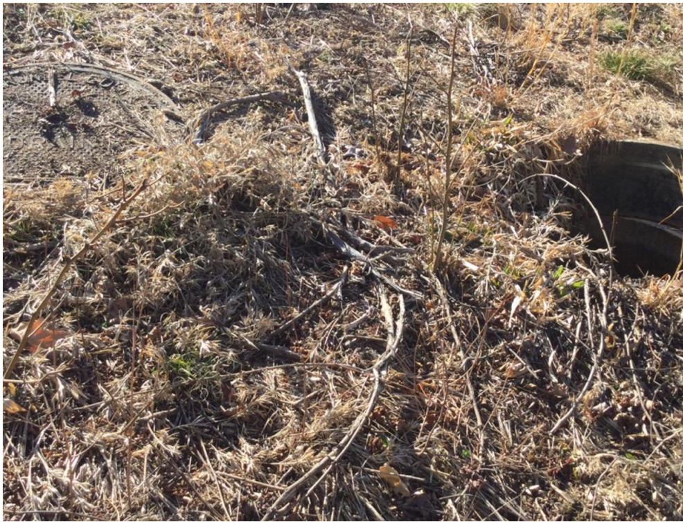
3/21/2023 Inspection – Manhole cover off.
