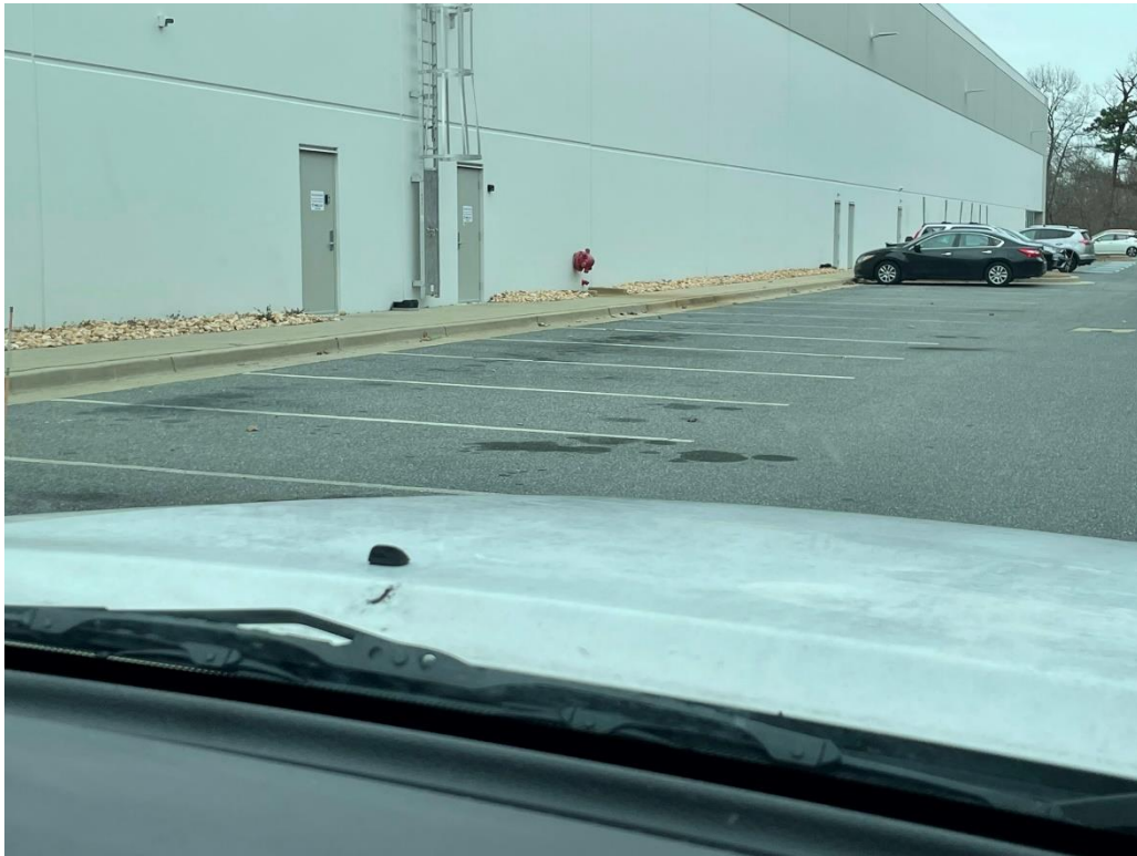
2/24/2023 Inspection – Numerous stains on parking spaces.
