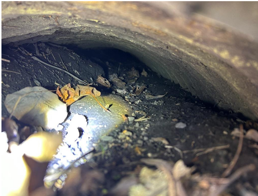
3/15/2023 Inspection – Sedimentation in the barrel.
