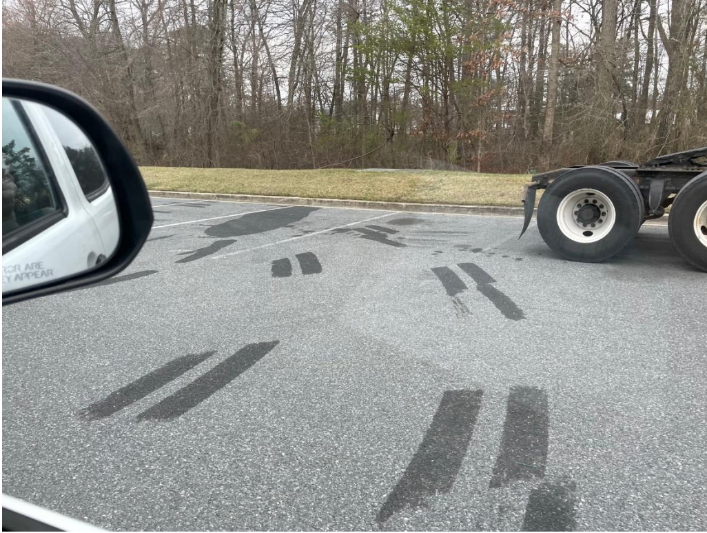
2/24/2023 Inspection – Dark staining with tire tracks.
