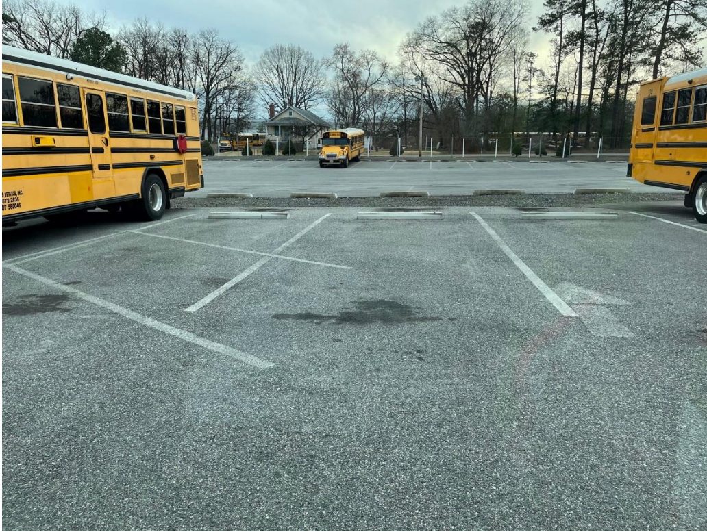
2/24/2023 Inspection – Staining on bus parking spots.
