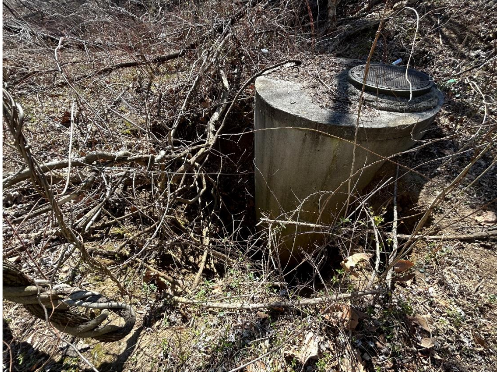
3/15/2023 Inspection – Outfall R200005 manhole erosion.
