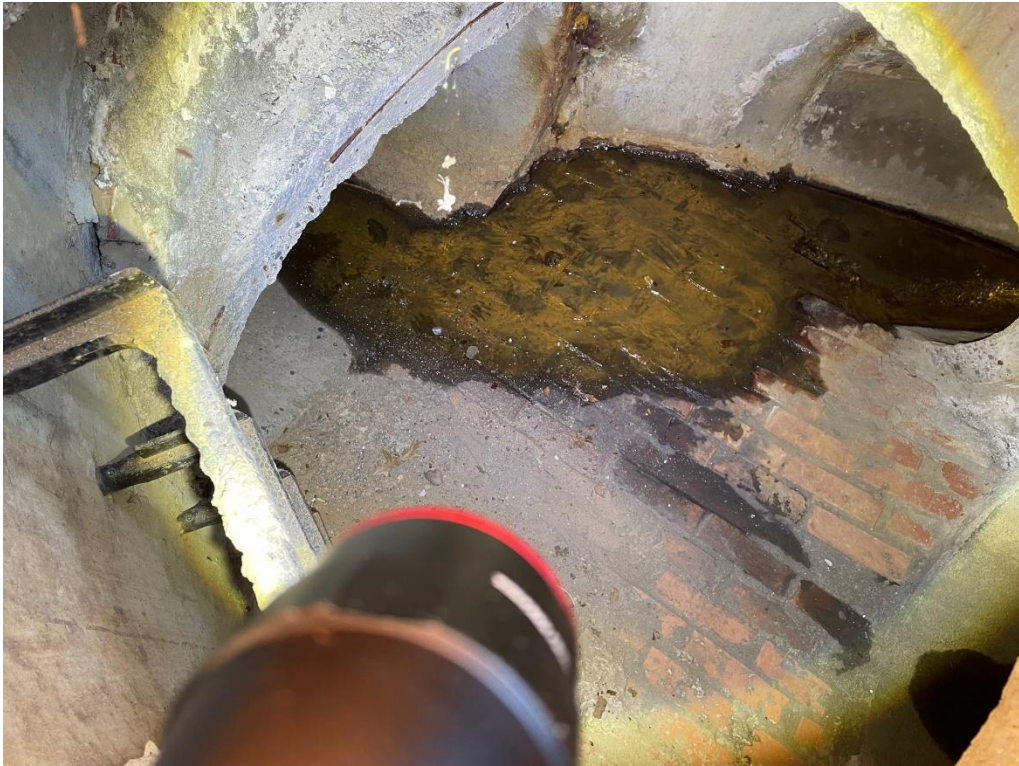
P5 3/30/2023 Inspection – Flow convergence upstream. Clear source in top pipe.
