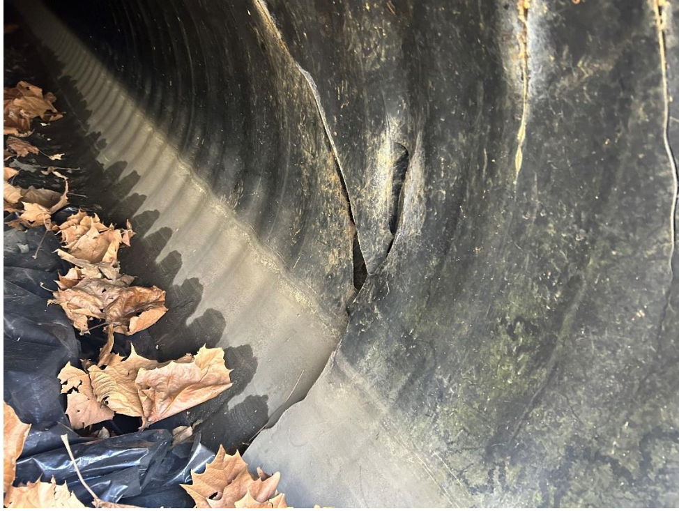
3/15/2023 Inspection – Outfall R200005 damage.
