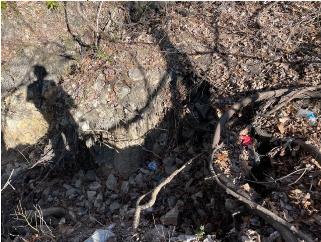
3/16/23 Inspection – Downstream erosion and headcut.
