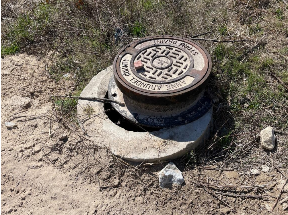
3/30/2023 Inspection – Loose manhole cover.
