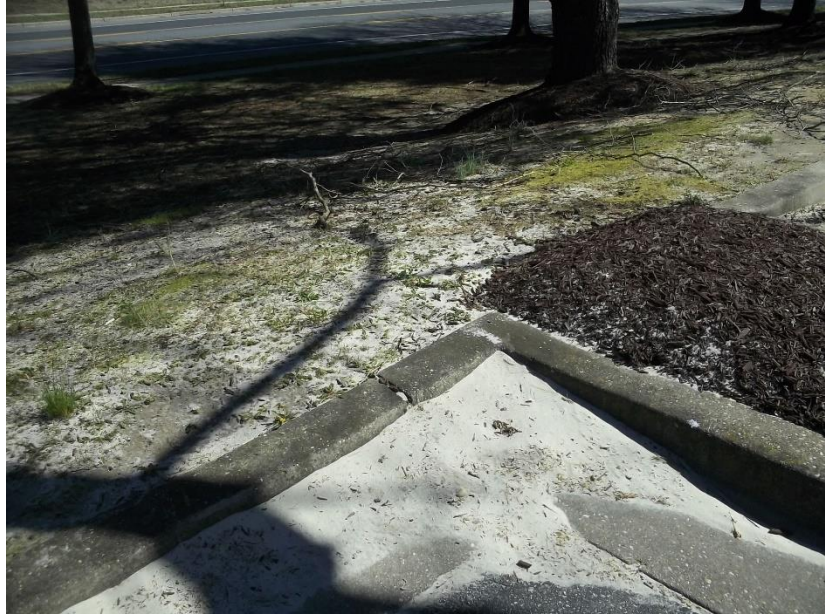
3/20/2023 Inspection – Sand migrating throughout parking lot
