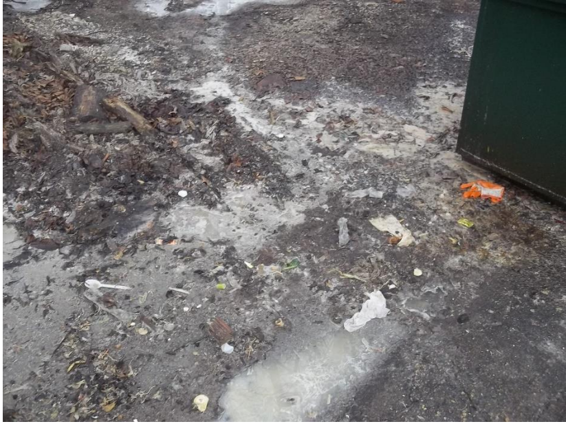
2/23/2023 Inspection – Grease on pavement
