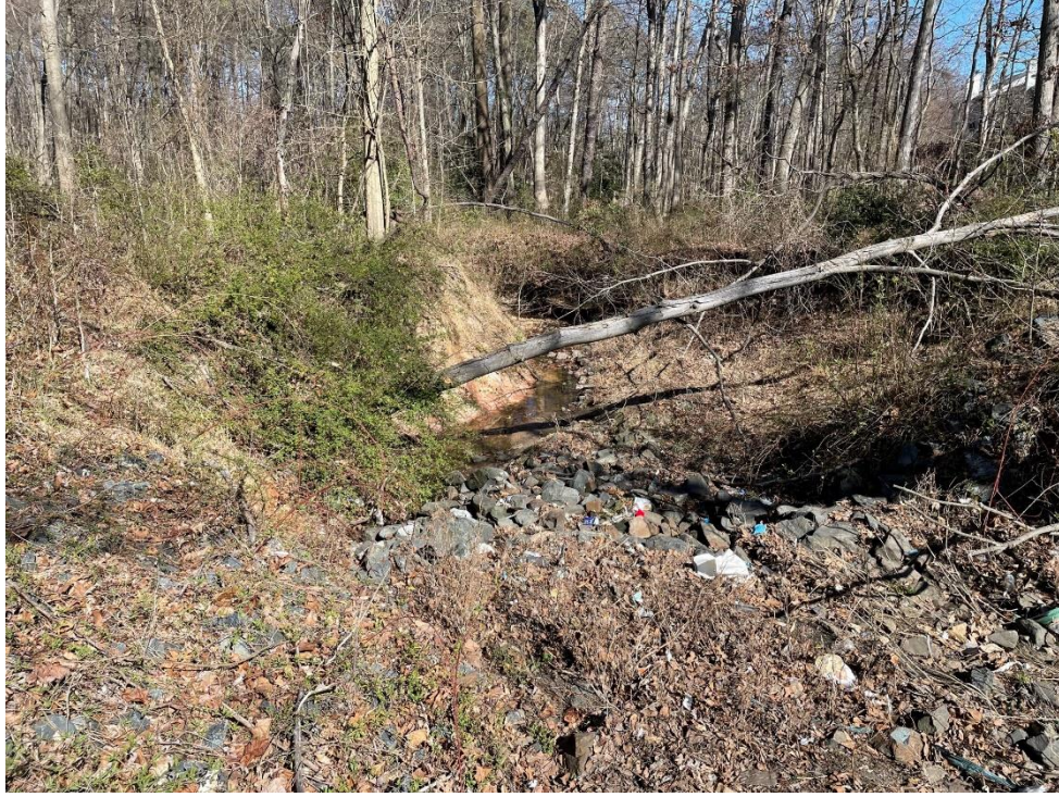
3/15/2023 Inspection – Outfall B110011 downstream erosion.
