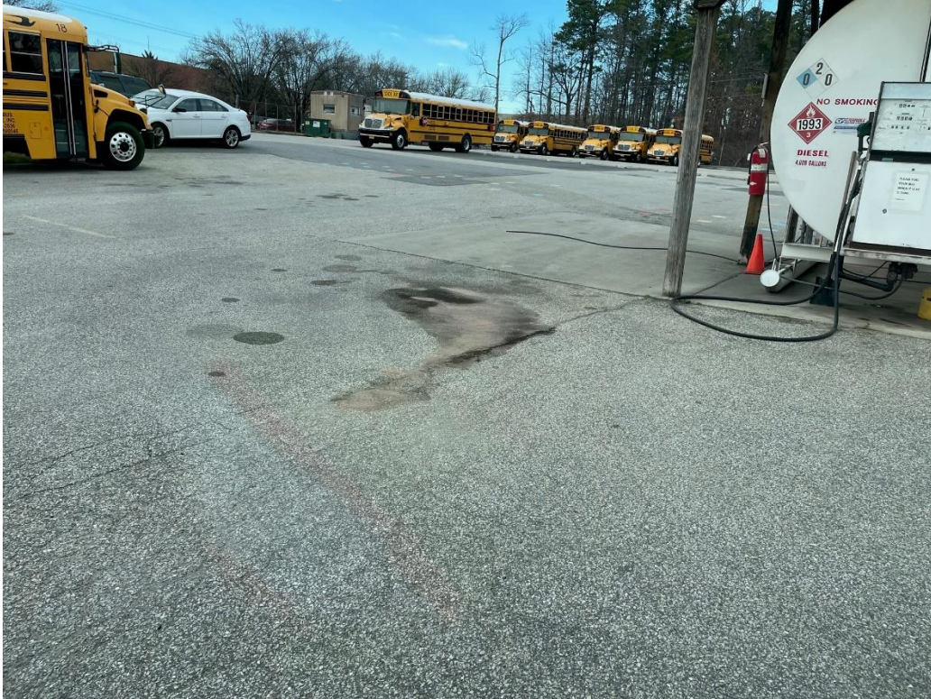
2/24/2023 Inspection – Spill with absorbent that has not been cleaned up.
