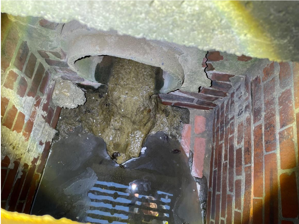
P3 3/30/2023 Inspection – Infall to above inlet, odd deposit.
