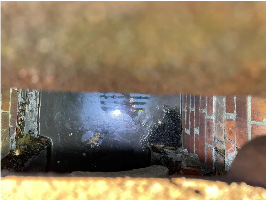
P2 3/30/2023 Inspection – Inlet upstream in the system with heavy sheen.
