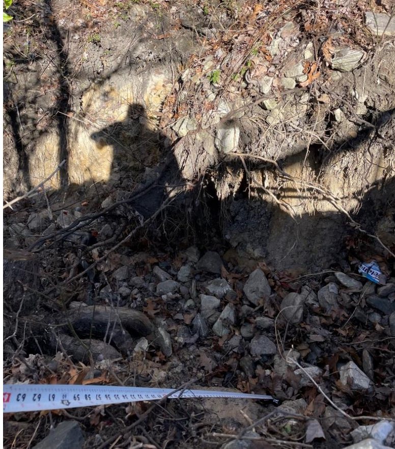
3/16/23 Inspection – Downstream erosion, 5ft deep.
