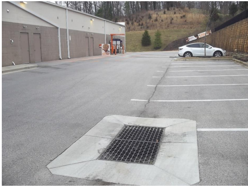
2/22/2023 Inspection – Catch basin containing kitchen grease
