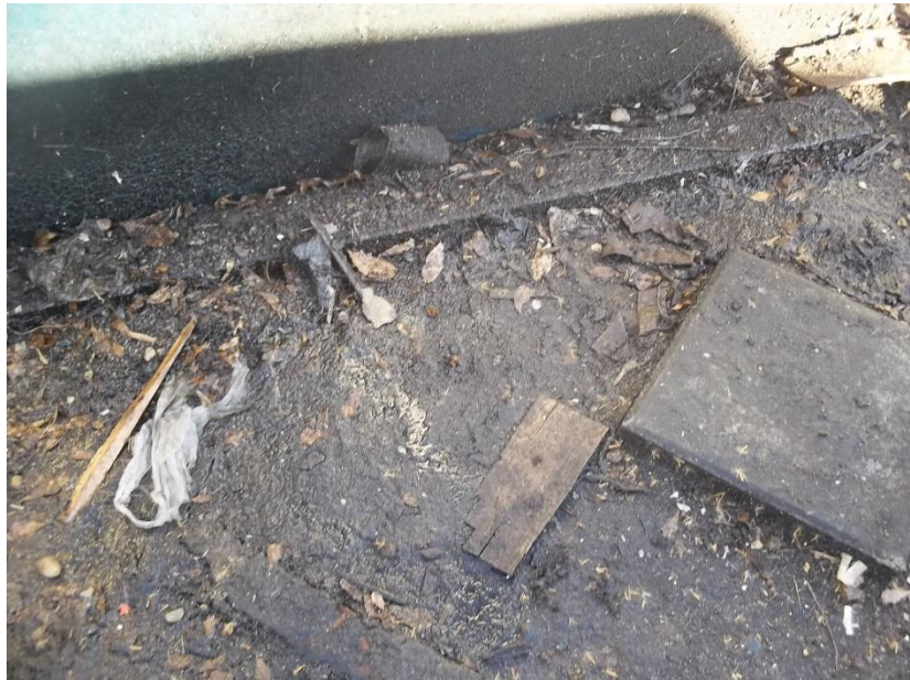
3/20/2023 Inspection – Grease on pavement
