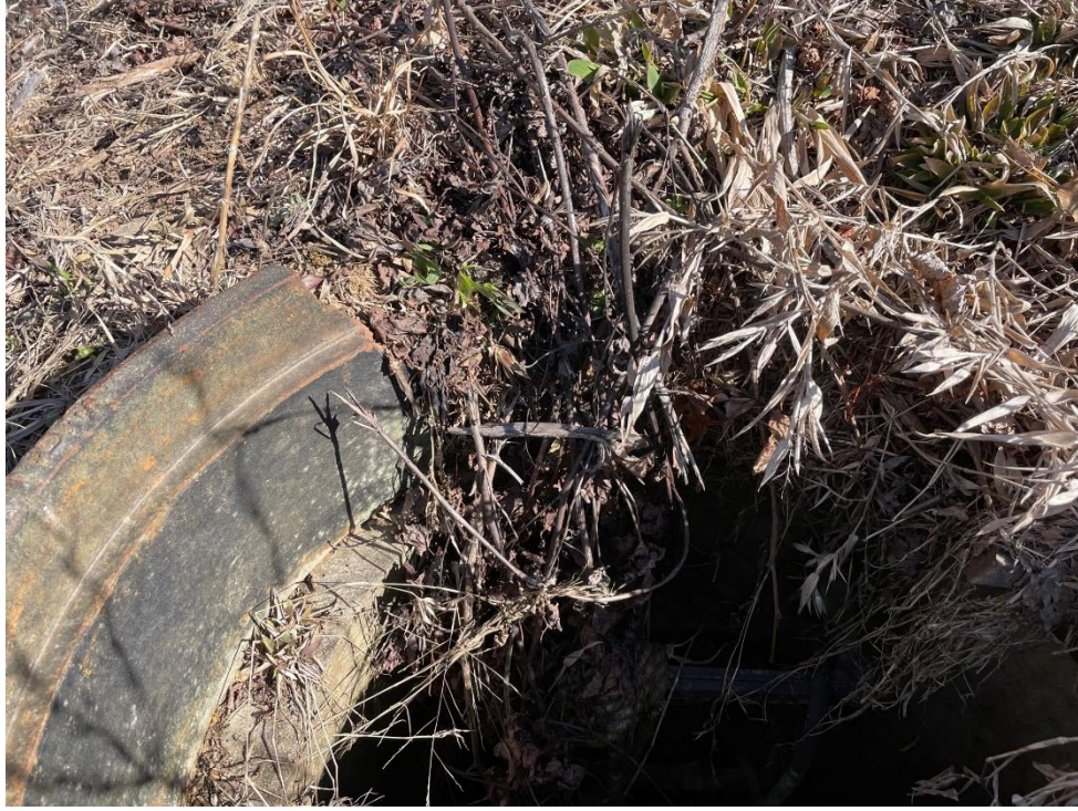
3/21/2023 Inspection – Broken manhole housing.
