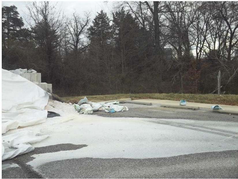
2/23/2023 Inspection – Salt staining on pavement
