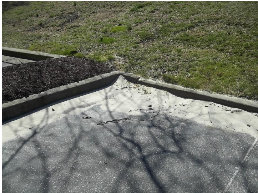
3/20/2023 Inspection – Sand migrating throughout parking lot
