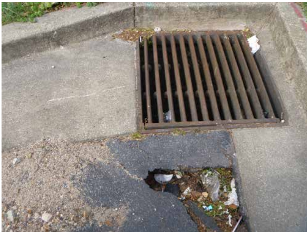
Figure 1. A view of a collapsed section of the parking lot, adjacent to an inlet, found near the Get Air Trampoline Park
