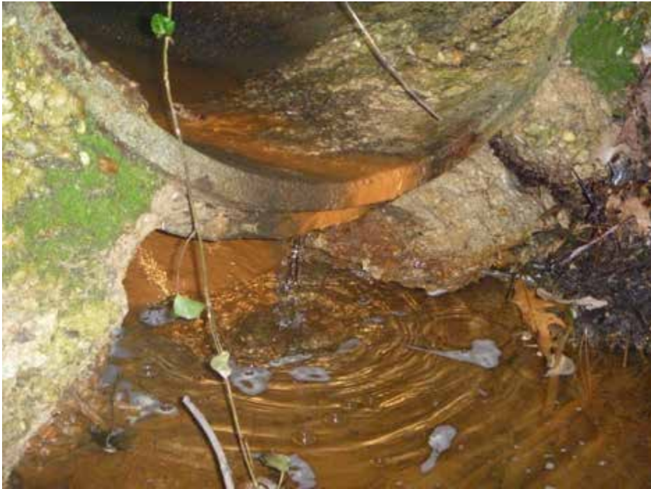
Figure 2. Evidence of undercutting below the outfall pipe (Facility ID: S14O014)
