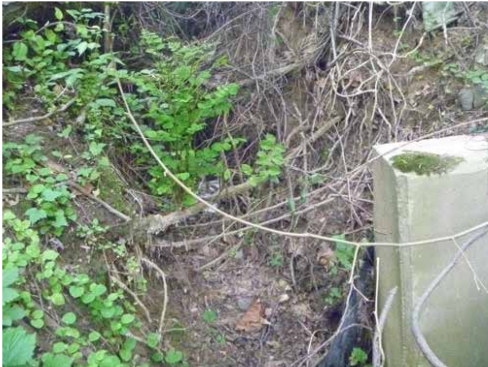
Figure 1. Evidence of erosion behind the endwall of outfall N04O045
