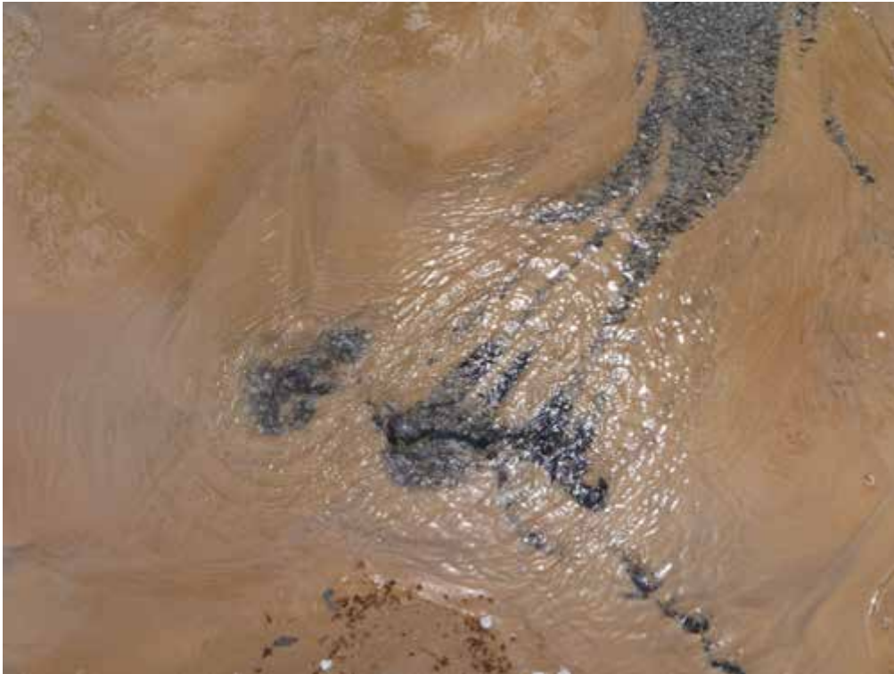
Figure 2. Evidence of water escaping from cracks in the parking lot; this appeared to be the source of the flooding
