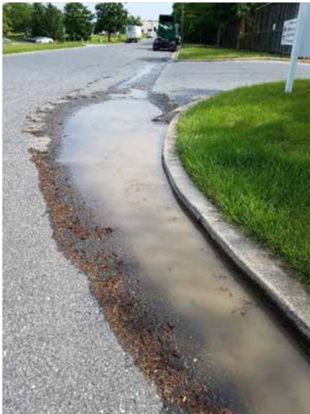
Figure 4. A view of accumulated water on the east side of the cul-de-sac
