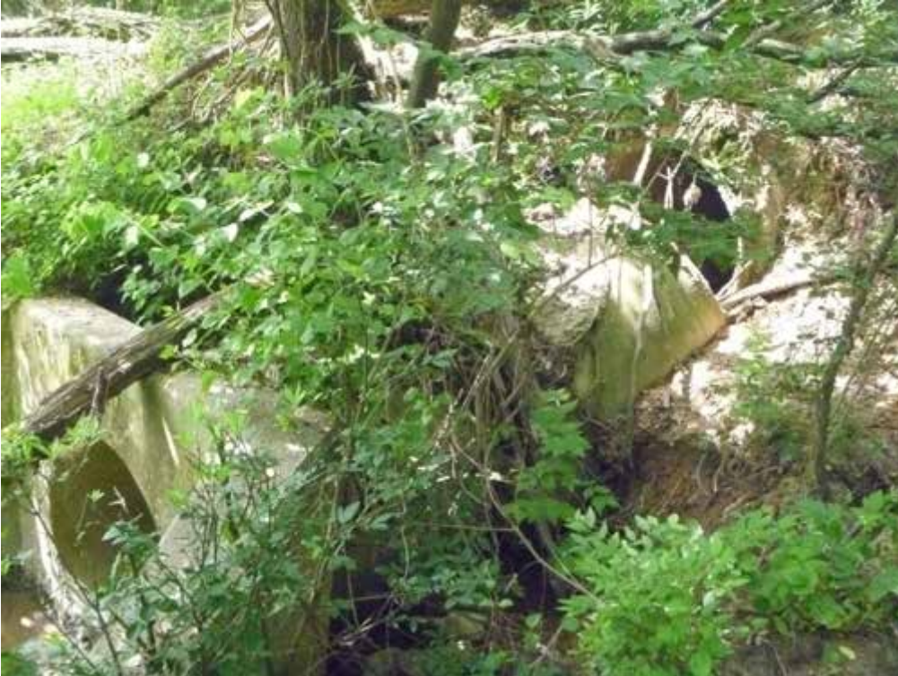
Figure 3. A view of the collapsed pipe sections (upper right and center) near outfall O04O005 (lower left)
