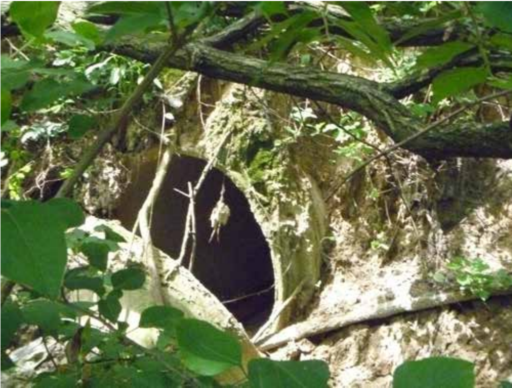
Figure 2. Evidence of erosion removing the bank surrounding the pipe network leading to outfall O04O005
