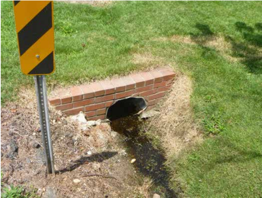
Figure 2. A view of the standing water in the pipe of inlet Q34C8I00003
