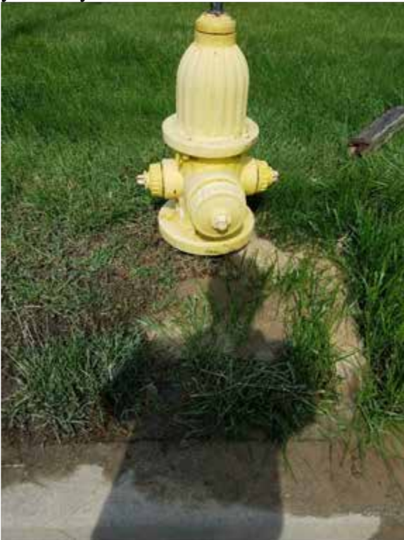
Figure 2. A view of beige foam found around the base of the fire hydrant (in front and to the right)
