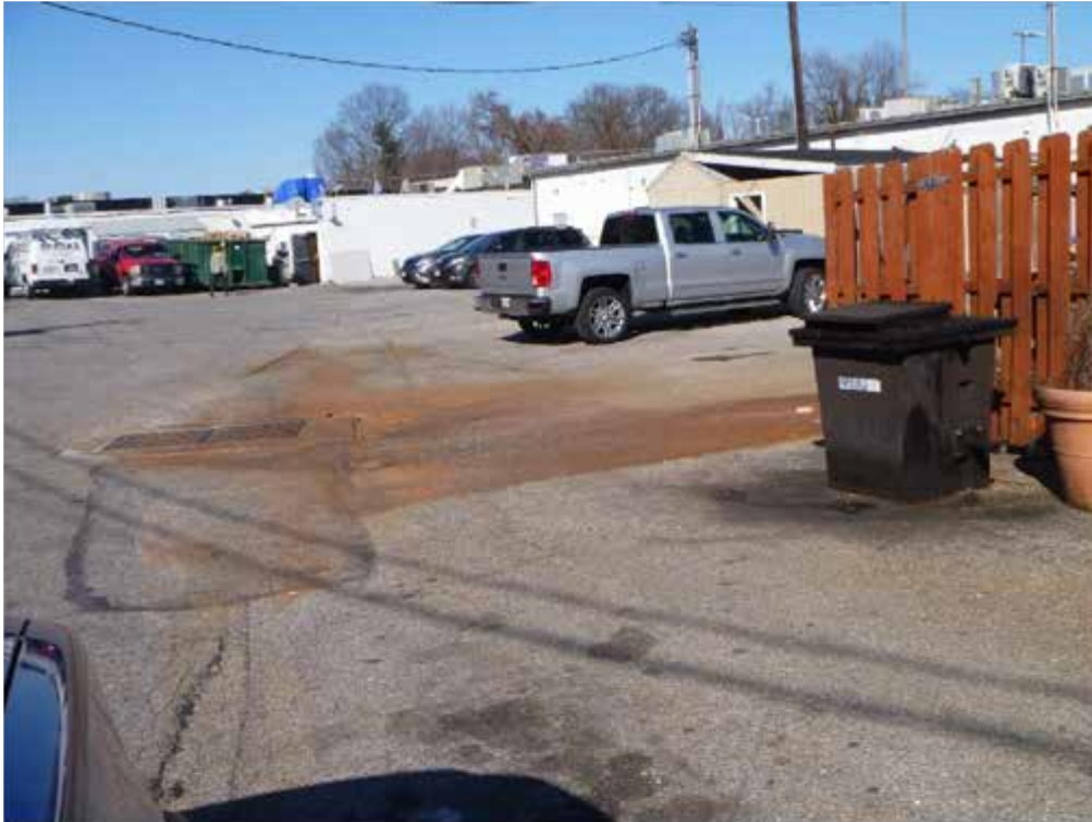
Figure 2. Signs of staining runoff and a kitchen waste grease bin near an inlet
