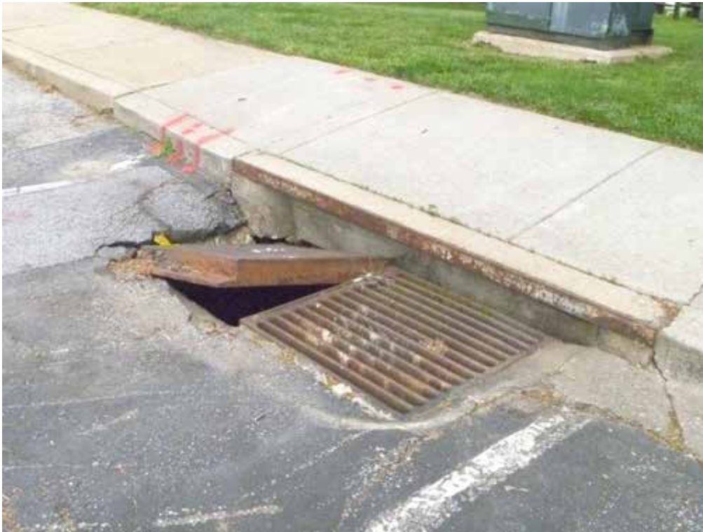
Figure 1. Evidence of inlet damage on Gatewater Court
