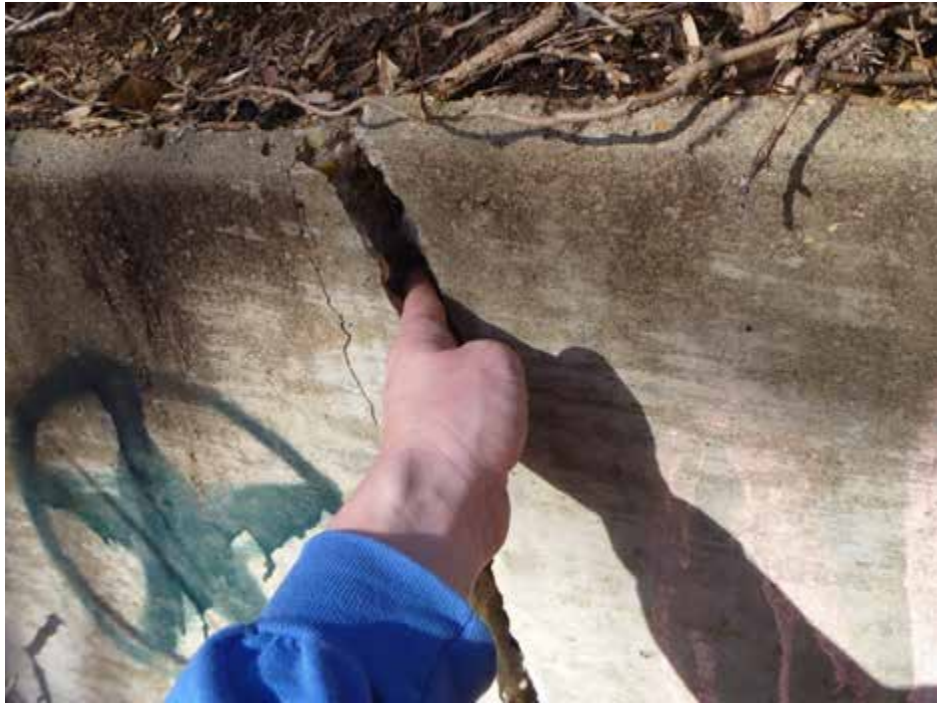
Figure 2. Detail view of the large crack (also shown in Figure 1) in the face of the endwall (Facility ID: S150022)
