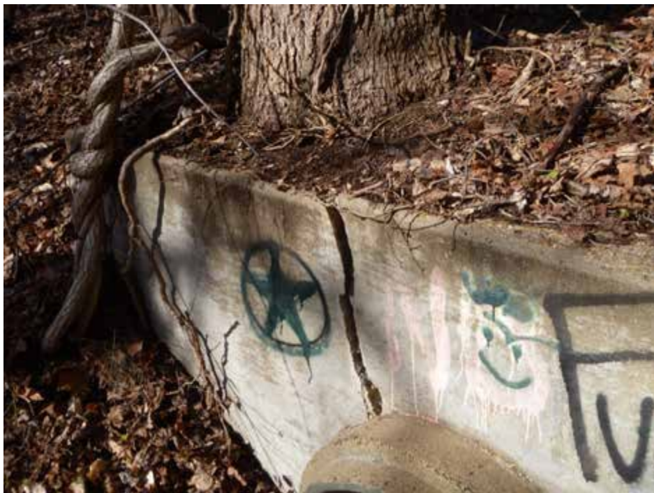
Figure 1. Evidence of a displacement in part of an endwall (Facility ID: S15O022) at the base of a large tree
