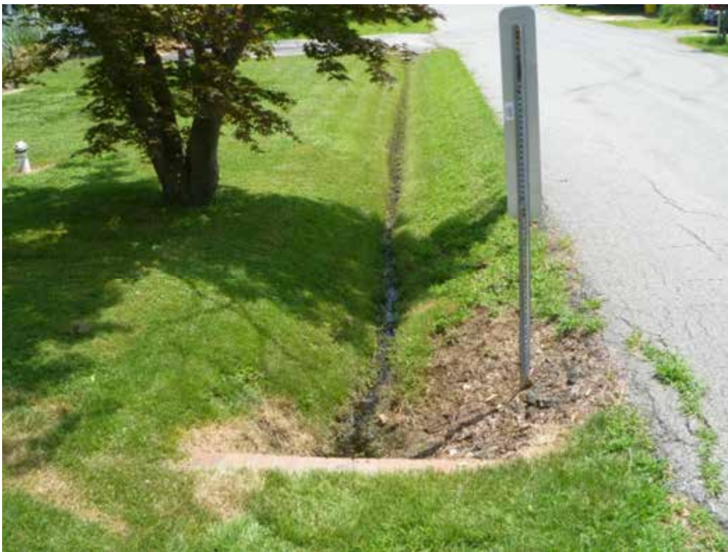
Figure 3. A view of the narrow ditch that drains toward inlet Q34C8I00003; the inlet headwall is seen in the foreground
