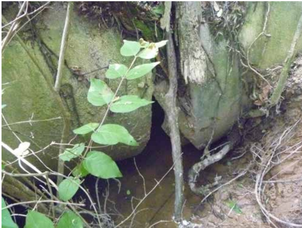
Figure 1. Evidence of erosion and water collecting under the pipe network leading to outfall O04O005
