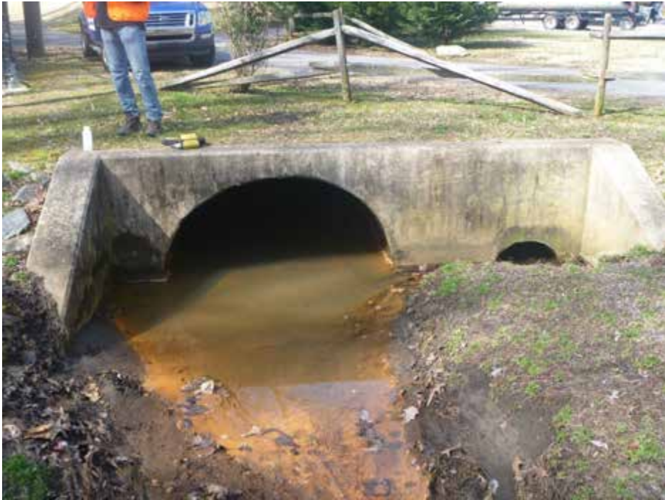
Figure 1. Conditions at outfall O22O014 on March 13
