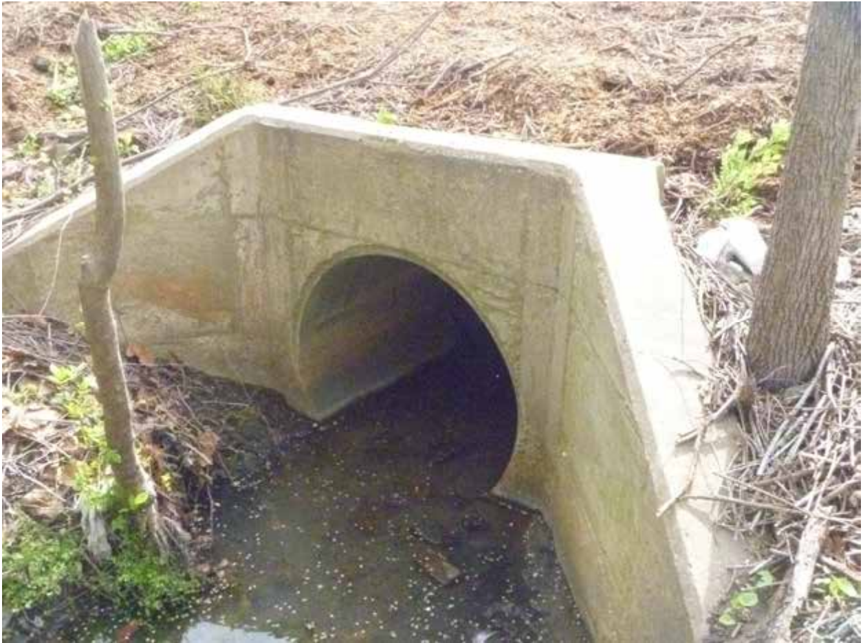
Figure 1. A view of conditions at Outfall S07O017 on April 24, 2019
