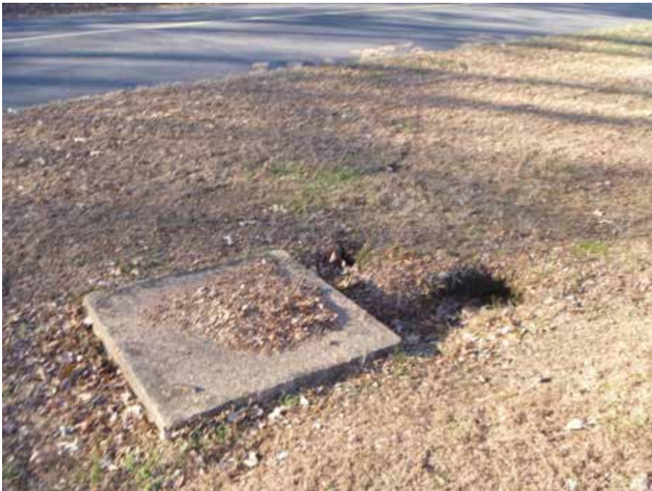
Figure 1. Evidence of soil subsidence immediately adjacent to the inlet, Feature ID W10I023
