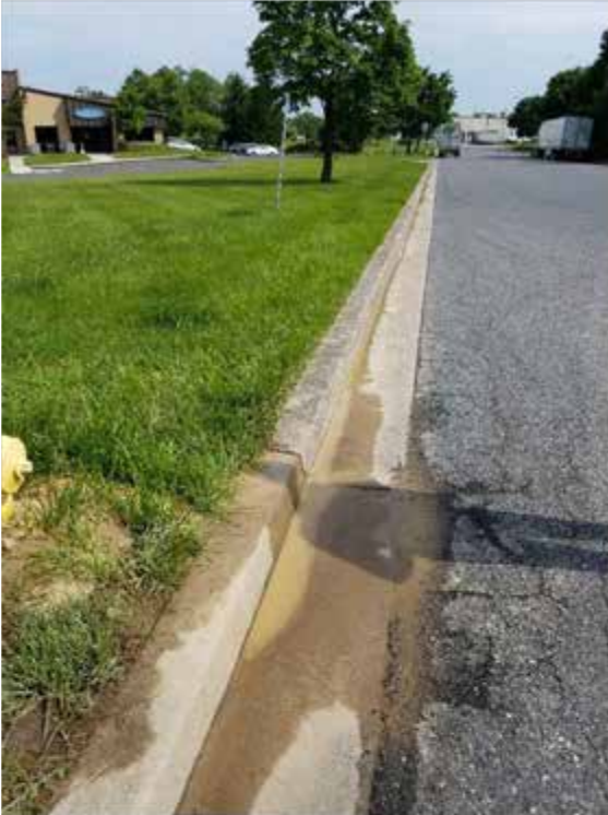
Figure 1. Flow observed from a leaking fire hydrant on the west side of Waterview Court; the yellow hydrant is visible on the left side of the photograph
