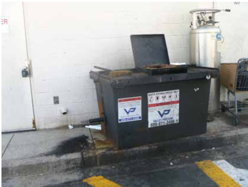
Figure 1. A kitchen waste grease bin found with an open lid, and dark grease stains on the pavement surrounding the bin, behind the Passion Asian Bistro restaurant on December 6
