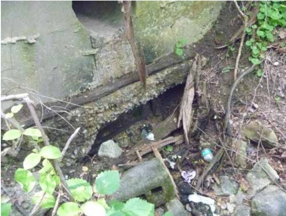
Figure 2. Evidence of erosion below the endwall of outfall N04O045
