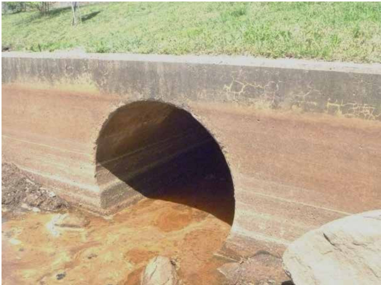
Figure 1. A view of conditions at Outfall S10O009 on April 24, 2019
