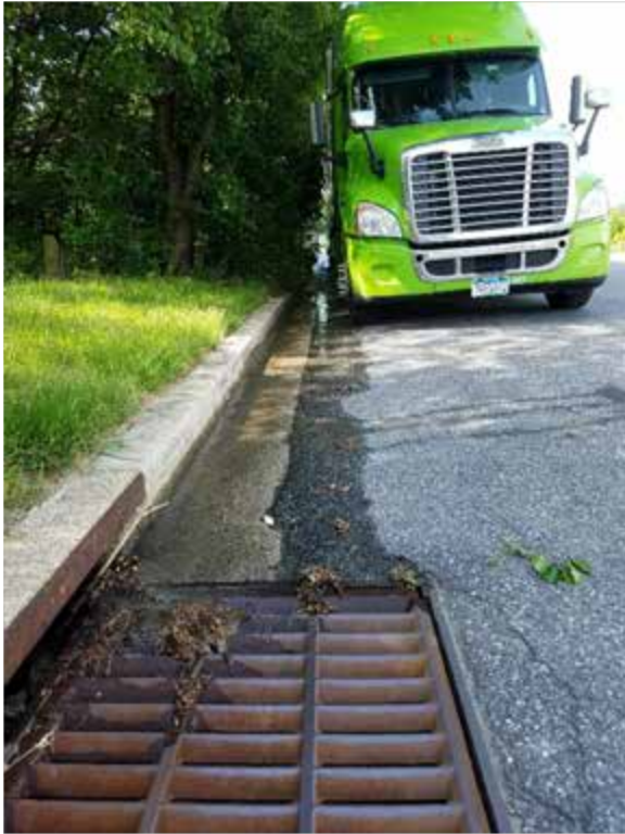
Figure 3. A view of flow entering the inlet from the east side of Waterview Court
