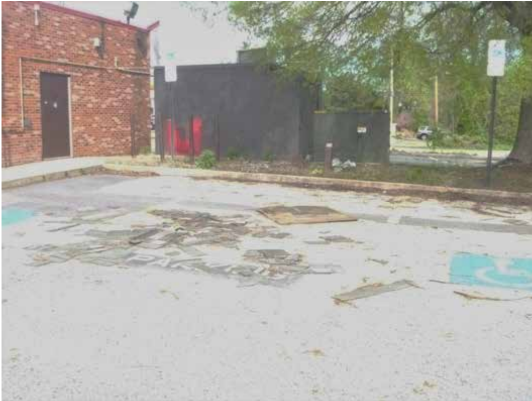
Figure 3. A view of some of the roof shingles observed in the parking lot
