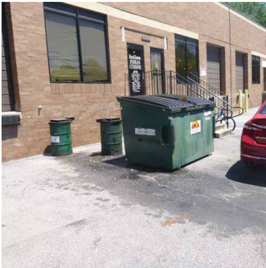
Figure 1. Stains near a kitchen waste oil bin and a dumpster found on July 9
