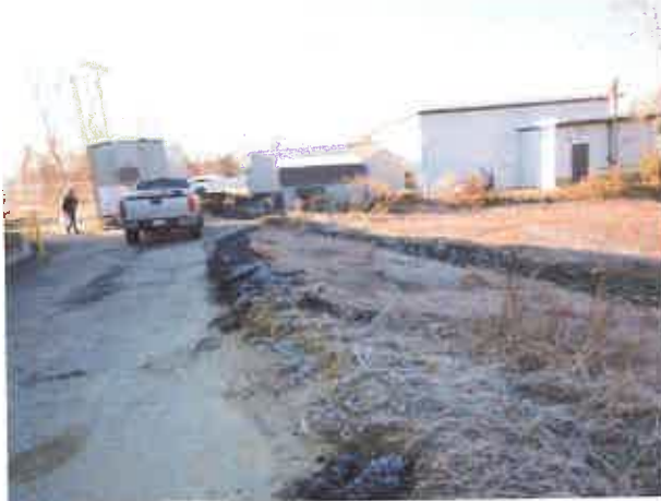
Asphalt berm required maintenance
