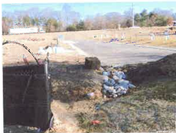
Curb cut where runoff exits and created erosion; runoff pooled near inlet protection; maintenance required
