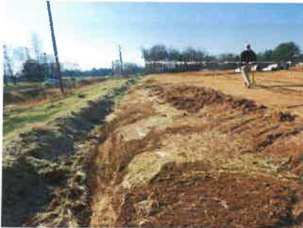
Re-grading and re-stabilization required
