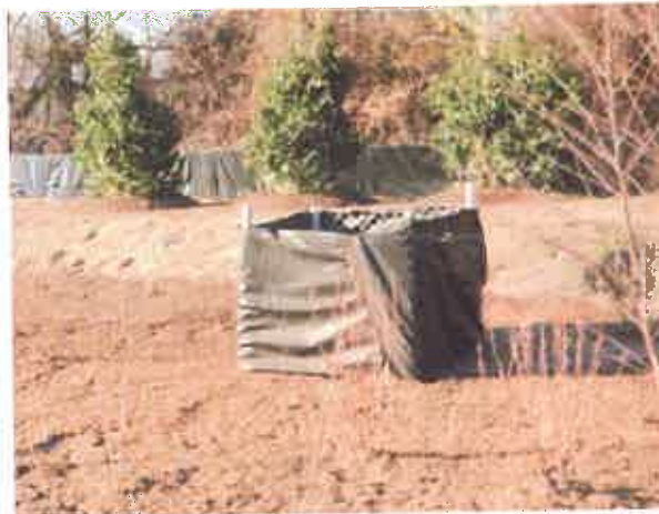
Inlet protection not per specification
