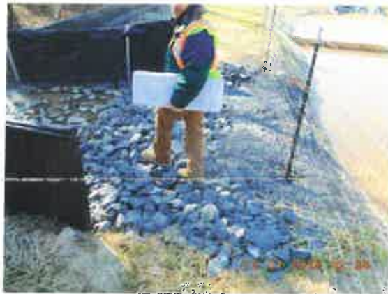
Sediment trap outlet with pooled sediment laden water
