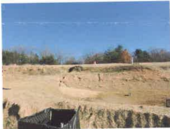
Re-stabilization required; rill erosion near future environmental site design (ESD) practice
