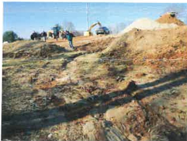
Re-stabilization required; rill erosion
