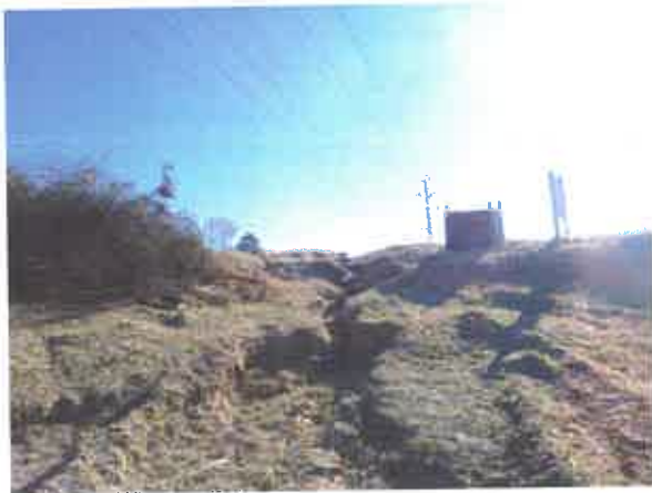
Re-stabilization required; rill erosion
