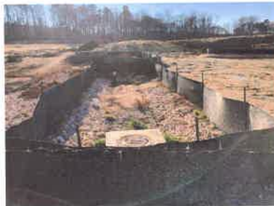
Runoff not diverted around practice
