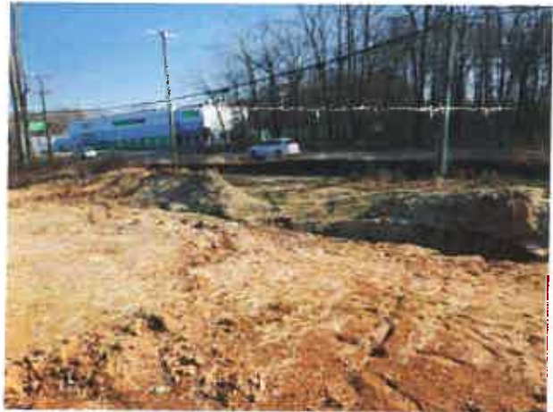
Re-grading and re-stabilization required; unapproved dike concentrated flow
