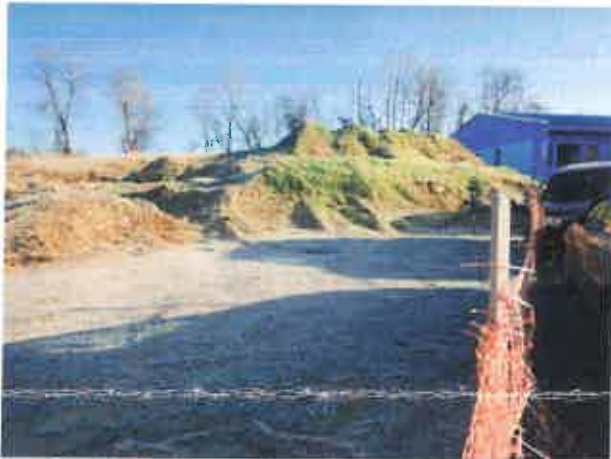
Stockpile larger than indicated on plans
