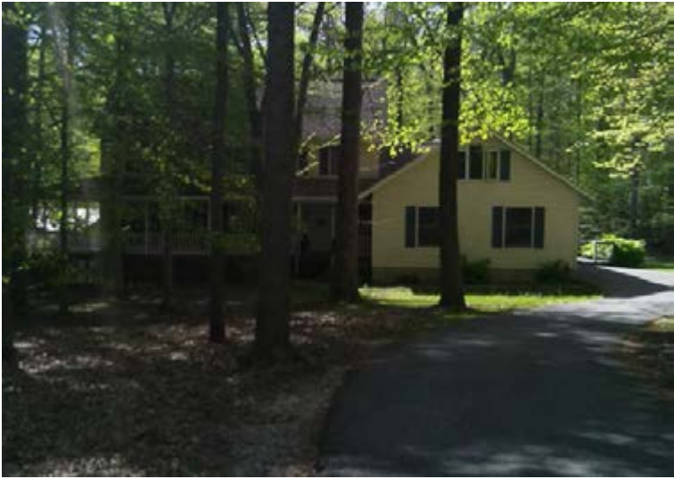
This house did not have any downspouts. As evidenced from the photo, the driveway area sheet flows into the adjacent wooded area.
