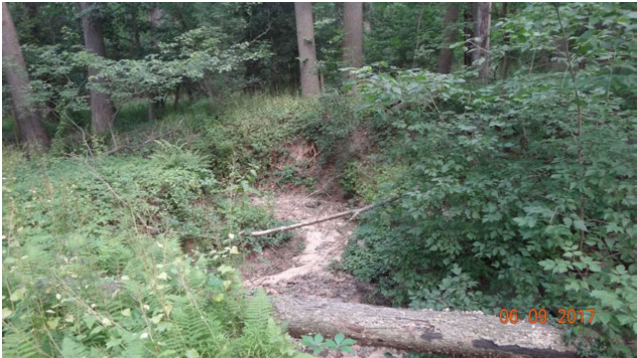
Figure 4. Further evidence of erosion observed downstream of the plunge pool of the outfall
