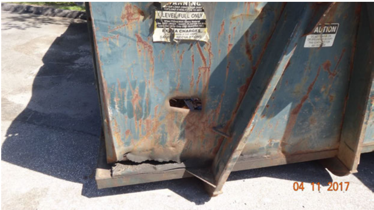
Figure 6. A rusting rollaway dumpster exhibiting a puncture hole on the side and a tear at the bottom; note stains on the pavement (left)
