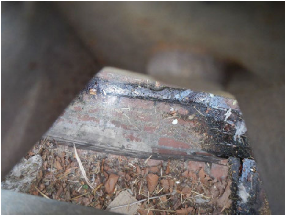
Figure 3. View inside the first inlet up the network from outfall R20B5O005, showing wet conditions
