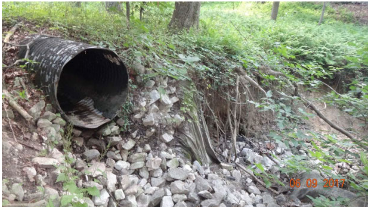
Figure 1. View of outfall M12E4O001 (left) showing an eroded channel (right) that has developed, probably from strong discharge flows; note the drop in elevation covered in a plastic sheet to the right of the pipe opening in the photograph
