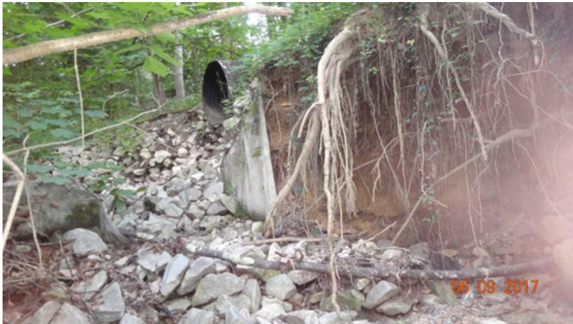
Figure 2. View of the eroded bank, showing exposed roots, that has developed to the right of the pipe (as seen looking at the pipe opening); note the plastic sheeting that covers the ground near the pipe which has developed into a channel guide for flows
