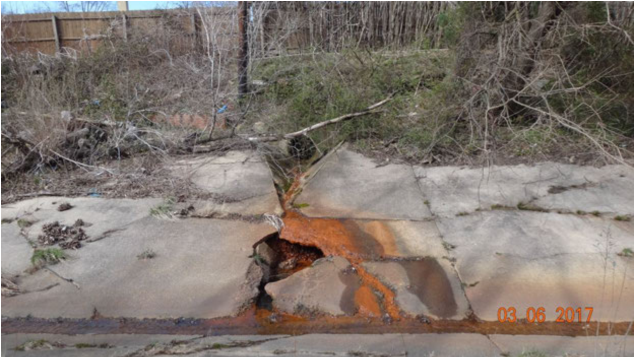
Figure 2. View looking across the channel, showing the extent of damage immediately downstream of outfall M08H2O008 (top center); note that discharge from either outfall may enter the large opening due to its location near the base of the main channel
