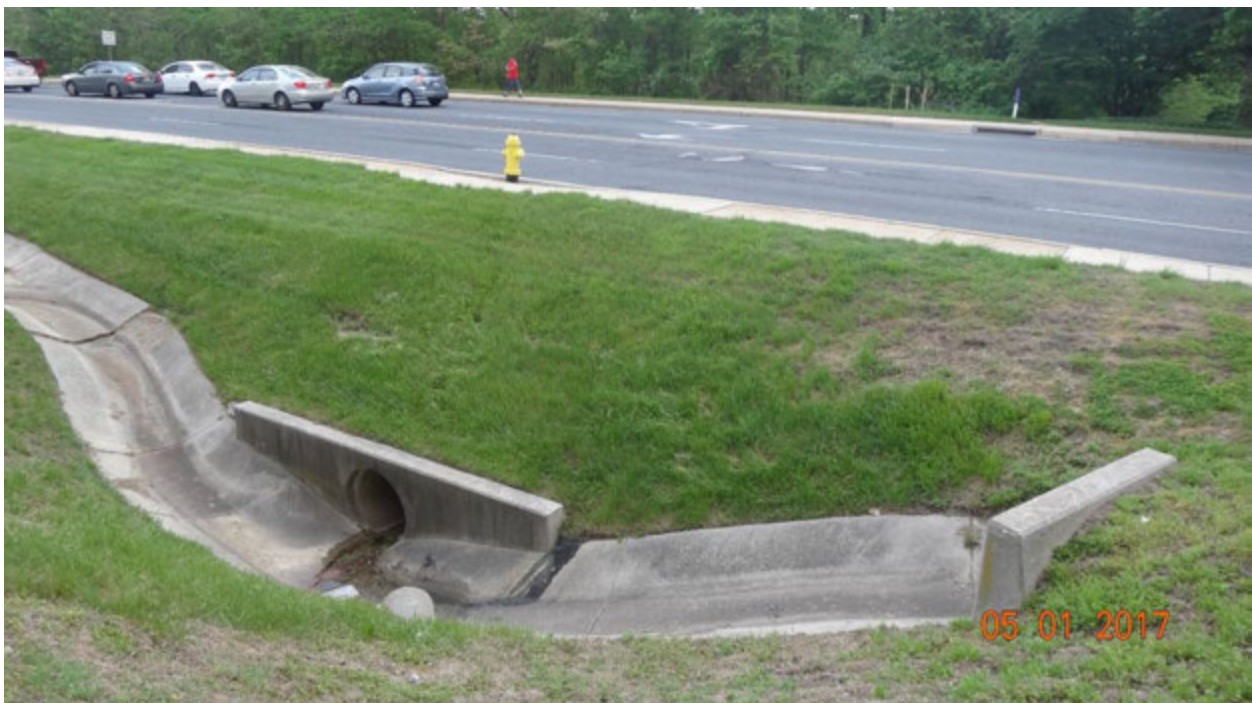
Figure 3. View of the channel relative to the culvert under Hospital Drive, note the small pipe jutting out of the side of the channel (lower left, facing away from the viewer) and releasing effluent that flows toward the culvert opening
