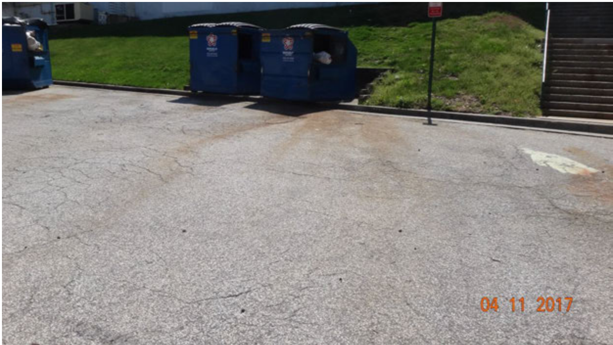
Figure 2. Orange stains evident on the pavement near three of the dumpsters that suggest prior leakage
