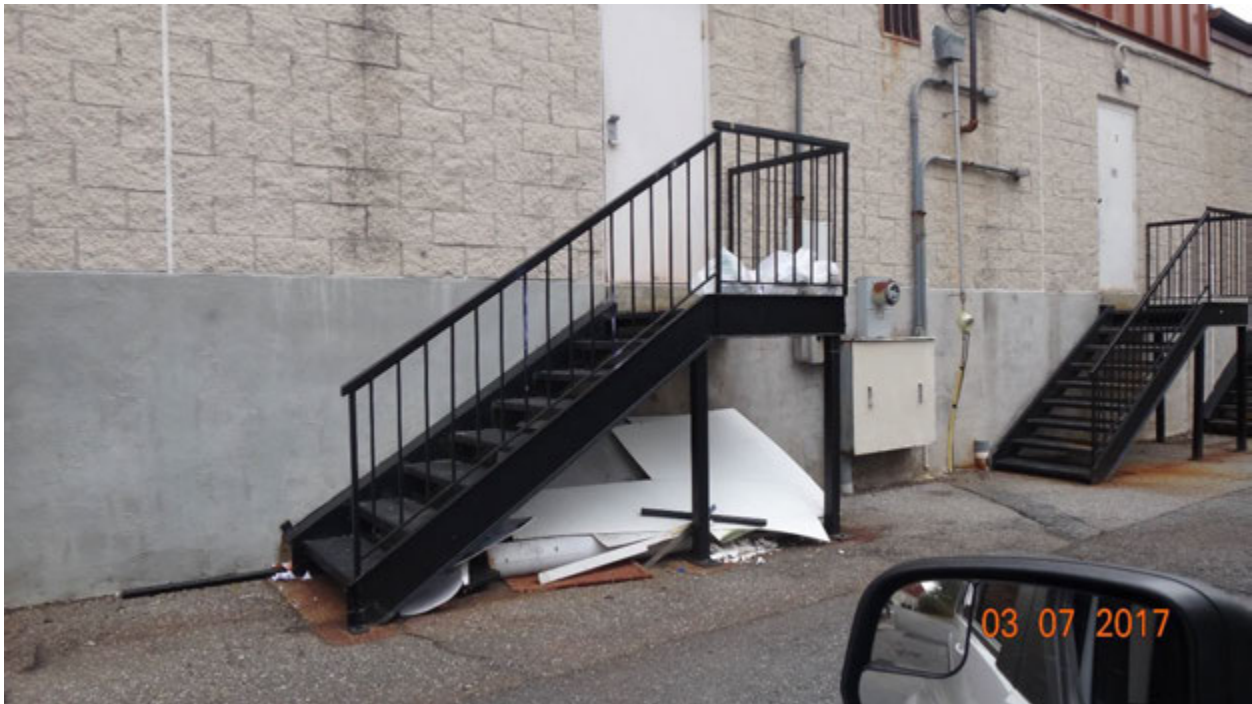
Figure 3. Bags of trash and loose debris behind and beneath the rear door for Suite R
