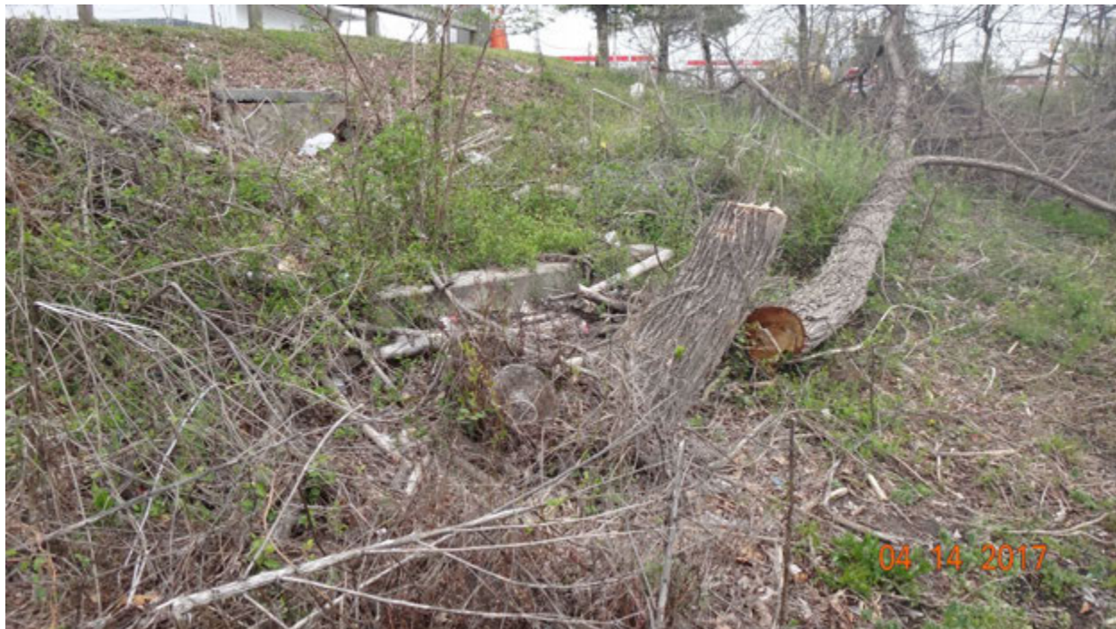
Figure 1. View of the visible headwall of outfall F09G5O001 (center) and the arranged sticks placed at the pipe opening, which is effectively blocked by plant material; note that the tree trunk in the foreground had been sliced once with a saw, but not further divided into sections
