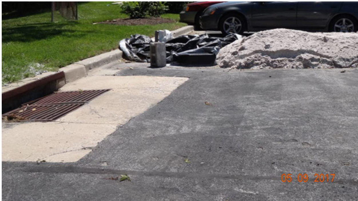
Figure 1. A pile of road salt found uncovered on the parking lot near a stormwater inlet; note the black tarp and concrete blocks to the left of the pile in the photograph
