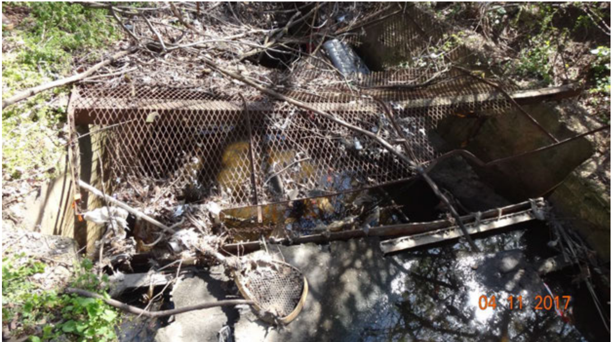
Figure 3. View of a supported expanded metal panel and at least two panels that had fallen into the stream; a portion of one is seen just above the head of the lacrosse stick in the photograph, portions of another can be seen under and around the grey plastic (top center) which was part of a broken shopping cart
