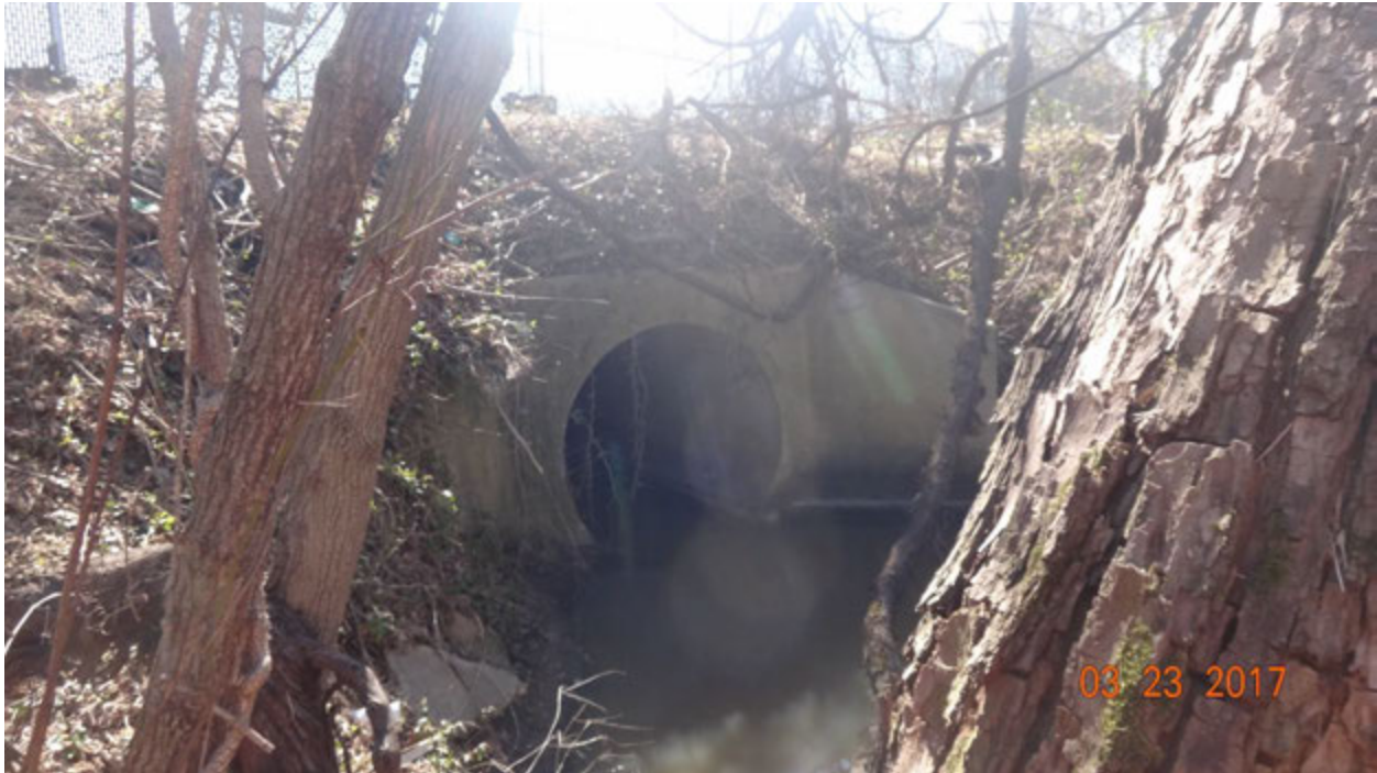
Figure 1. Conditions at outfall M06C4O008, showing pooled opaque water on March 23
