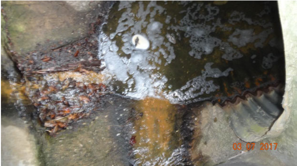
Figure 2. Evidence of pooled water in the nearest curb inlet; note flow from the two lines entering the inlet box (below and left)
