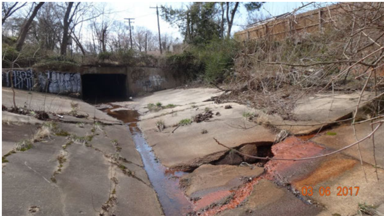
Figure 1. Collapsed infrastructure (foreground right) found in the receiving channel for target outfall M08H2O011
