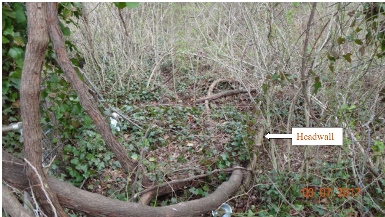
Figure 1. Outfall M08D5O001 found buried with sediment and vegetation
