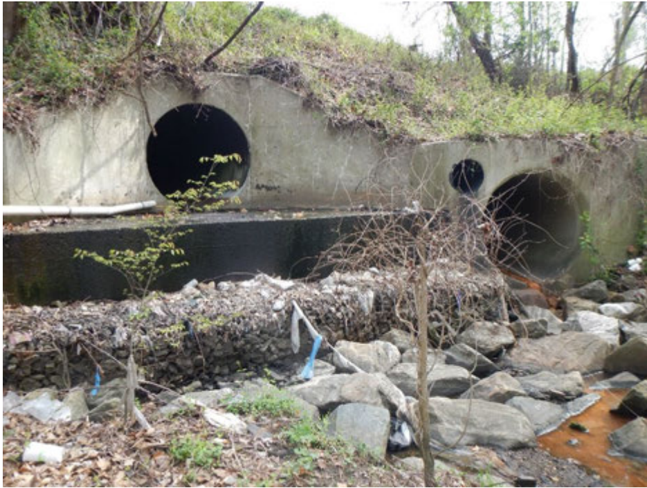
Figure 1. Conditions at outfall R20B5O001 where the team documented and collected samples of the flowing effluent seen in the rightmost pipe opening; the other two pipes discharging at the headwall (left and center) did not have flowing conditions at the time of the site visit
