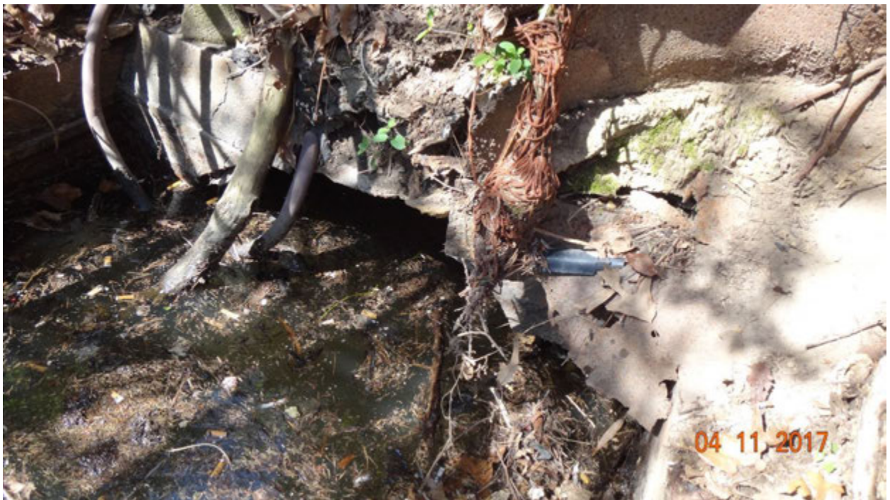
Figure 4. View of some of the impeded water that extends back into the culvert under Cloverleaf Drive
