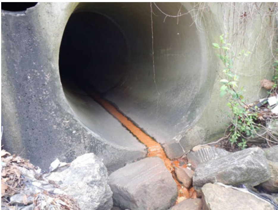
Figure 2. View of the orange silty effluent flowing in the rightmost pipe of outfall R20B5O001
