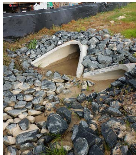
Sediment laden water was being discharged off-site from an outlet. Fabric needed under outlet protection.
