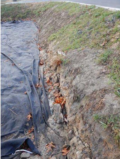
Area reserved for future stormwater management (SWM) not adequately protected
