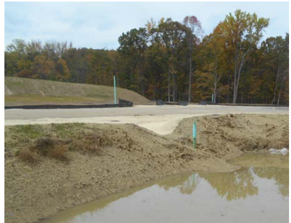
Riprap inflow protection (RIP) required
