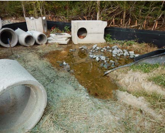
A clear water diversion pipe (CWDP) was not installed correctly; clear water was being discharged onsite instead of off-site.
