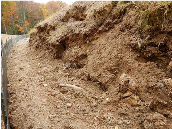
Stockpile required re-stabilization
