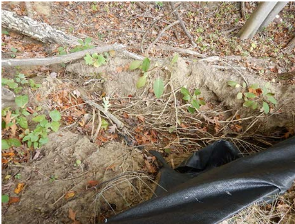
RSF not installed per specifications; sediment was exiting site
