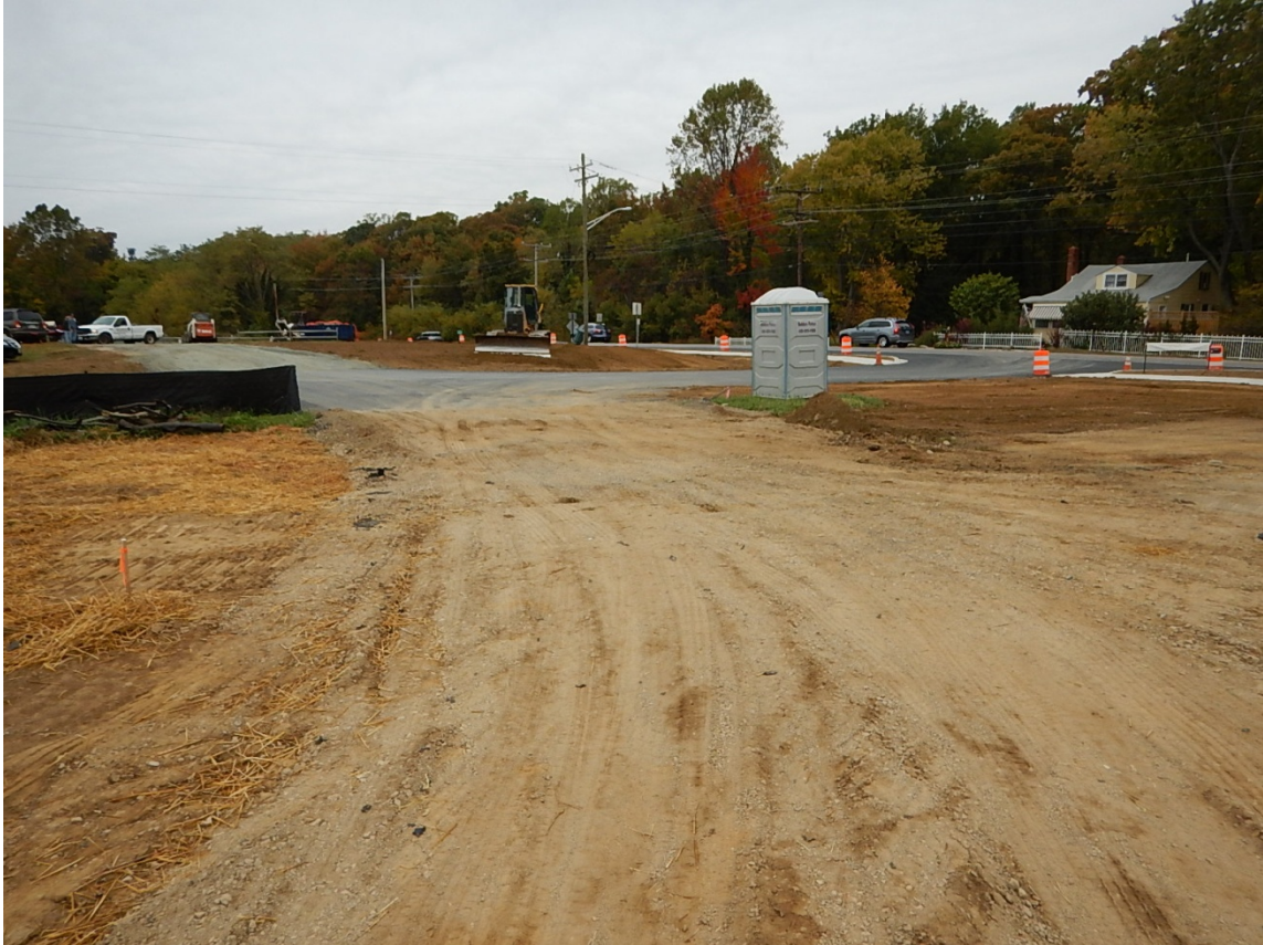
An SCE was required; the inspection report requested that one be installed
