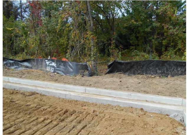
RSF required maintenance
