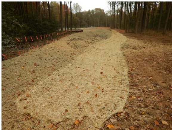
Dike to basin not constructed per plan and modification not approved by the SCD
