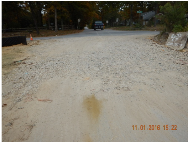
Stabilized construction entrance (SCE) required maintenance
