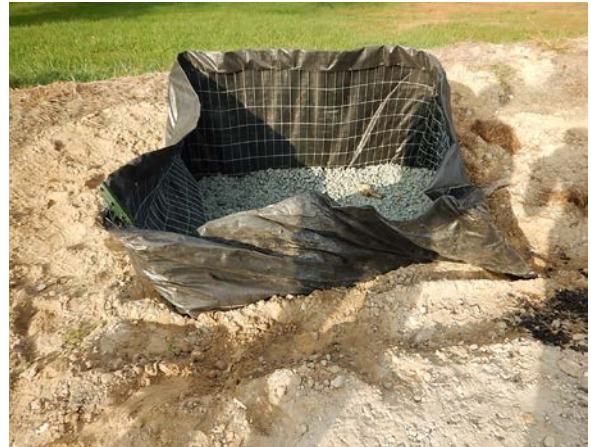
Inlet protection not installed per specification
