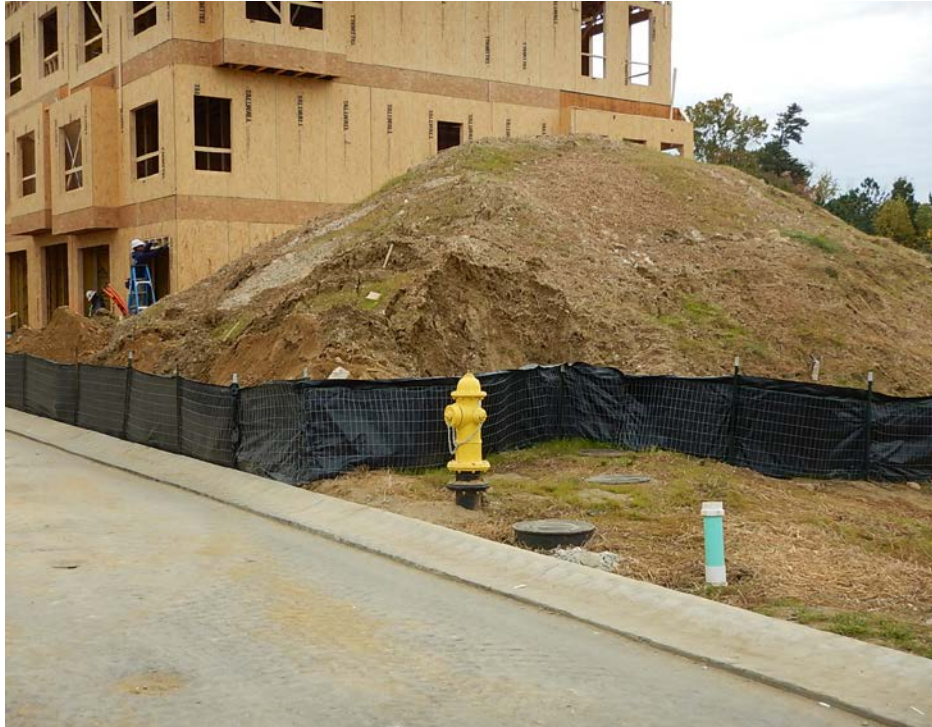
Stockpile required re-stabilization
