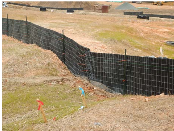
RSF receiving concentrated flow
