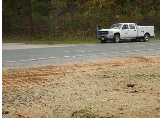
Per inspector's instruction, RSF along the roadway was not installed as required by the plan
