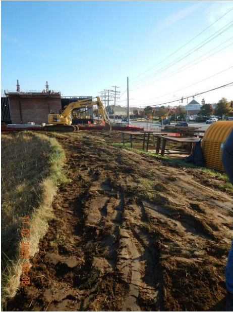
Disturbed earth above sediment trap required stabilization
