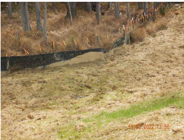
RSF in need of maintenance
