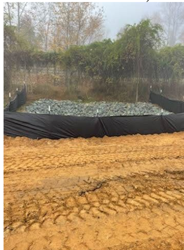
RSF installed to protect headwall from sediment contamination (County submitted 11/15/2022)
