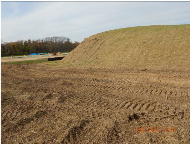
Stockpile missing RSF
