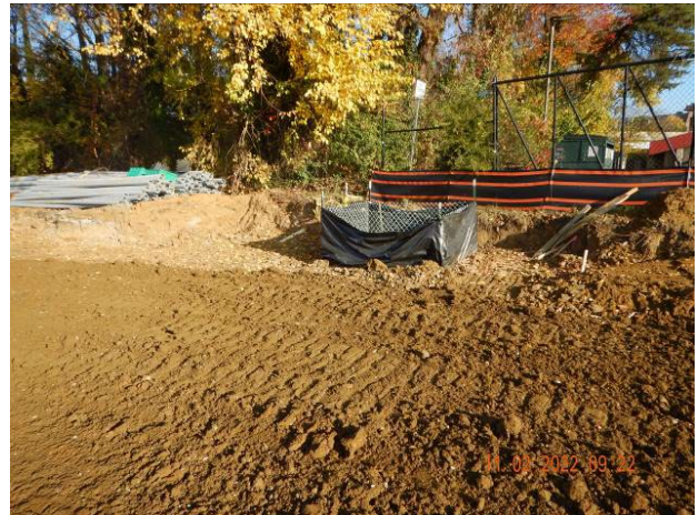
SIP in need of maintenance (11/15/2022 follow-up inspection report noted site was in compliance and 11/22/2022 inspection report noted SIP no longer required due to curb and gutter installation)
