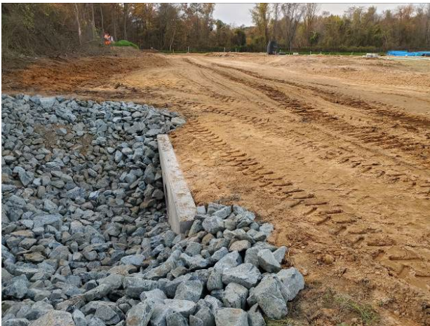
RSF missing from headwall and adjacent disturbed area unstabilized
