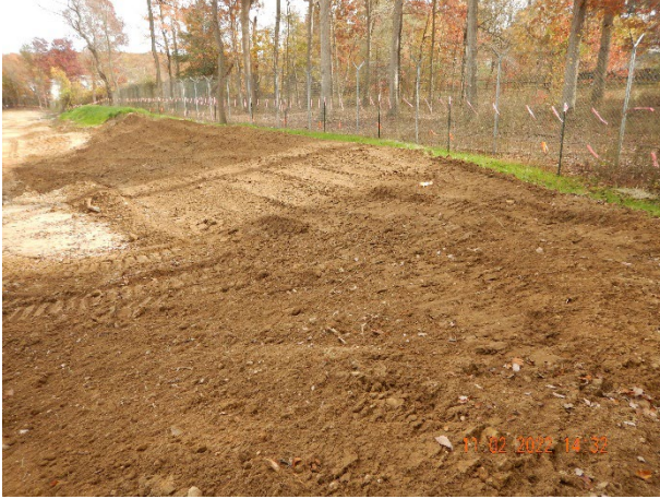
Perimeter in need of stabilization
