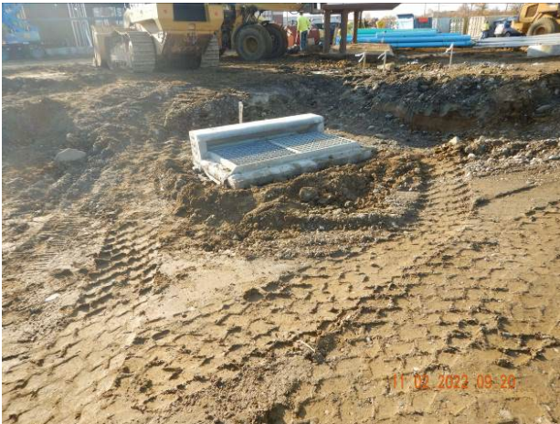
Missing SIP (11/15/2022 follow-up inspection report noted site was in compliance and 11/22/2022 inspection report noted SIP no longer required due to curb and gutter installation)
