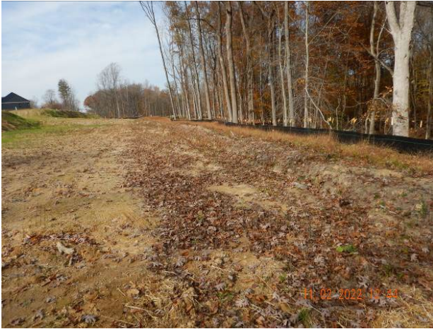
Unstabilized disturbed earth near sediment trap
