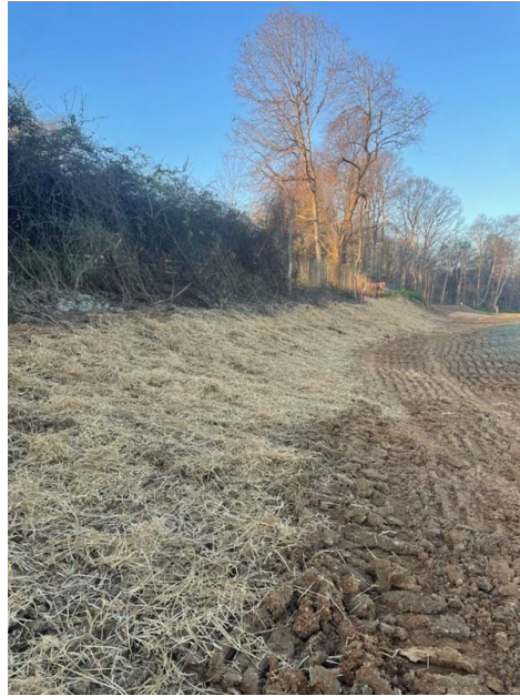
The temporary bypass swale was removed for mass grading and the perimeter stabilized near the headwall (County submitted 11/19/2022)
