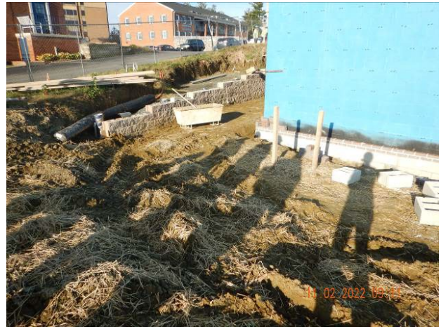
Disturbed earth requiring stabilization around building (11/15/2022 follow-up inspection report noted site was in compliance and the 11/22/2022 inspection report noted area disturbed due to active water line installation)
