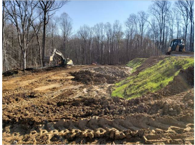
Follow-up documentation depicts active grading of site to remove trap. (County submitted 11/19/2022)
