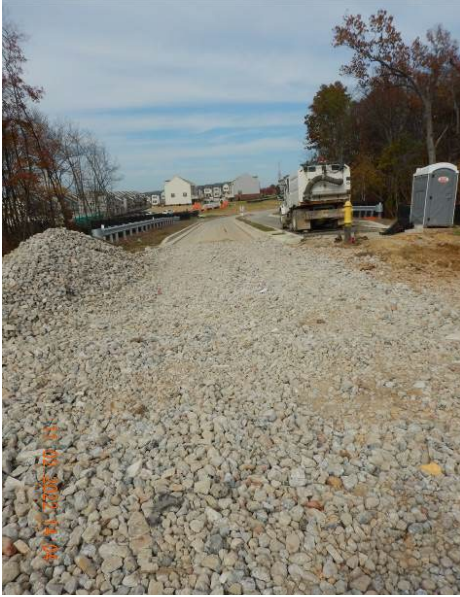
SCE in need of maintenance
