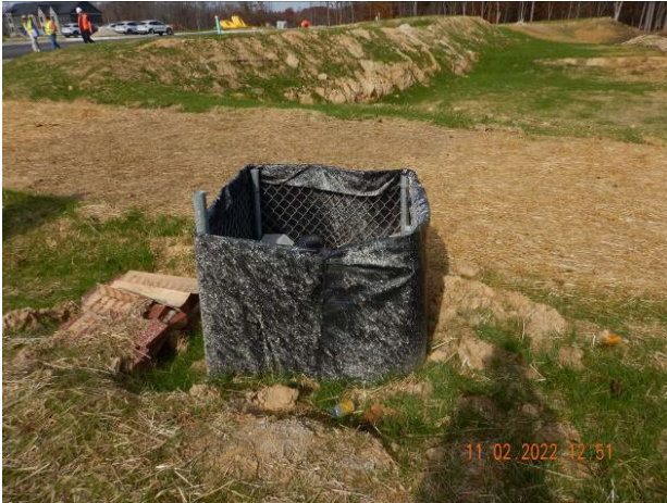
SIP in need of maintenance
