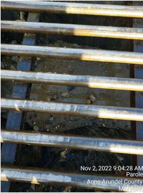
Wash rack in need of sediment cleanout
