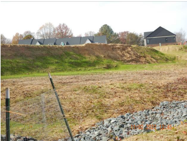
Unstabilized disturbed earth
