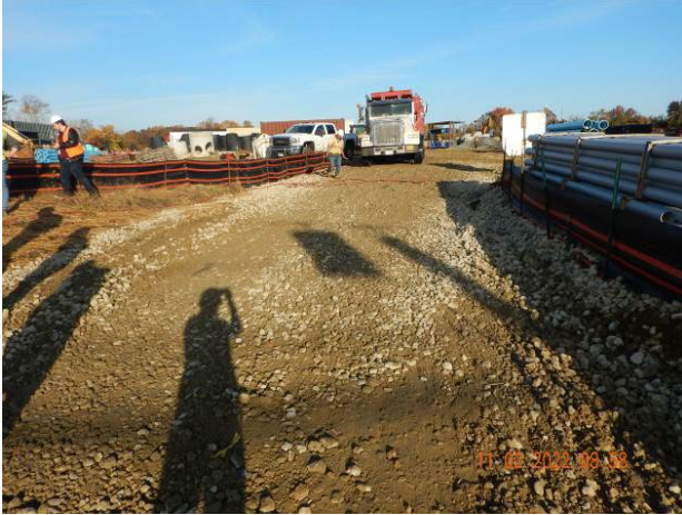
SCE in need of maintenance
