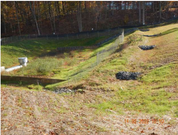
RIP not installed per specification
