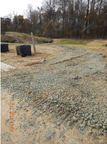
SCE to stockpile required maintenance
