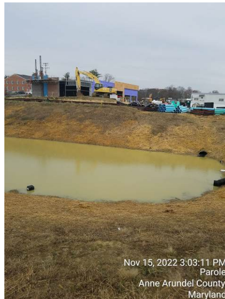
Restabilized slopes (County submitted 11/15/2022)
