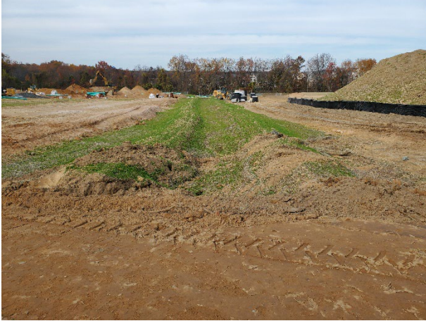
Unstabilized earth disturbance at the high side of the temporary bypass swale
