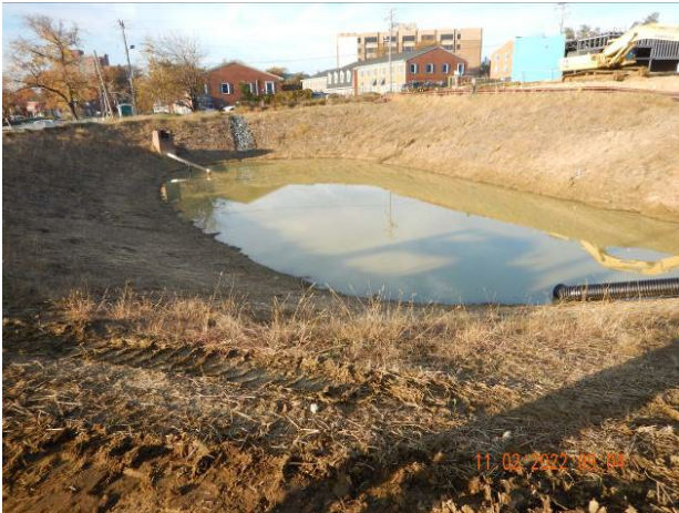
Sediment trap slopes in need of stabilization
