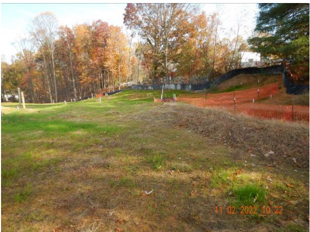
Earth dike not on the approved plan installed
