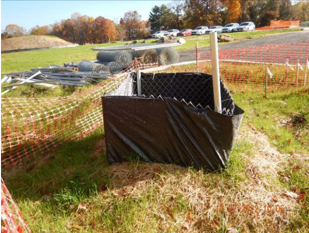
SIP in need of repair
