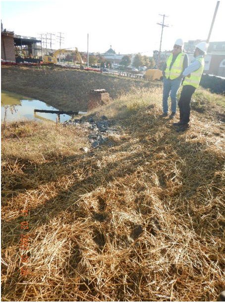
RIP not installed per specification (11/15/2022 follow-up inspection report noted site was in compliance)
