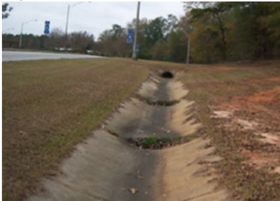
Cracks and joint separation in concrete channels, removal of vegetation may prevent future damage.
