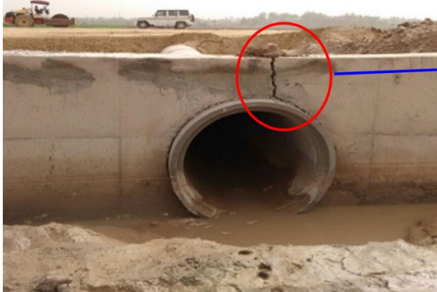
A crack in the culvert headwall.
