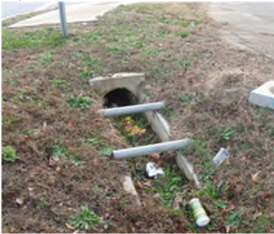
Pipe conveyance filled with vegetation.
