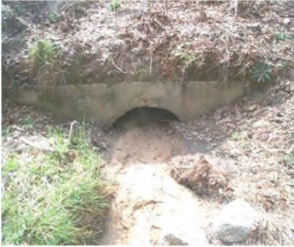
A pipe filled with sediment, inhibiting flow.
