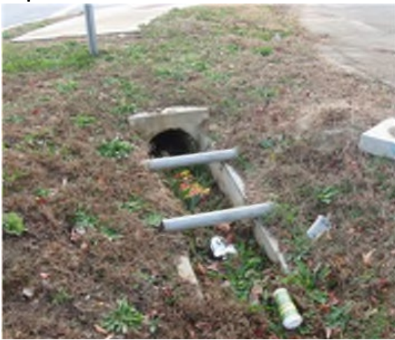
Pipe conveyance filled with vegetation.
