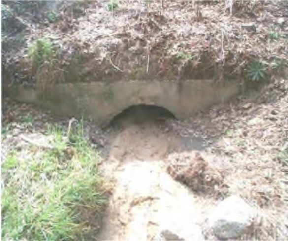
A pipe filled with sediment, inhibiting flow.
