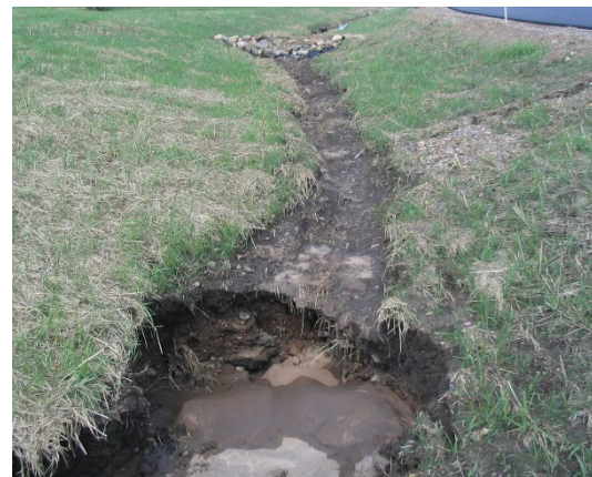
Slumping within a drainage swale.
