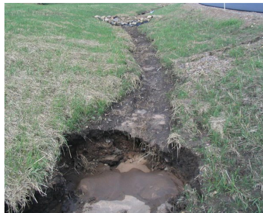
Slumping within a drainage swale.
