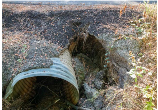
Evidence of erosion around a culvert.
