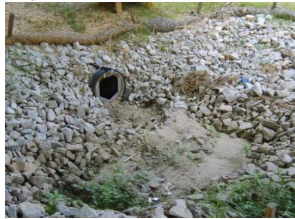
Sediment accumulation at swale inlet.
