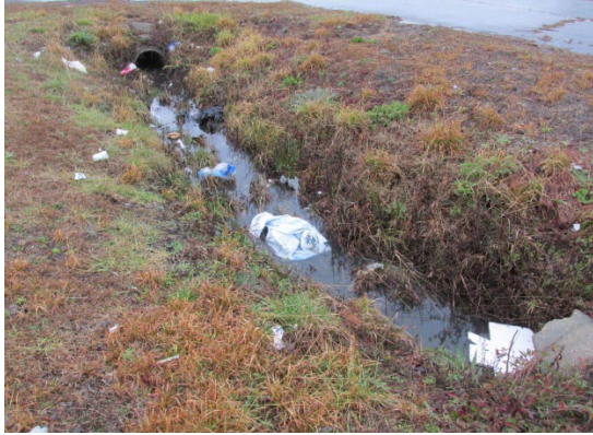
Litter and debris within a ditch.
