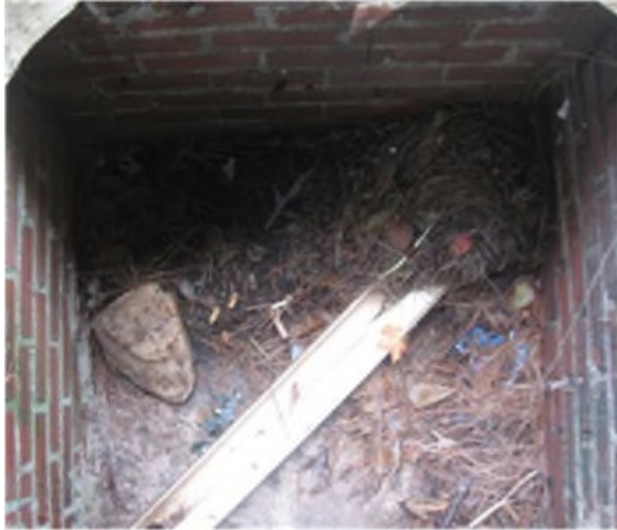
Sediment and debris inside stormwater inlet
