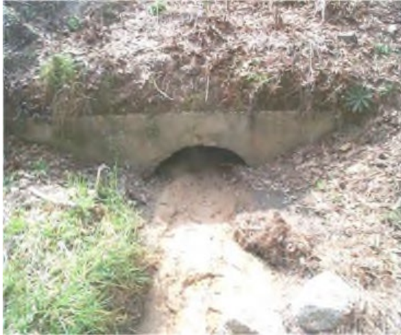
A pipe filled with sediment, inhibiting flow.
