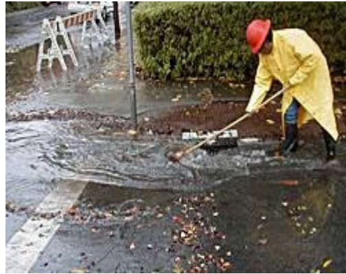
Standing water around an inlet may indicate a blockage.
