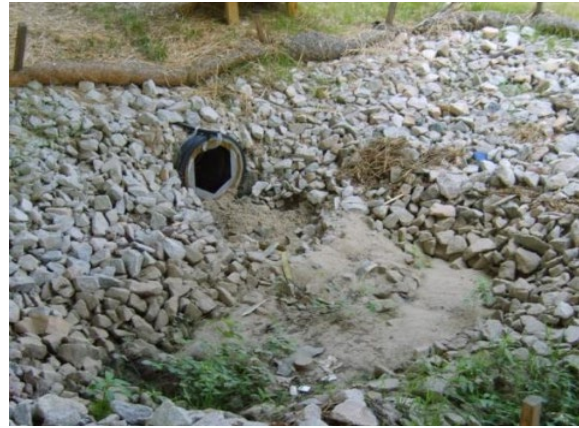
Sediment accumulation at swale inlet.
