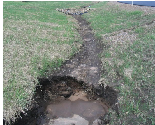
Slumping within a drainage swale.
