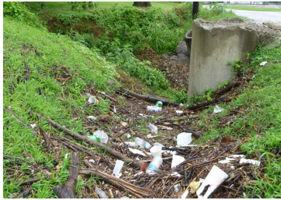
Litter and debris within a swale.
