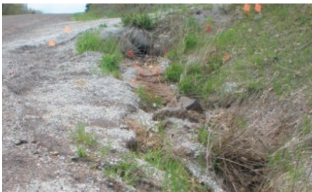
Erosion and slumping within a drainage ditch.
