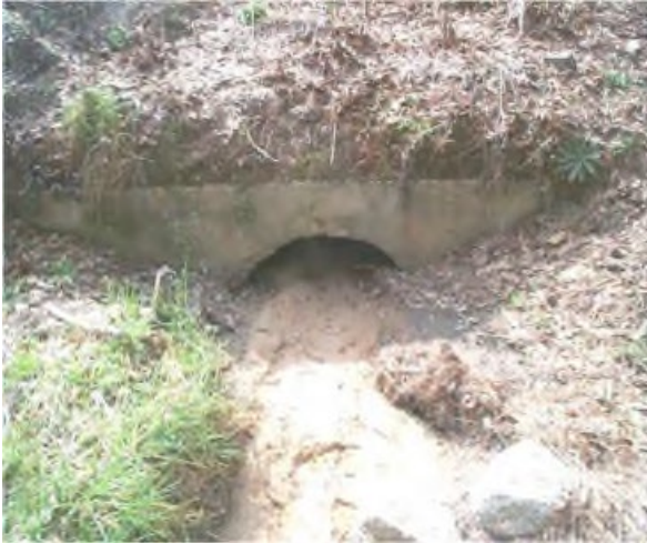
A pipe filled with sediment, inhibiting flow.
