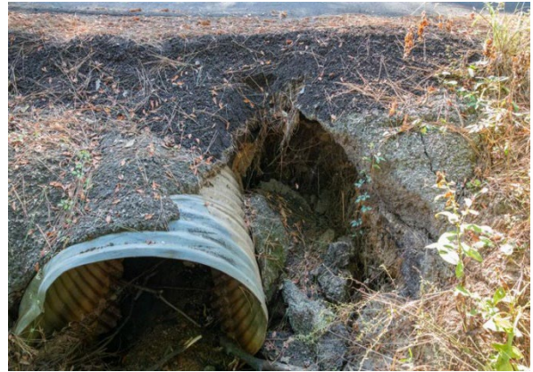
Evidence of erosion around a culvert.
