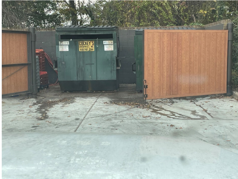
11/7/2023 Inspection – Dumpster area staining.
