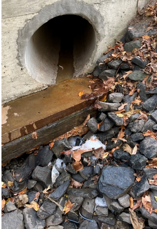
Outfall M08C8O00003 on 11/17/23 with foam at rip rap.
