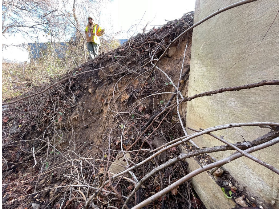
11/30/2023 Inspection – Erosion on the sides of the endwall.
