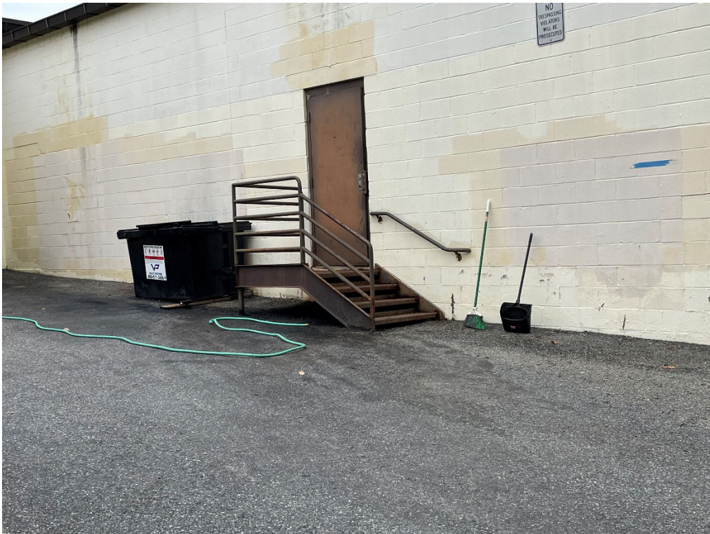
11/7/2023 Inspection – Cleaning supplies near grease bin.
