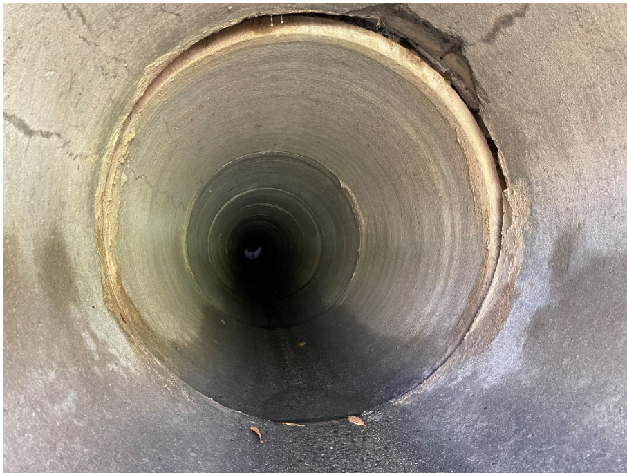
11/30/2023 Inspection – Outfall M06C1000001 barrel.
