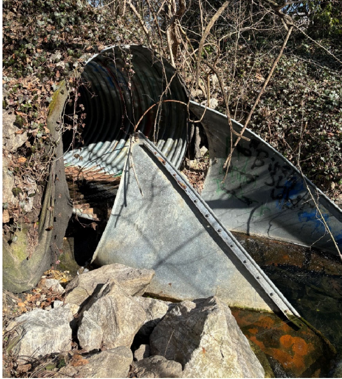
02/08/2024 Inspection – Overview of M05B5O00001 and separation of the end section from the pipe.
