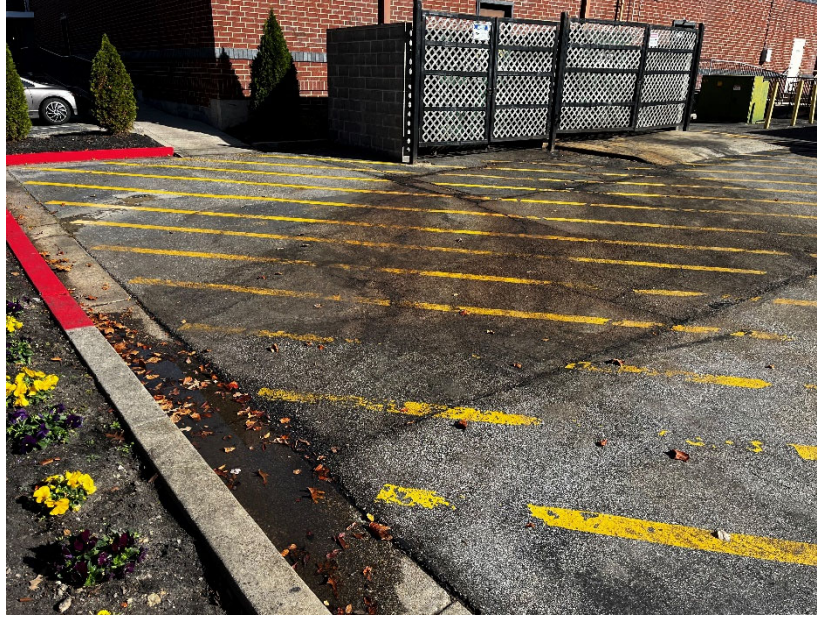
11/7/2023 Inspection – Dumpster area staining.
