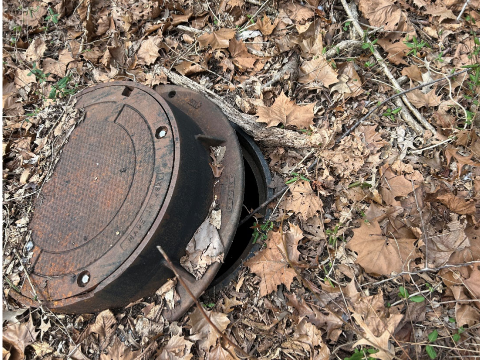
2/8/2024 Inspection – First upstream manhole, metal cast fallen off.
