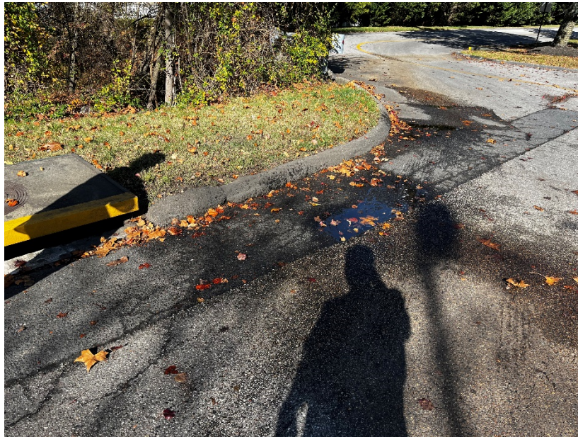
11/7/2023 Inspection – Dumpster area staining/sudsy fluids.
