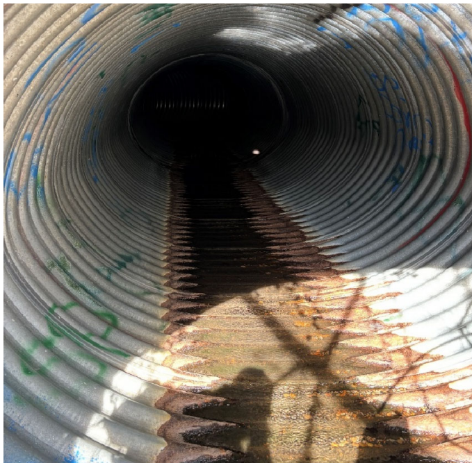
02/08/2024 Inspection – Outfall M05B5O00001 corroded pipe.
