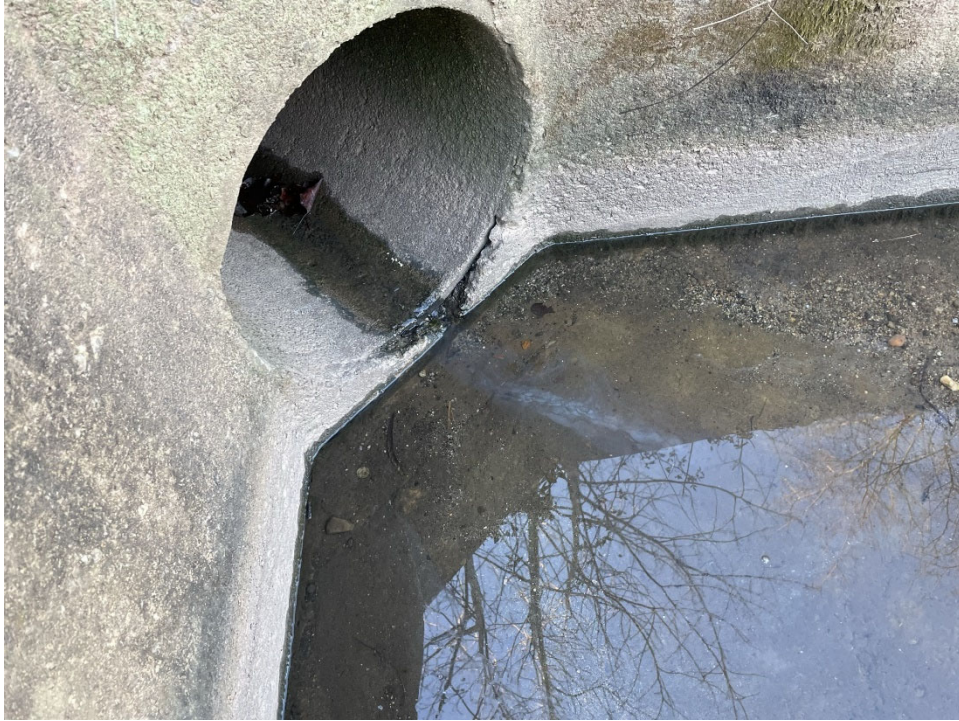
Outfall B11G7O00012 overview.
