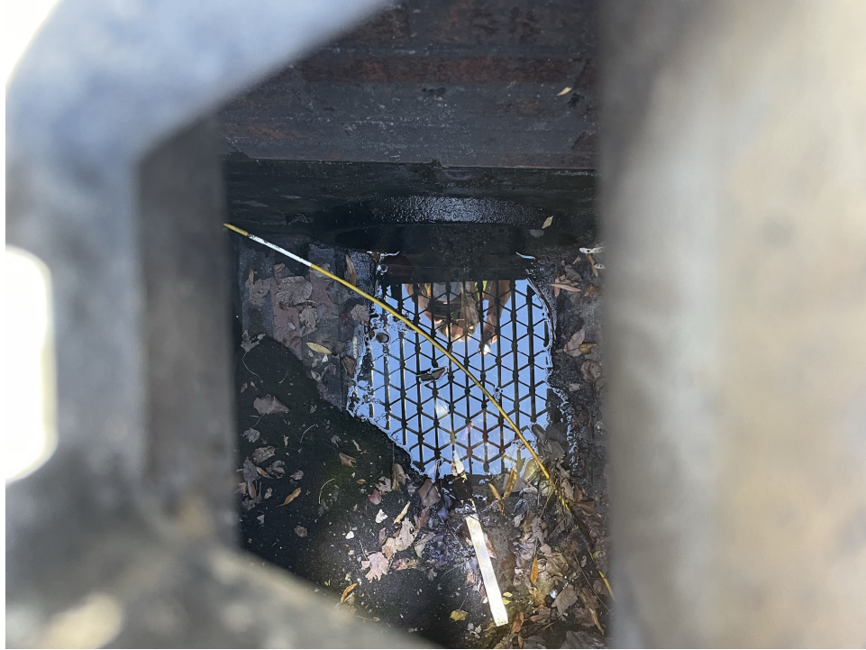
Pooling water at upstream inlet.
