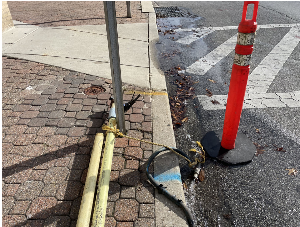
11/30/2023 Inspection – Unattached hose with open valve leak.
