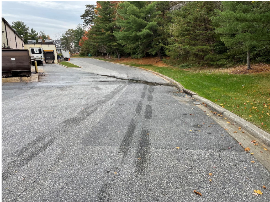
11/7/2023 Inspection – Staining from greasy wash water.
