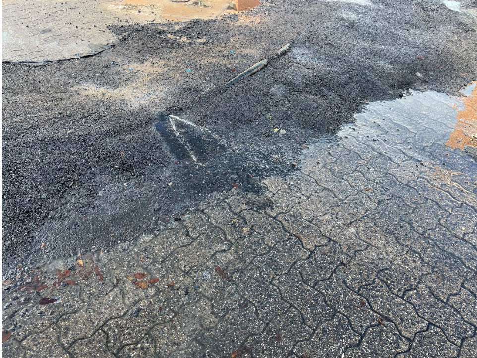
11/30/2023 Inspection – Water line leak.
