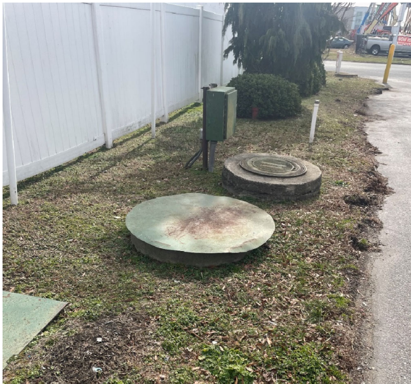
2/8/2024 Re-inspection – Possible water treatment system for soapy water runoff.
