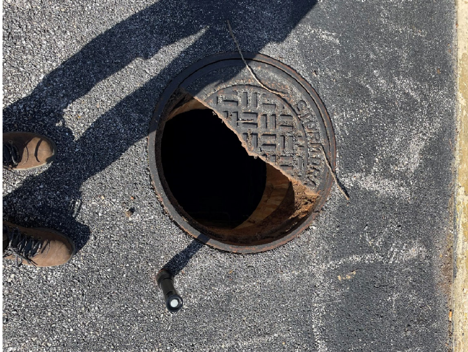
02/09/2024 Inspection – Broken manhole lid.
