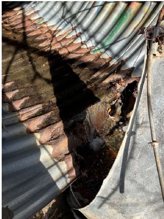
02/08/2024 Inspection – Corrosion on the pipe bottom.
