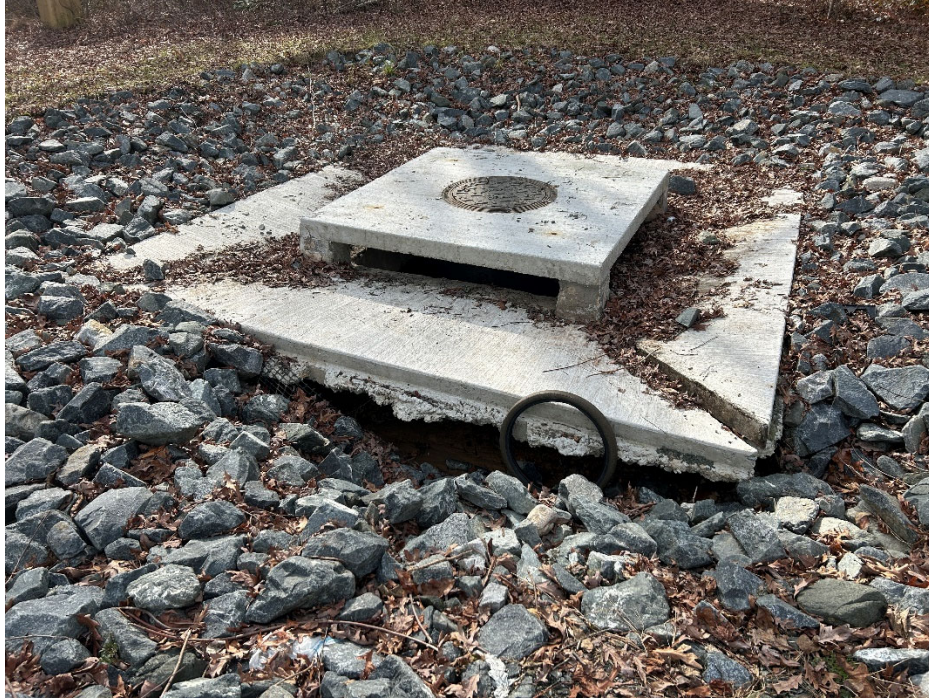
02/08/2024 Inspection – Concrete of first upstream structure being undermined
