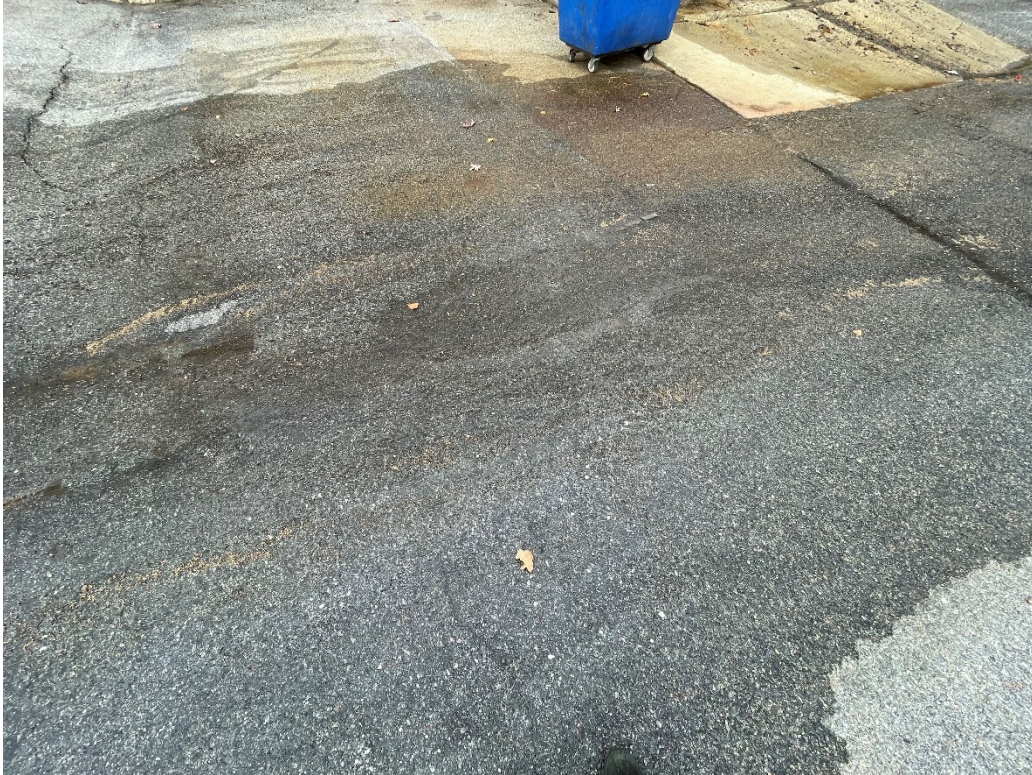
11/7/2023 Inspection – Greasy wash water.
