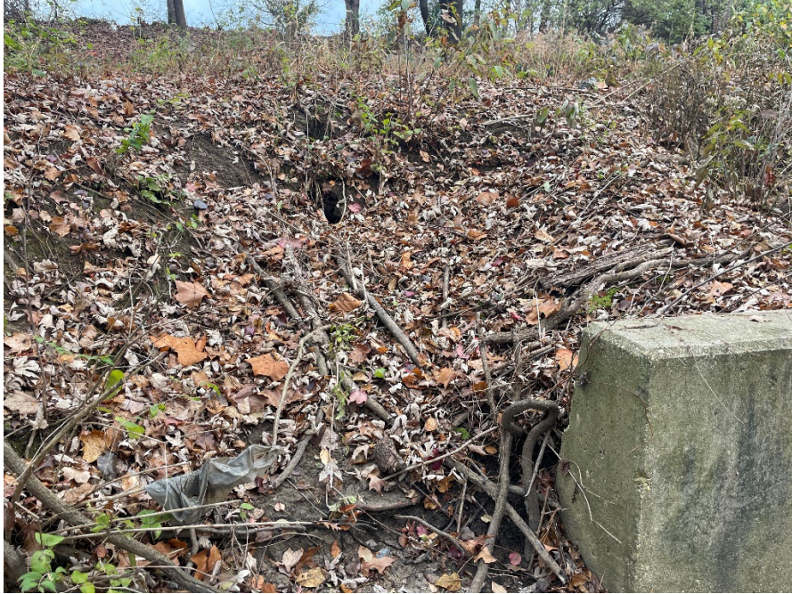
12/01/2023 Inspection – Outfall N04E7O00008 bank erosion above endwall.
