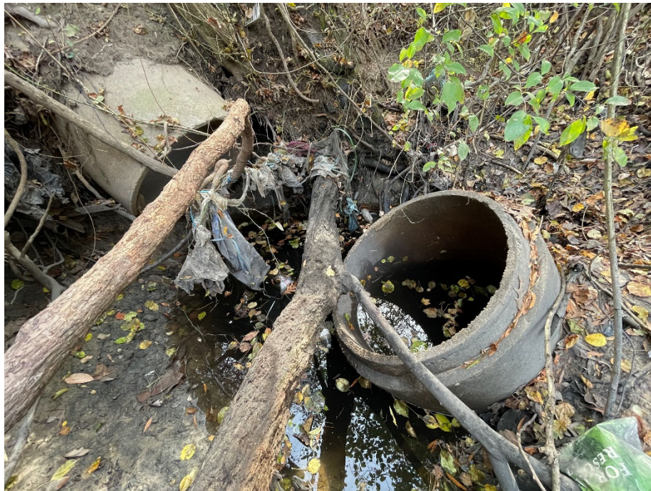
11/15/2023 Inspection – Collapsed sections of pipe.
