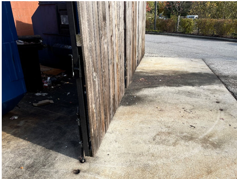
11/6/2023 Inspection – Grease staining on pavement
