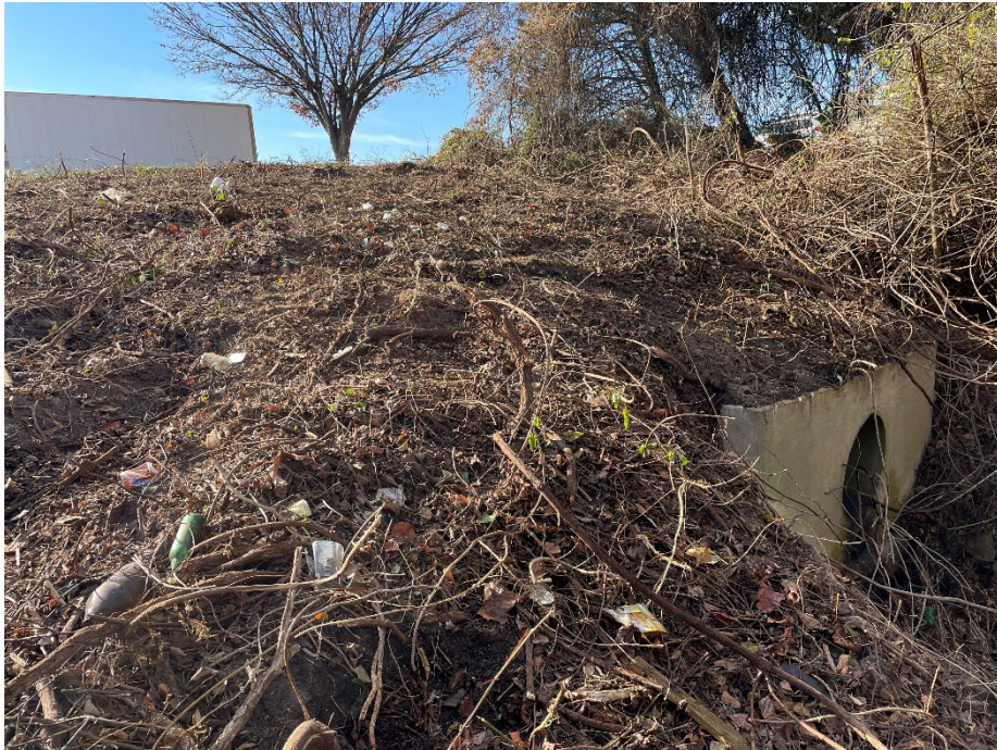
11/30/2023 Inspection – Unstable soil.
