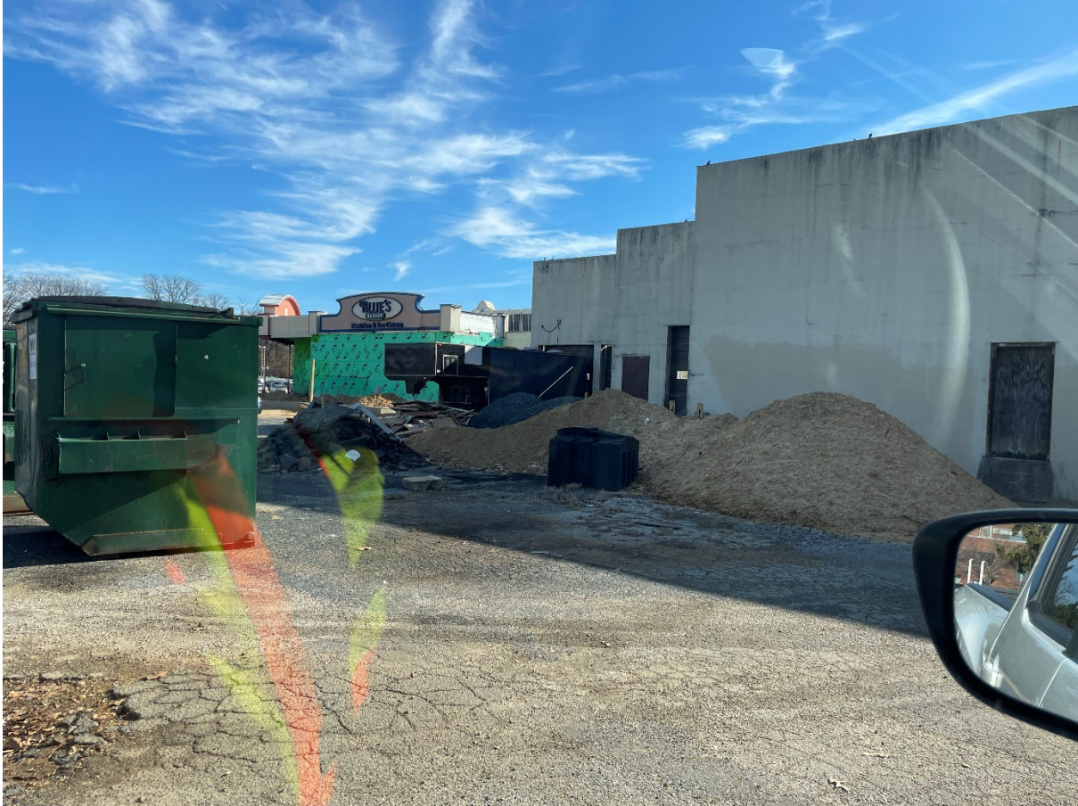
11/30/2023 Inspection – Construction materials in parking lot, no controls in place.
