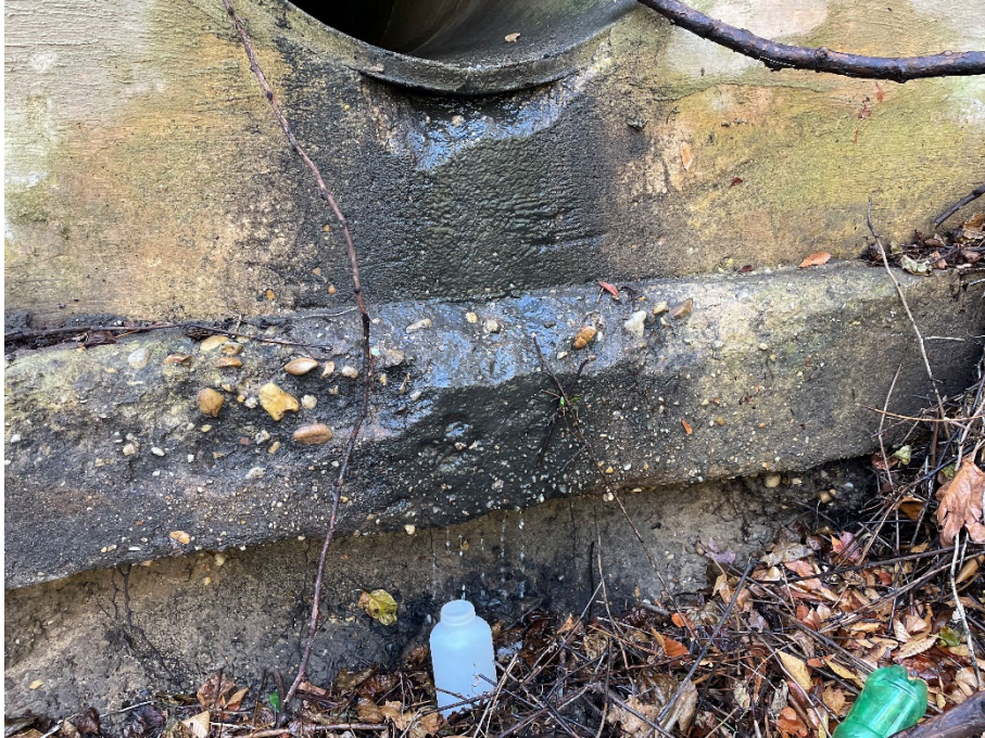
11/30/2023 Inspection – Flow undermining outfall.
