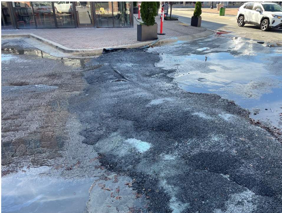
11/30/2023 Inspection – Pooling water with ice melt pellets.
