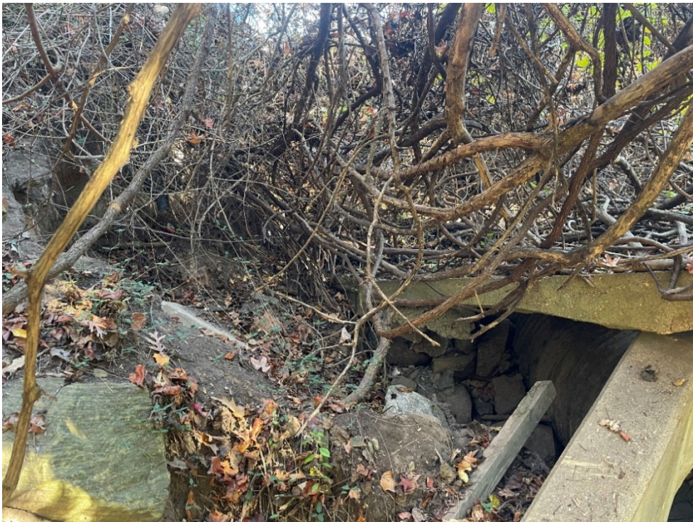
11/16/2023 Inspection – Erosion above the outfall with the exposed pipe and concrete slab.
