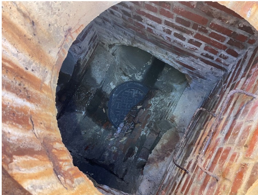
02/09/2024 Inspection – Manhole interior with broken lid.
