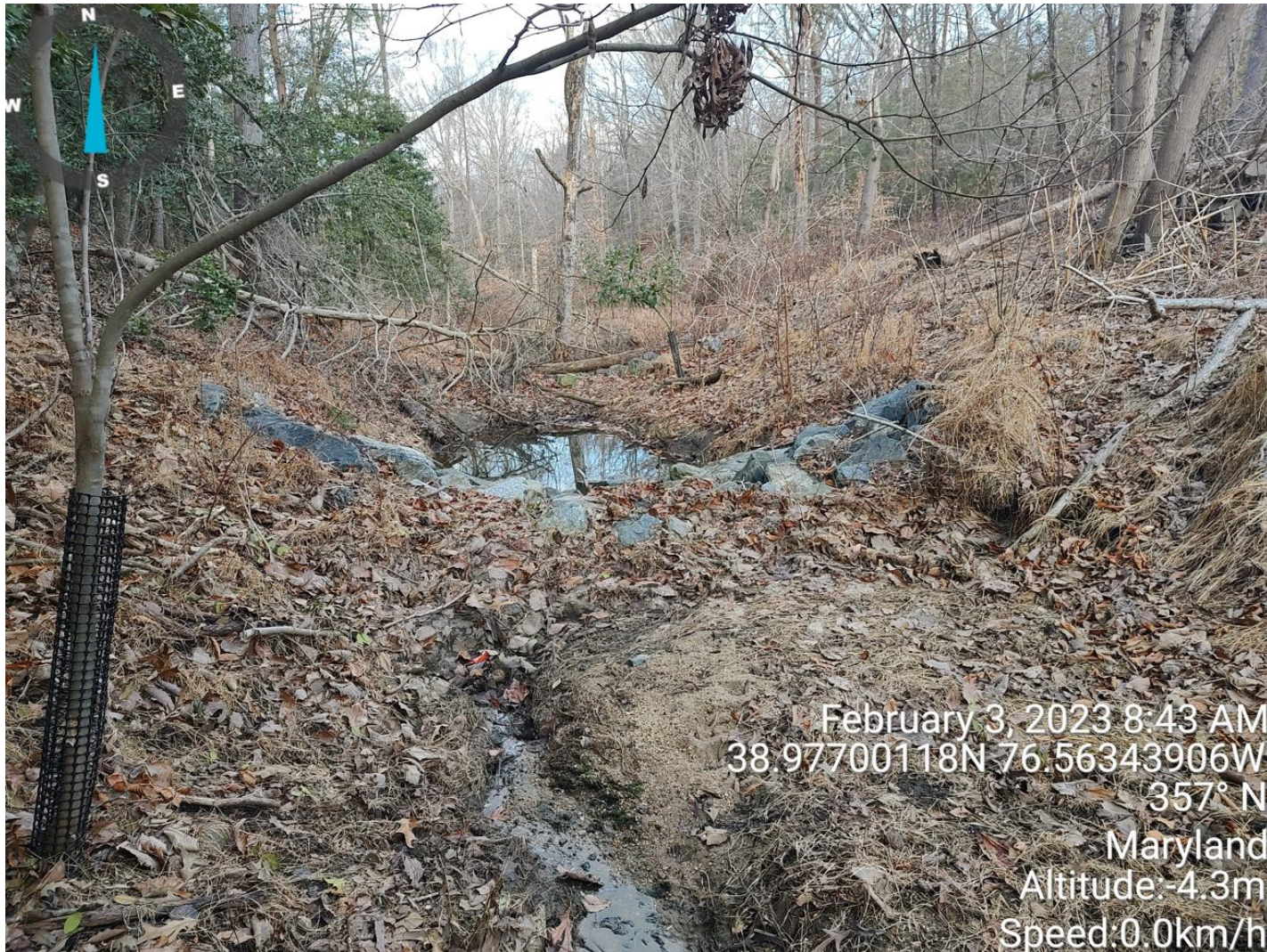
Downstream view of Broad Creek with check dam and step pool show. POI location can be seen in the distance (see map 1)
