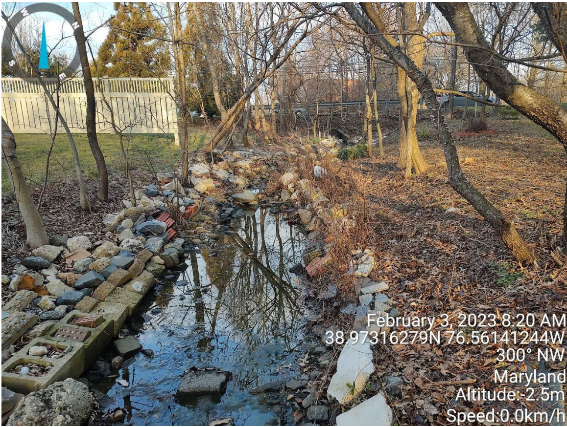
View of the reinforced channel facing the outlet. Area appears stable with no erosion present.
