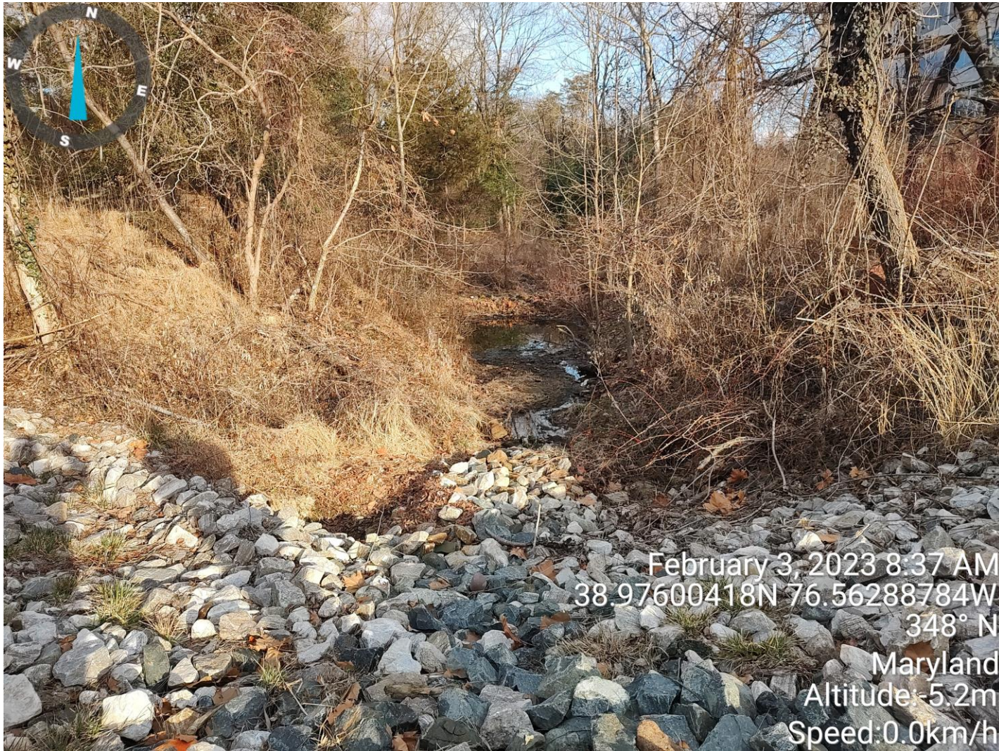
Site outfall (see map 2 and overall site map) discharging from the stormwater basin into Broad Creek
