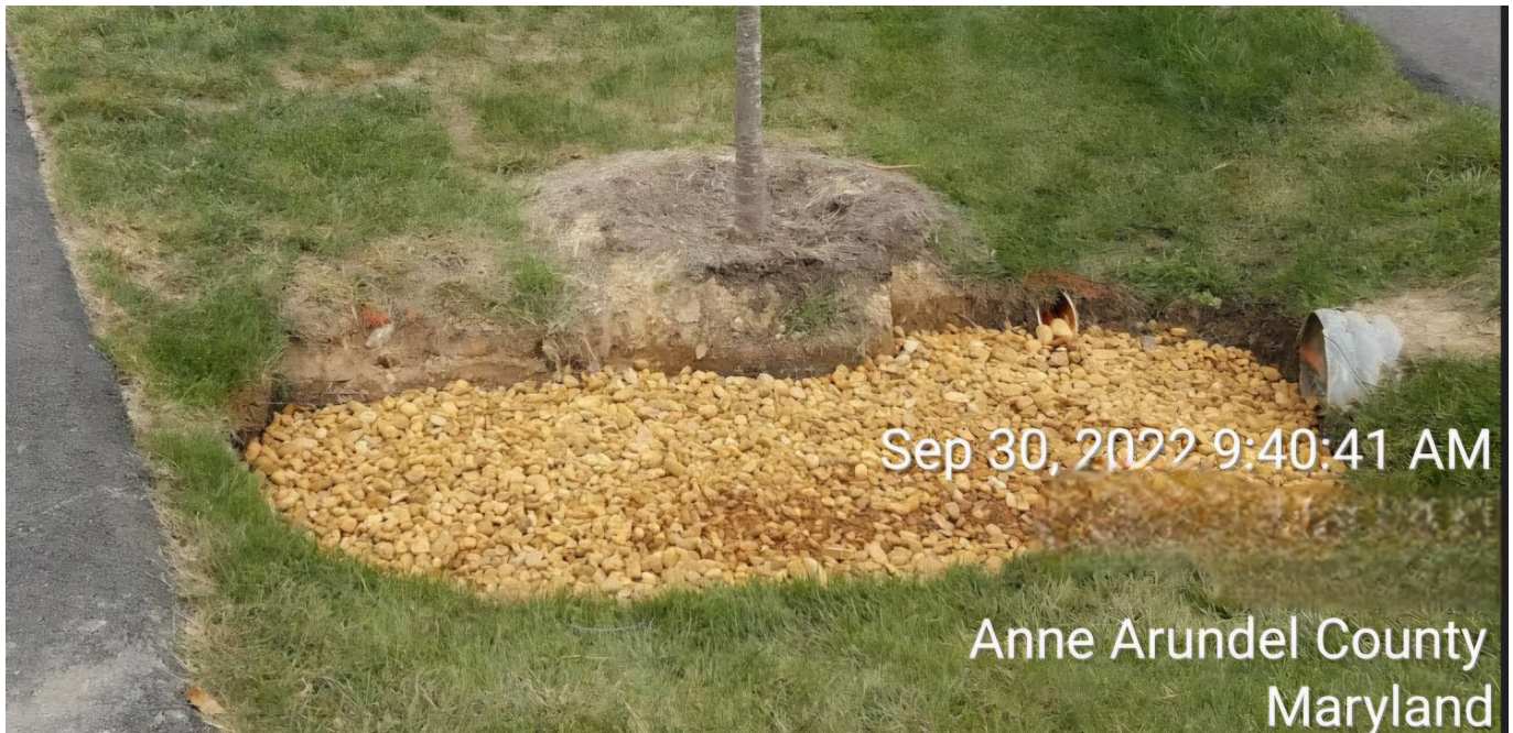
Sump pump discharge into roadside bioswale – design plans did not show details, account for this runoff.
