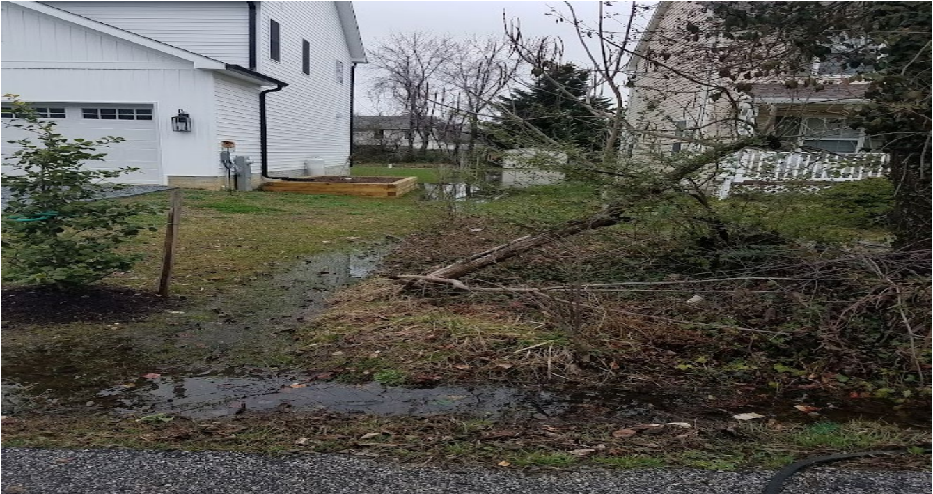
PB#3 installed with no underdrain provided (outfall not feasible due to lack of grade elevation). Note the lack of detail on the plans to show how the runoff would be conveyed from the overflow, onsite and offsite runoff (coming from the existing home on the right).
