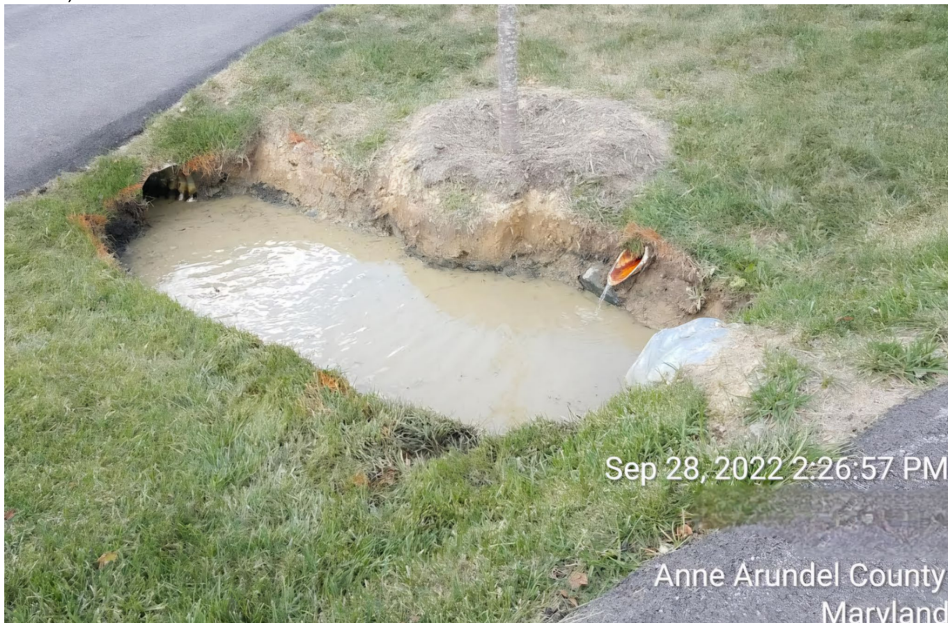
Sump discharges into roadside swale- these were not accounted for as a part of the site design.
