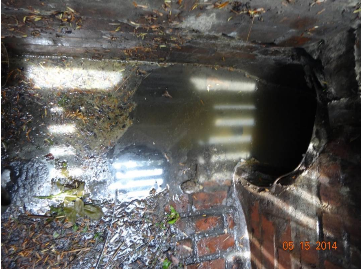
Figure 3. Interior of curb inlet in the loading dock area of Embassy Suites, 1300 Concourse Drive, showing off-color water; detergent concentration was 0.75 mg/l
