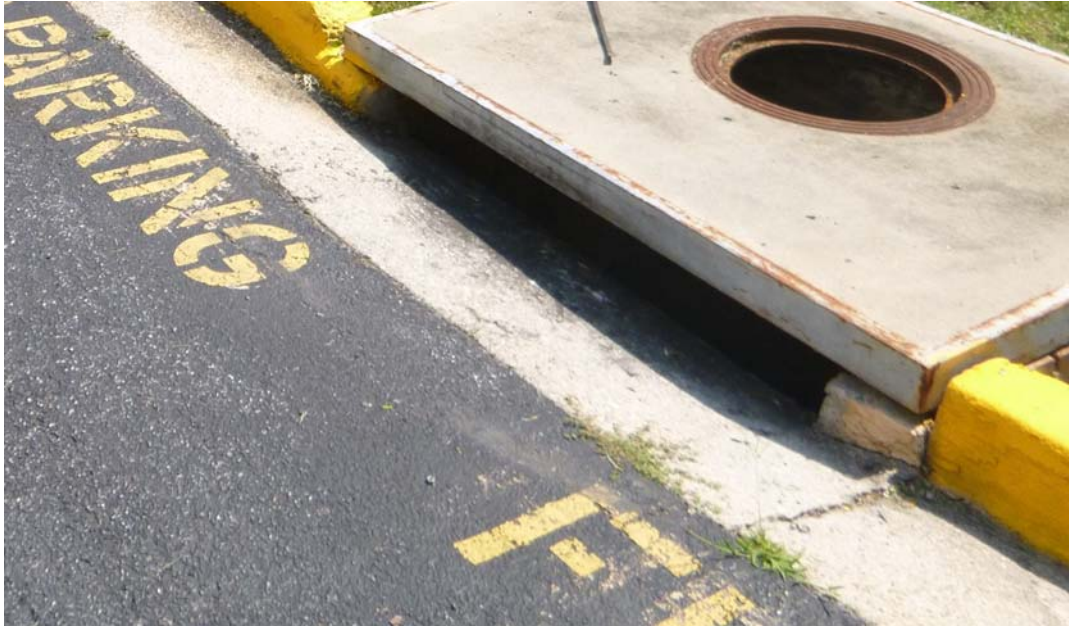
Figure 2. Evidence of a possible separation of the supporting block and a split in the gutter (lower right corner of the photograph)
