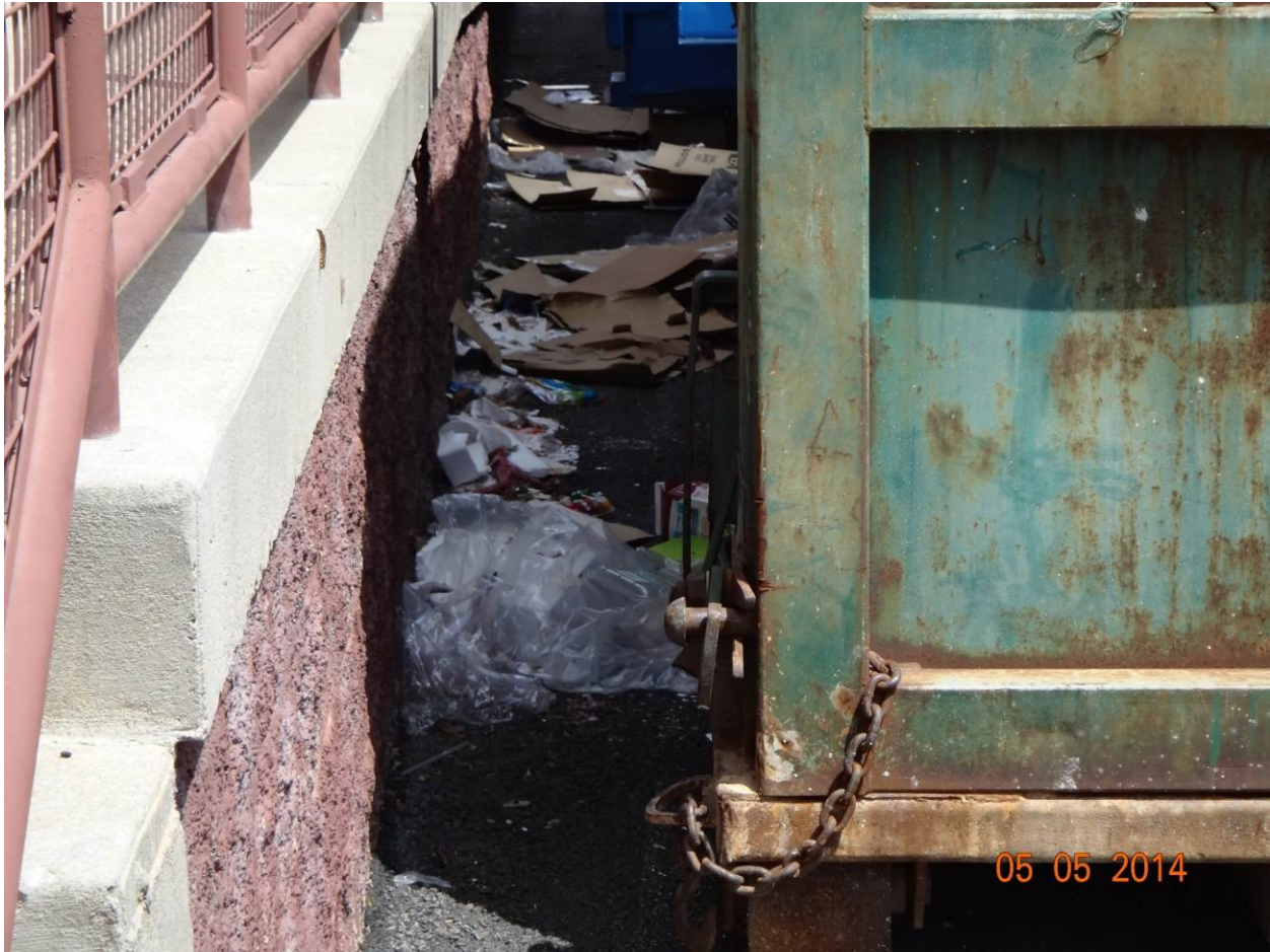
Figure 2. Debris between the roll-off dumpster and the Target building
