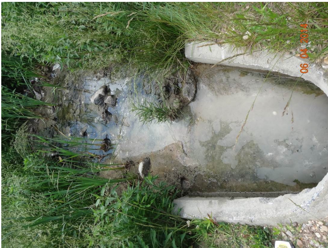
Figure 2. Whitish film on water surface at outfall
