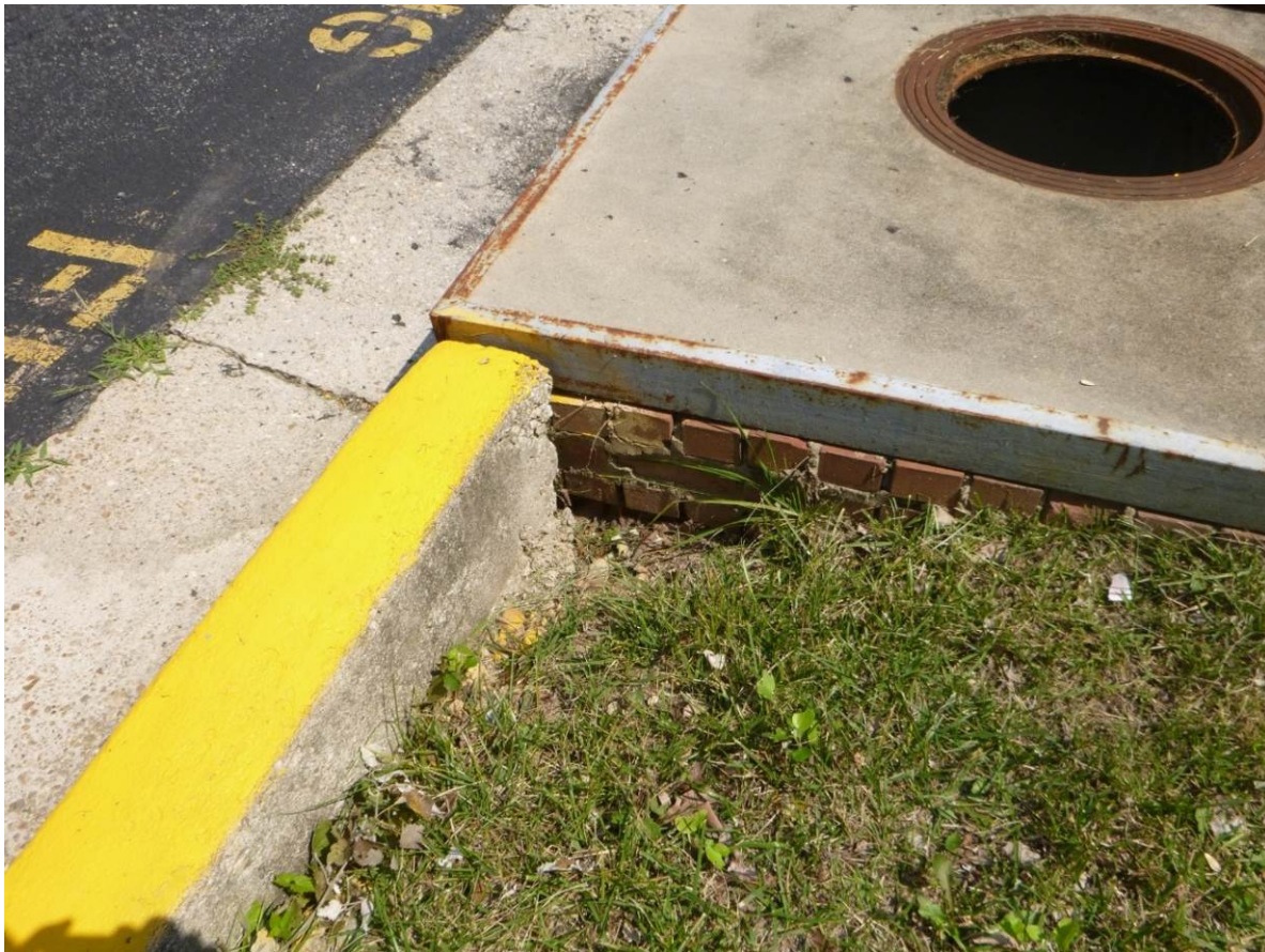
Figure 1. Evidence of ground support missing from the corner of the curb inlet
