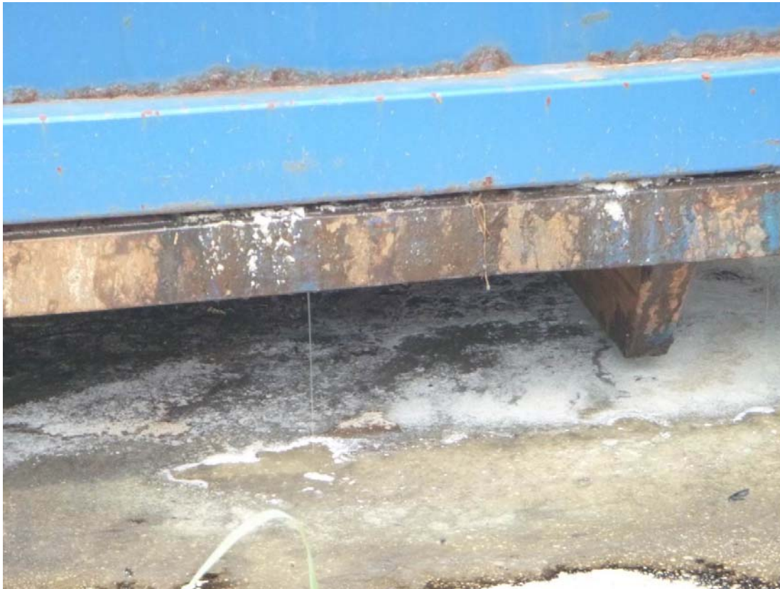
Figure 2. Fluid observed leaking from the dumpster on June 16, 2014
