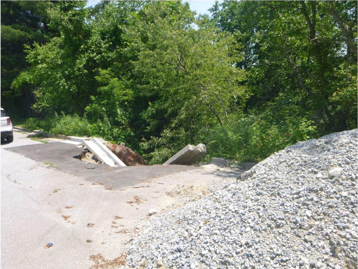
Figure 2. A view of the extent of the collapse and the jutting curb sections
