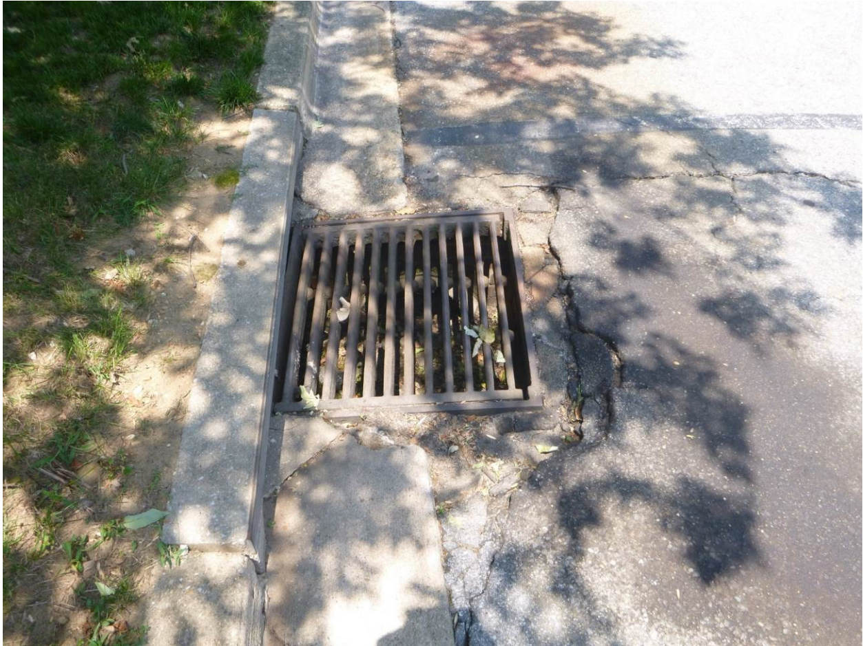
Figure 2. View of the asphalt and gutter damage and partial collapse as seen from the left of the inlet grate
