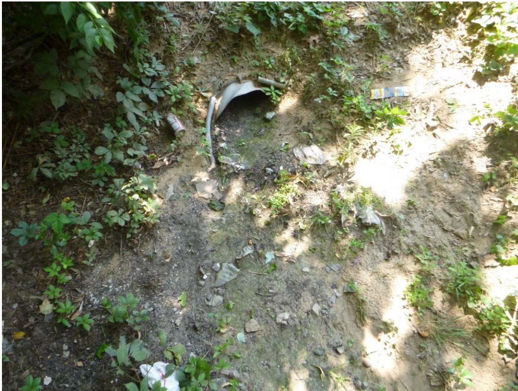
Figure 1. Evidence of sediment accumulation in and around the pipe outlet draining the Motel 6 parking lot; there is algae growth extending downstream of the pipe opening
