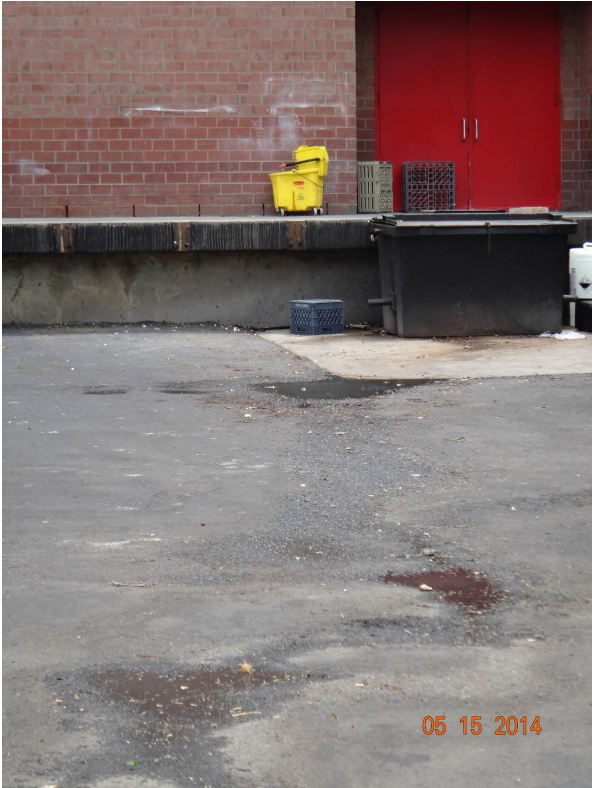
Figure 6. Loading dock area showing mop pail and puddles of water
