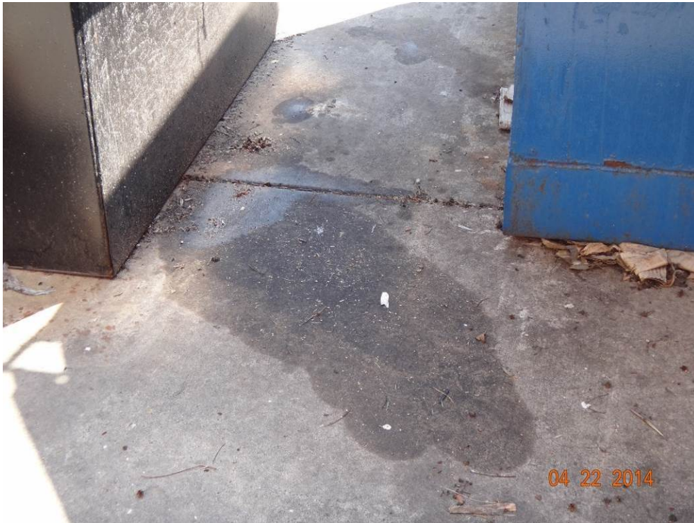
Figure 2. Detail of a grease spill near the waste grease container
