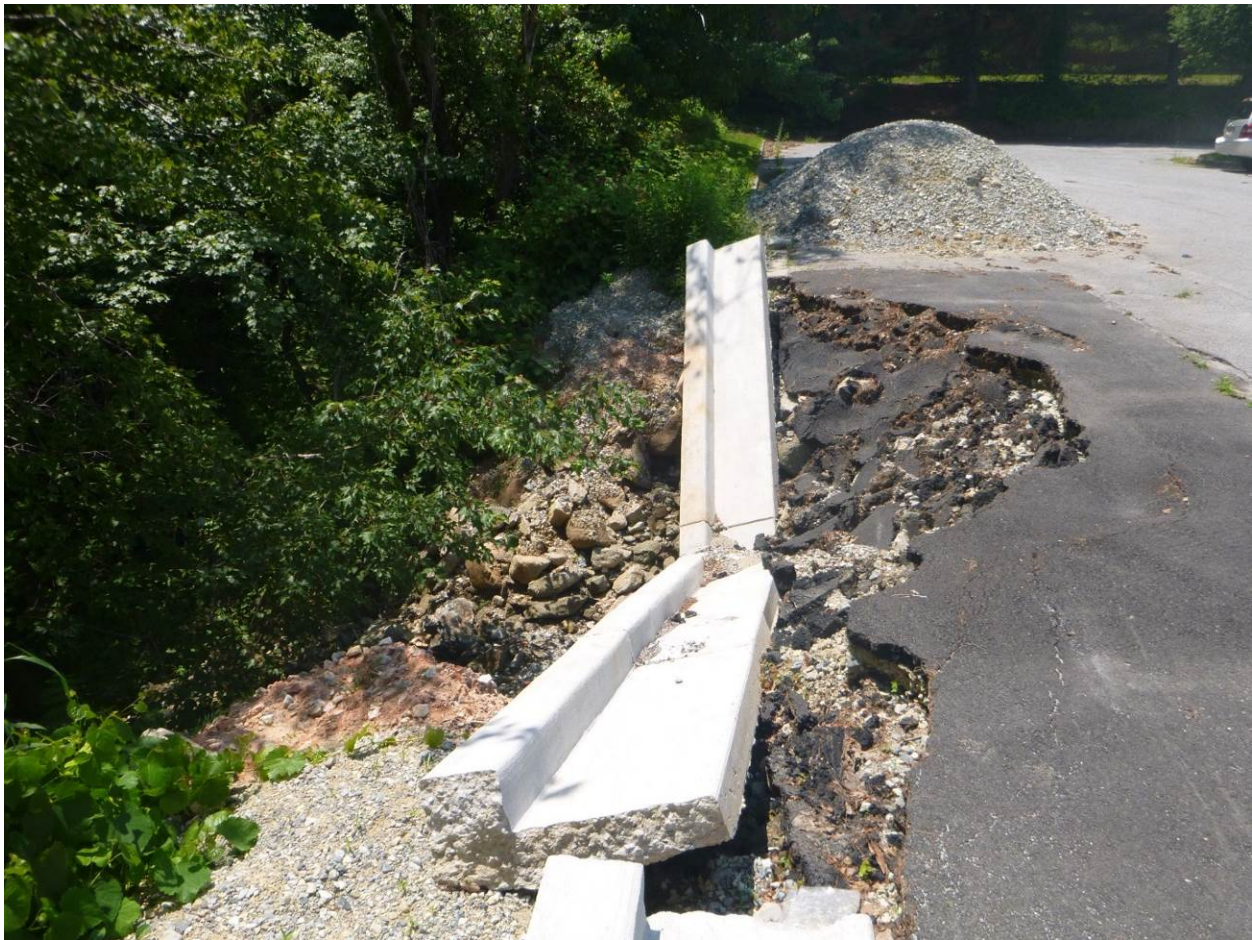
Figure 1. A section of parking lot pavement that had collapsed and the associated damaged curb
