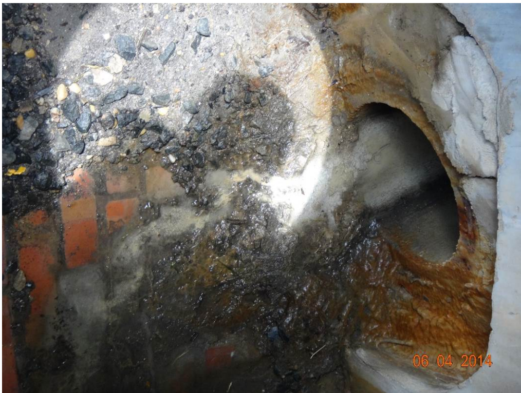
Figure 4. View of inside of first curb inlet showing mineral buildup and whitish residual staining
