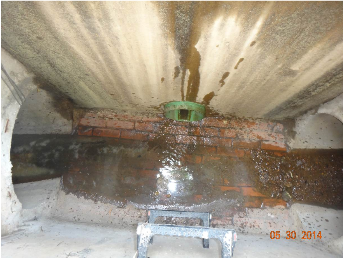
Figure 4. Sanitary sewerage discharging into catch basin (green pipe, center)
