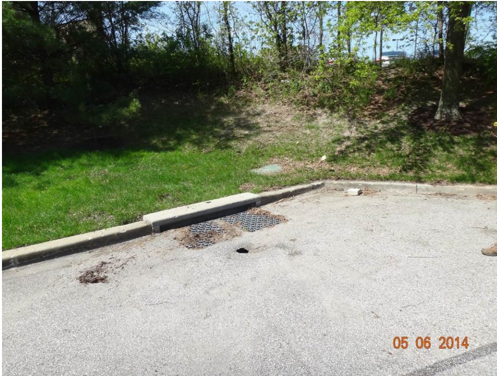
Figure 2. Inlet with nearby hole in asphalt
