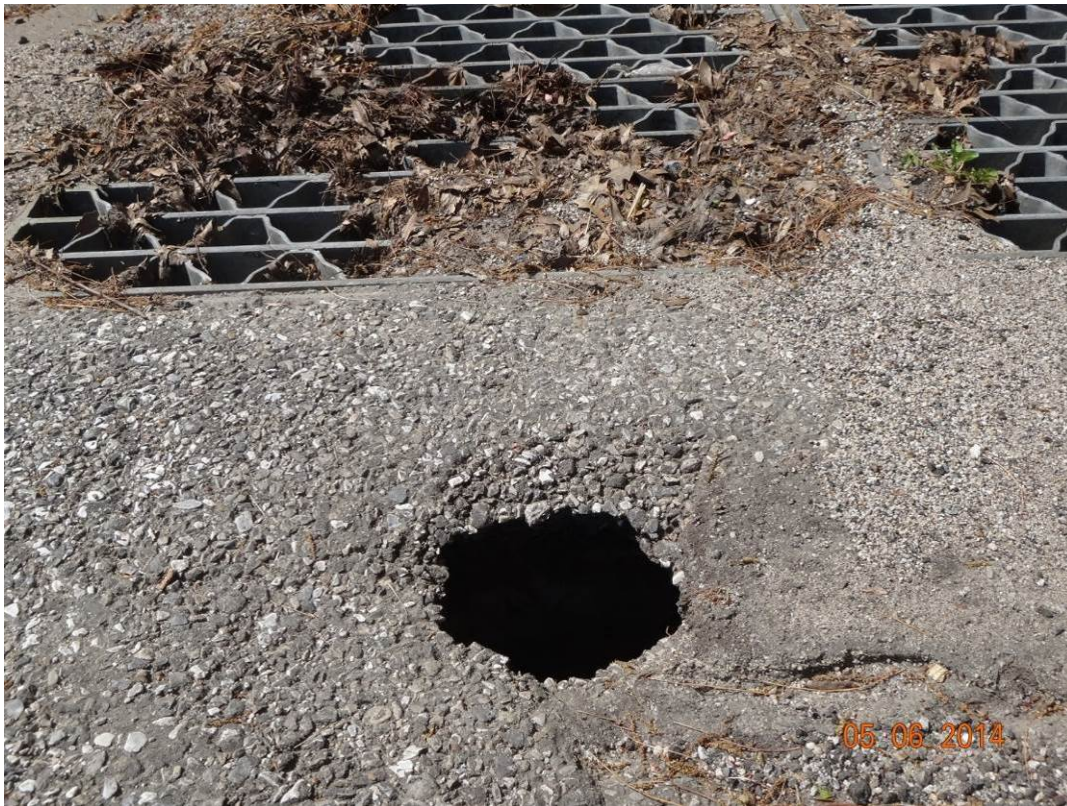
Figure 1. Hole in asphalt near grated inlet, 510 McCormick Drive
