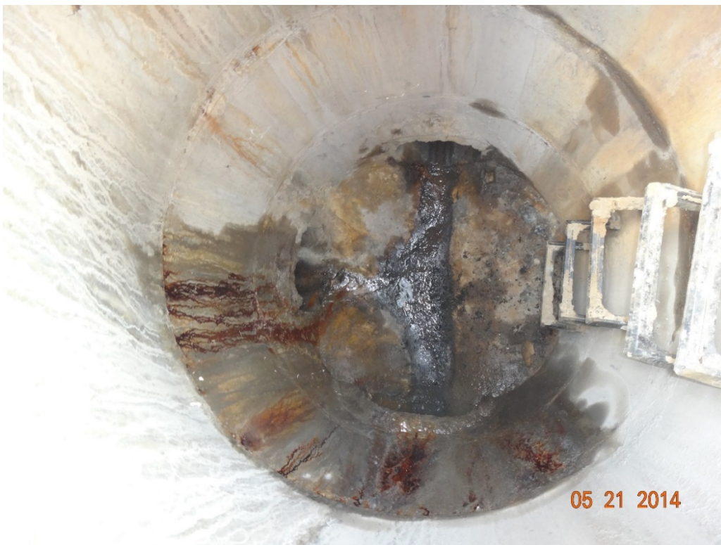
Figure 3. Interior of a junction manhole near the car wash showing moisture but no flow entering from the side pipe
