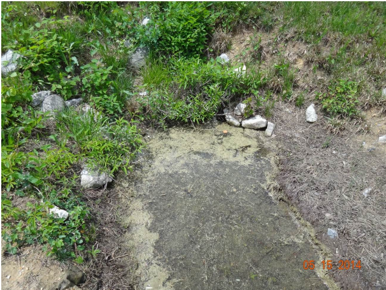
Figure 1. Evidence of a storm infrastructure outfall blocked by sediment
