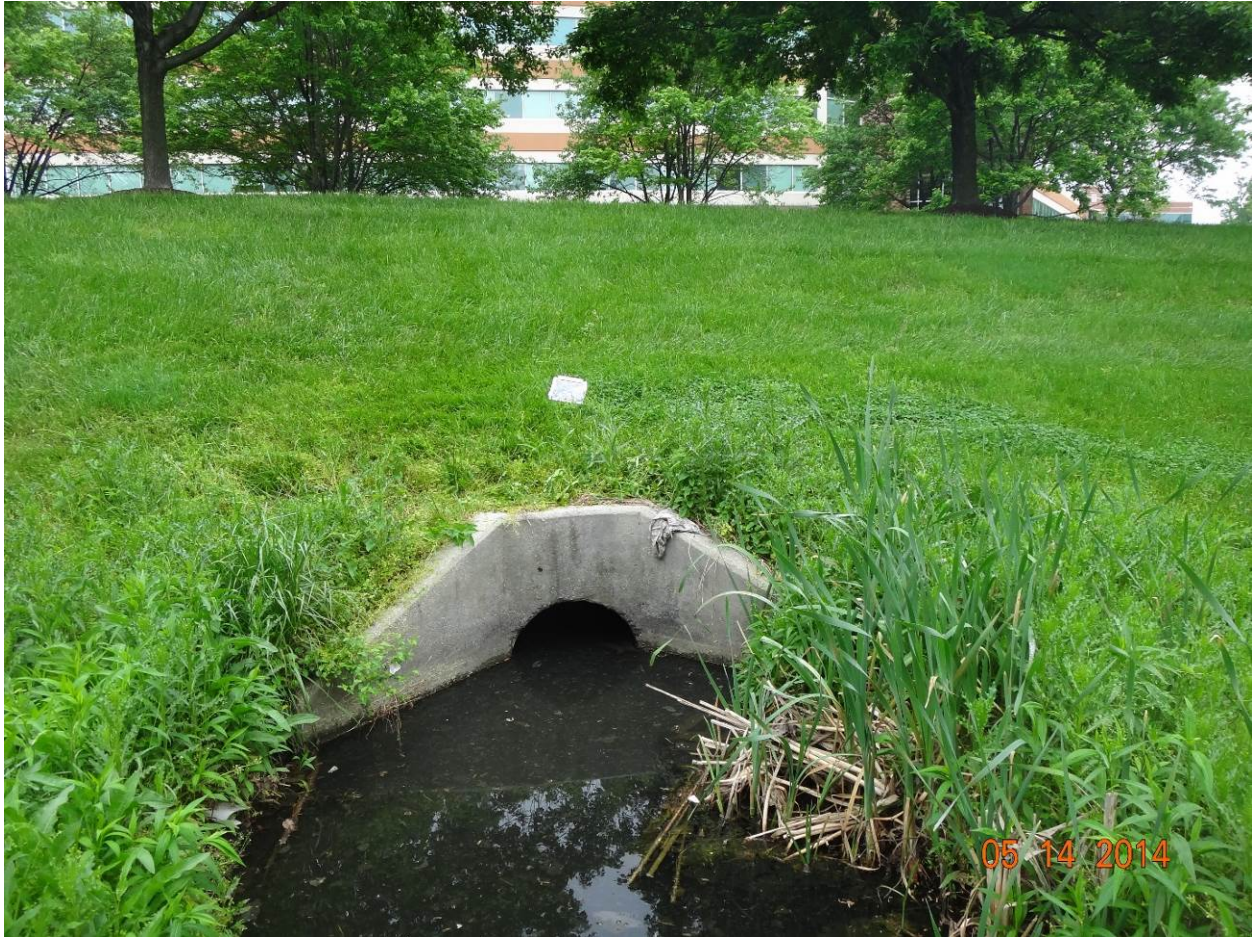
Figure 1. Outfall I03E8O015 with standing water in the orifice
