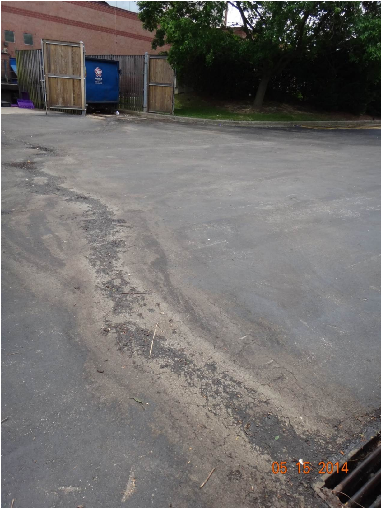
Figure 4. Stains leading from the loading dock area to the curb inlet, behind Embassy Suites, 1300 Concourse Drive
