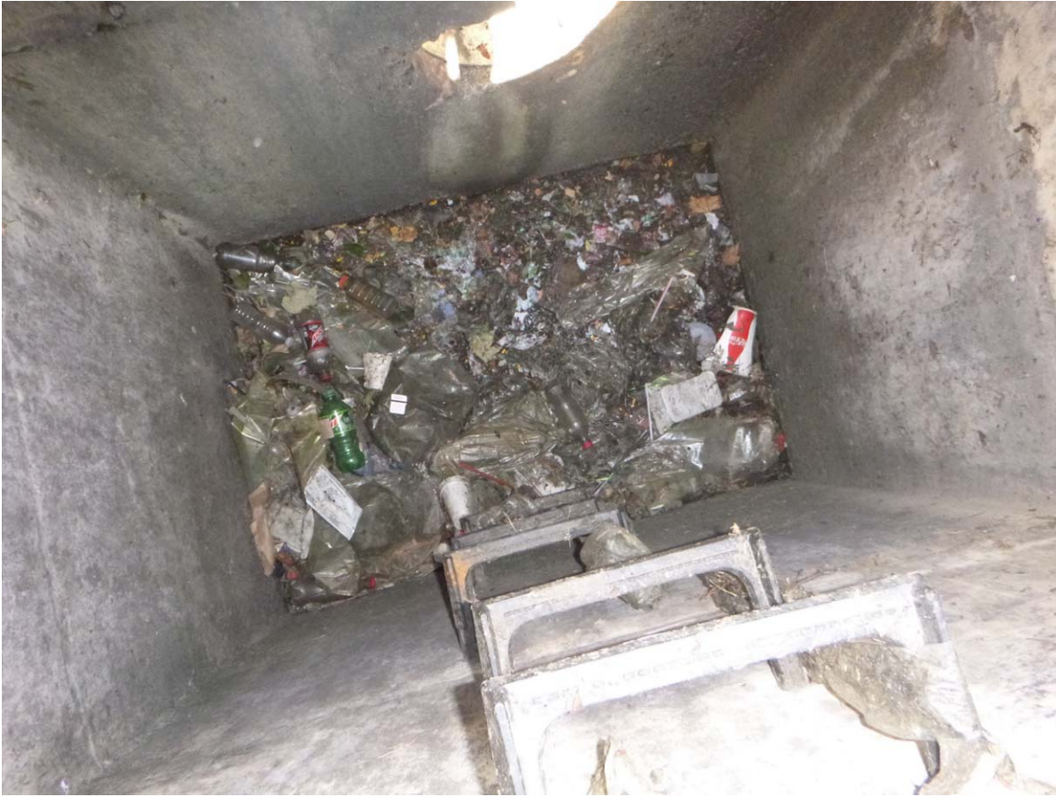
Figure 2. Foul-smelling debris observed within the curb inlet
