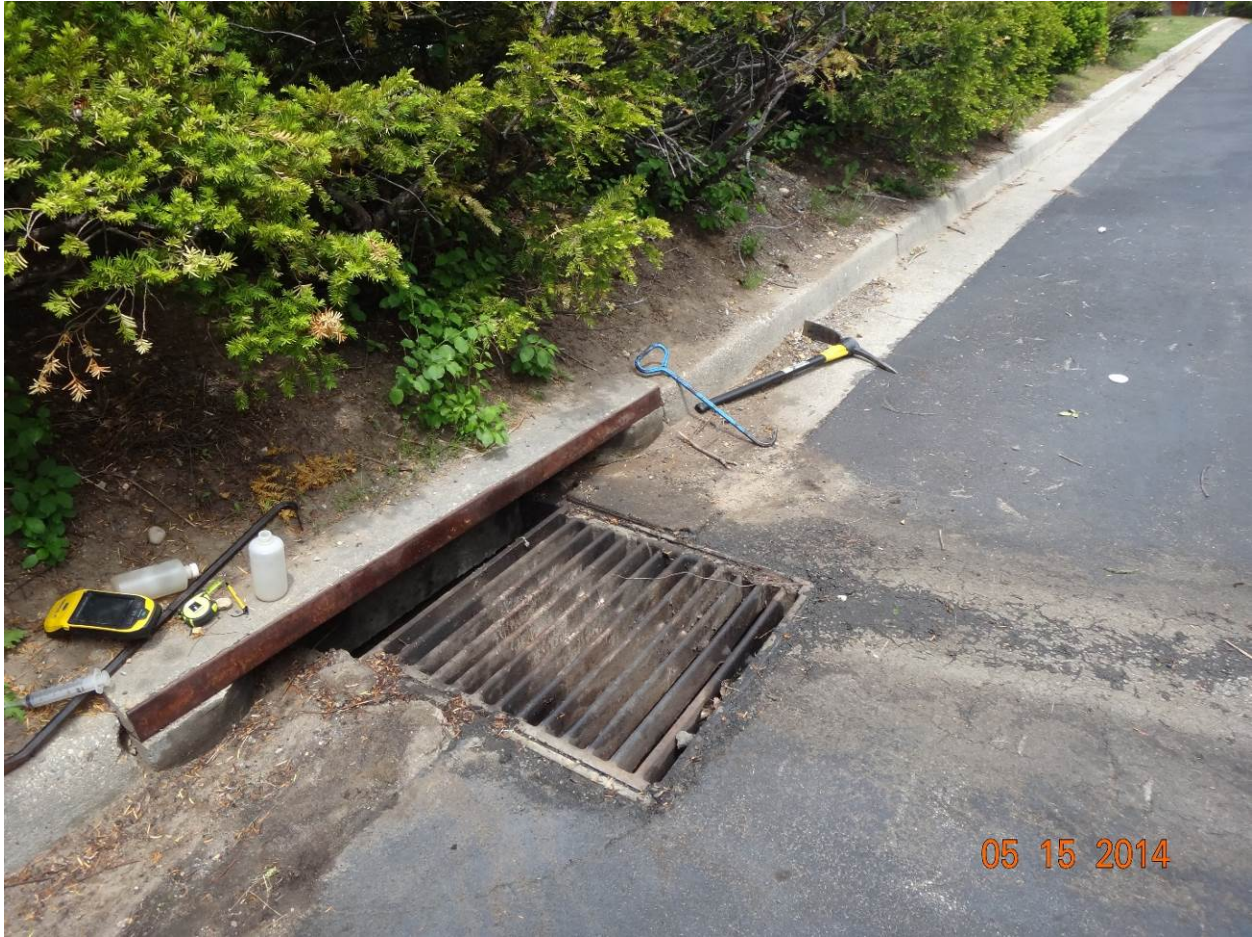
Figure 2. Curb inlet in the loading dock area of Embassy Suites, 1300 Concourse Drive
