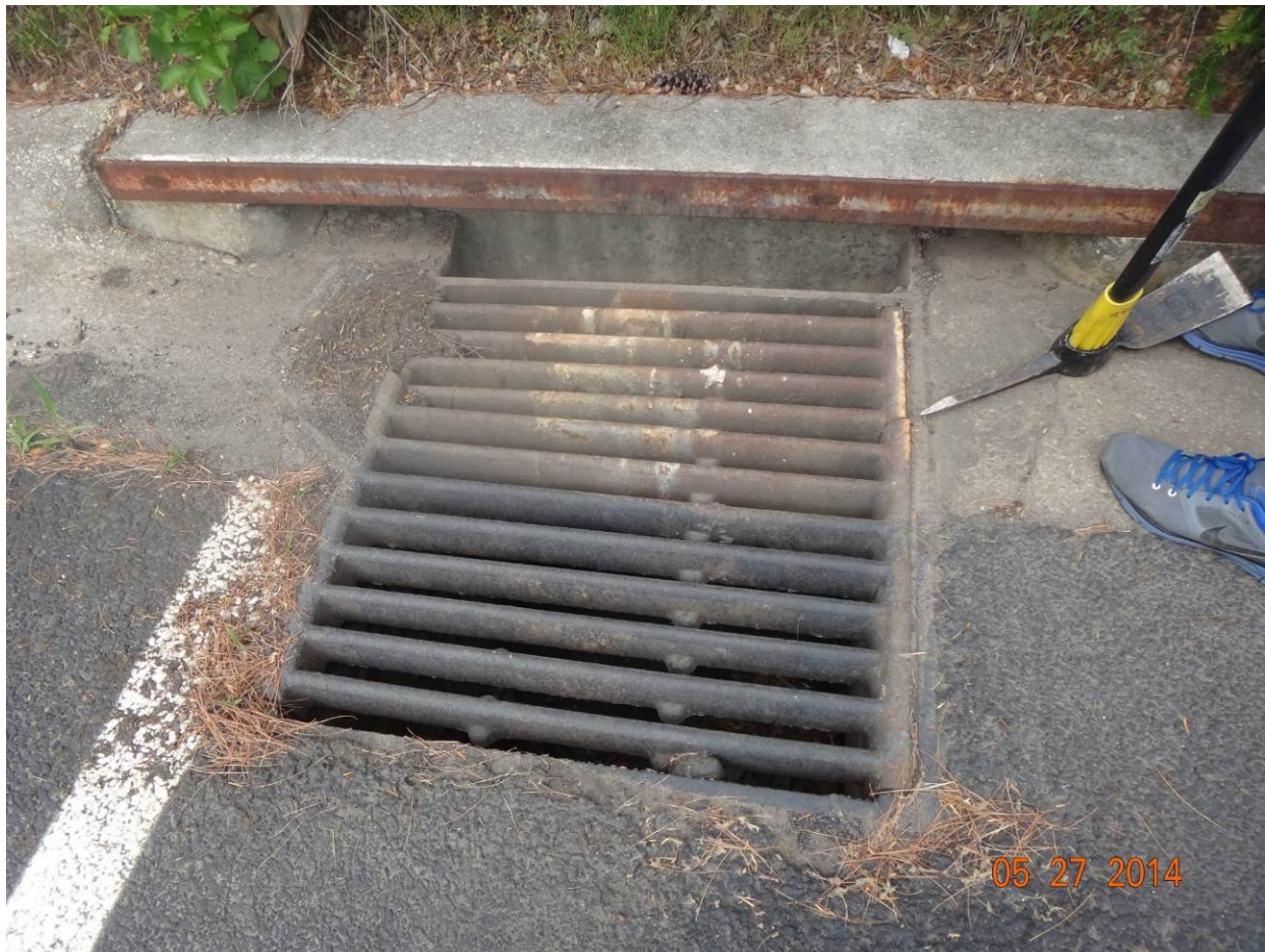
Figure 1. Cracked inlet grate, indicated by pointed end of the pick axe, 1300 Concourse Drive
