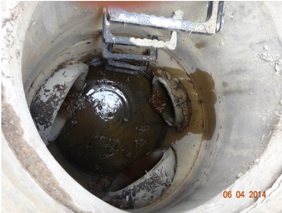
Figure 3. Inside of manhole upstream of outfall; the pipe on the left flows toward the outfall; the smaller pipe on the top right seen flowing and with depositional buildup is the probable source of the high pH levels
