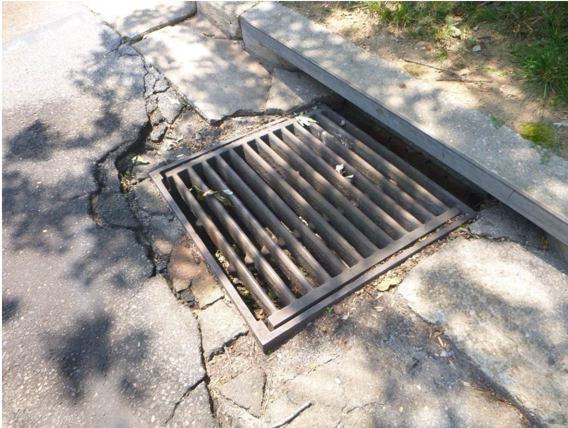
Figure 1. View of the asphalt and gutter damage and partial collapse as seen from the right of the inlet grate
