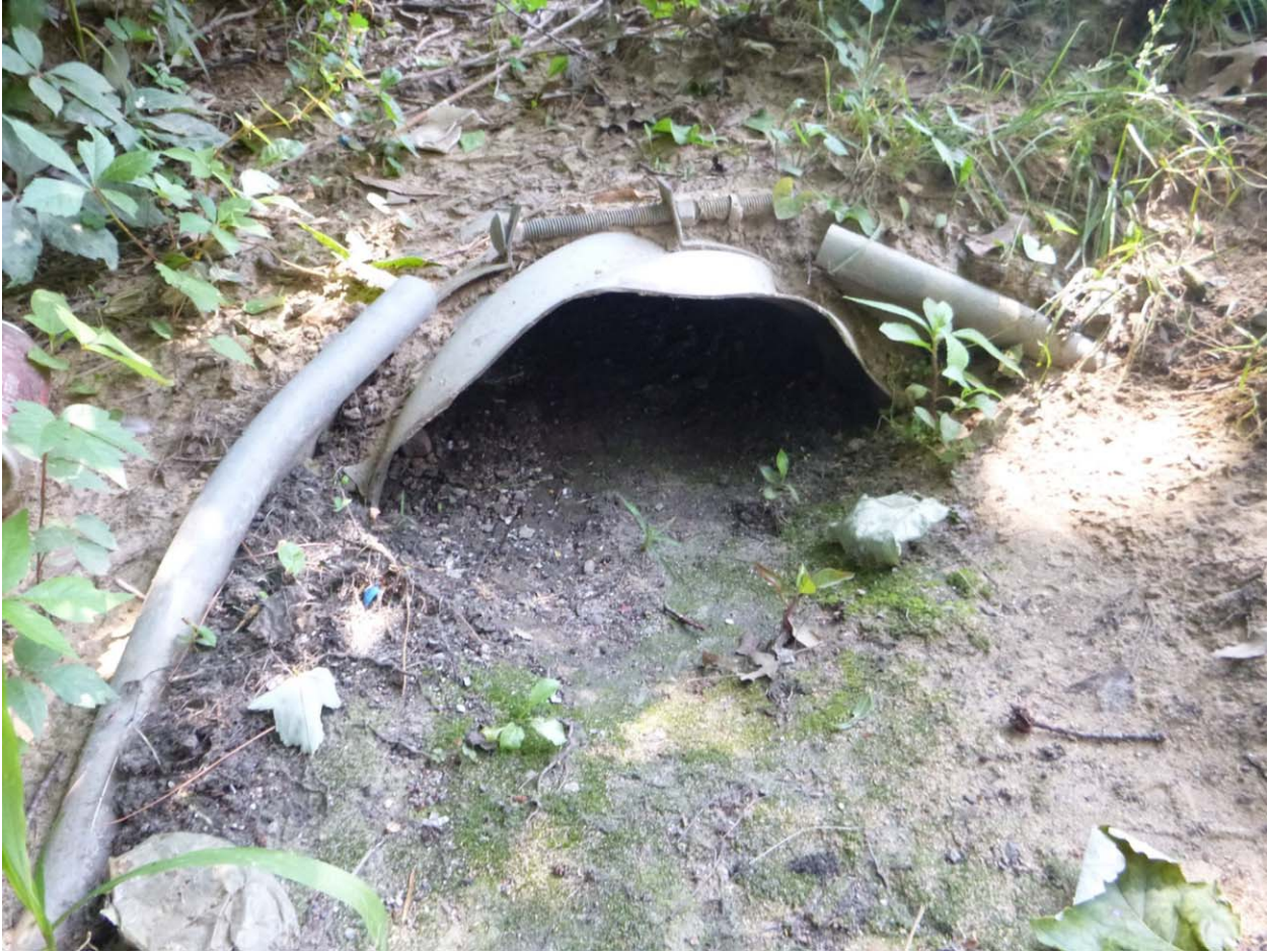
Figure 2. Close-up view of the pipe opening showing the level of accumulated sediment; the interior of the pipe is also occluded with sediment
