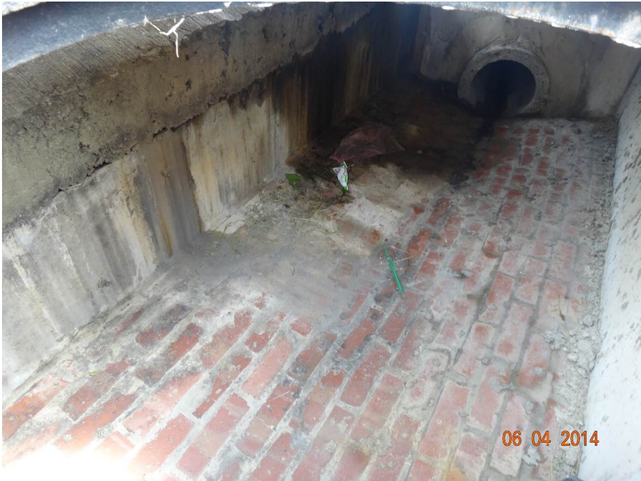
Figure 5. View inside second curb inlet; seepage and staining can be seen originating from a gap in the concrete on the left wall
