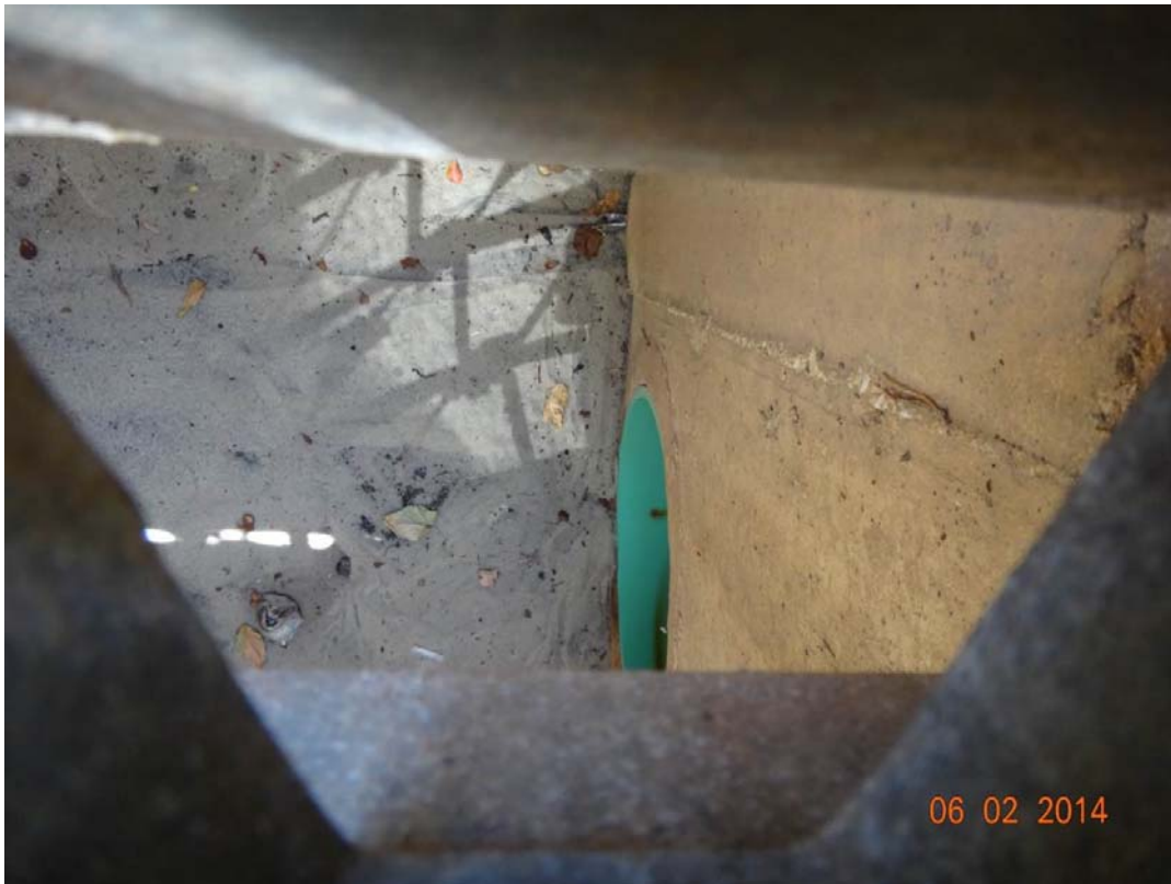
Figure 3. Sand observed in the storm drain at the corner of the parking lot
