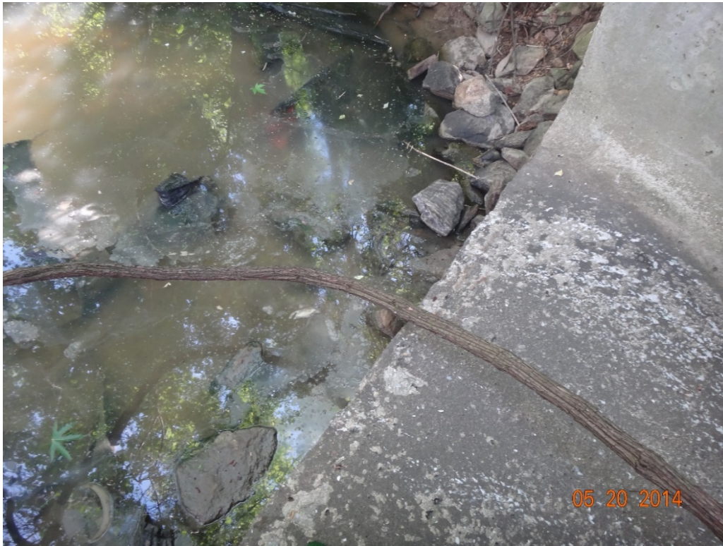
Figure 2. Close-up of Outfall J04C1O018 showing the paper-like material on the apron
