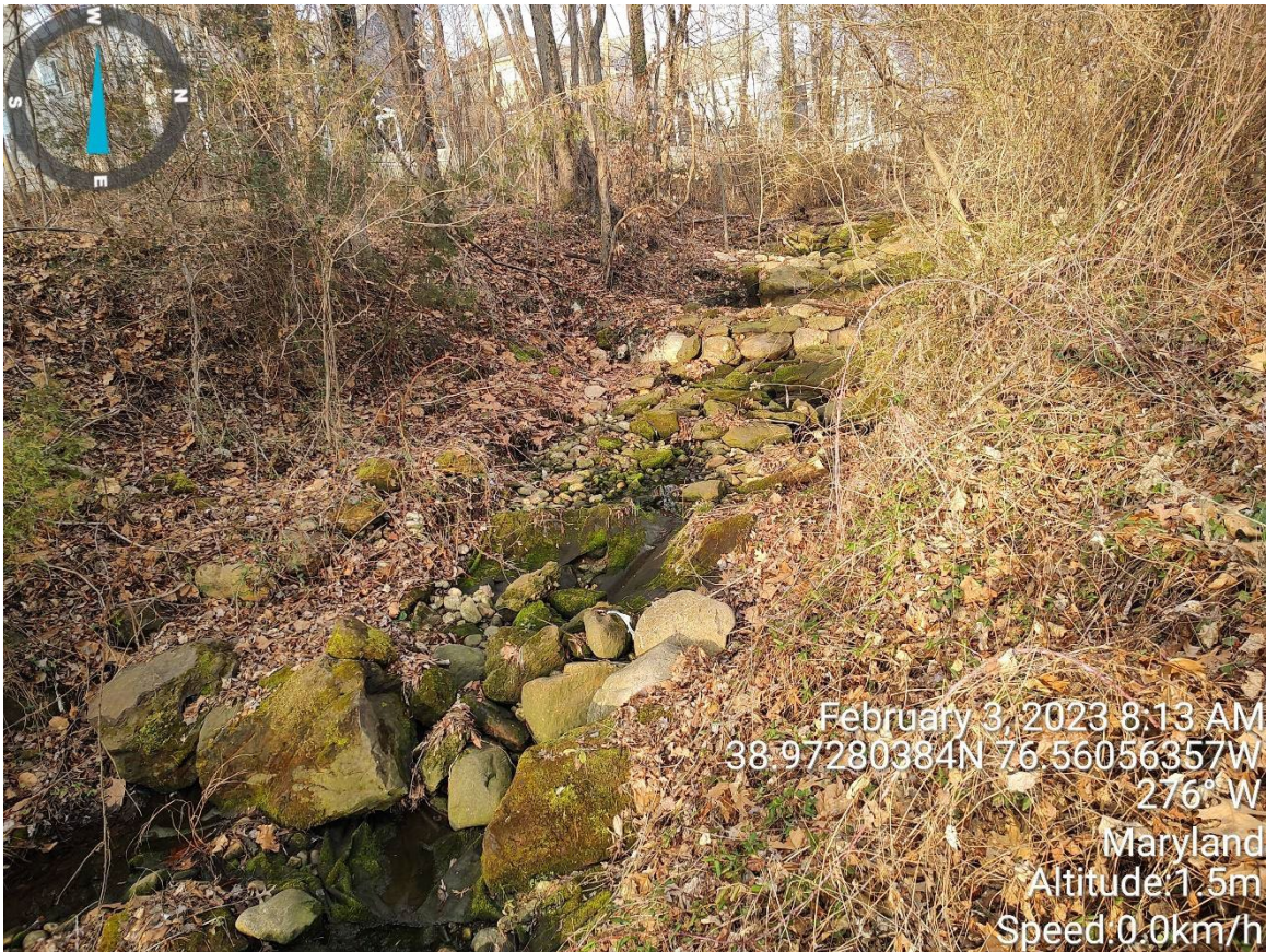
View of the stable channel facing west. Area appears stable with no signs of erosion.
