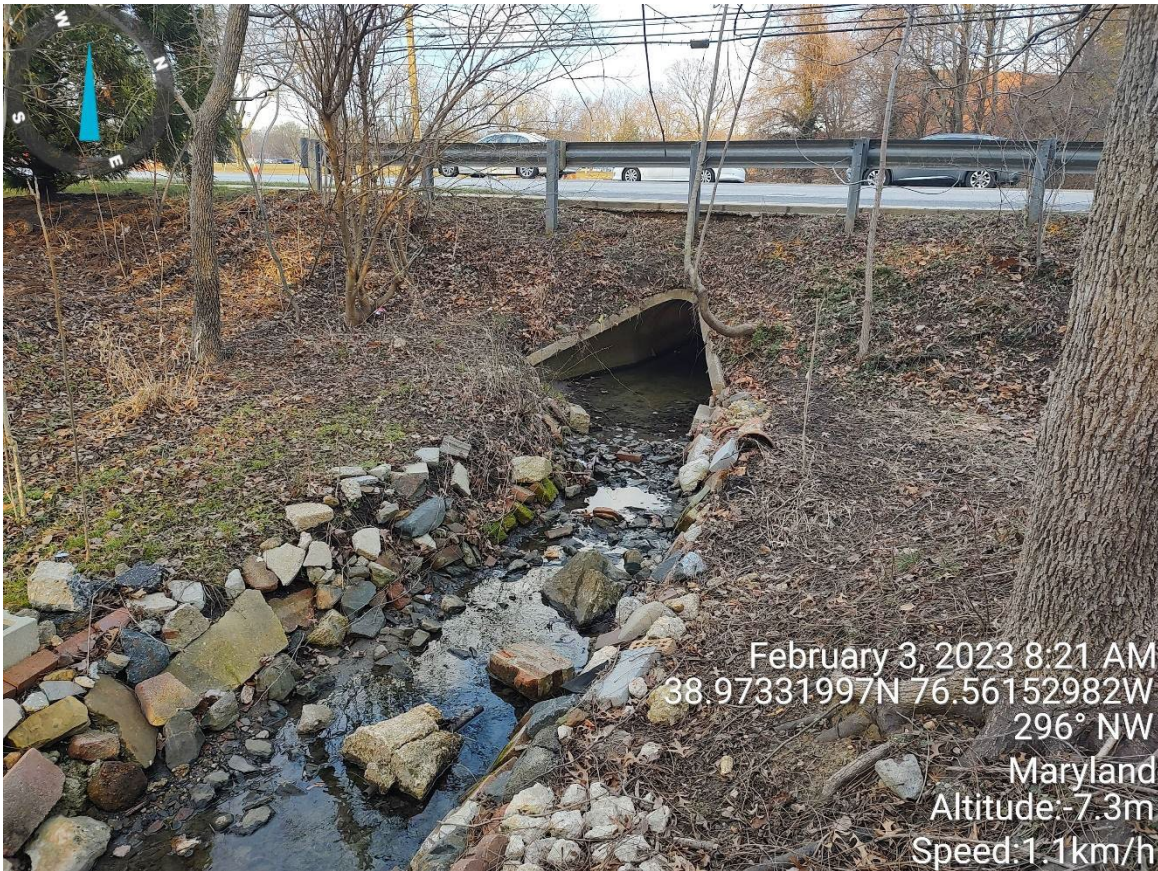
View of the Discharge Point 1, a 48" storm drain, an outlet, and rip rap to the south of Riva Road. Displaced rip rap is present. The area appears to be stable with no erosion present.
