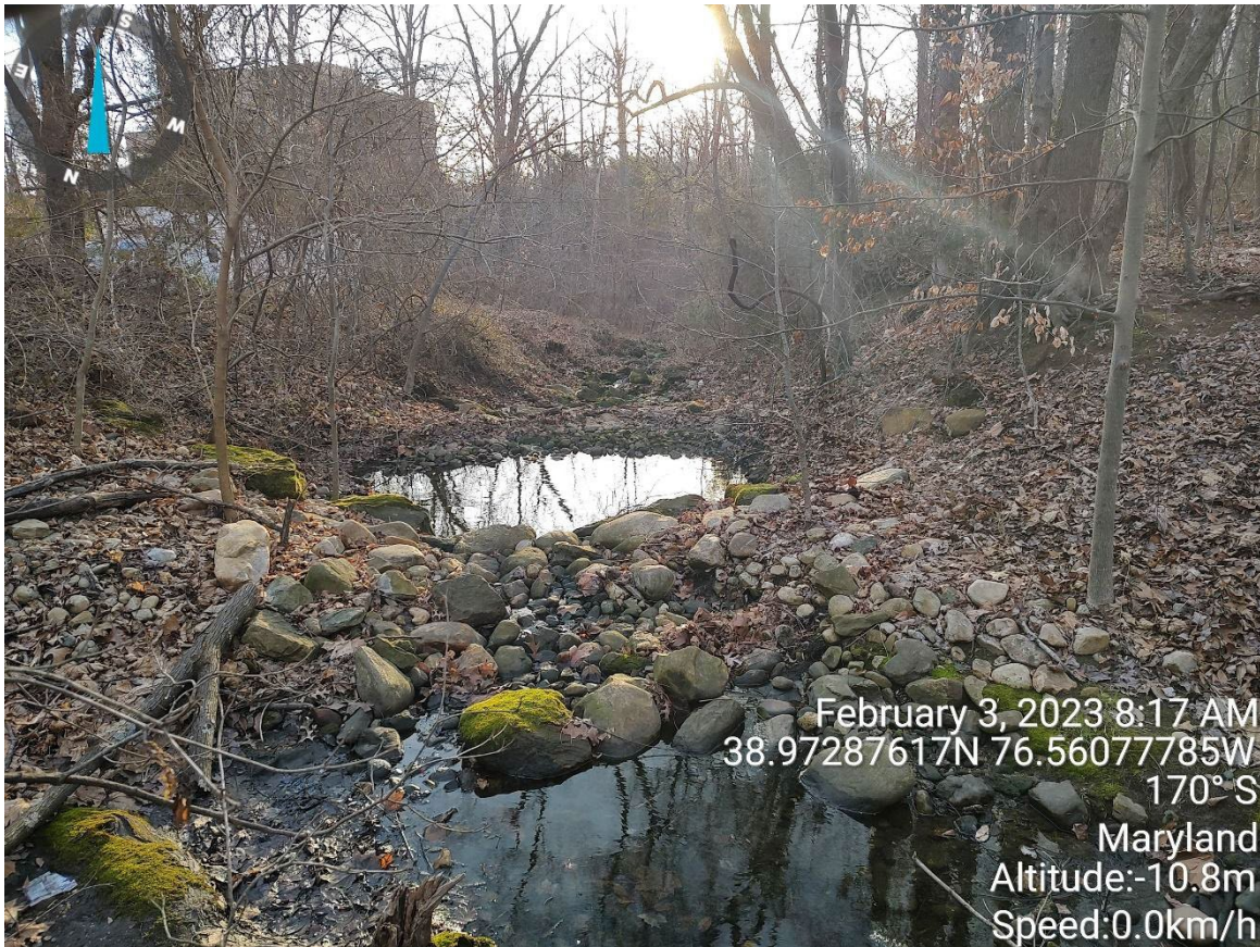
Step pool conveyance facing south along the channel. Area appears stable with no signs of erosion.
