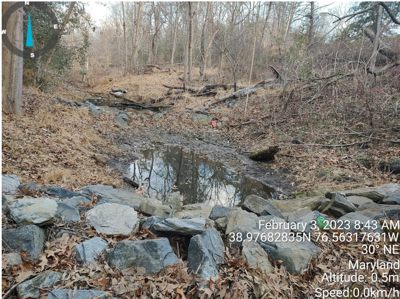
Downstream View of Broad Creek; Check dam and step pool can be seen in picture
