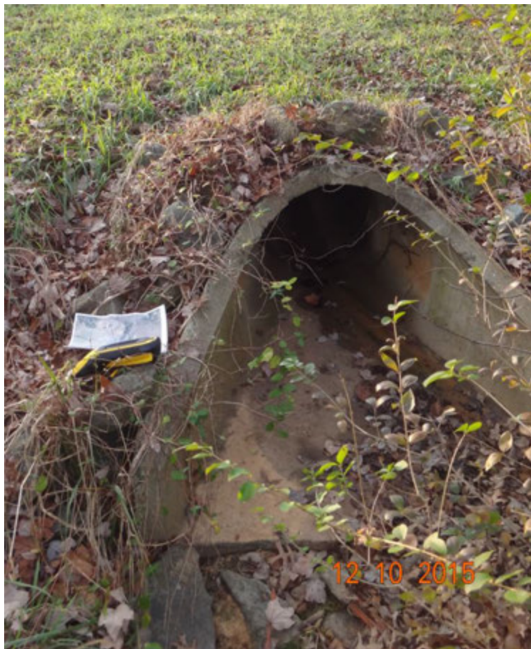
Figure 3. Sand deposit on outfall apron (left side when facing outfall)
