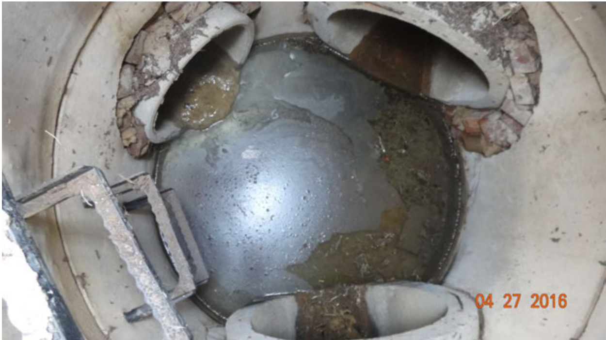
Figure 2. Three pipes connecting at the first manhole (MH1); note the thick slurry of minerals in the flowing water from the north pipe (upper left)
