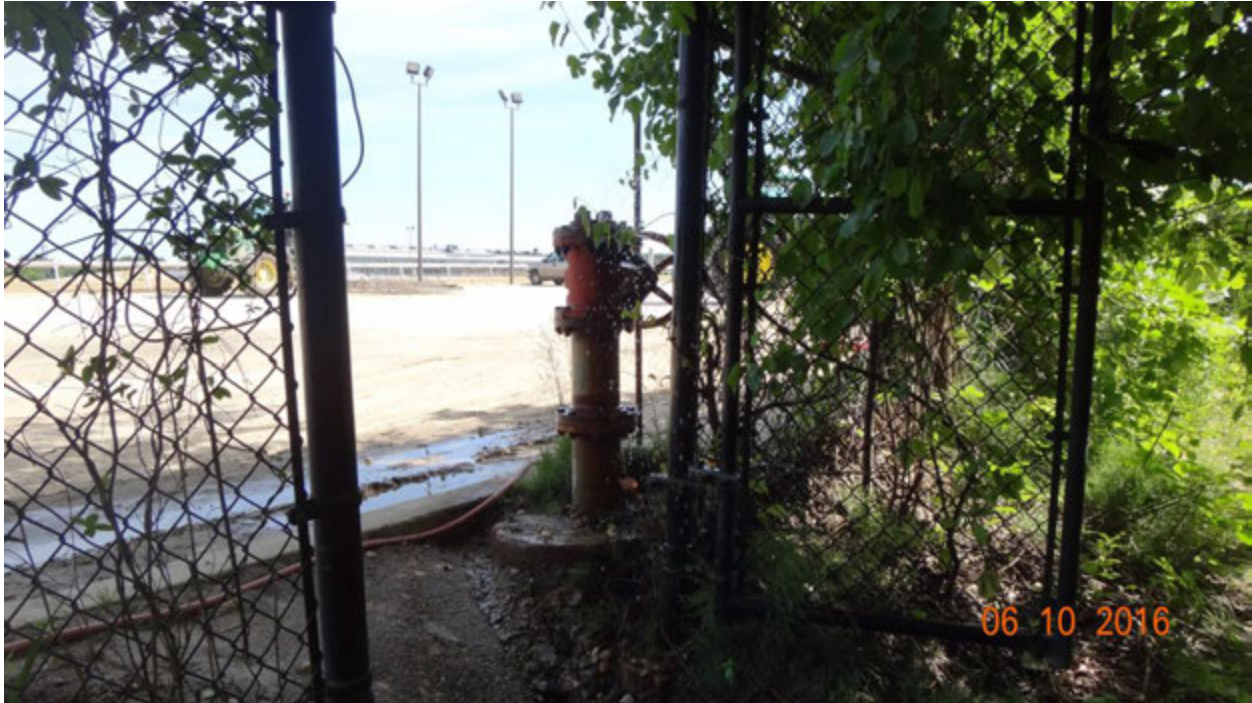
Figure 5. A red post hydrant with a valve inside the fenced maintenance area; at the time of the field visit in June 10, this hydrant was leaking water (spraying it into the air)
