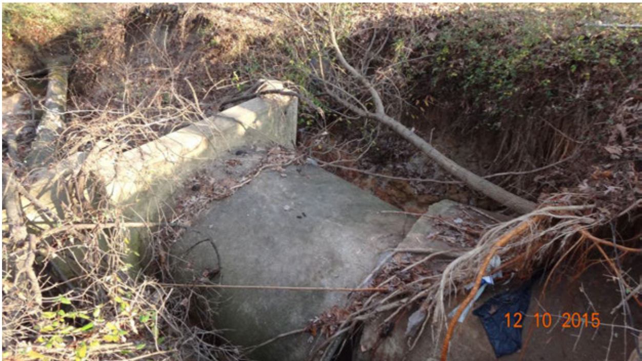
Figure 3. Detail of collapsed outfall pipe infrastructure showing misaligned junction between the End Section (left) and Section 2 (right)
