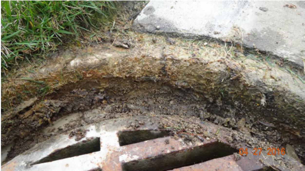
Figure 4. Signs of crumbling concrete at the opening for the yard grate, YG1
