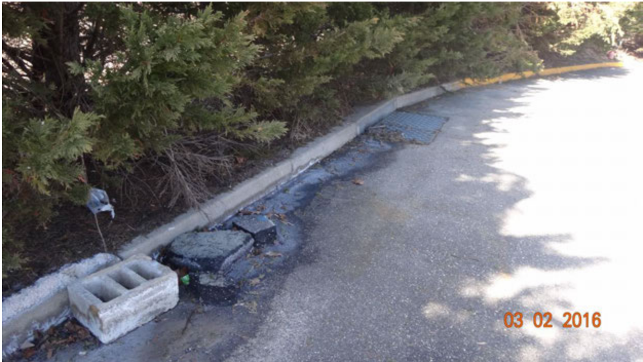
Figure 2. Evidence of the distribution of salt residue from the exposed pile of road salt along the edge of the parking lot toward the storm drain
