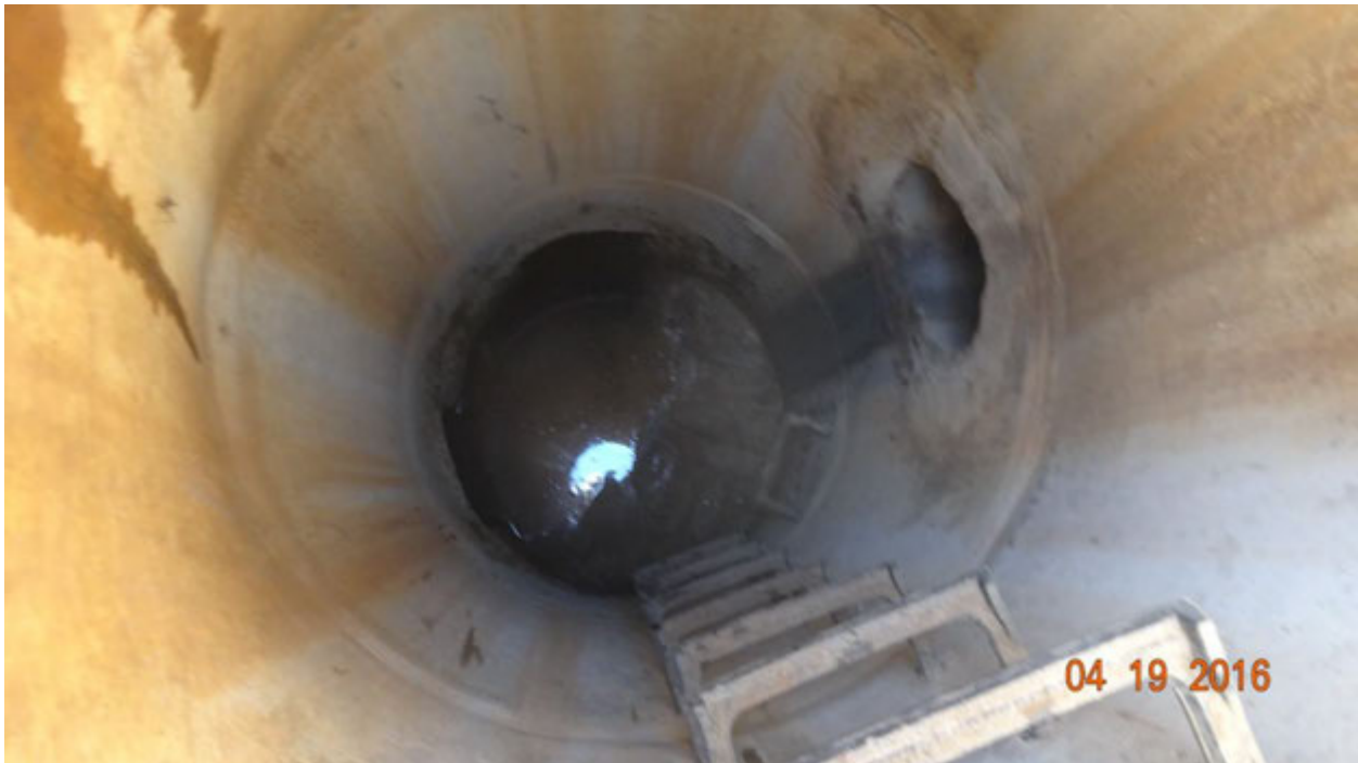
Figure 3. Evidence of standing water in the stormwater system on the western side of Escalon Avenue on April 19
