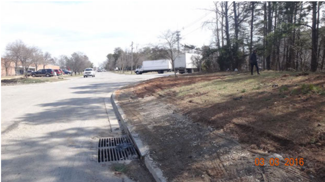
Figure 4. A photograph of the storm drain inlet to the west of the cul-de-sac of Midway Road, as seen facing east-southeast; note the tire tracks on the ground above the inlet and toward the cul-de-sac
