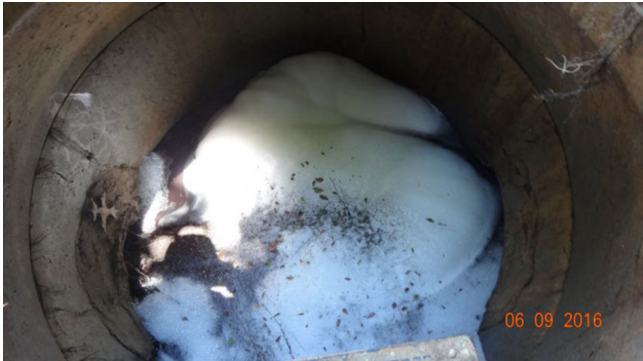
Figure 7. View of excessive suds inside the third manhole as observed on June 9
