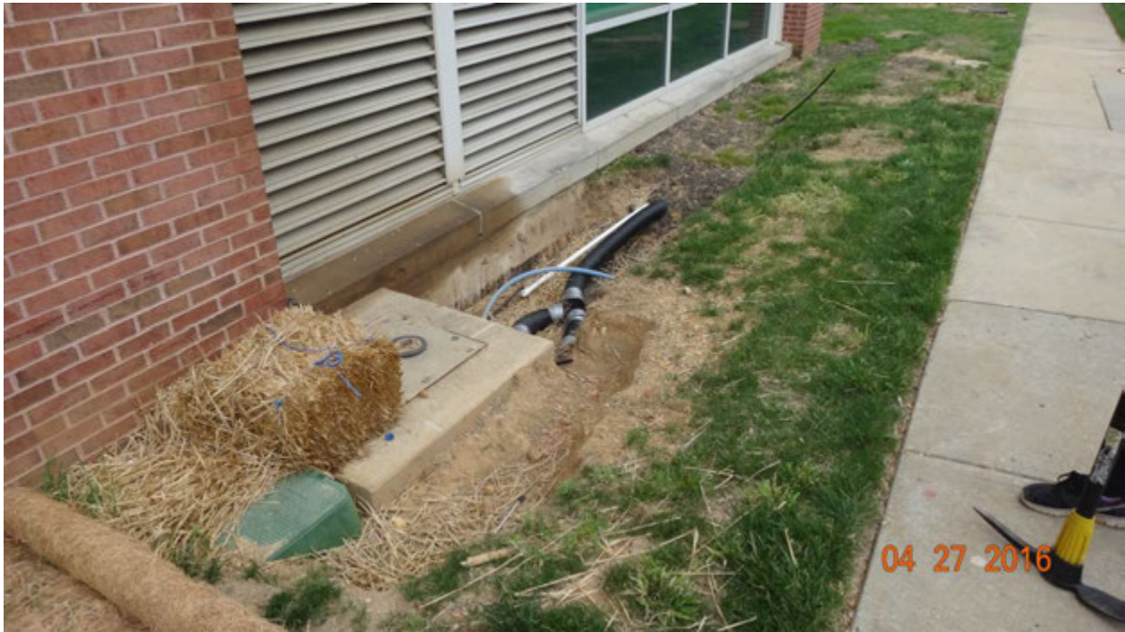
Figure 3. Signs of a hole opened alongside the building and exposed lines; note the dark stain on the sill
