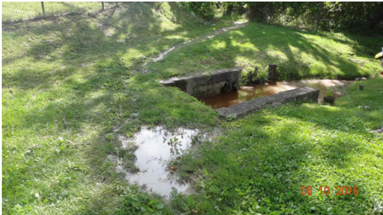
Figure 1. A pool of water (foreground) observed adjacent to outfall A11C7O001 on June 10
