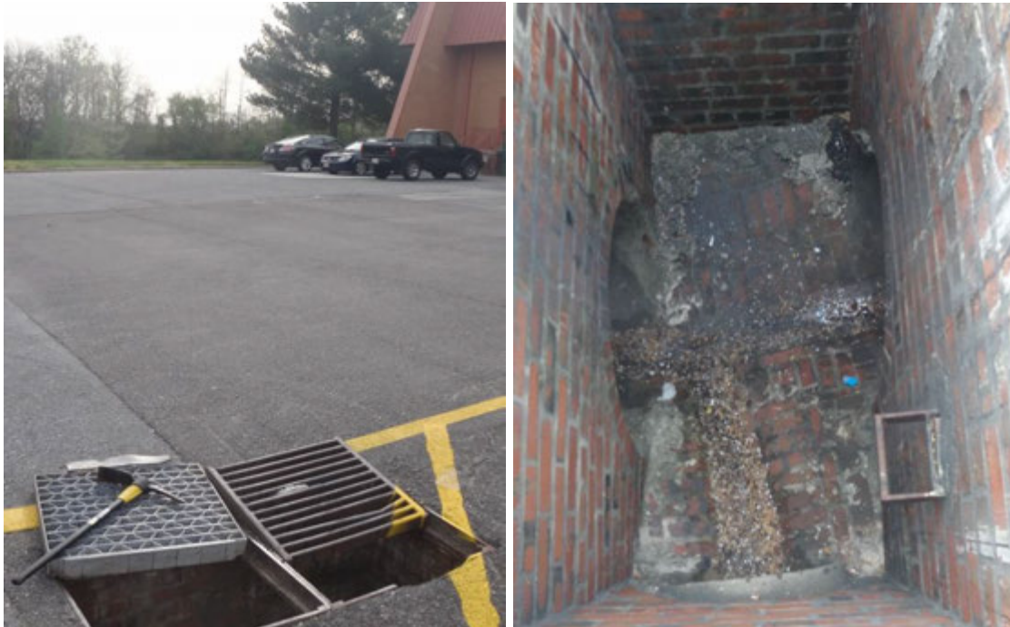
Figure 2. Yard grate (left) in the parking lot between the buildings at 601 and 611 Hammonds Ferry Road where the northwest and southwest drainage lines intersect (right) before draining into the pipe leading to the target outfall
