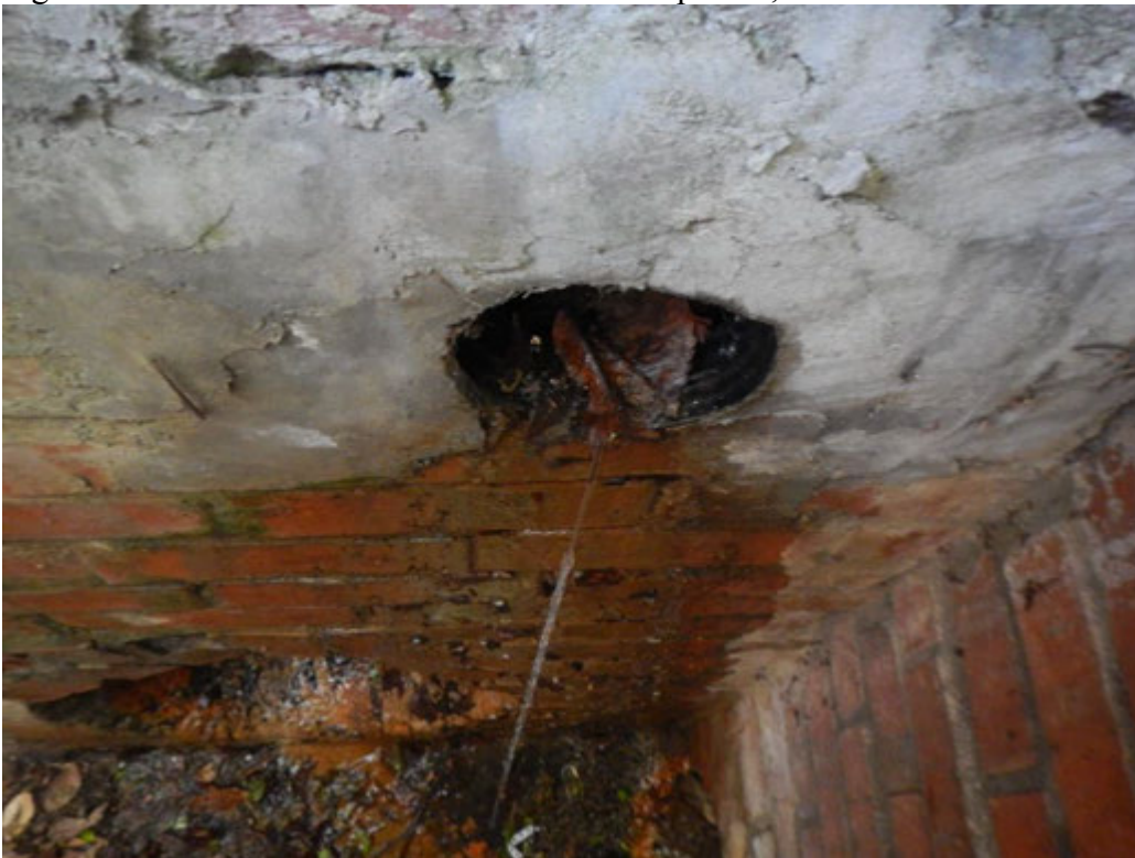
Figure 2. Flow observed from a 4-inch pipe entering a network curb inlet (third catch basin up the network from the outfall) on April 19
