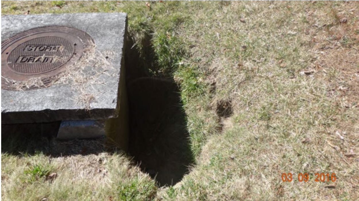
Figure 2. Evidence of collapsed soil on the northwest side of the inlet frame, seen facing southwest
