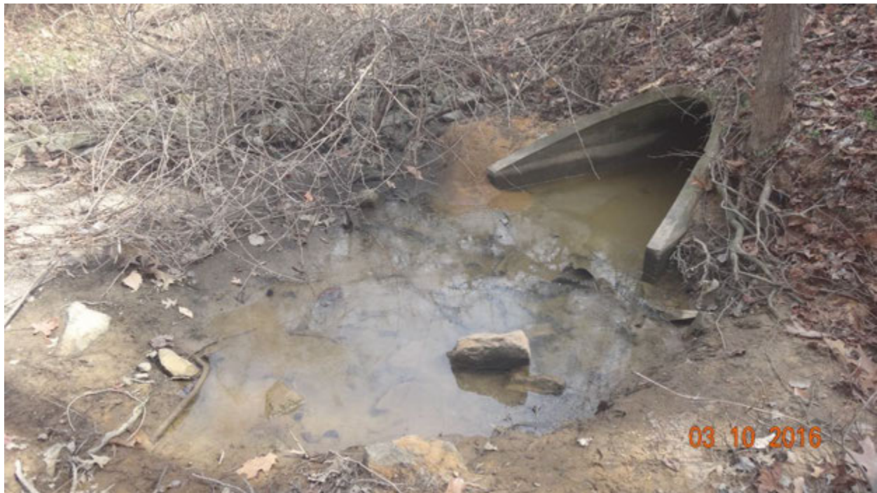
Figure 1. Stagnant water found at outfall G13G7O006 on March 9
