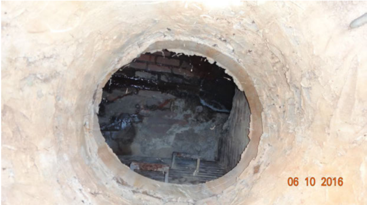
Figure 2. View inside the fourth manhole; note the trail of water from the west (right)
