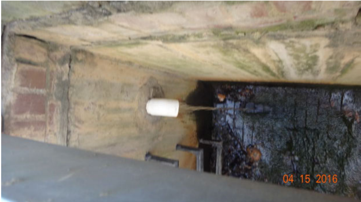
Figure 2. Evidence of strongly flowing effluent from a PVC pipe in the curb inlet box on April 15
