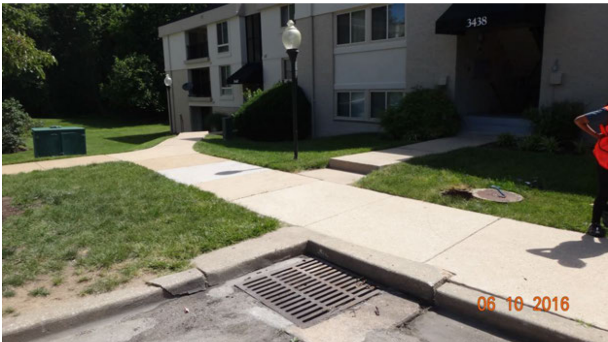
Figure 2. View showing the relative location of the manhole (center-right) to the curb inlet; the team obtained a sample of water for testing from the opened manhole
