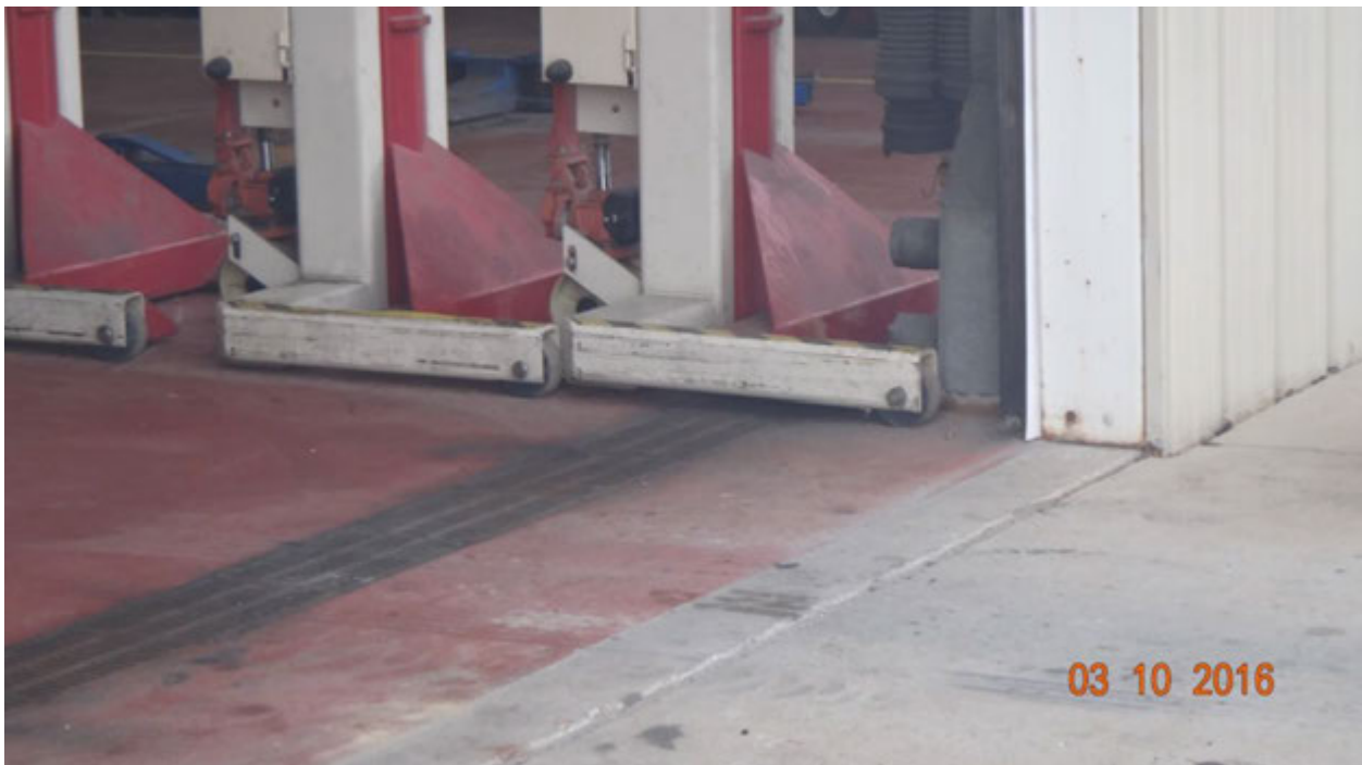
Figure 5. Photograph showing trench inlets in the bays; staff presumed that these were also connected to the stormwater network via new pipes
