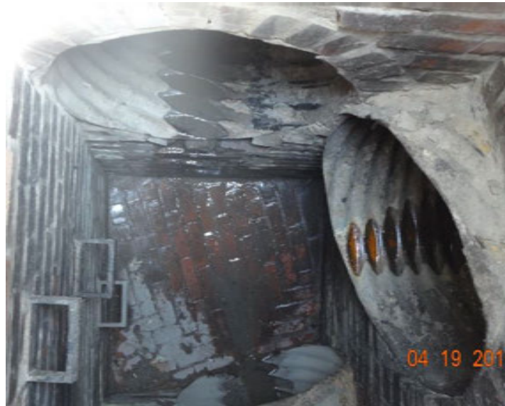
Figure 2. Flowing water observed from one of the pipes (from the east) contributing to the network, as documented from within a manhole to the east of the outfall
