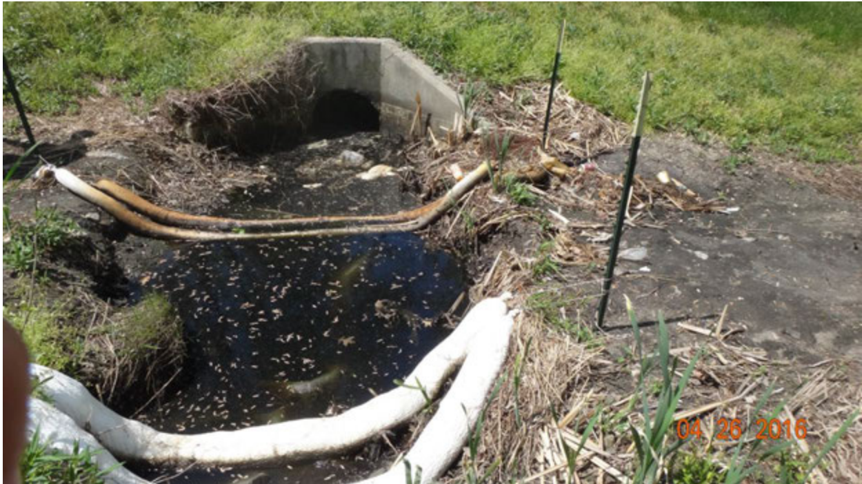
Figure 1. Outfall I03E8O003 as observed on April 26, 2016, with the absorbent socks installed to constrain the fuel in the water
