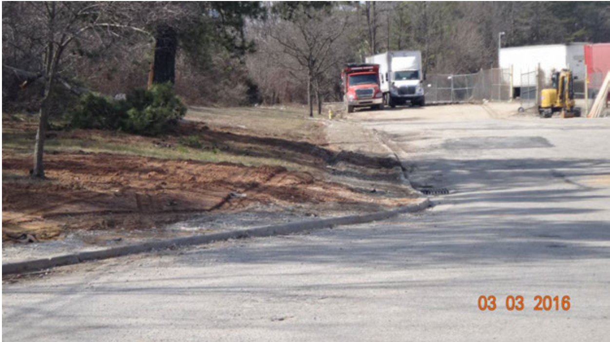
Figure 3. A photograph of the storm inlet just west of the cul-de-sac of Midway Road (center right), as seen facing west-northwest
