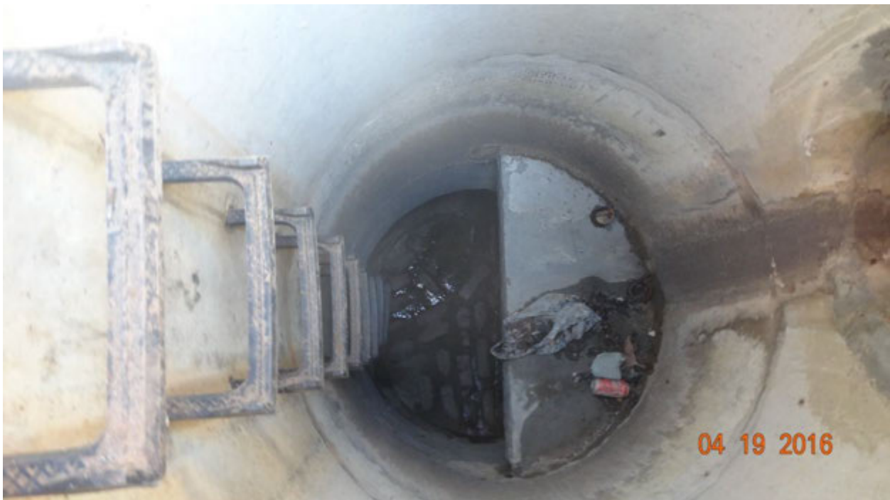
Figure 2. Flowing water observed in a manhole on the eastern side of the Escalon Avenue neighborhood on April 19; the water flowed from the west
