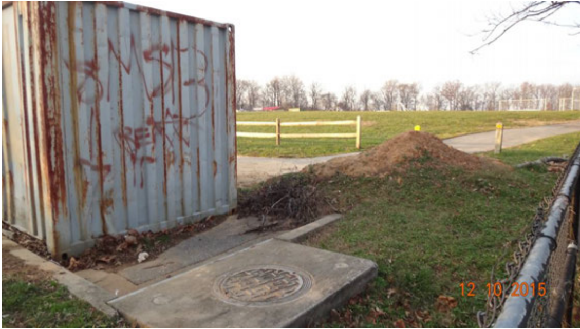
Figure 2. A view of the impervious surface leading to the storm drain inlet; the flows to the inlet are almost completely blocked by the storage trailer and the large pile of sand and sediment
