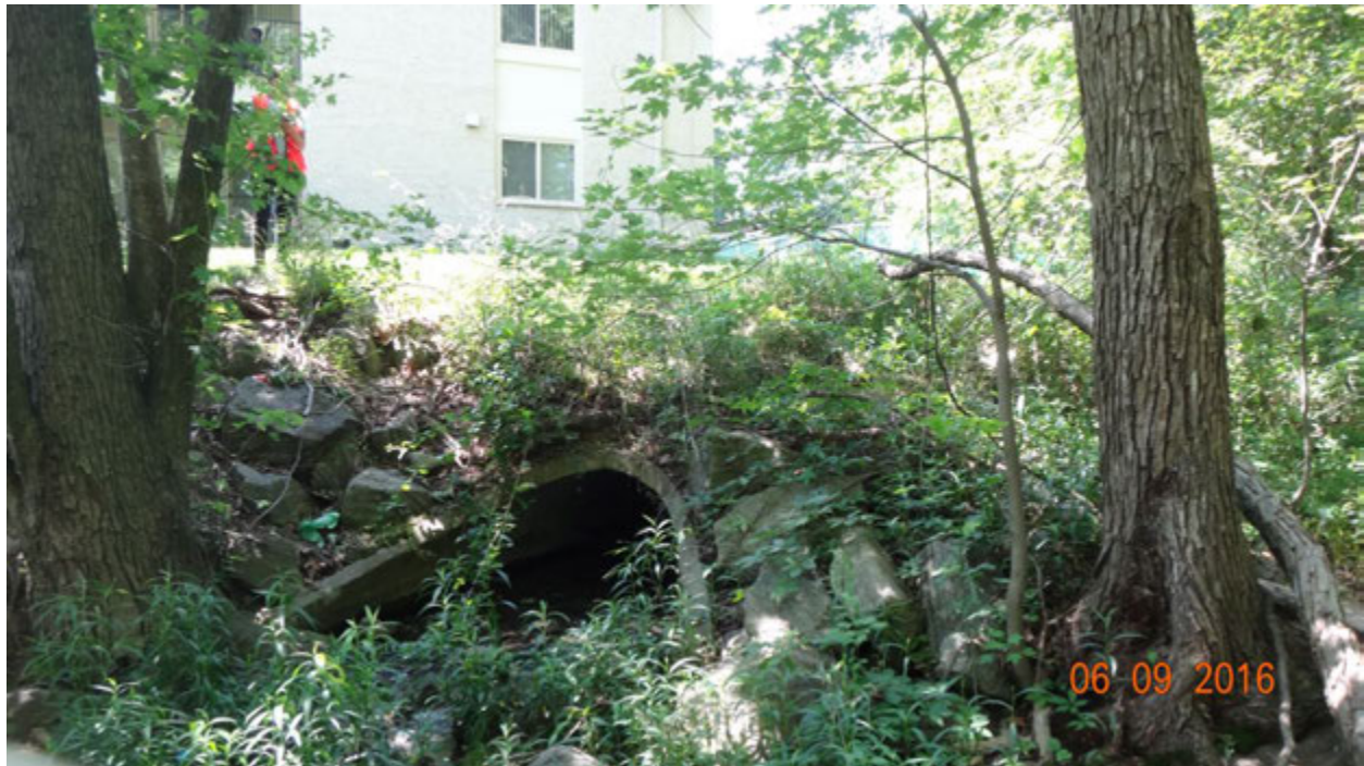
Figure 1. Outfall B12G2O001 as observed on June 9, 2016
