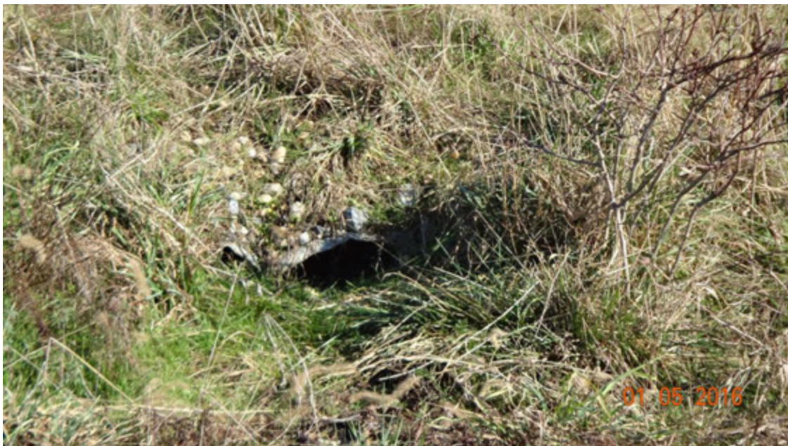
Figure 1. Photograph showing detail of the outfall C10E4O001 and the narrowed opening of the crushed pipe; note the small rocks on the top of the pipe, possibly associated with fill dirt, and the extensive vegetation partially blocking the opening
