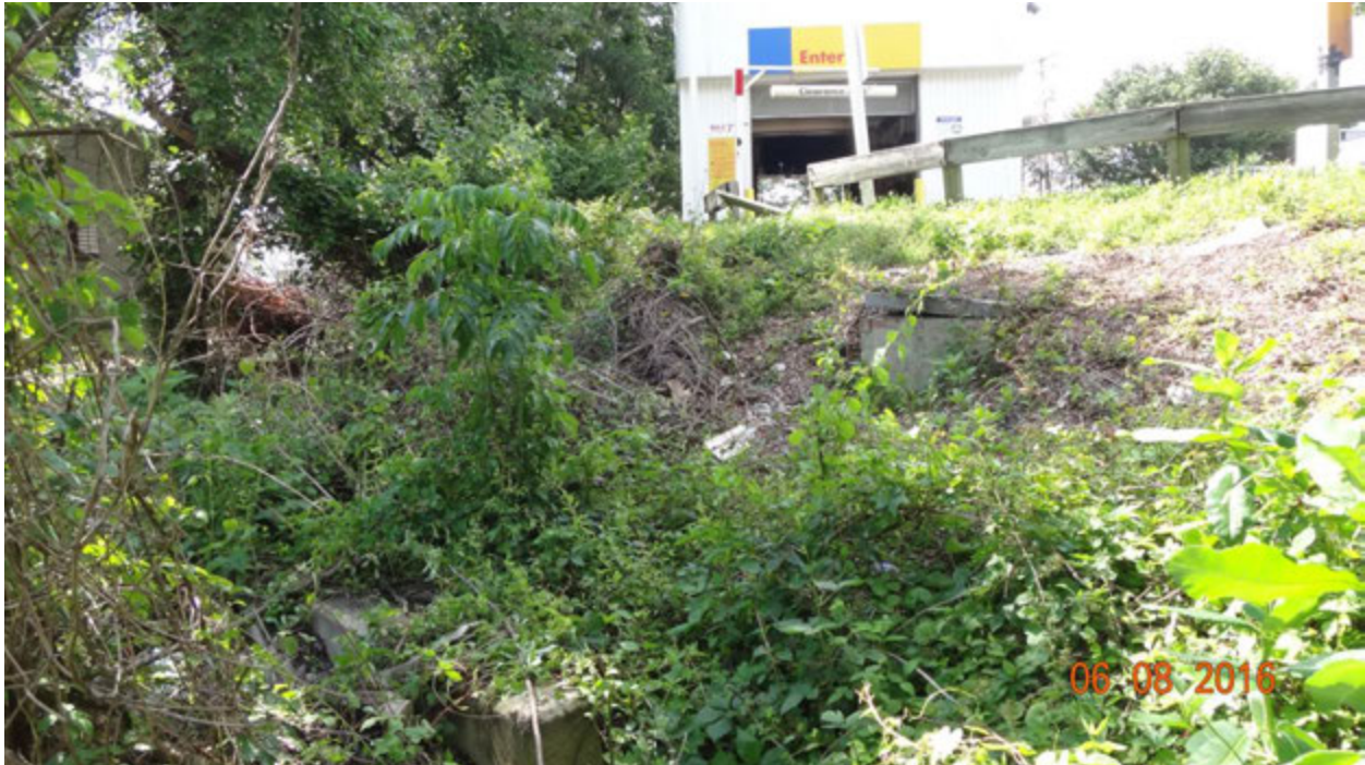
Figure 5. View showing the relative location of the outfall F09G50001 (lower left), the first manhole (center right) and the entrance to the car wash (top)
