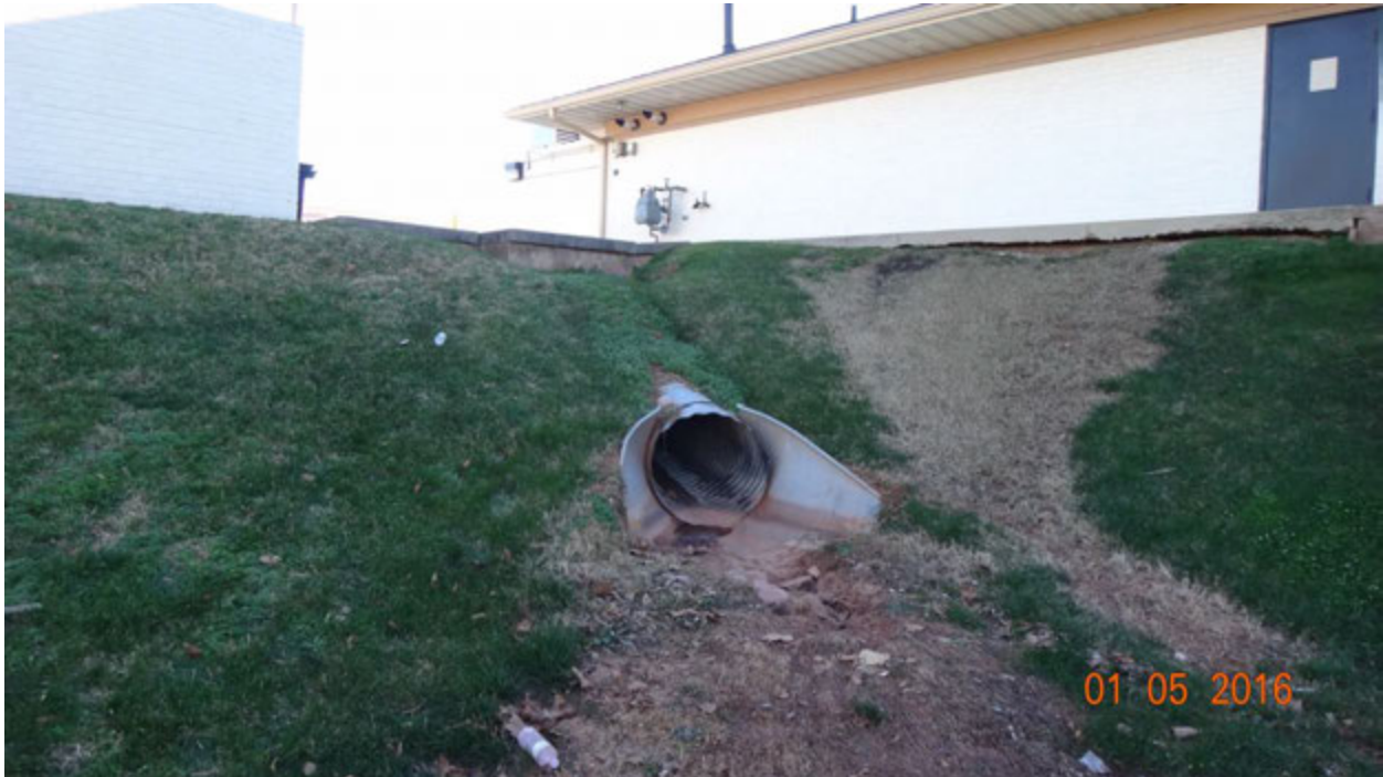
Figure 2. View looking uphill from the stormwater management facility; note the separation of the catch basin from the top slab (upper center left), the sunken ground around the outfall pipe (center), and the erosion under the sidewalk (upper right)
