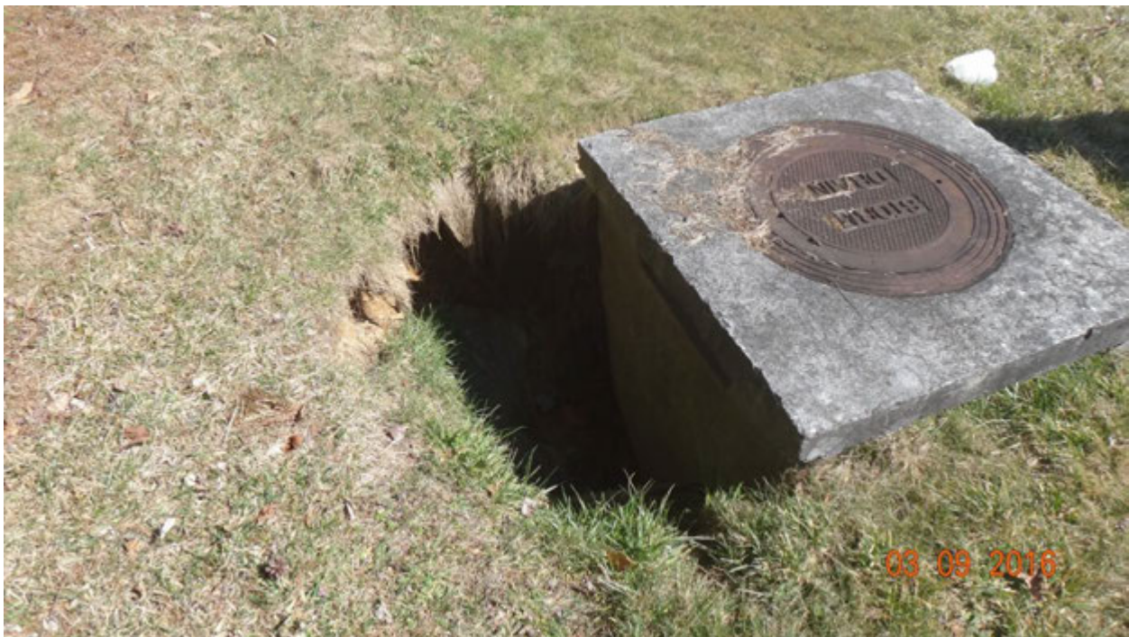
Figure 3. Evidence of collapsed soil on the northwest side of the inlet frame, seen facing northeast
