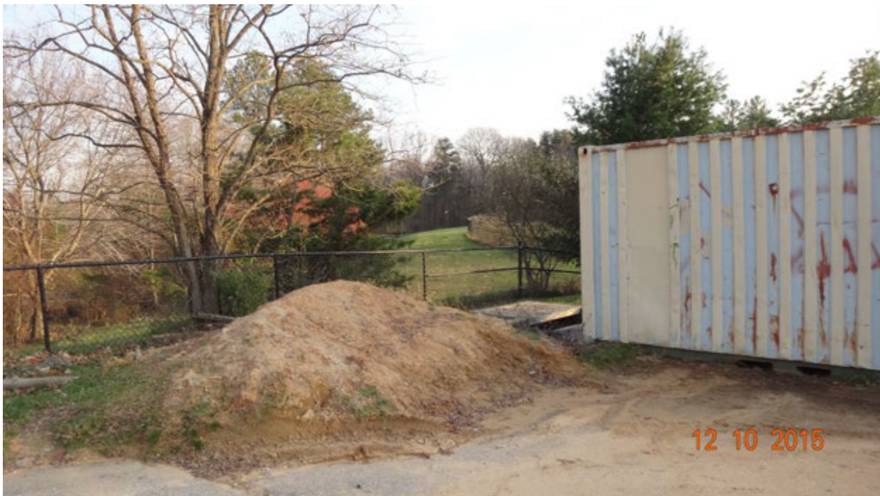
Figure 1. An uncovered pile of sand and sediment found on the parking lot adjacent to a storage trailer; note the curb inlet which can be seen between the two
