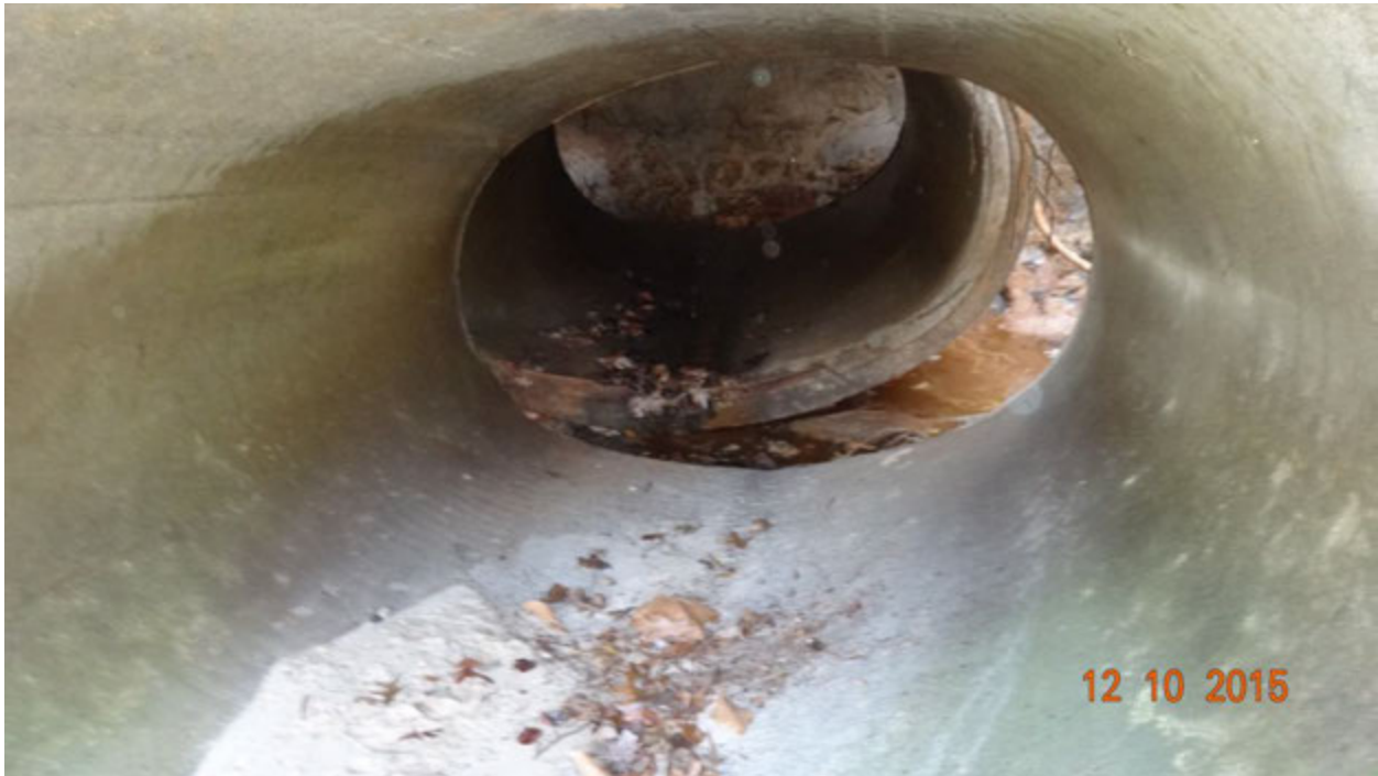
Figure 4. Photograph taken inside the End Section, showing the extent of disconnection with Section 2
