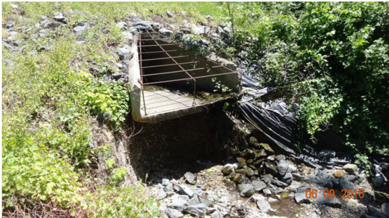
Figure 8. Flowing effluent from outfall F09F5O001, as observed on June 9, 2016; note white suds among the rocks in the plunge pool
