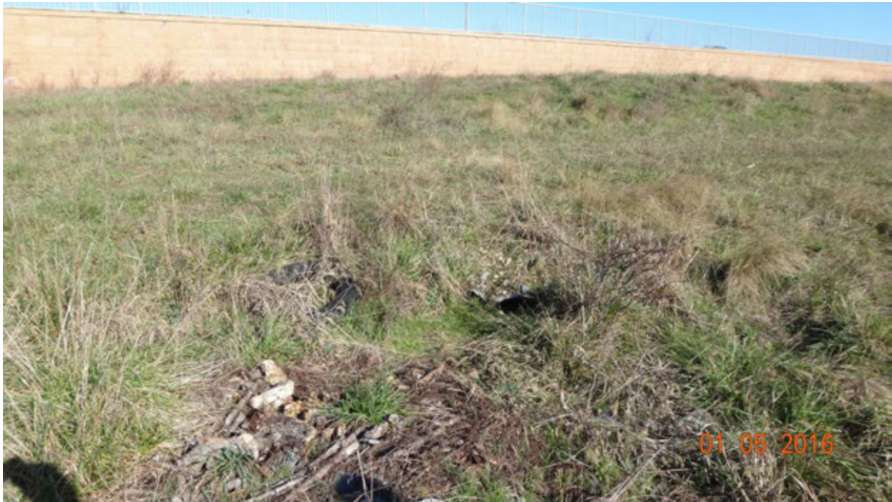
Figure 2. Photograph showing the opening for outfall C10E4O001 (seen as a dark oval in the center right) in context with the retaining wall for the parking lot for 8201 Dorsey Run Road
