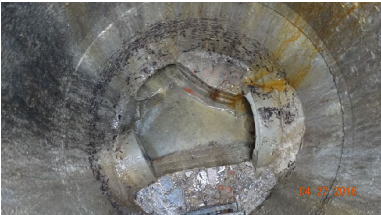
Figure 3. View inside third manhole (MH3) showing mineral deposits in the flowing water and signs of seepage along the walls
