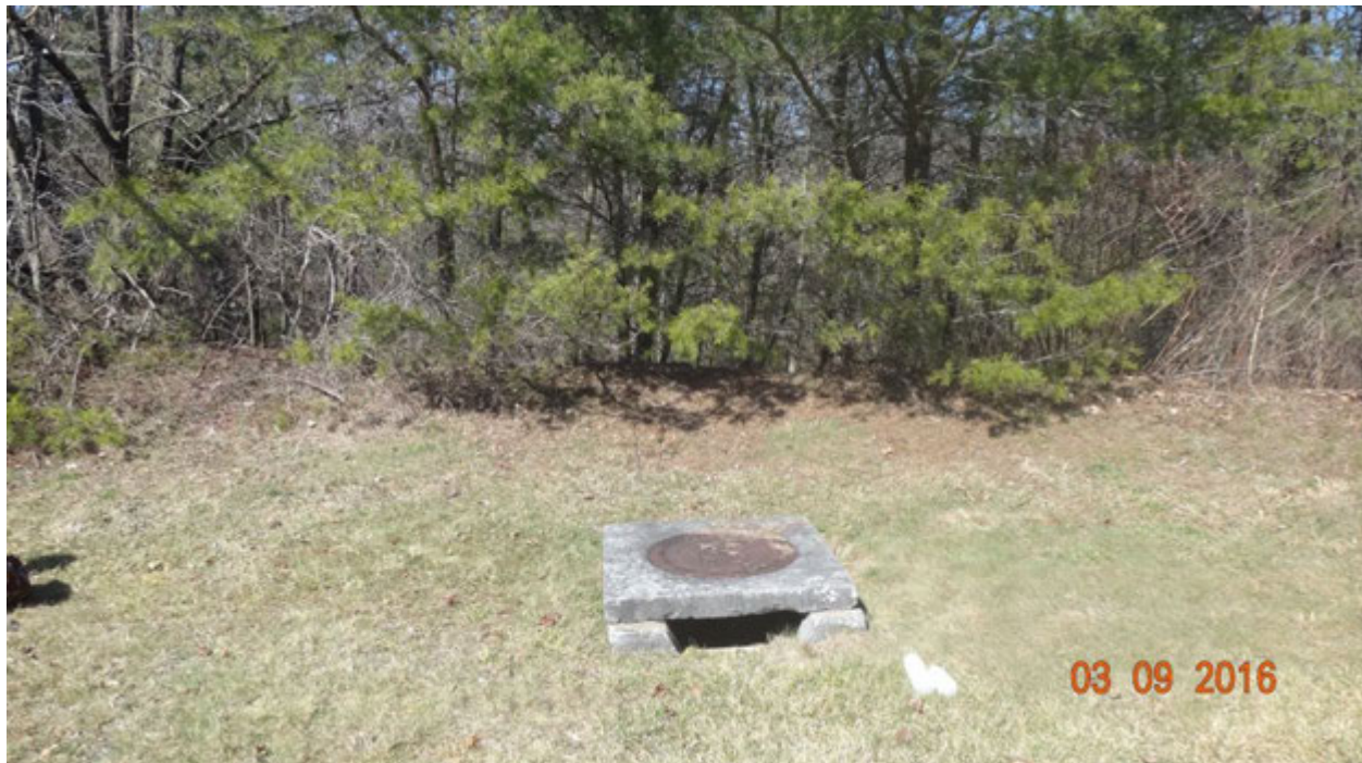
Figure 1. Slab top yard inlet found in damaged condition during the field visit
