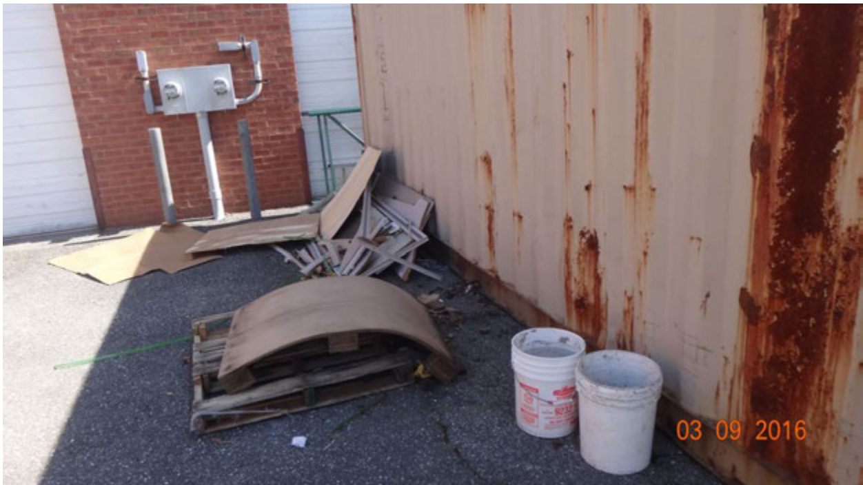
Figure 4. Loose debris found in the alcove behind National Carpet, including wood pallets, cardboard, metal framing, and two reused plastic buckets found on March 9
