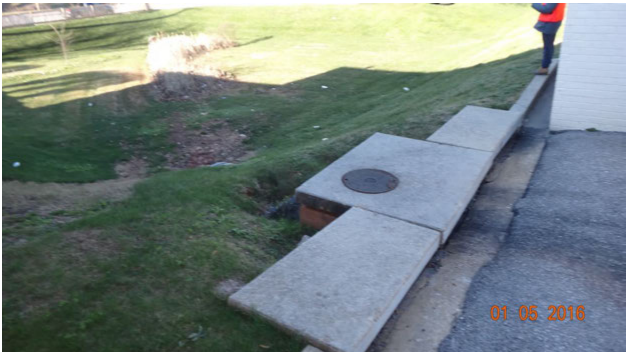
Figure 3. View from the curb inlet toward the stormwater management facility showing the depression behind the catch basin and side structures; also note stains leading into the curb inlet
