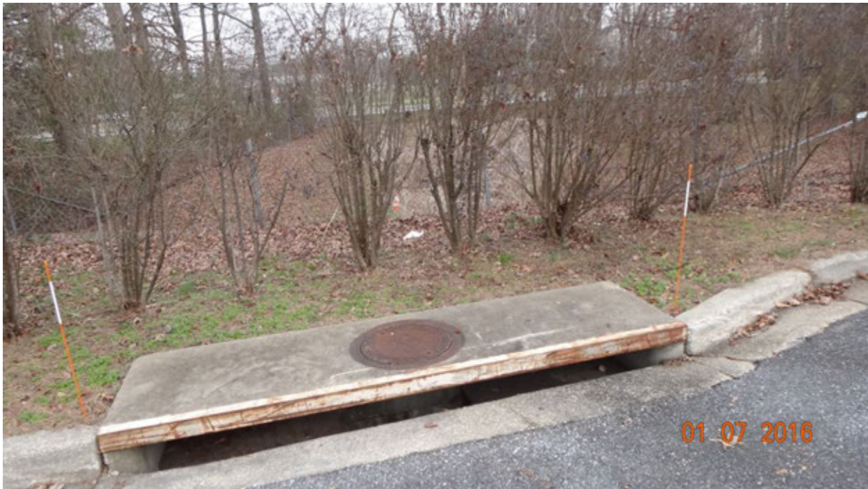
Figure 1. View from the curb inlet at the parking lot toward outfall I13B1O009; note the position of the orange cone (center) which serves as a reference in Figure 2
