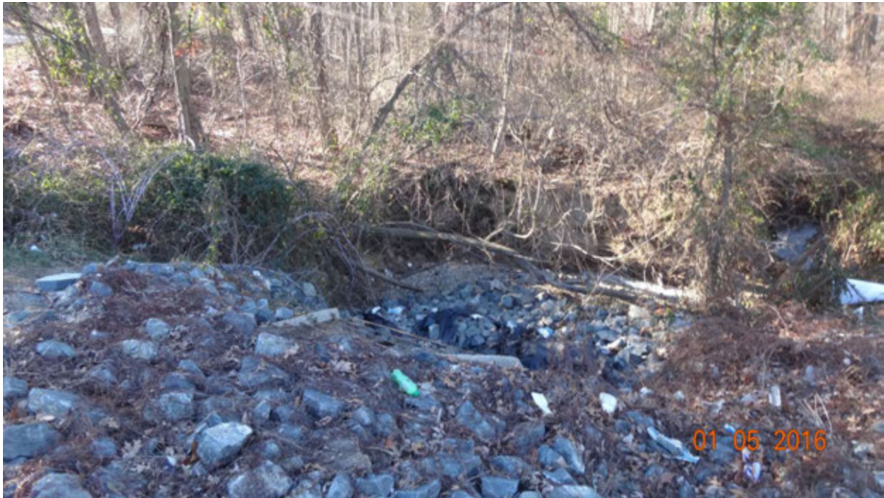
Figure 2. View looking over the top of the outfall showing the extent of erosion on the opposite bank caused by excessive, uncontrolled flows; note the collection of rip rap rocks in the plunge pool which may be acting as a partial blockade for the water, forcing the flows to veer left after exiting the pipe
