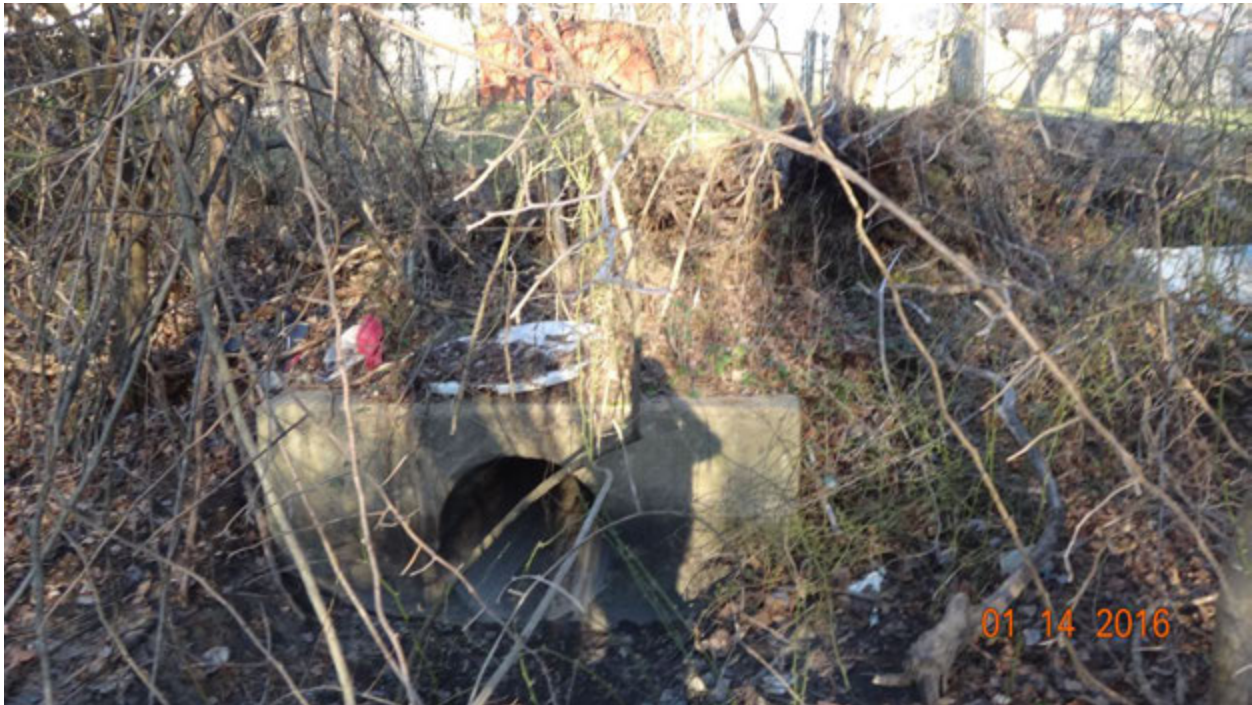
Figure 2. Photograph of outfall H10E5O001 with debris scattered around it; note the mattress on the right side of the photograph
