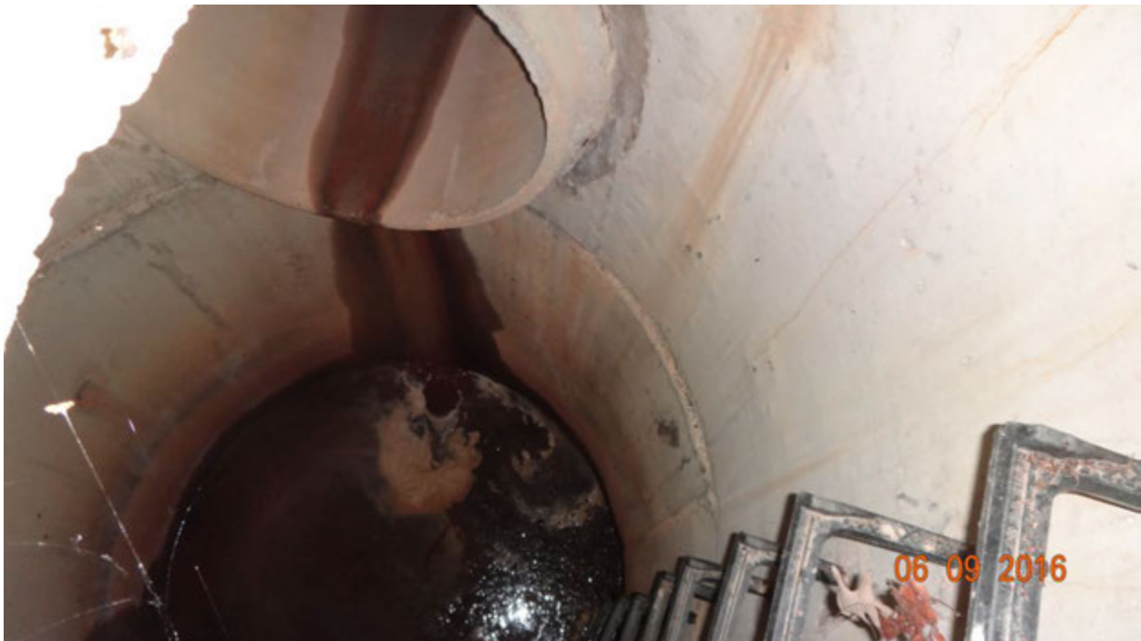
Figure 2. View inside the first manhole; note the slight trickle of water from the main pipe (top)
