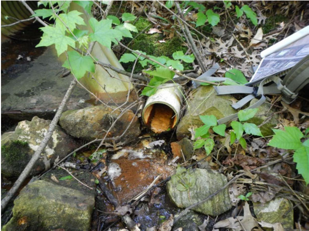
Figure 1. The conditions of Outfall J15H5Onew1 as observed on May 20; note the orange material evident in the pipe and the orange staining on the rocks near the opening. The discharge's blue oil sheen can be seen in the lower center of the photograph. Part of the adjacent 18-inch corrugated metal pipe is shown on the left side of the photograph.
