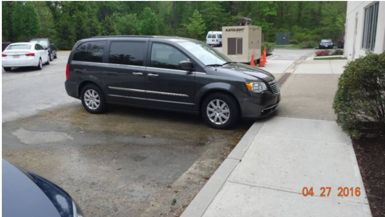
Figure 6. Signs of groundwater seeping through the parking lot on the east side of the hotel; note the trench drains in the parking lot (upper right)
