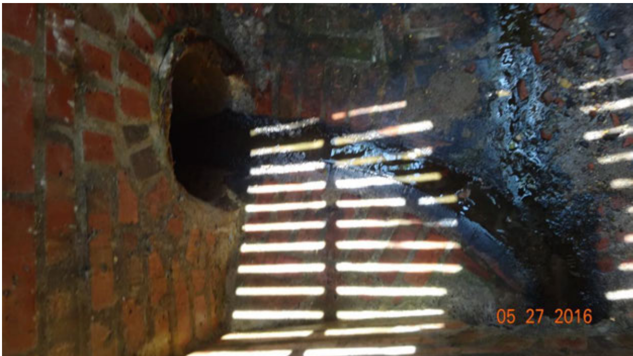
Figure 3. View inside the first curb inlet, showing the discharge flowing from the direction of the second curb inlet (left); note the line of moisture in the upper right which indicates a second pipe input to this inlet (from the southeast)
