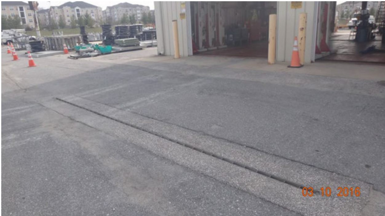
Figure 4. Photograph showing the end of the repaved portion of the parking lot that extends to the trench inlets by the bay doors; note that staff documented the presence of water in these inlets on March 10 but did not obtain samples for testing
