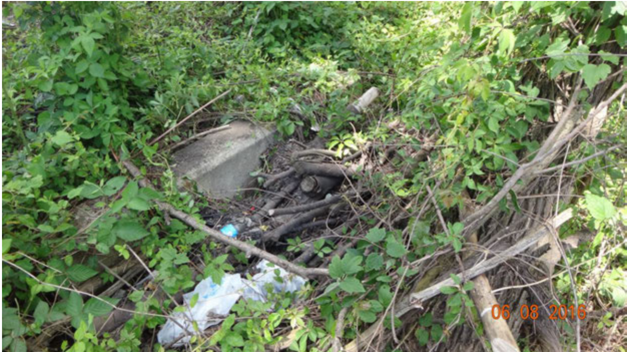
Figure 1. Outfall F09G5O001 as observed on June 8, 2016; note that cut limbs had been placed across the opening to the extent that the outfall appeared to be almost totally blocked during the field inspection
