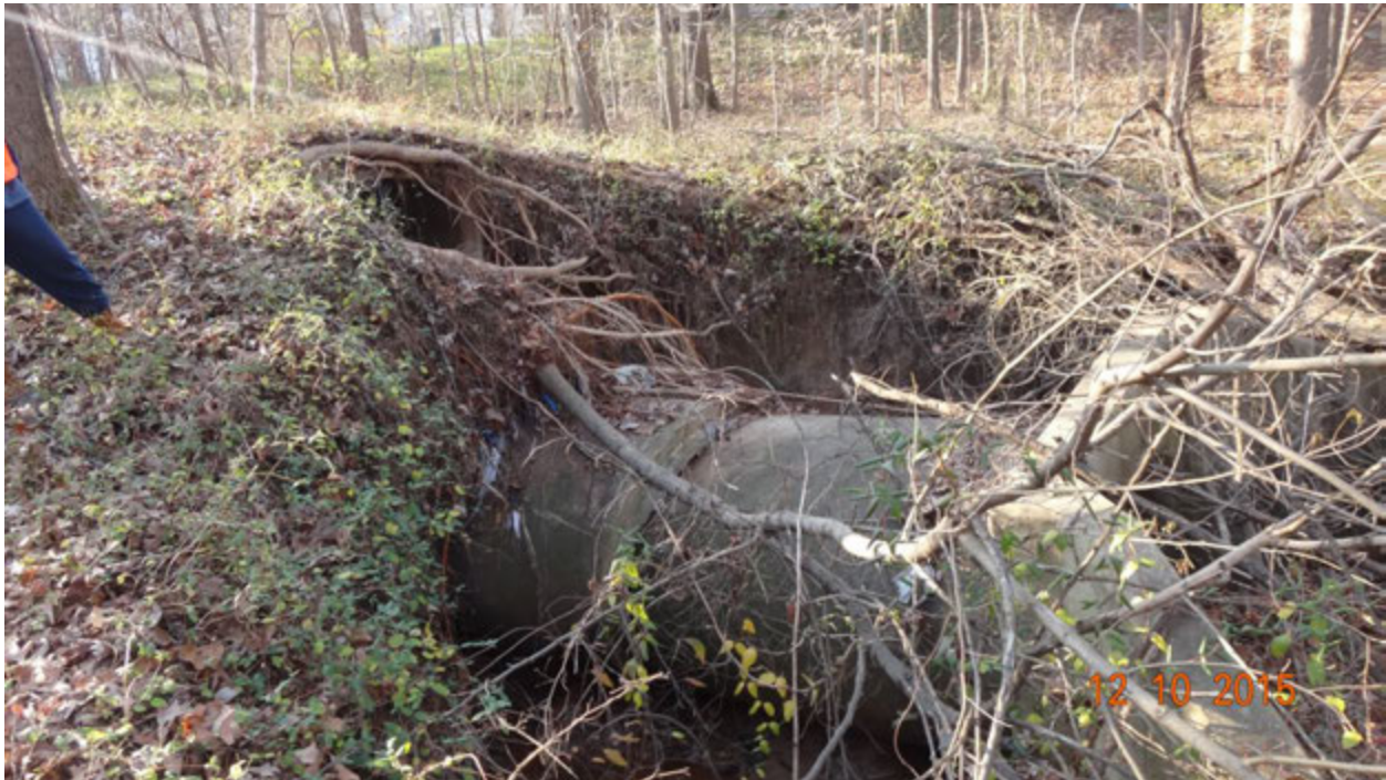
Figure 2. Collapsed outfall pipe showing extent of erosion along disconnected pipe sections (photograph taken facing approximately northwest)
