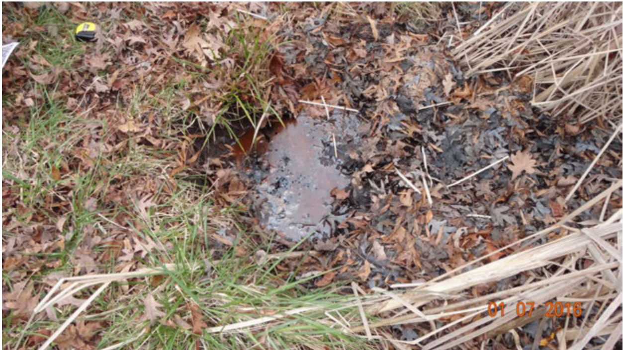
Figure 4. Detail of effluent from outfall I13B1O009 (presumed) showing oily sheen
