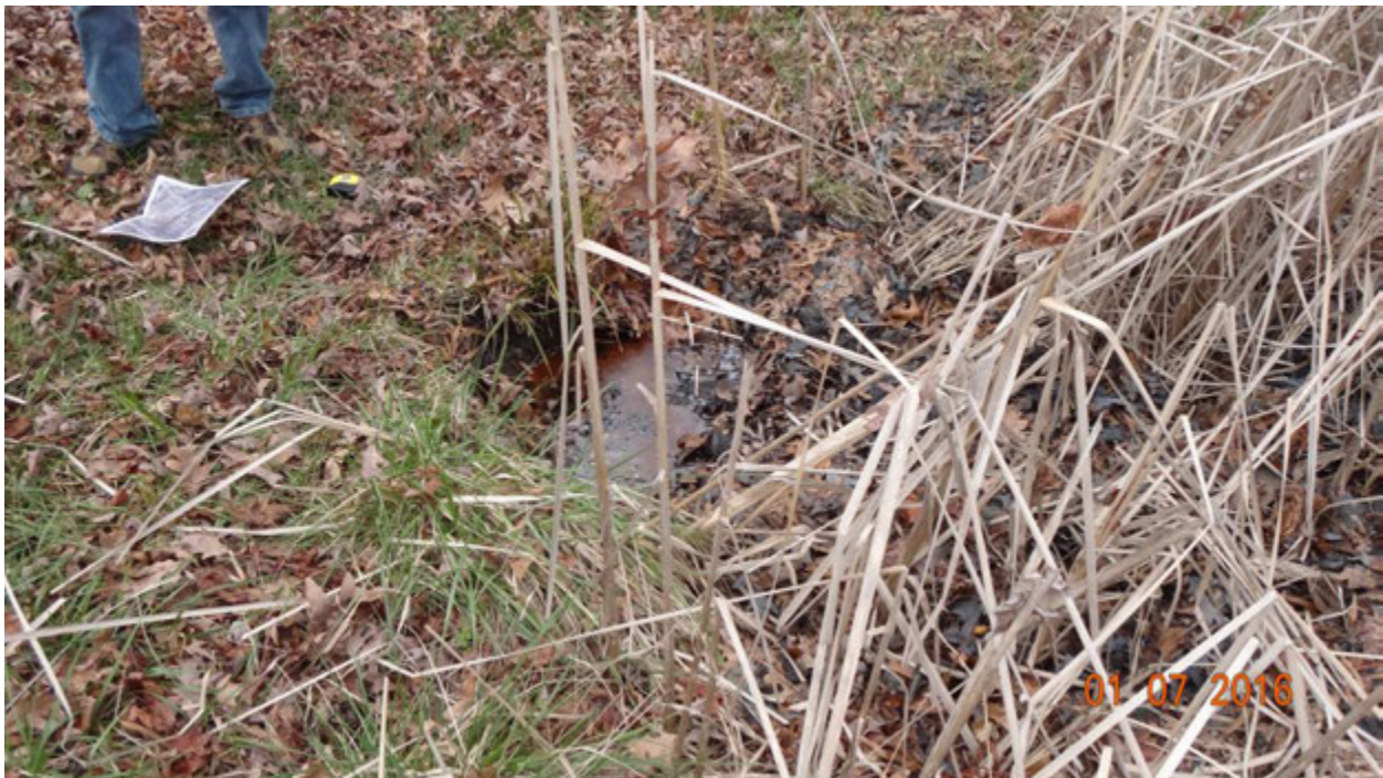
Figure 3. Photograph showing the conditions at outfall I13B1O009; the pipe was found almost completely buried in sediment at the time of the site visit
