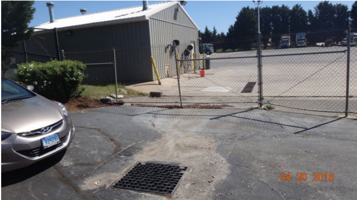
Figure 4. Yard grate adjacent to the maintenance lot and washdown area associated with Patuxent Materials, Inc.; although there is evidence of flow into the grate, as suggested by the accumulated sediment, the field team did not find flowing discharge at this location on April 20
