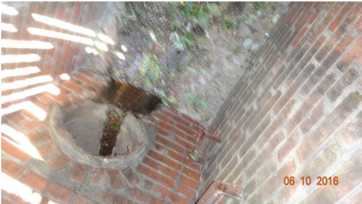
Figure 3. View inside the curb inlet south of the fourth manhole, showing a faint flow of water
