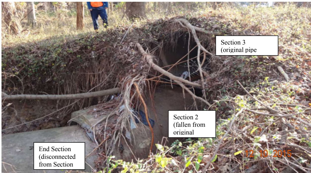
Figure 1. Three disconnected sections of pipe infrastructure associated with outfall B11F5O001; note original height of outfall pipes and ground level at Section 3, and erosion along all sections
