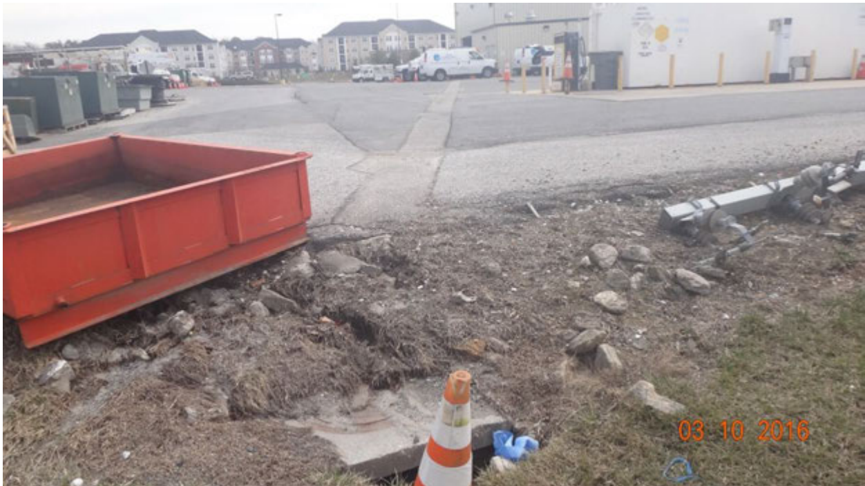
Figure 3. Photograph showing part of the repaved portion of the parking lot that correlates with the stormwater network; note that staff did not open the curb inlet in the foreground
