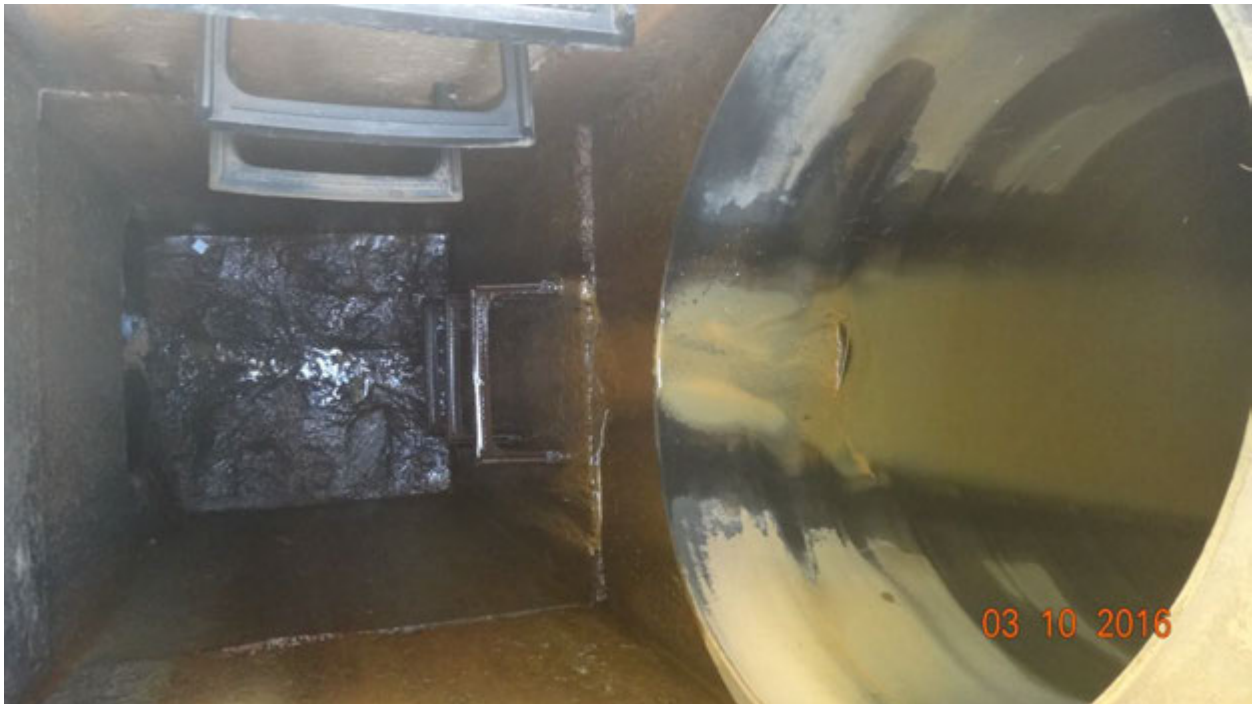
Figure 2. Evidence of flowing effluent in the yard grate, the nearest access point on the network from the outfall; note that this photograph was taken on March 10
