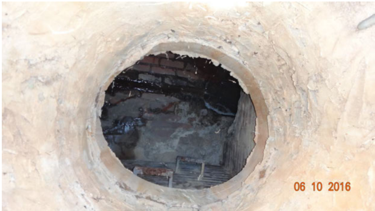
Figure 3. View inside the manhole; note the soapy waste water pooled on the right
