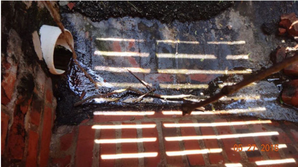
Figure 4. A white PVC pipe (left) contributing flow to the stormwater system from a source to the east of the second curb inlet up-network from the outfall
