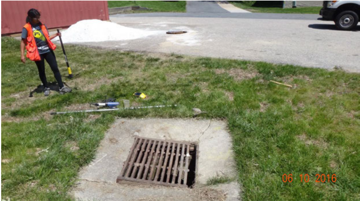
Figure 4. A yard grate (foreground) that appeared to be connected to and contributing water to the manhole in the parking lot (background)
