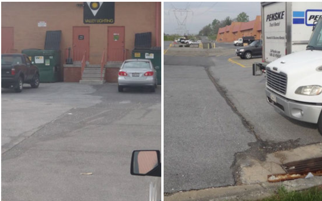
Figure 3. Damp pavement evident around a personal vehicle behind Valley Lighting (left) and evidence of runoff to the curb inlet at the east end of the parking lot (right)
