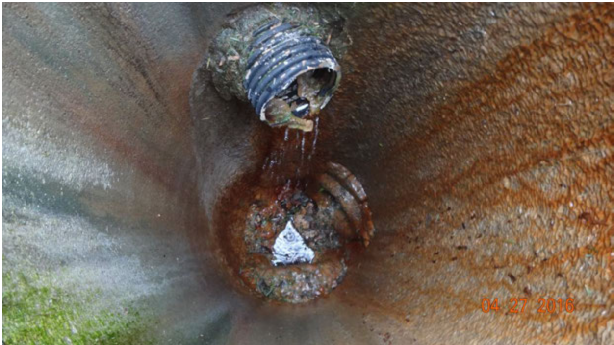
Figure 5. View inside the yard grate, YG1, showing the flow of water from a black PVC pipe drawing flow from the east side of the lot
