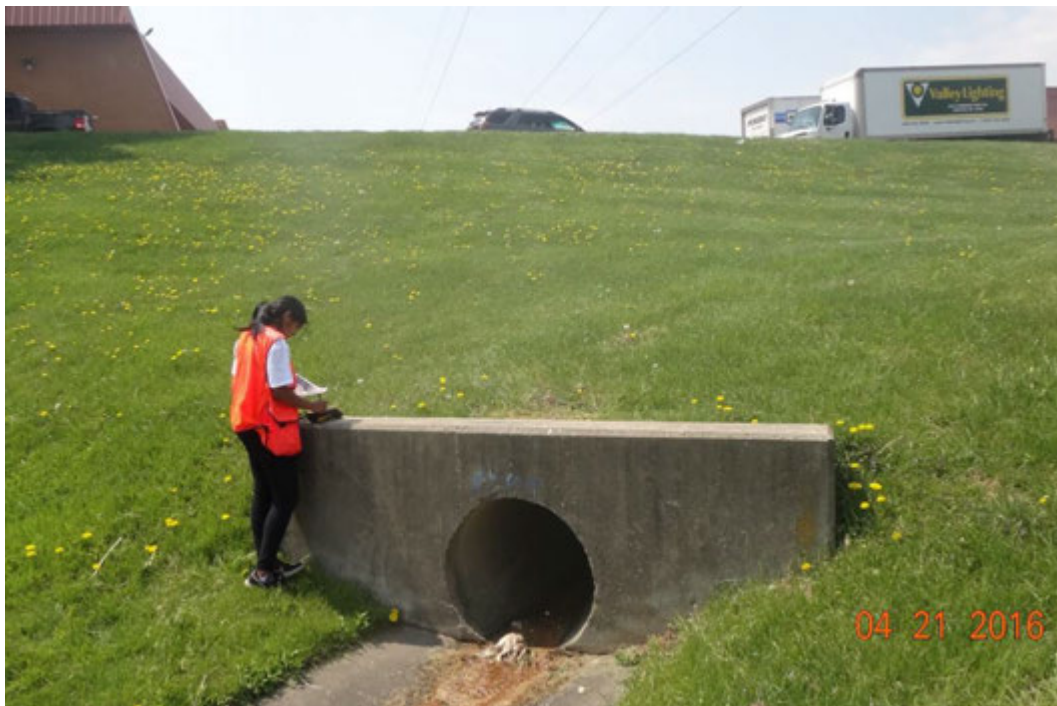
Figure 1. The target outfall, K02B8O002, located in a stormwater retention pond east of 601 and 611 Hammonds Ferry Road, as observed on April 21, 2016
