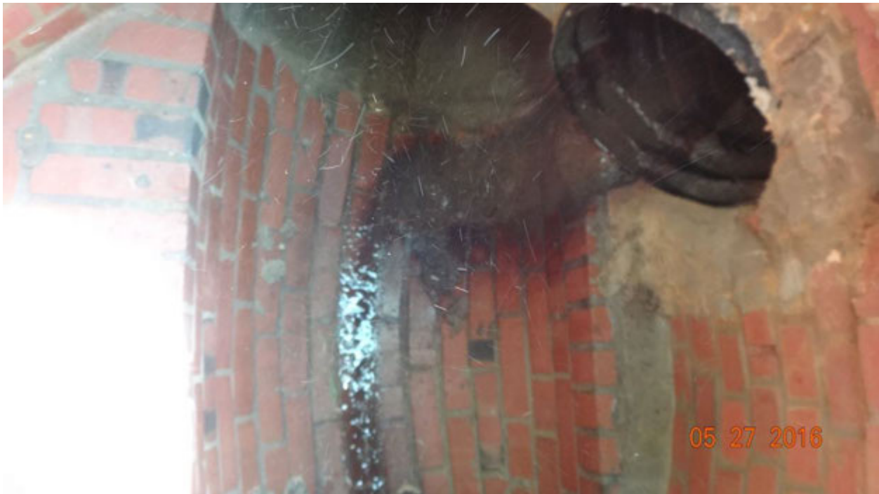
Figure 2. Two input pipes for the manhole up-system from the outfall; the large concrete pipe (top) was dry and the black pipe (top right) had flowing effluent from a source in line with the curb inlet to the east
