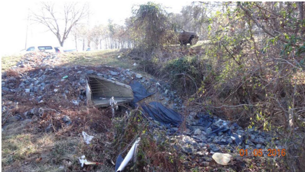
Figure 1. Photograph of outfall F09F5O001 showing the erosion and disturbed rip rap assembly on the southeast (right) side of the structure and the beginnings of undercutting erosion below the opening; note, also, the crumbling flared end on the right side of the outfall opening
