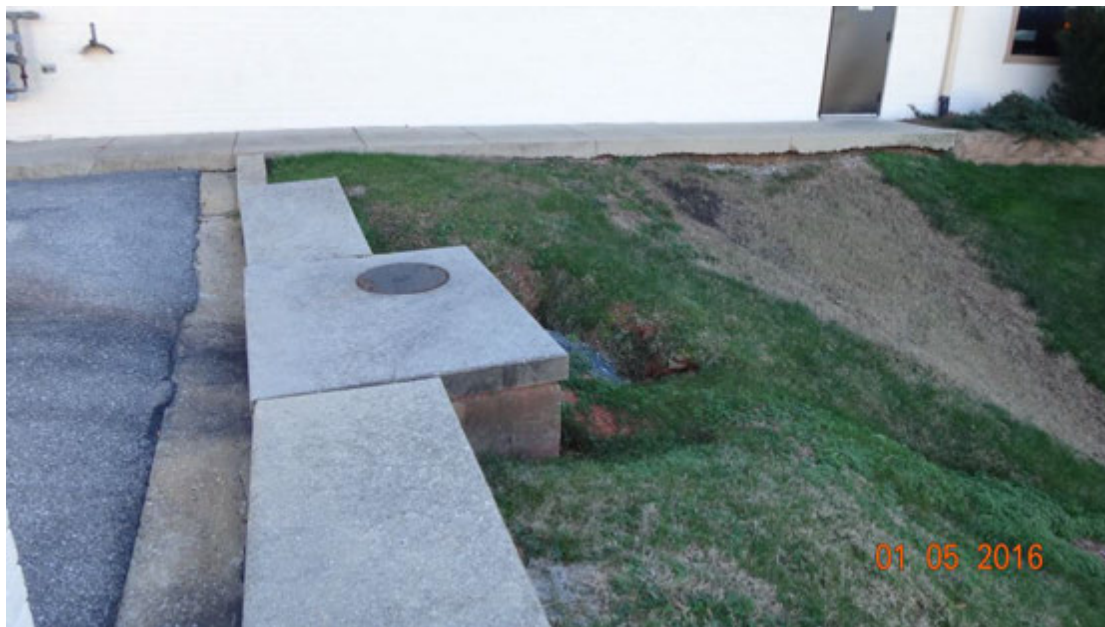
Figure 1. Photograph showing the curb-opening inlet with significant erosion behind it (center), and a nearby sidewalk area with erosion apparent underneath it and a distinct runoff pattern evident in the downslope vegetation (top right); note, also, stains in the parking lot leading from the Pizza Hut restaurant to the curb inlet (left)
