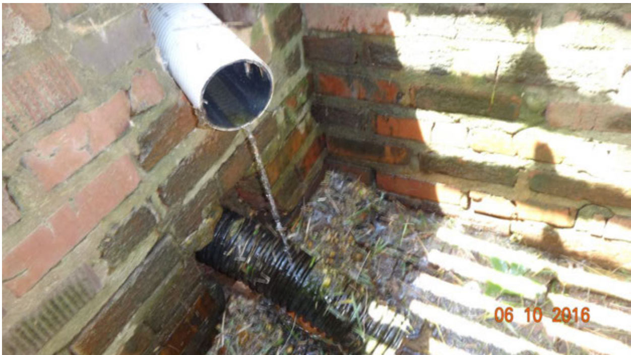
Figure 5. View inside the yard inlet showing flowing water from a small white pipe
