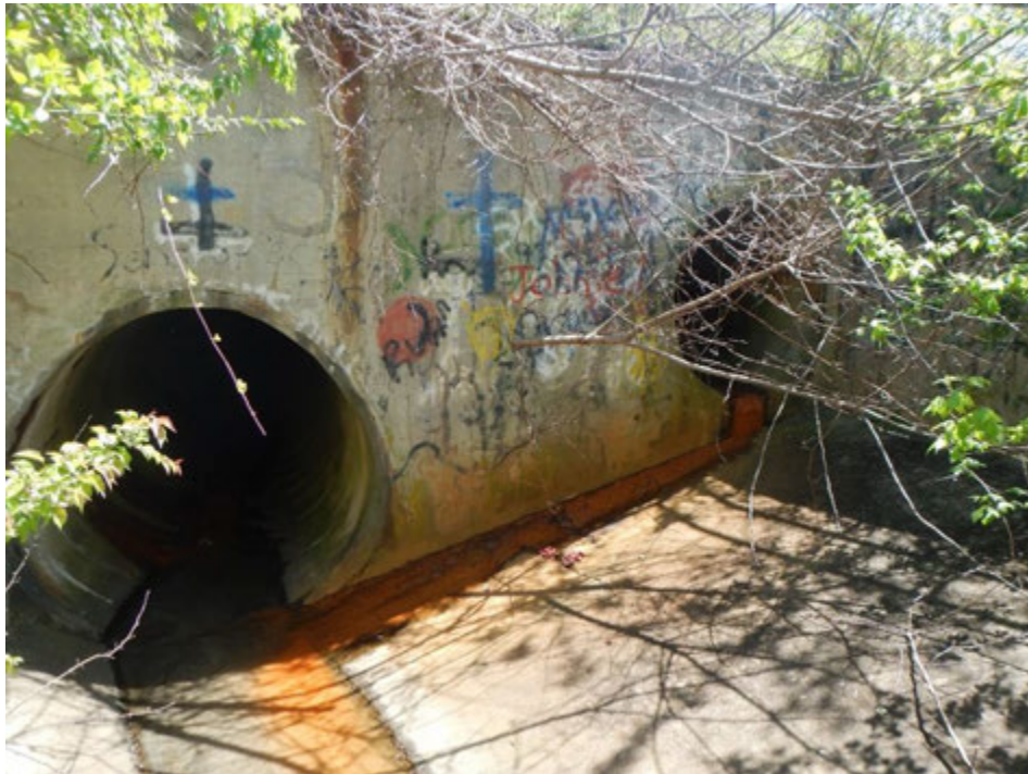
Figure 1. Outfall I17B6O007 exhibiting a rust-colored discharge, as observed by the LimnoTech field crew on April 18, 2016
