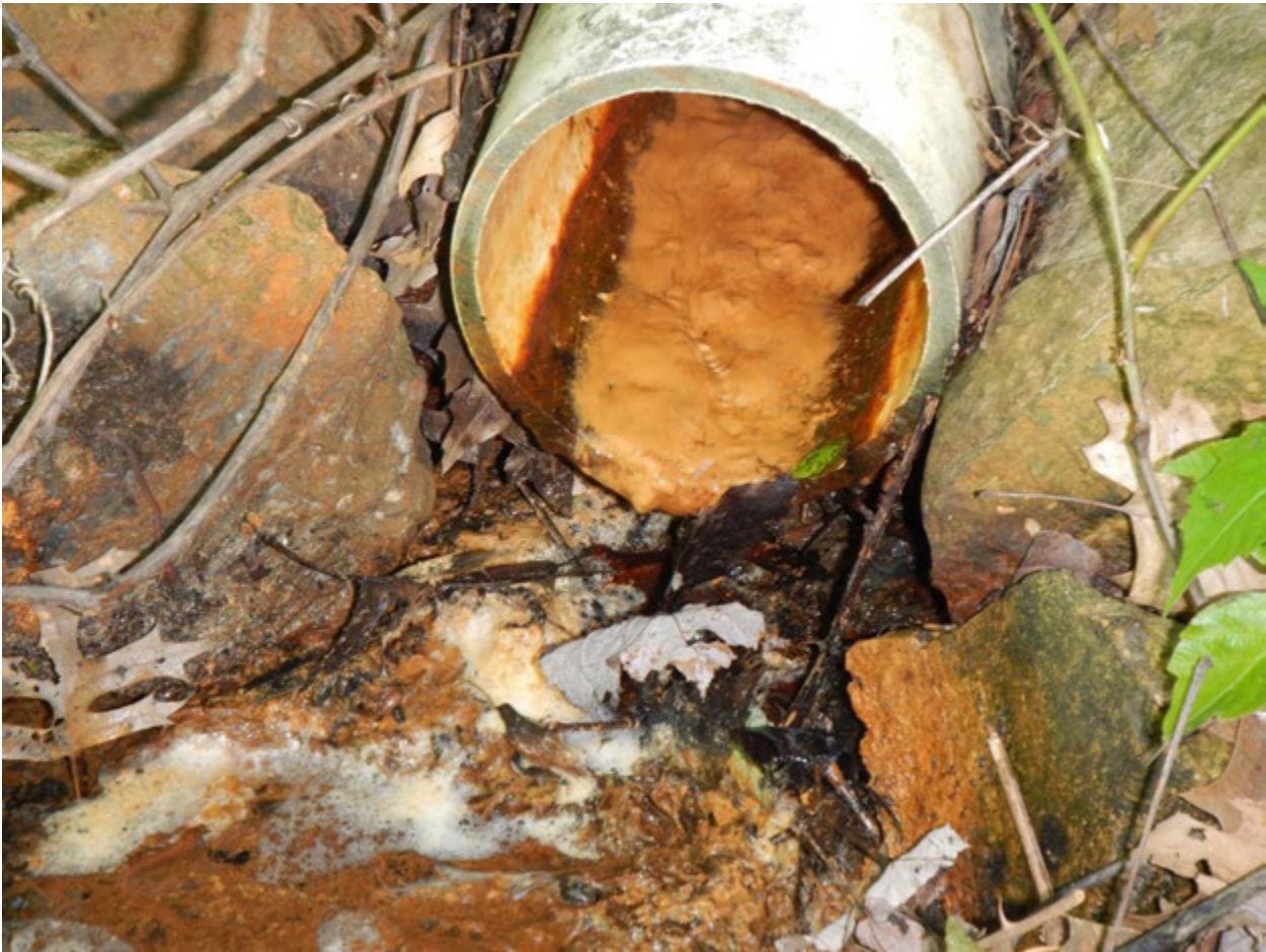
Figure 2. A close view of the opening for Outfall J15H5Onew1; note the thick orange material on the floor of the pipe and the staining on the walls of the pipe (this may be evidence of iron-oxidizing bacteria)
