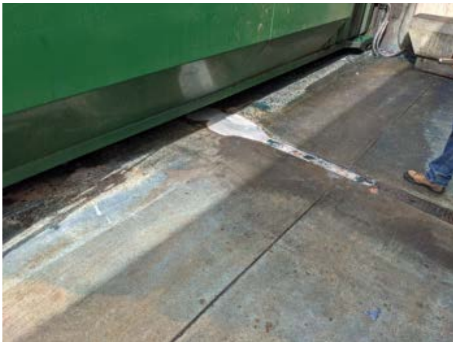
12/2/2021 Inspection – Trash compactor in the loading dock of C Care USA, showing dye and potentially additional substances leaking into the trench drain below.
