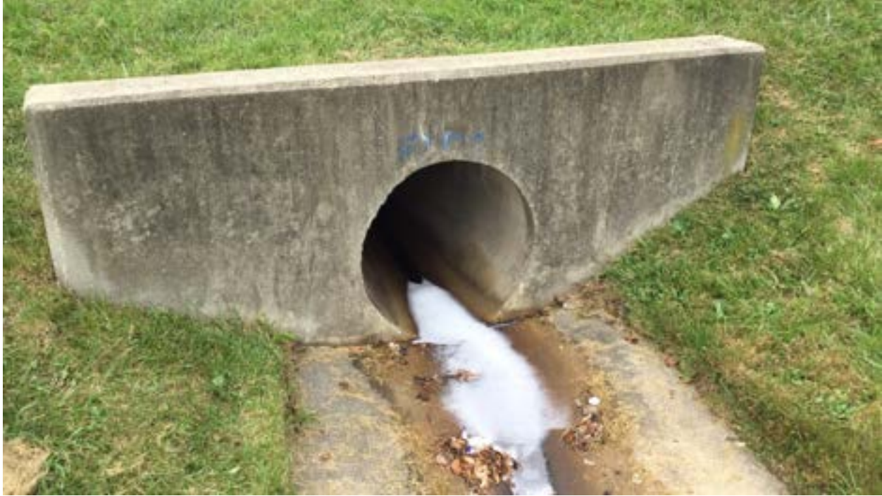
10/13/2021 Inspection – Outfall K020016 with a collection of suds.
