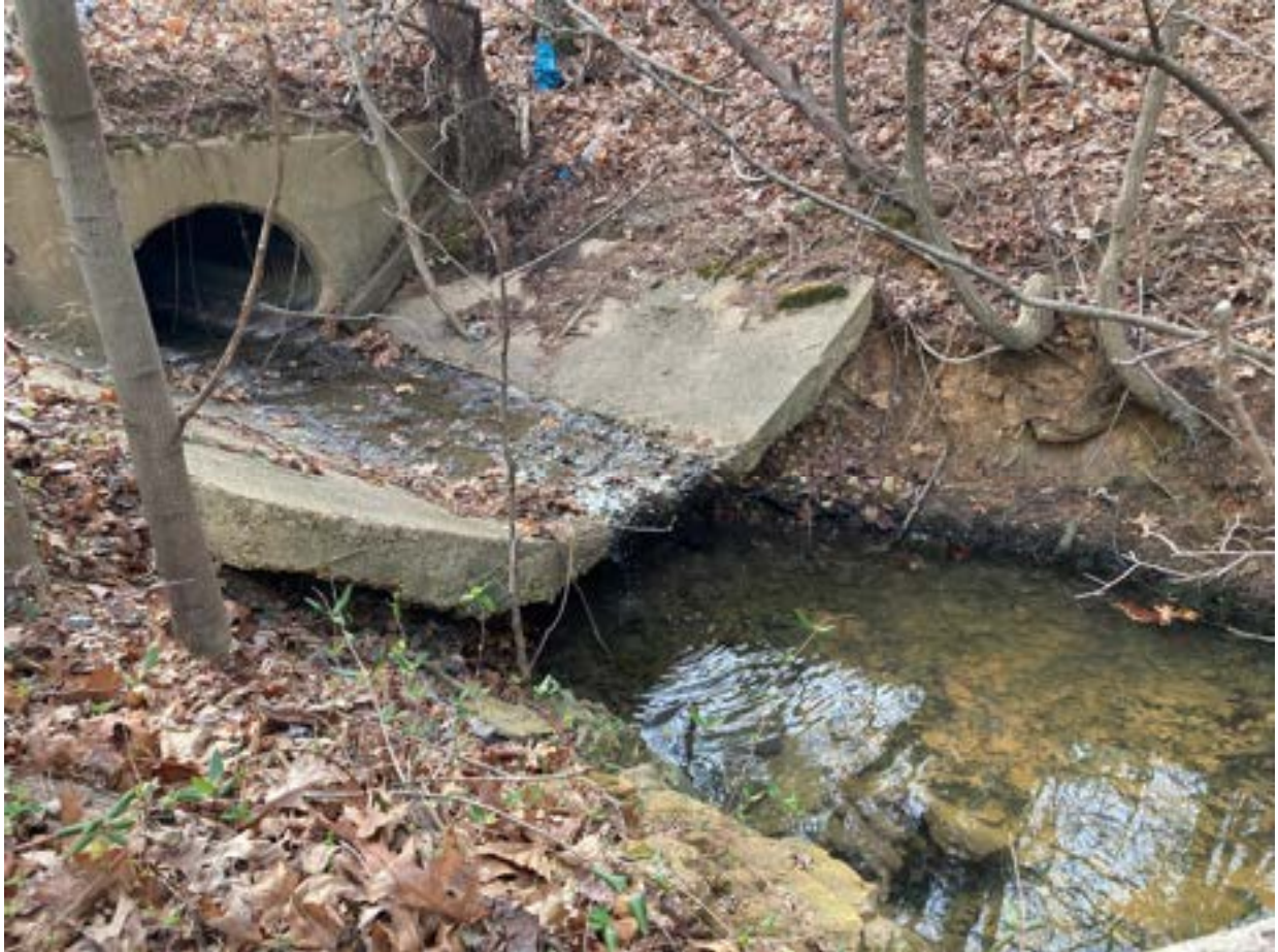
Inspection 3/1/2022 – Overview of outfall G060015 and erosion.
