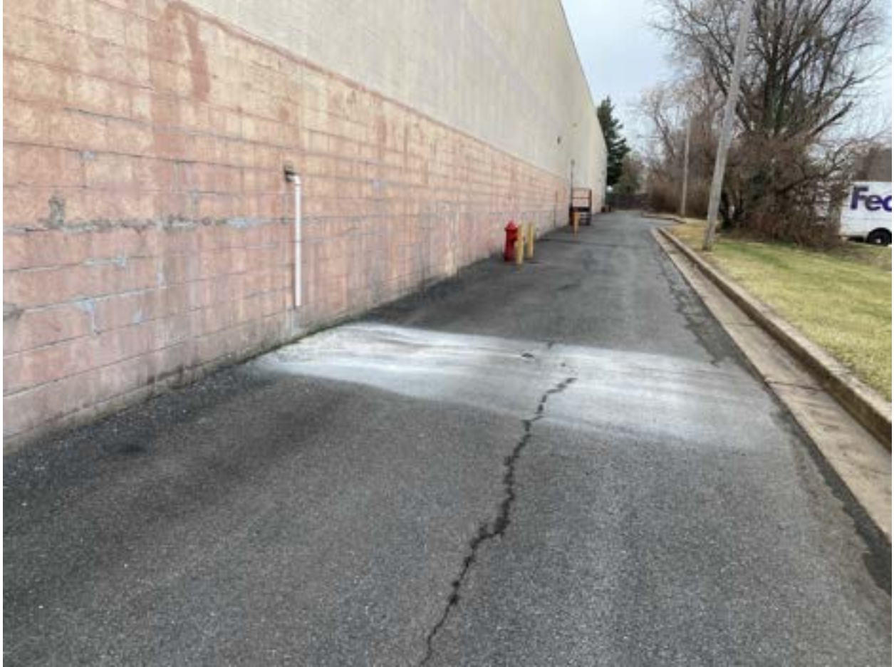
3/1/2022 Inspection – Location of white staining.
