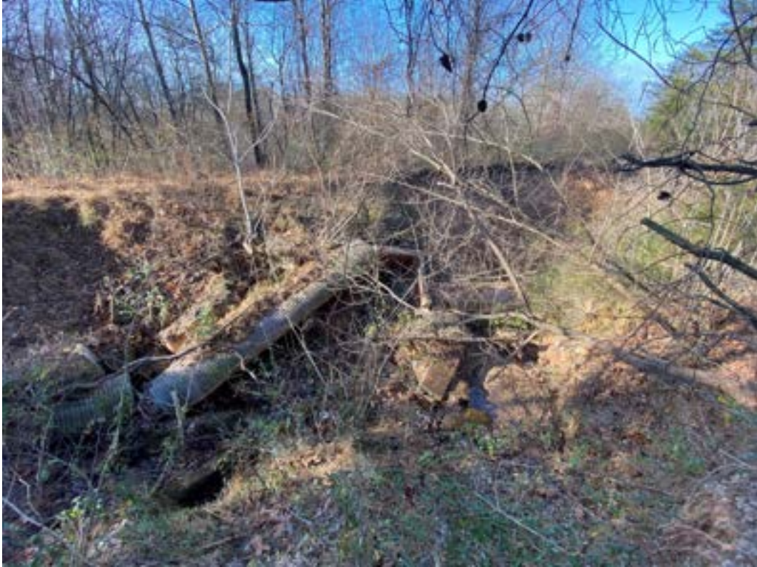
Inspection 12/15/2021 – Location of severe erosion and exposed pipe.
