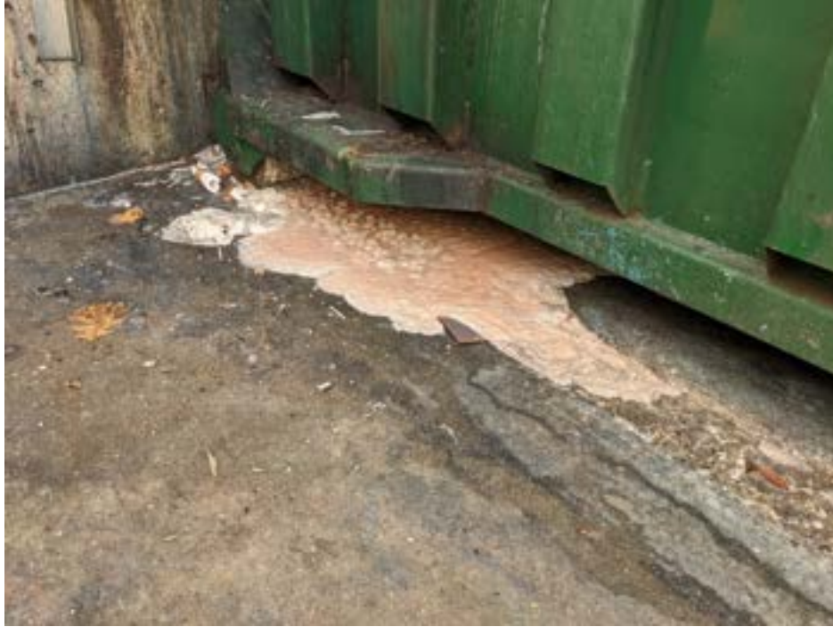
01/14/2022 Inspection – Trash compactor in the loading dock of C Care USA, showing soapy substances leaking into the trench drain below.
