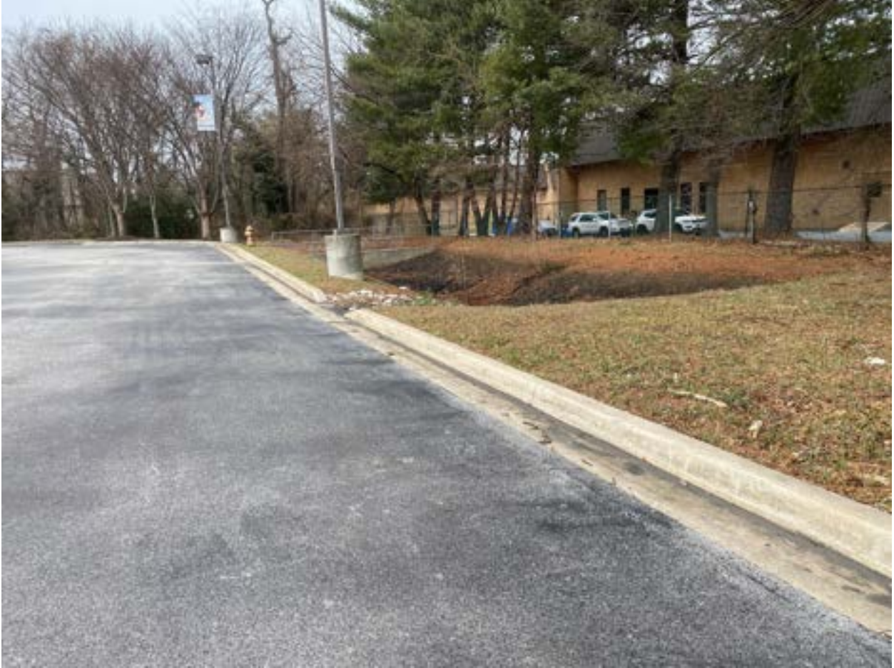
3/1/2022 Inspection – Stains appear to track along the curb to a curb cut opening.
