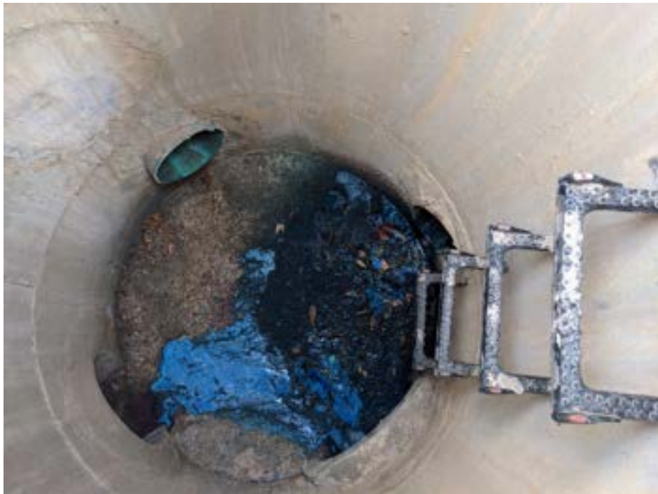
12/2/2021 Inspection – Manhole immediately downstream of trench drain, showing thick blue staining.
