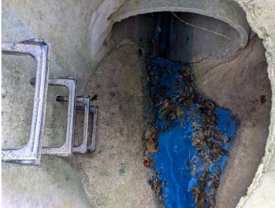
12/2/2021 Inspection – Thick blue staining is present throughout the upstream storm drain system.
