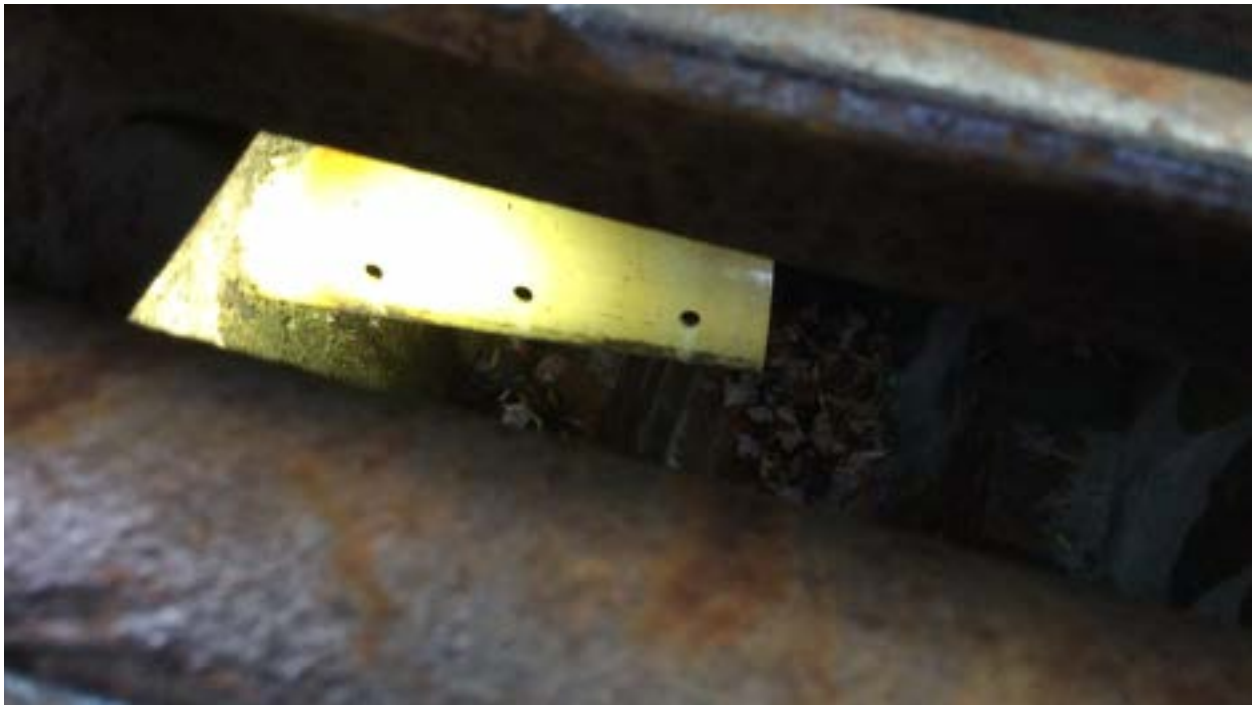
11/10/2021 Inspection – PVC pipe from unknown source in upstream inlet.
