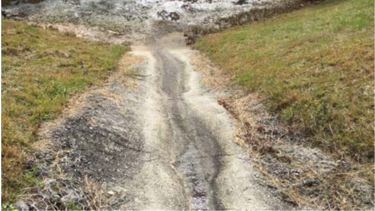
11/11/2021 Follow-Up Inspection – Downstream of outfall G06O006, no longer flowing.
