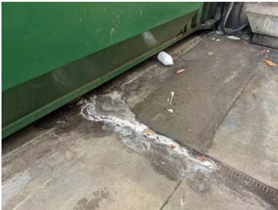
01/14/2022 Inspection - Trash compactor in the loading dock of C Care USA, showing soapy substances leaking into the trench drain below.
