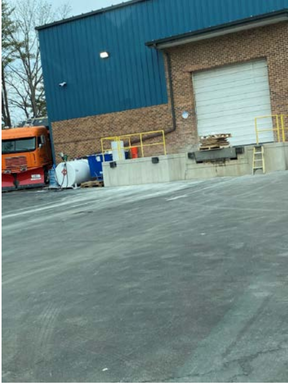
3/1/2022 Inspection – Location of white staining.
