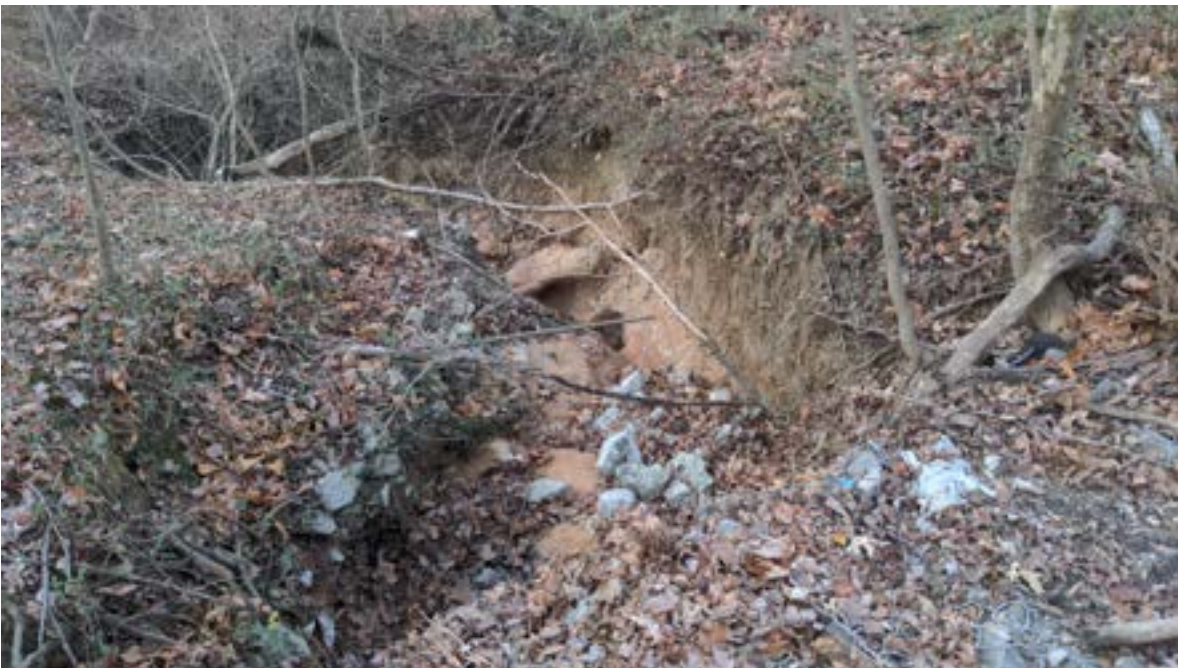
Inspection 12/16/2021 – Location of scouring erosion downstream of outfall, past gabion wall.
