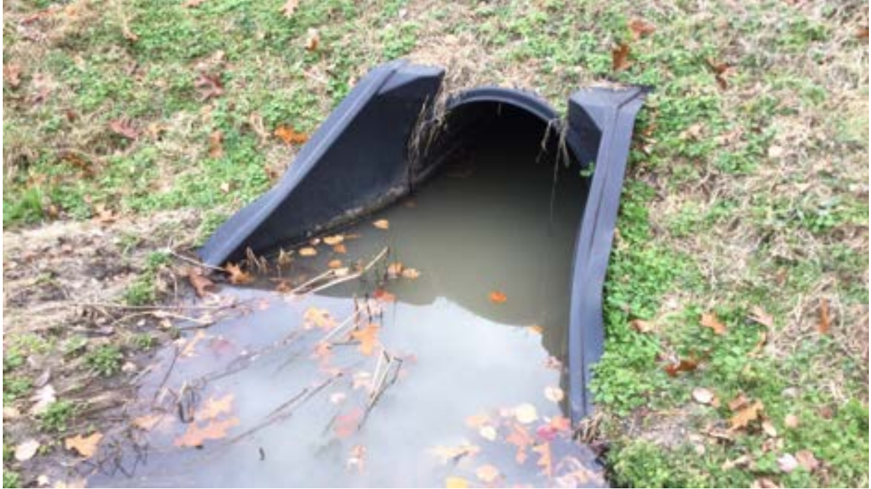
11/18/2021 Follow-Up Inspection – Overview of outfall J07O019, standing water remains.
