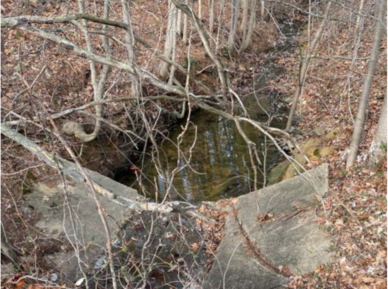
3/1/2022 Inspection – Location of erosion slightly downstream from outfall.
