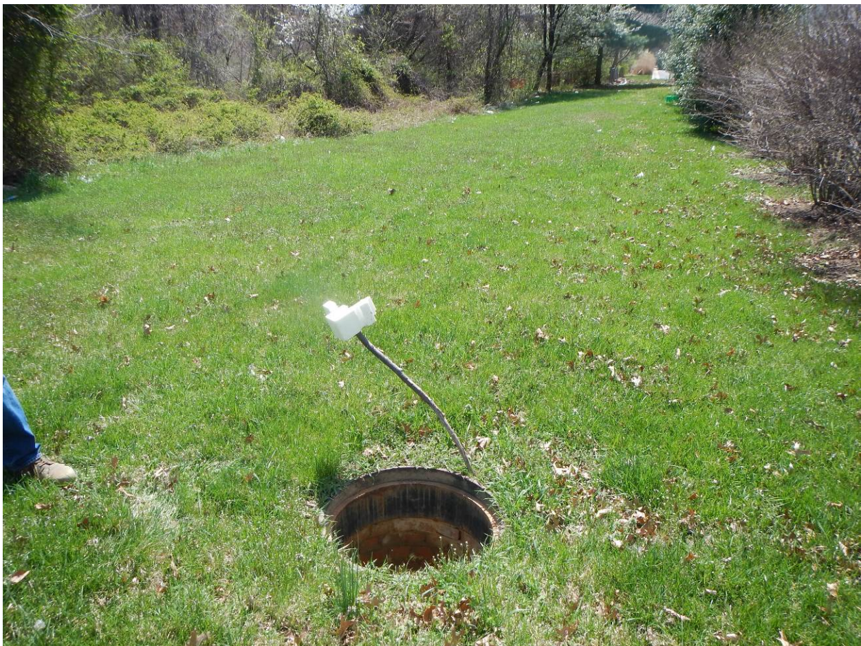
Figure 1. Stormwater system manhole found open
