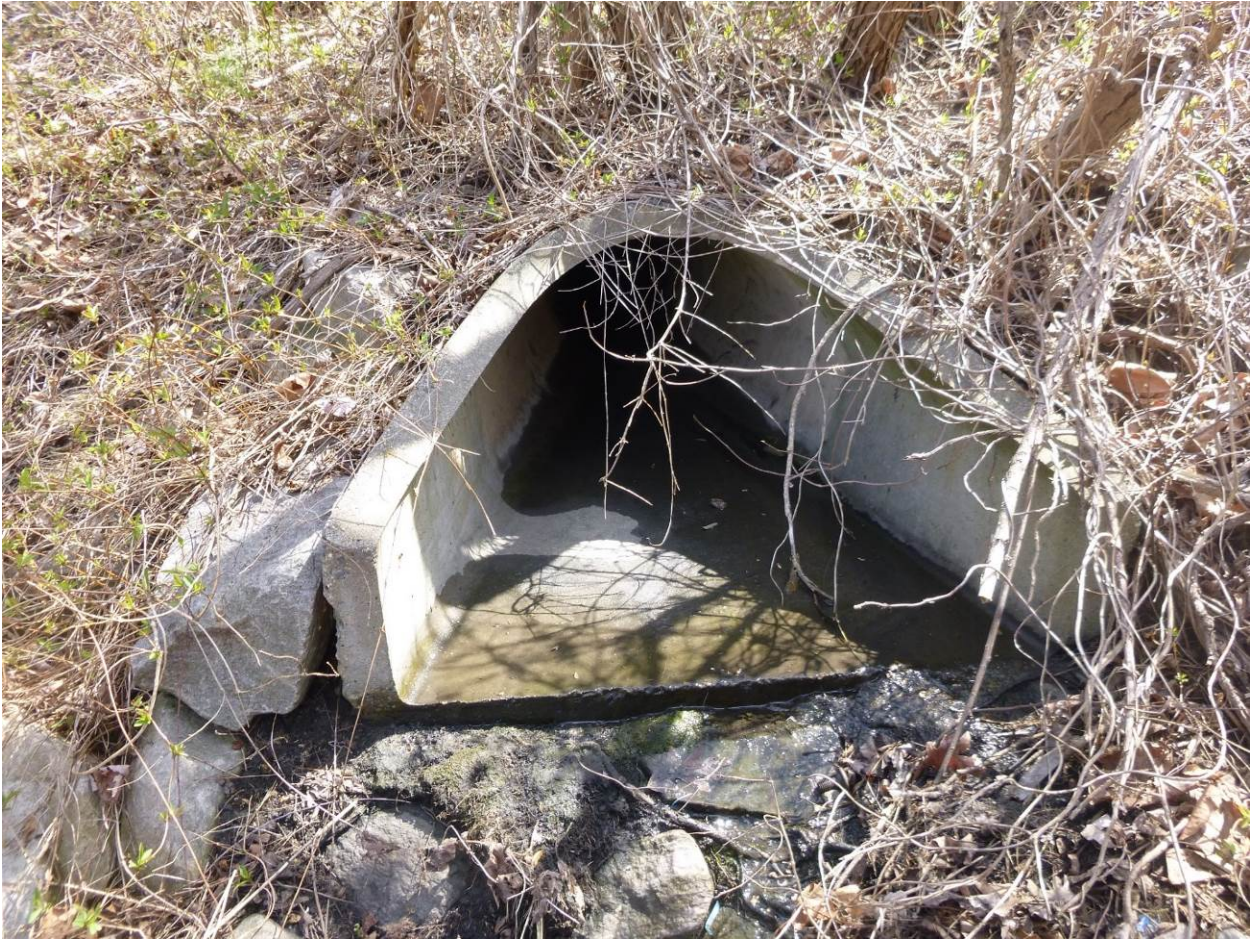
Figure 1. Outfall F06H4O016 showing a small amount of flowing water on April 13
