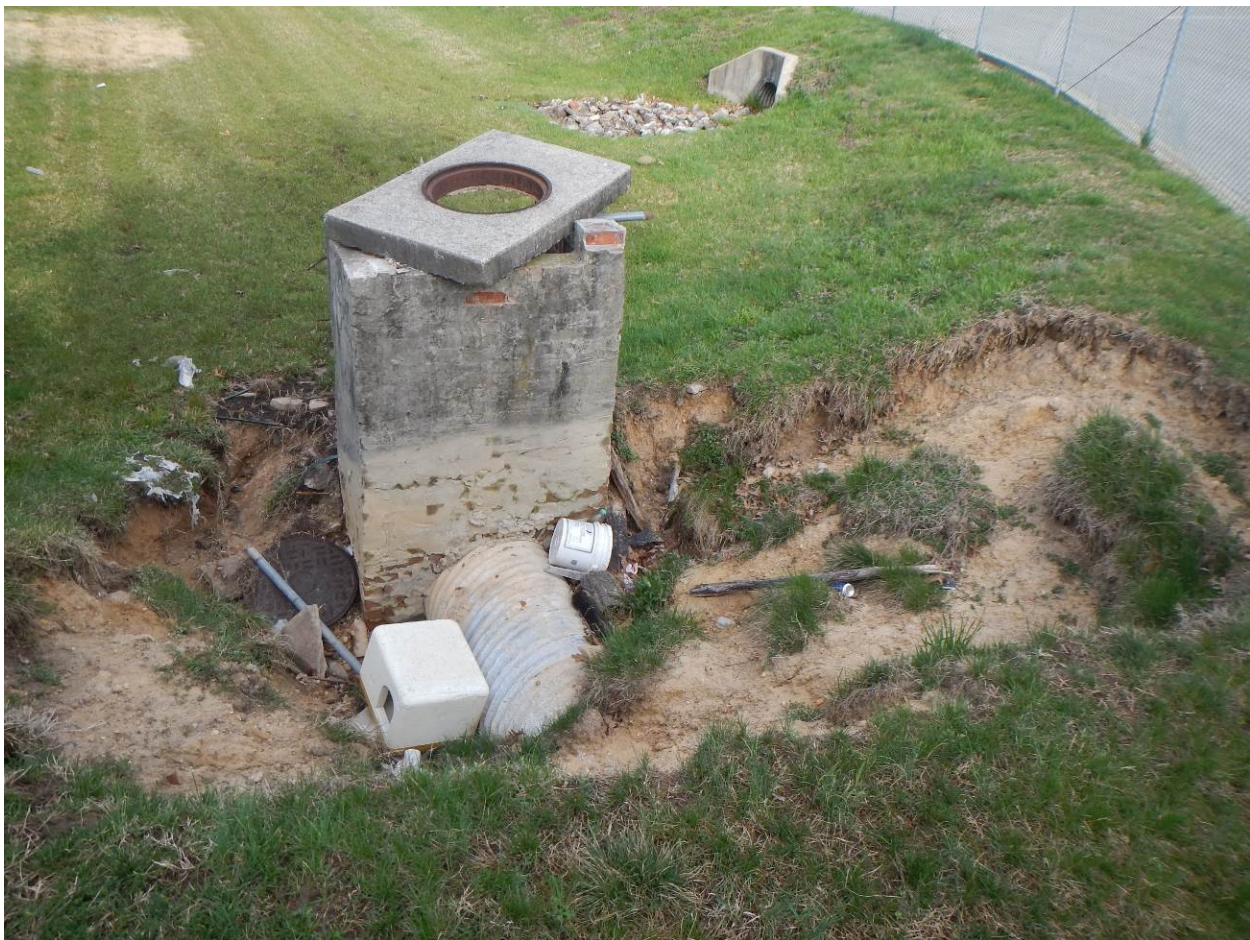
Figure 1. Stormwater riser structure condition showing dismantled top
