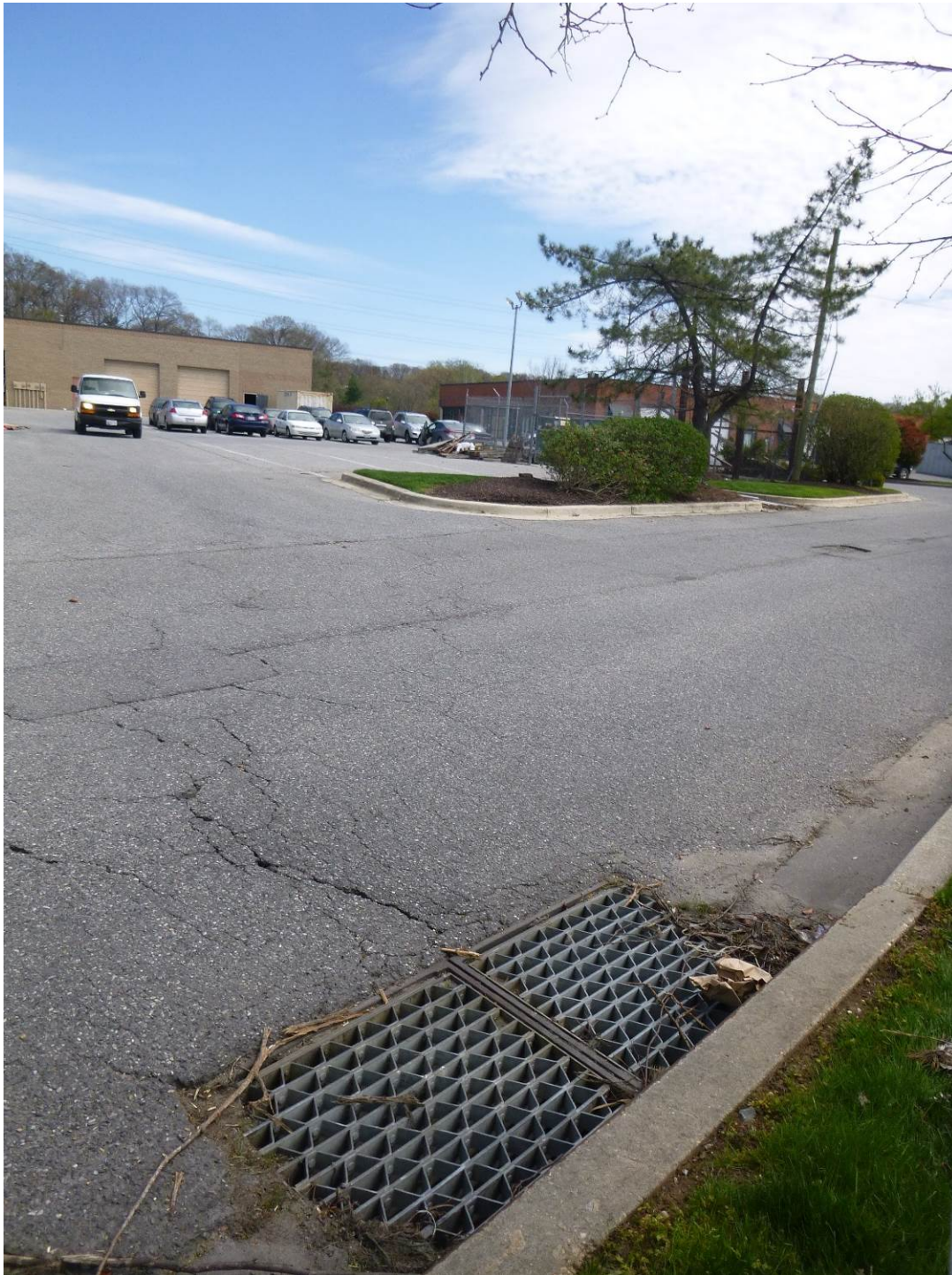
Figure 4. Relative location of the inlet that would receive drainage from the dumpsters and storage areas
