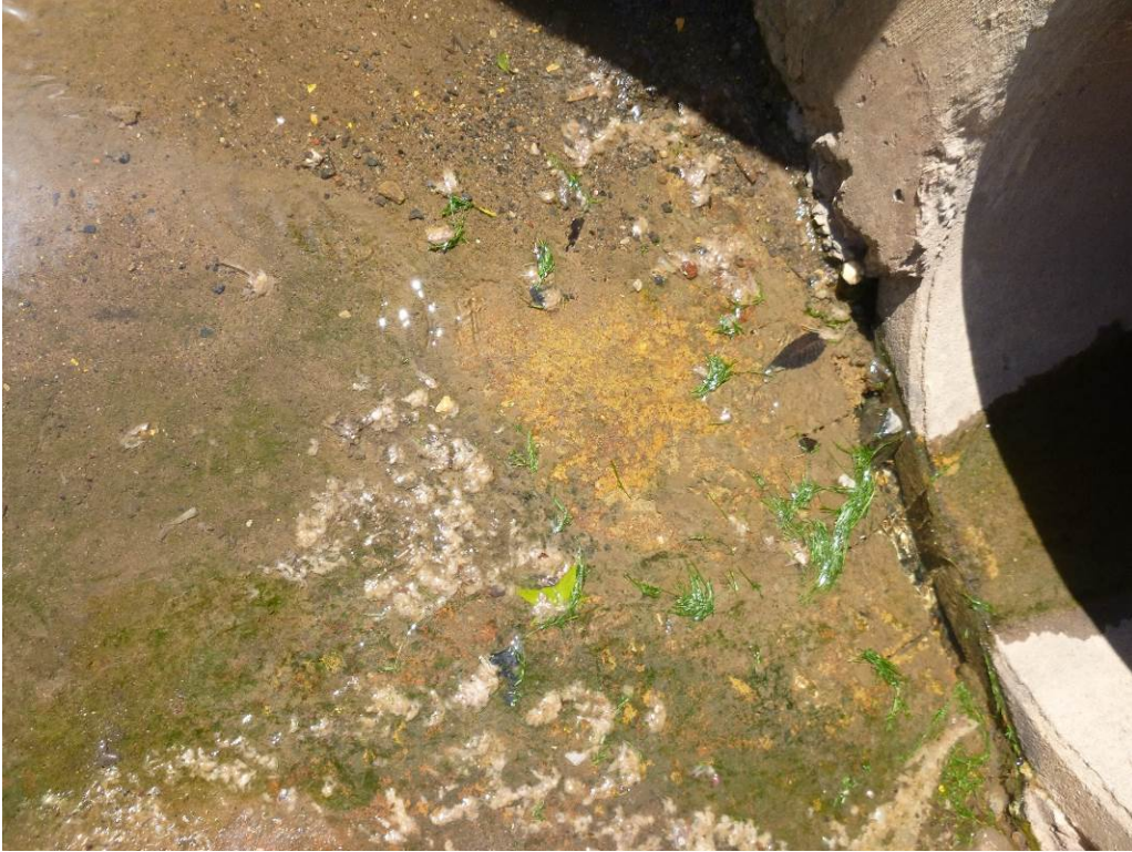
Figure 2. Noticeable toilet paper at the opening of outfall F07F8O003NEW
