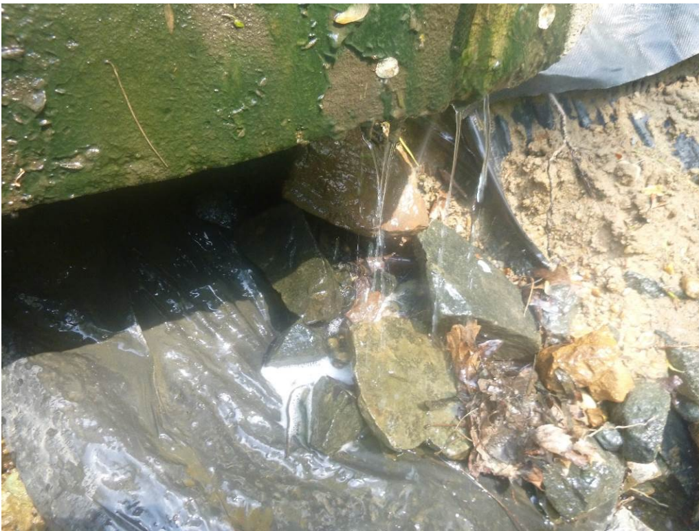
Figure 2. Discharge and suds below oufall F09F5O001
