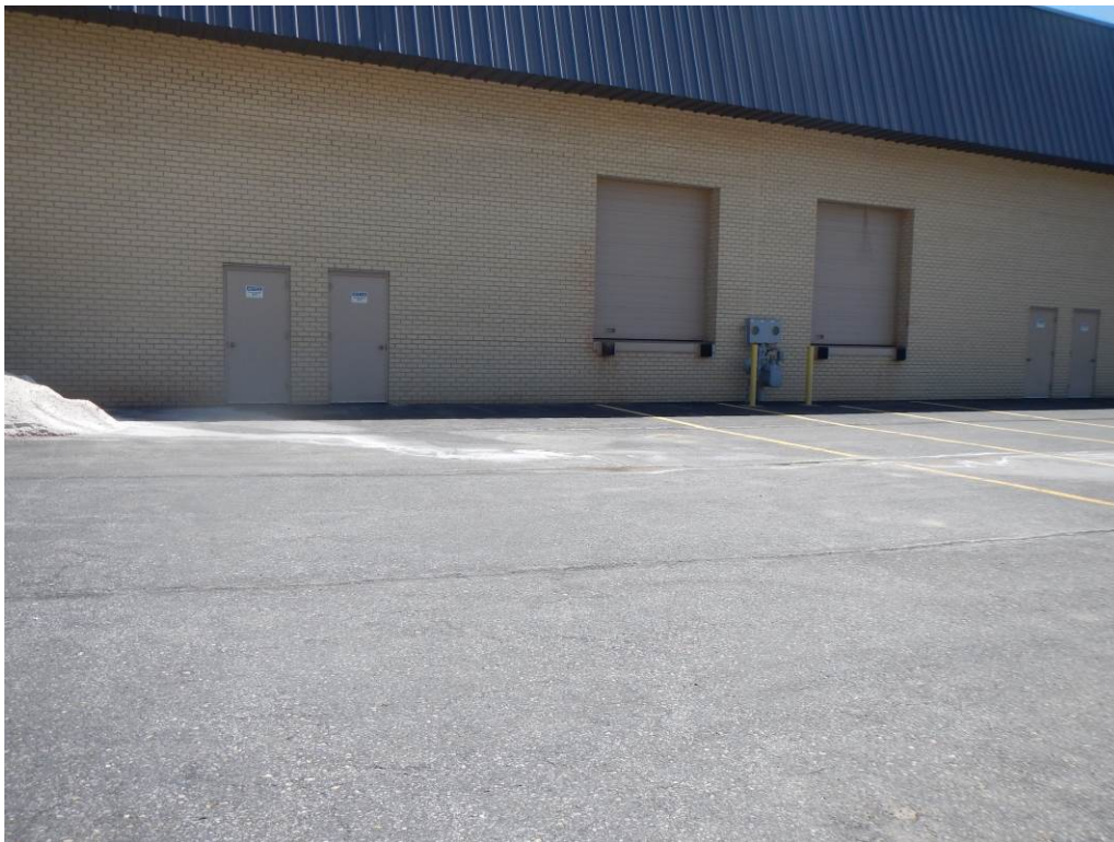
Figure 2 Evidence of the distribution of salt residue along the parking lot surface from the exposed pile of road salt
