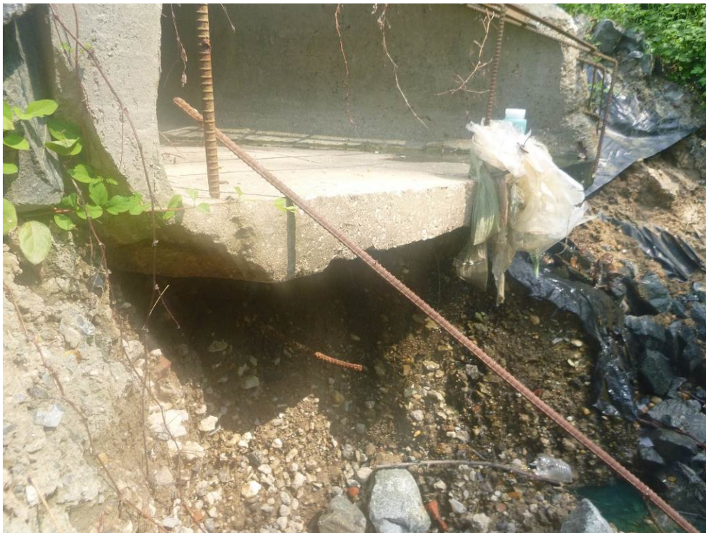
Figure 4. Erosion at outfall F09F50001
