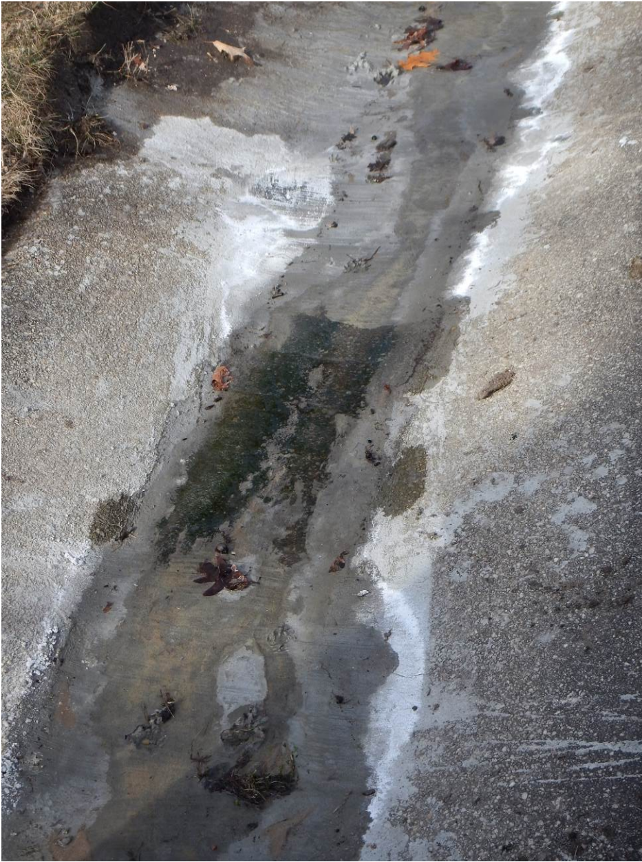
Figure 2. Whitish residue on concrete channel downstream of outfall.
