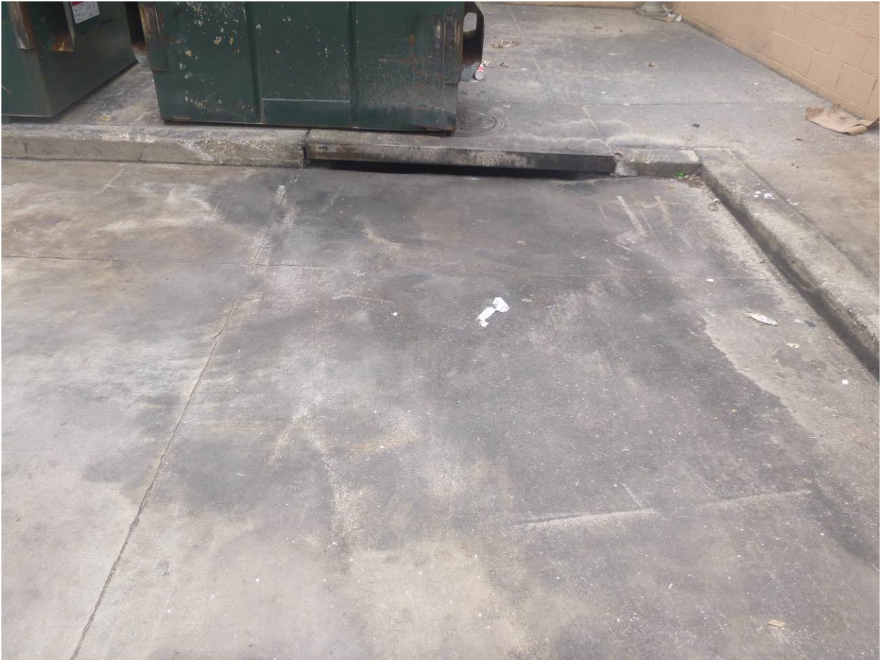
Figure 2. Stains found leading to the curb inlet
