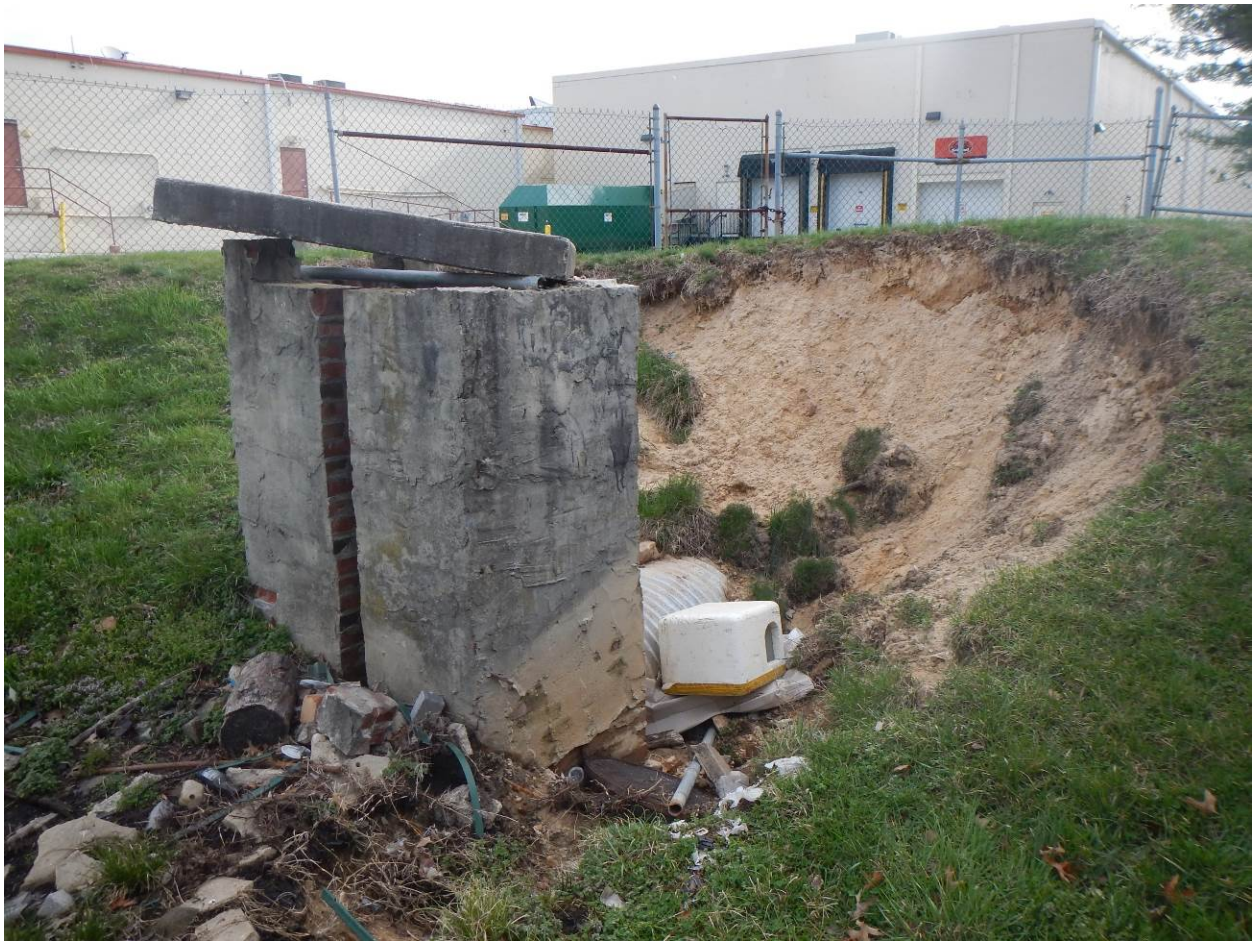
Figure 2. View from the detention basin showing the extent of erosion on the rear bank
